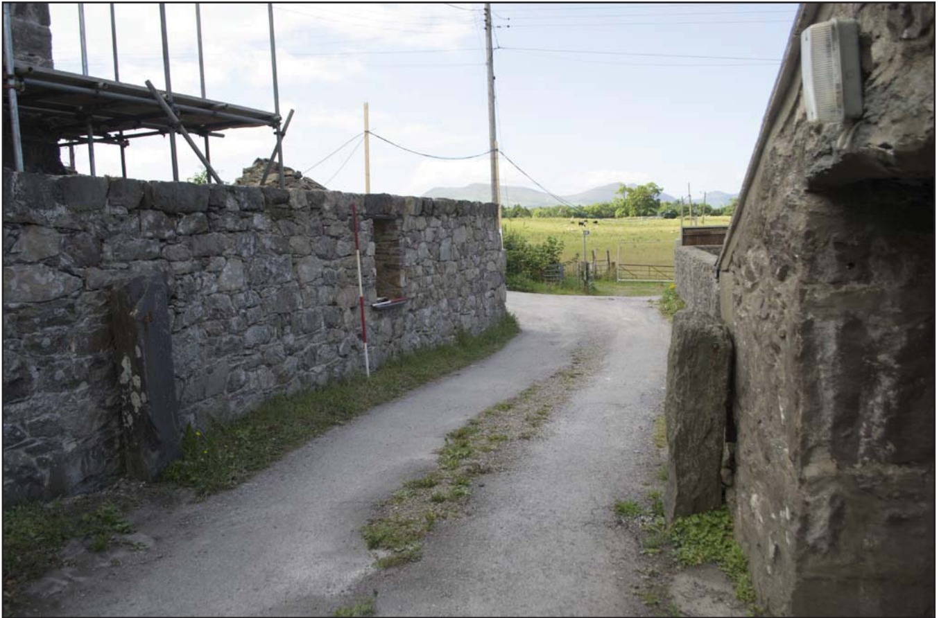
Plate 3: View of outer western wall of pigsty; scale 1x2m & 1x1m; view from N (archive reference: G2736_026).
