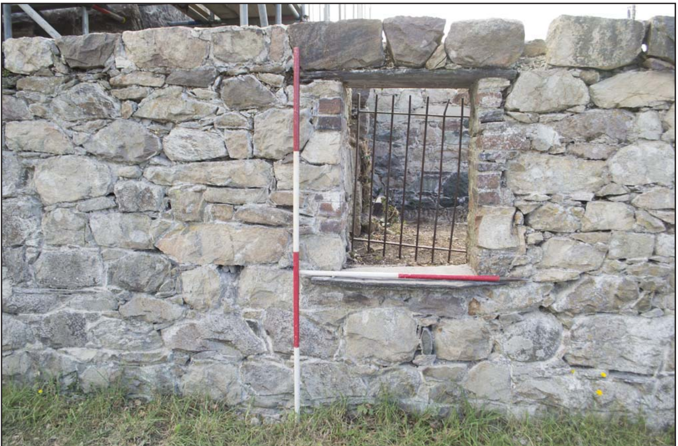
Plate 20: View of window opening located at western wall of Room 4; scale 1x2m & 1x1m; view from WNW (archive reference: G2736_027).
