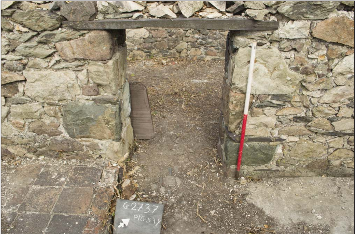
Plate 15: View of doorway between Rooms 3 and 4 showing slate lintel; scale 1x1m; view from ESE (archive reference: G2736_018).
