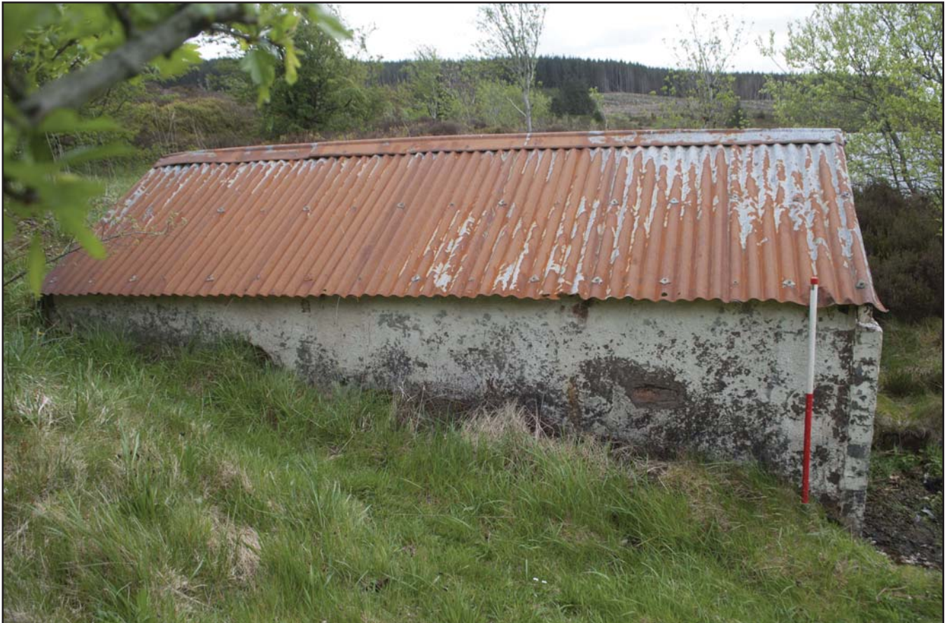
Plate 13: View of the boathouse from the north showing how it is set into the lakeside slope; scale: 1x1 m (archive reference: G2580_054).
