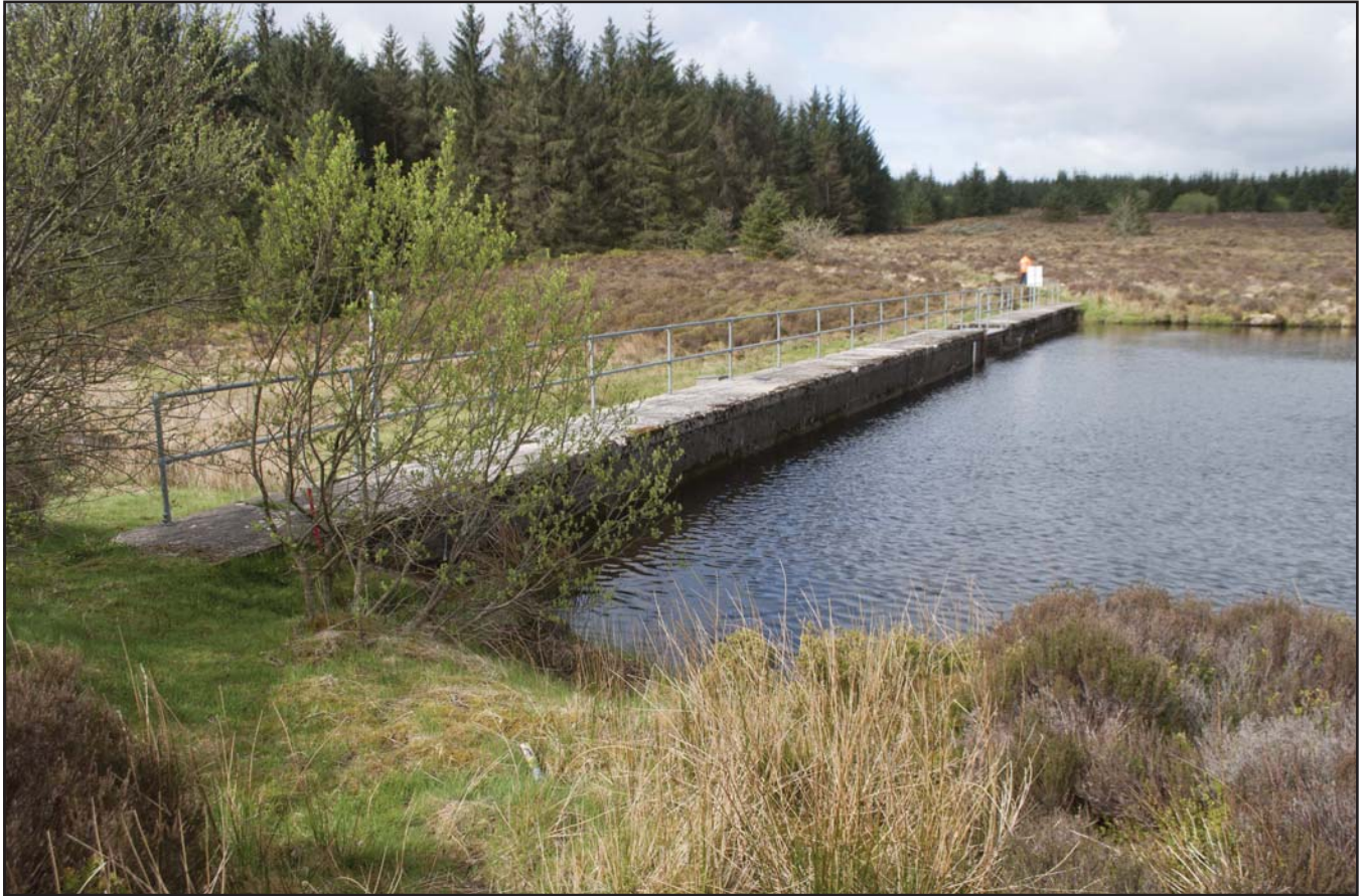
Plate 07: View along the dam from the east; scale: 1x1m (archive reference: G2580_038).
