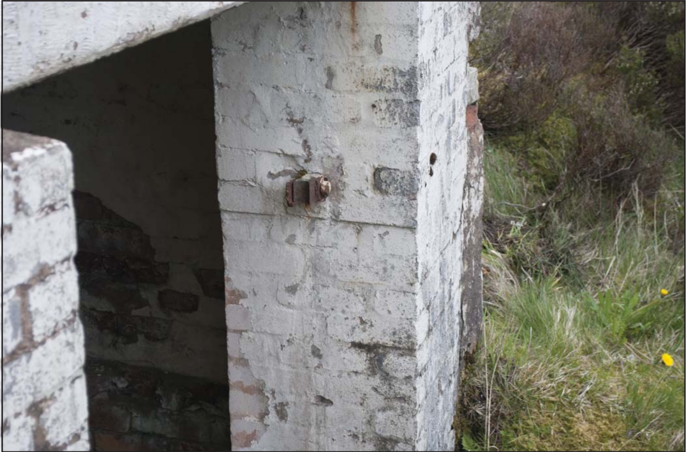
Plate 17: View of the entrance pier brickwork and pin for a former gate; (archive reference: G2580_058).
