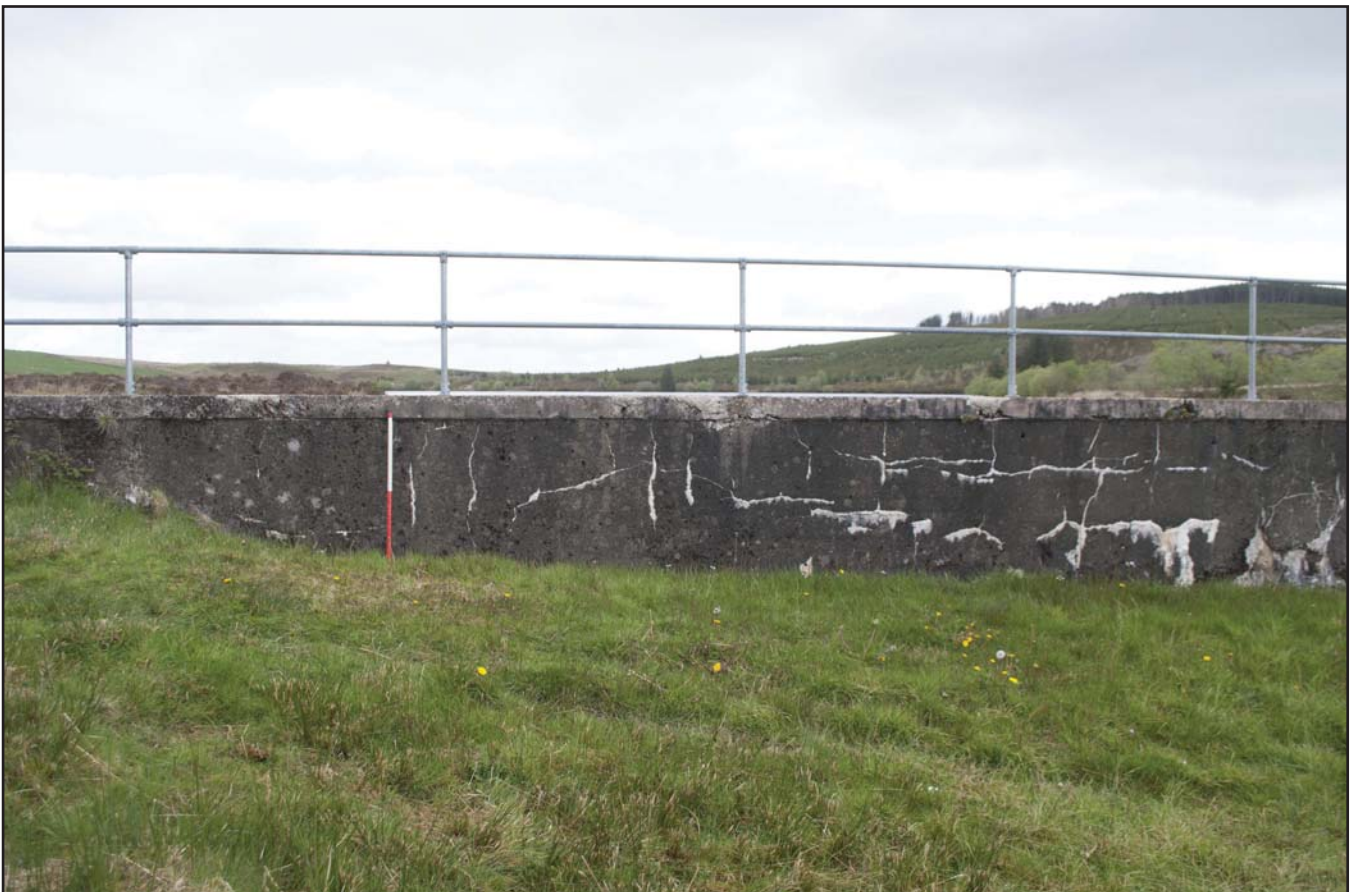
Plate 04: Detail showing the concrete render on the dam, with the protective barriers; scale: 1x1 m (archive reference: G2580_033).
