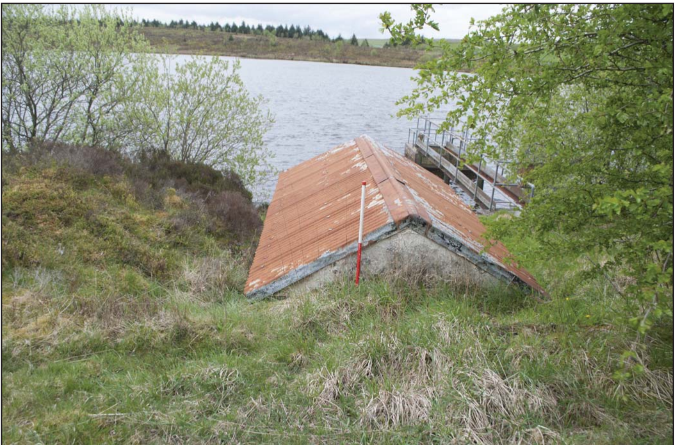
Plate 14: View from the east showing the rear gable elevation of the boathouse, and the extent to which it is cut into the bank; scale: 1x1 m (archive reference: G2580_055).
