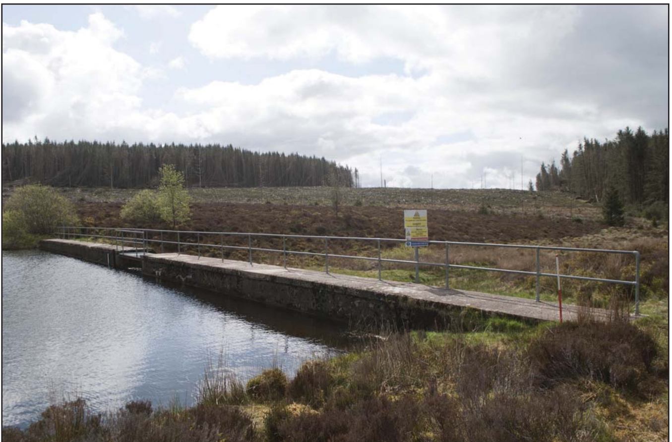
Plate 08: General view of the dam from the north west; scale: 1x1m (archive reference: G2580_039).
