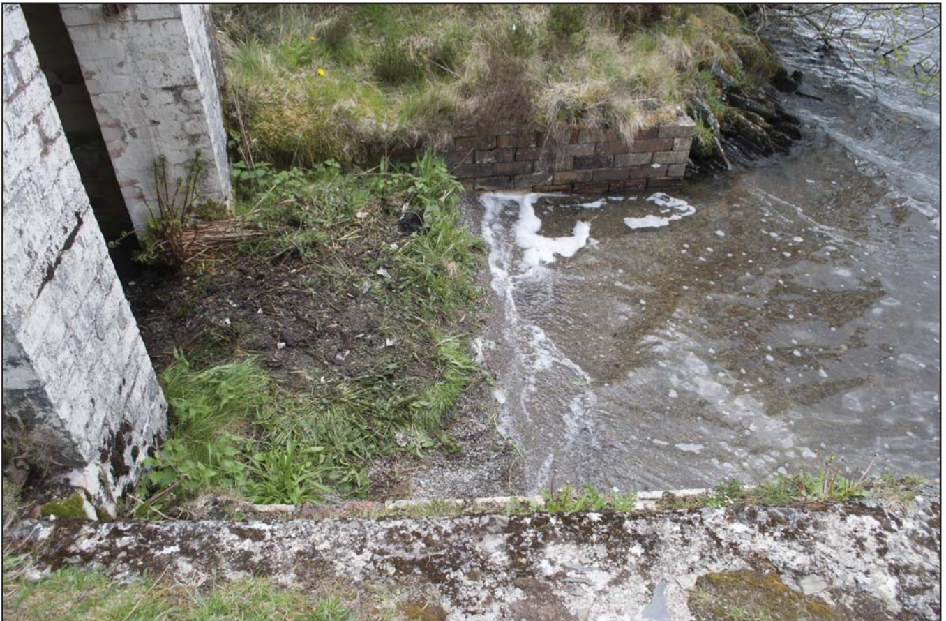
Plate 18: View of the entrance to the boathouse from the north, showing the revetment brickwork in the entrance (archive reference: G2580_059).
