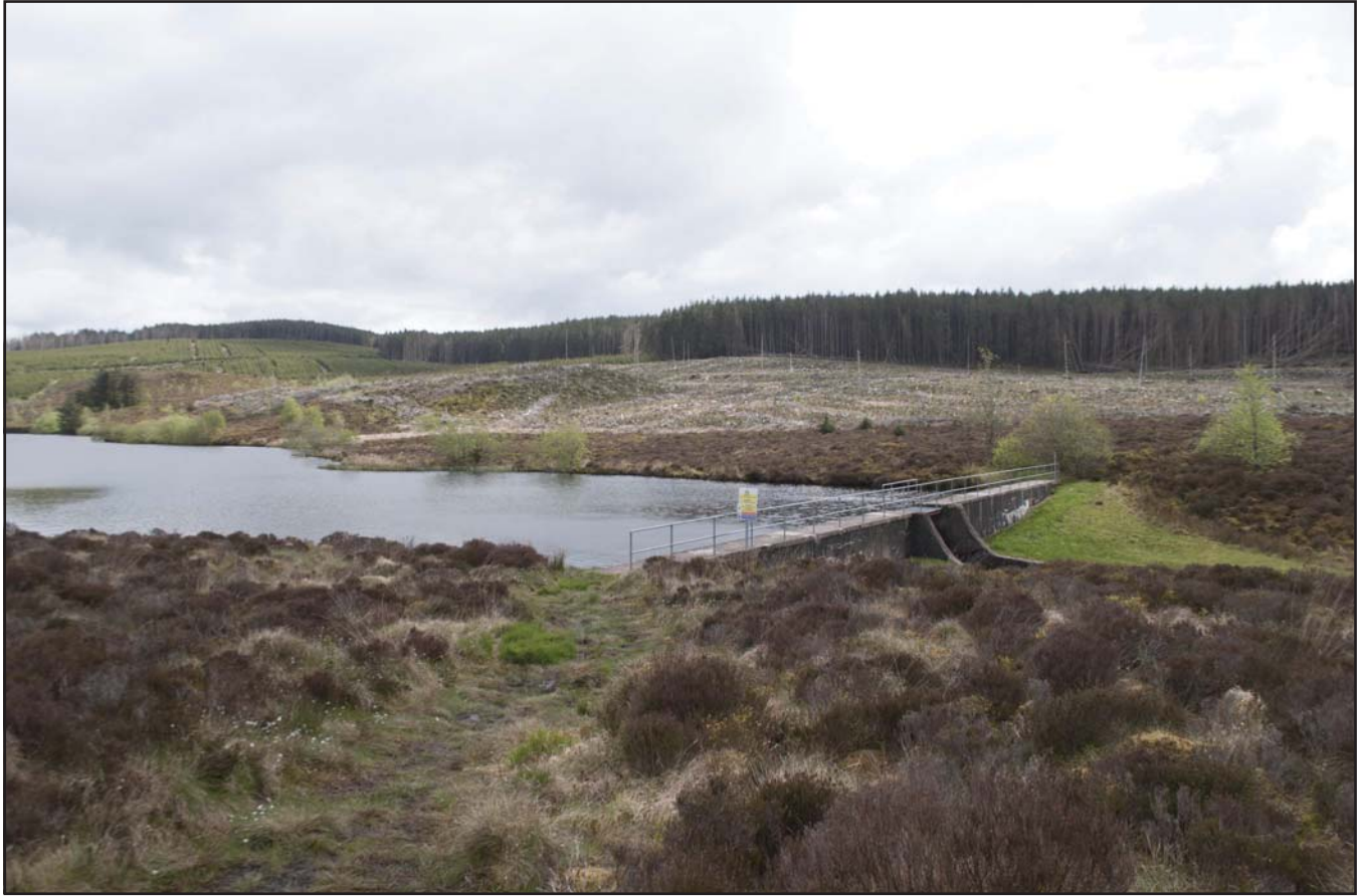
Plate 09: General view of the dam from the north west (archive reference: G2580_040).
