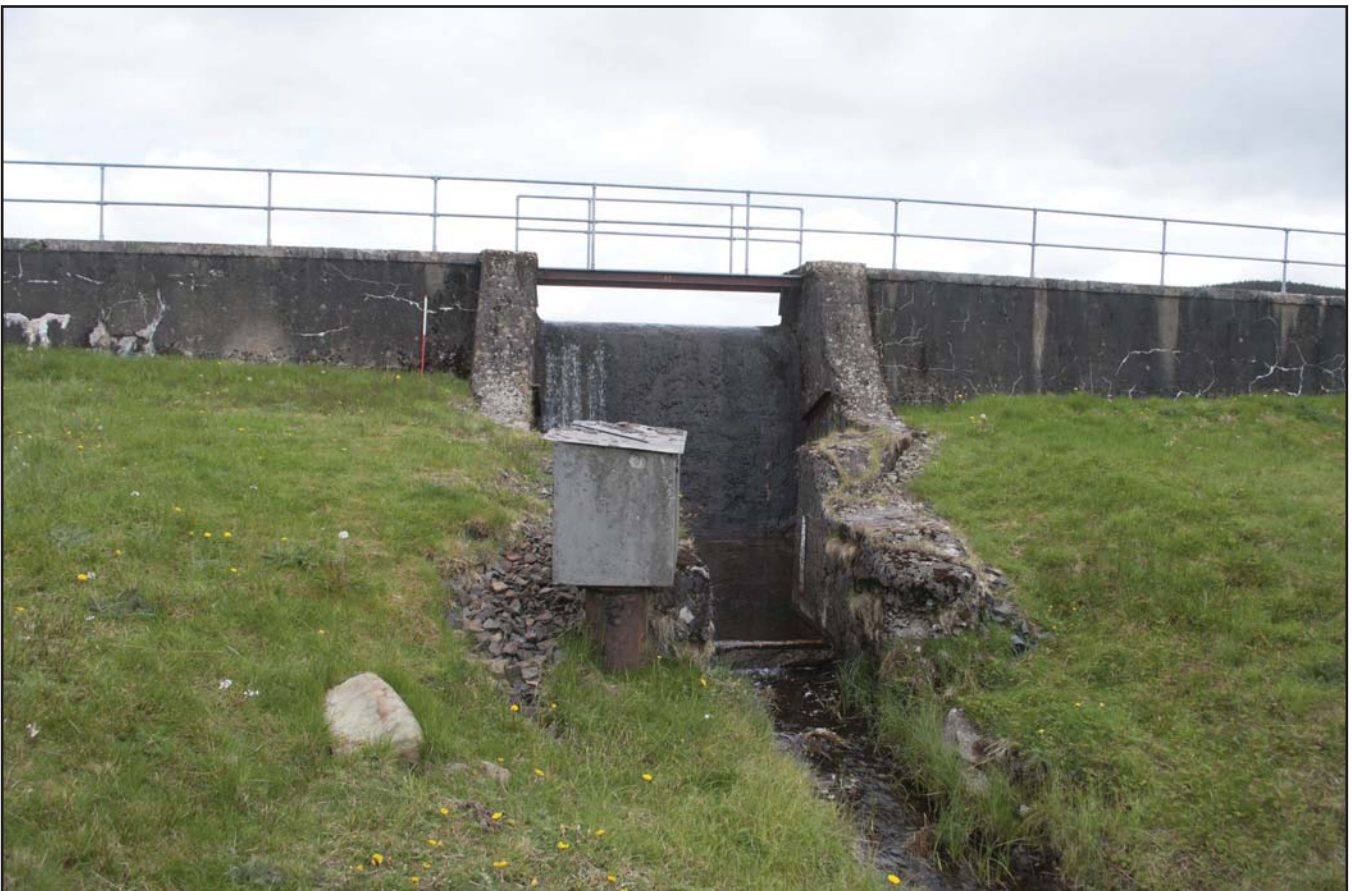
Plate 02: Detail of dam wall face showing the sluice debouching into the Afon Bran; scale: 1x1m (archive reference: G2580_034).
