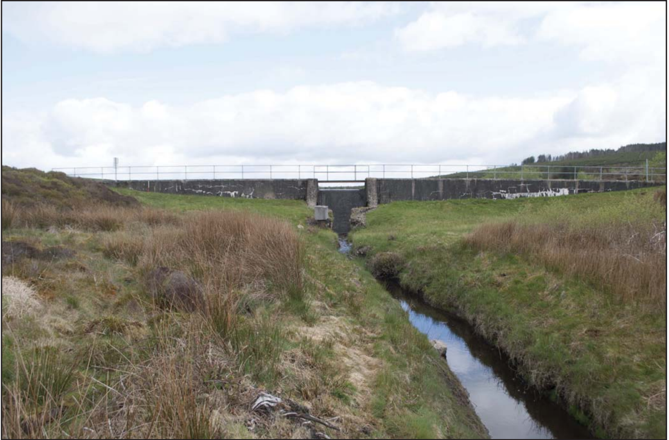
Plate 01: General view of the dam wall face from downstream; scale: 1x1m (archive reference: G2580_030).
