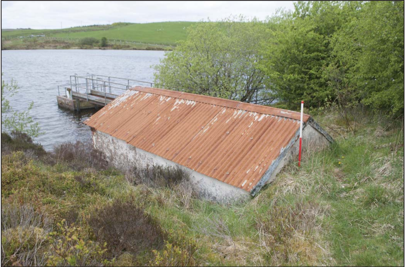
Plate 15: General view of the boathouse from the south east; scale: 1x1m (archive reference: G2580_056).
