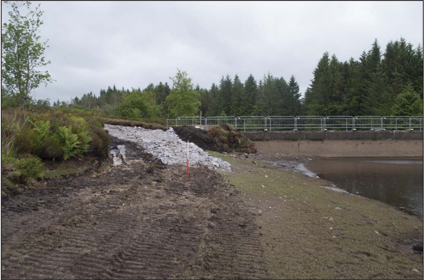
Plate 31: General view along the east bank showing the retreating waterline and bank works during peat removal; scale 1x1m; view from N (archive reference: G2580_109).
