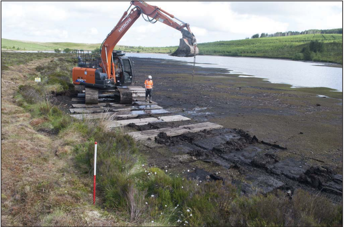
Plate 25: General view from the south showing the reduced level of the west bank of Llyn Brân with bog mats being laid; scale 1x1m; view from S (archive reference: G2580_096).
