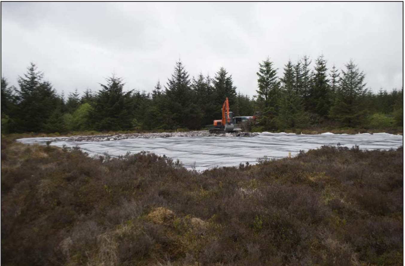
Plate 10: General view of the compound area. Showing terrain, matting down and stoning taking place; scale not used; view from NE (archive reference: G2580_073).
