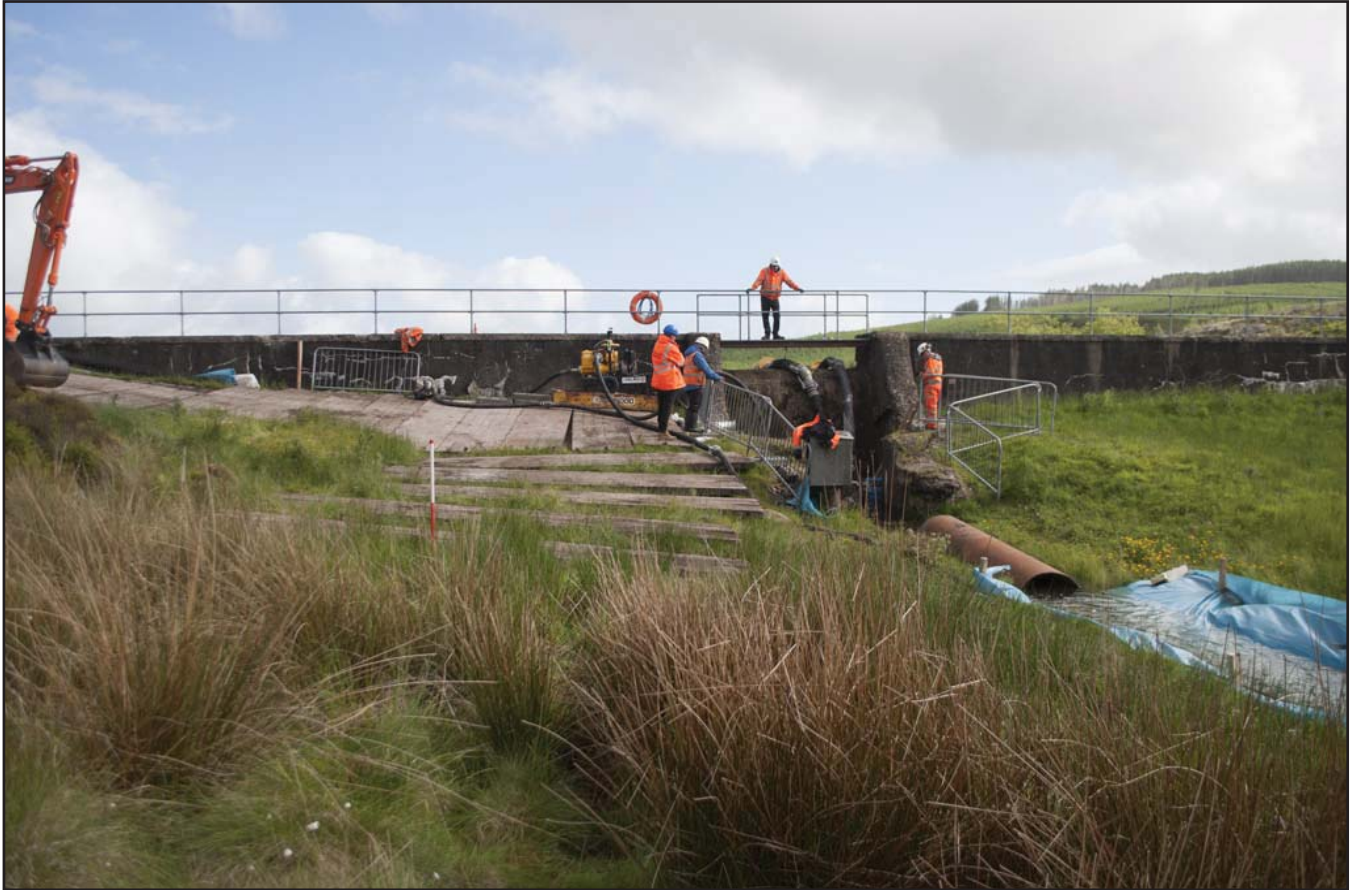
Plate 17: View of the area to be stripped from the south, looking at the dam face, and showing the water level reduction works; scale 1x1m; view from SSW (archive reference: G2580_084).
