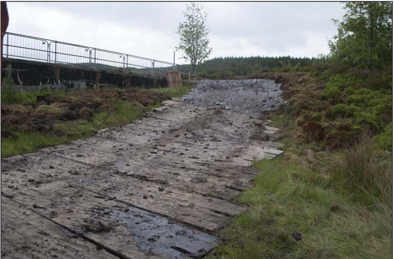
Plate 30: General view of log matting on the east bank of Llyn Brân dam; scale 1x1m; view from N (archive reference: G2580_108).
