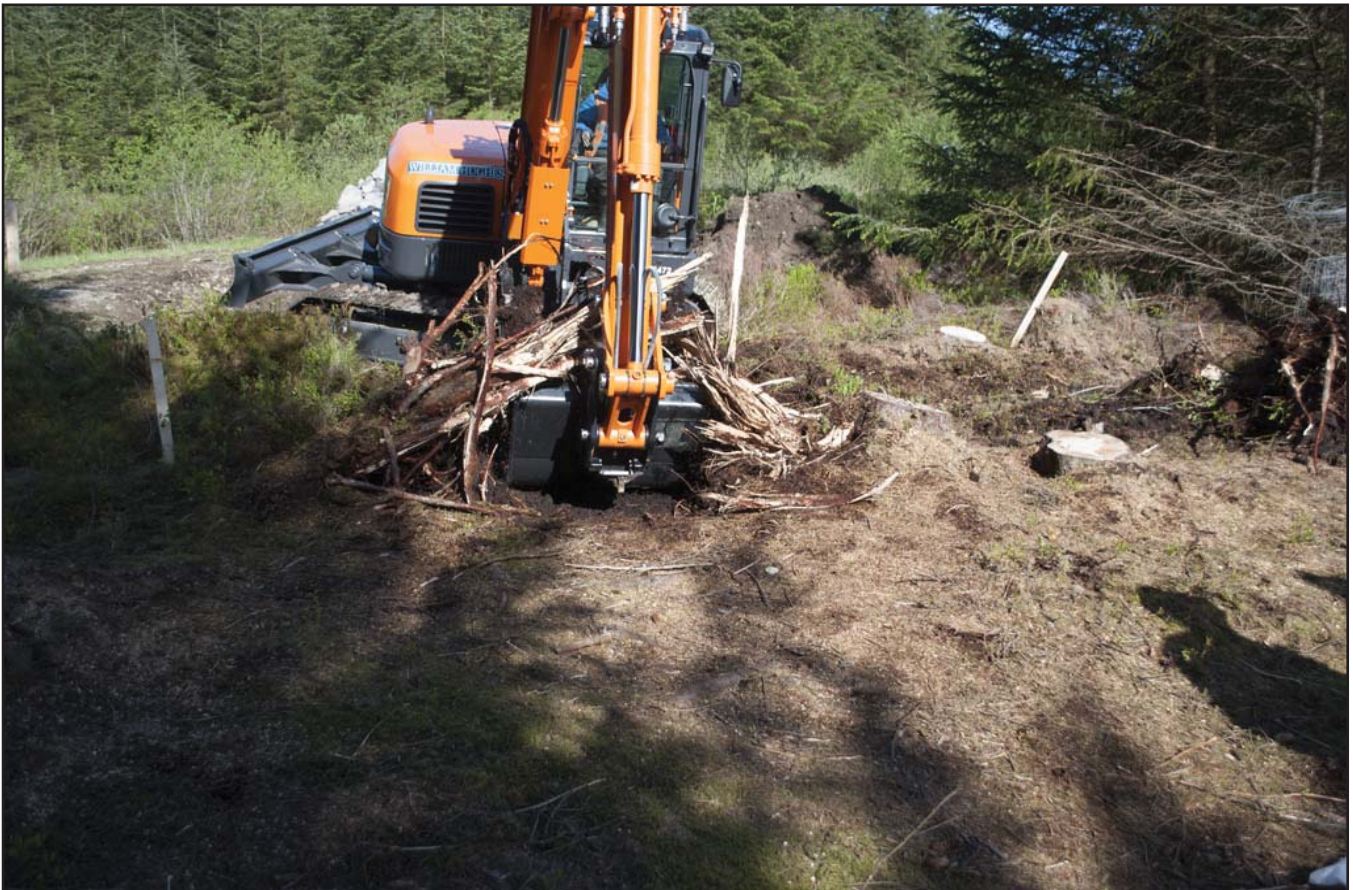
Plate 6: Tree stump removal; scale not used; view from SE (archive reference: G2580_069).
