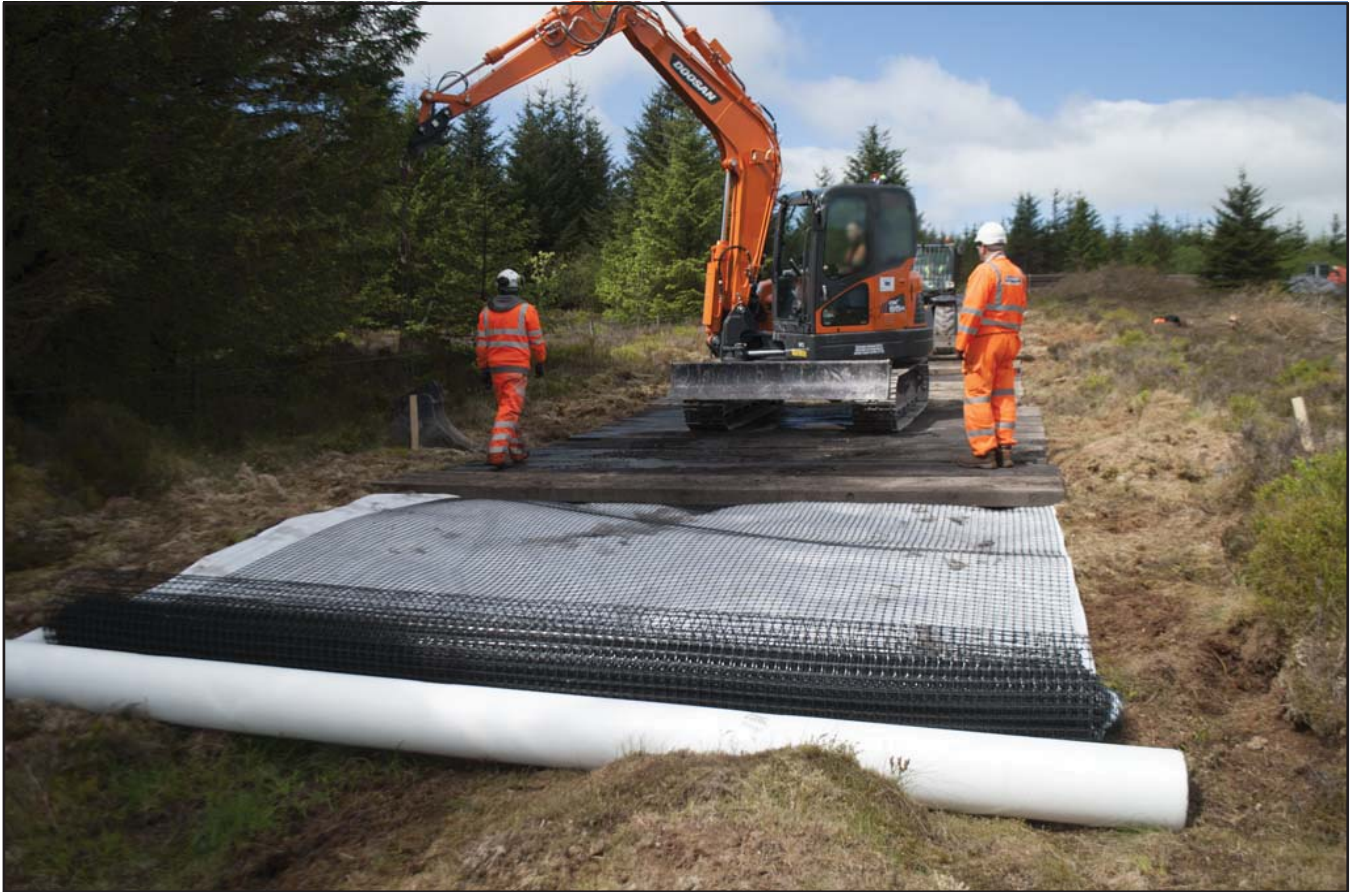
Plate 15: Close up view of bog mat laying; scale not used; view from ENE (archive reference: G2580_082).
