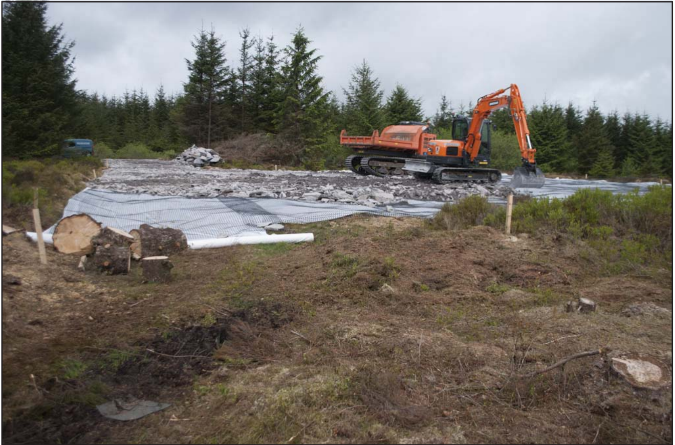
Plate 11: View of shale rubble laying from the west end of the track down to the dam; scale not used; view from E (archive reference: G2580_074).
