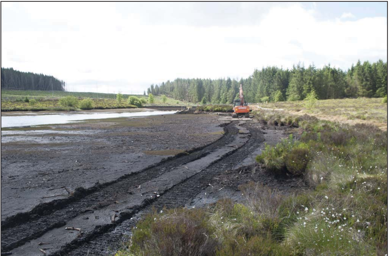
Plate 26: General view along the northern edge of Llyn Brân showing the log mat laying and the reduced water level in dam; scale not used; view from N (archive reference: G2580_097).
