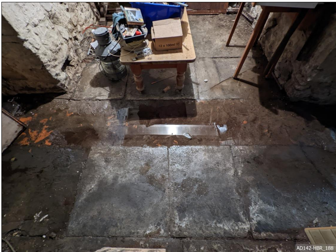
Plate 188 – View east, showing flagstone floor with red paver drainage channel to Cell B.
