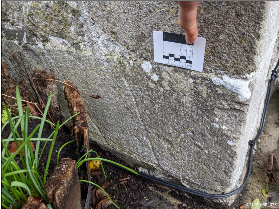
Plate 33 – View north, showing false voussoir window or doorway head reused as quoin.
