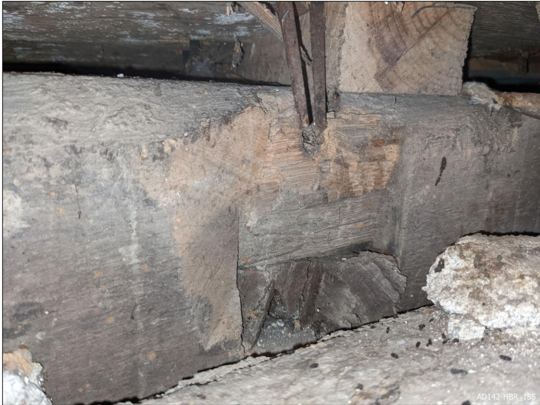
Plate 185 – View north, showing mortice for barefaced soffit tenon with diminished haunch. N.B. remains of tenon.
