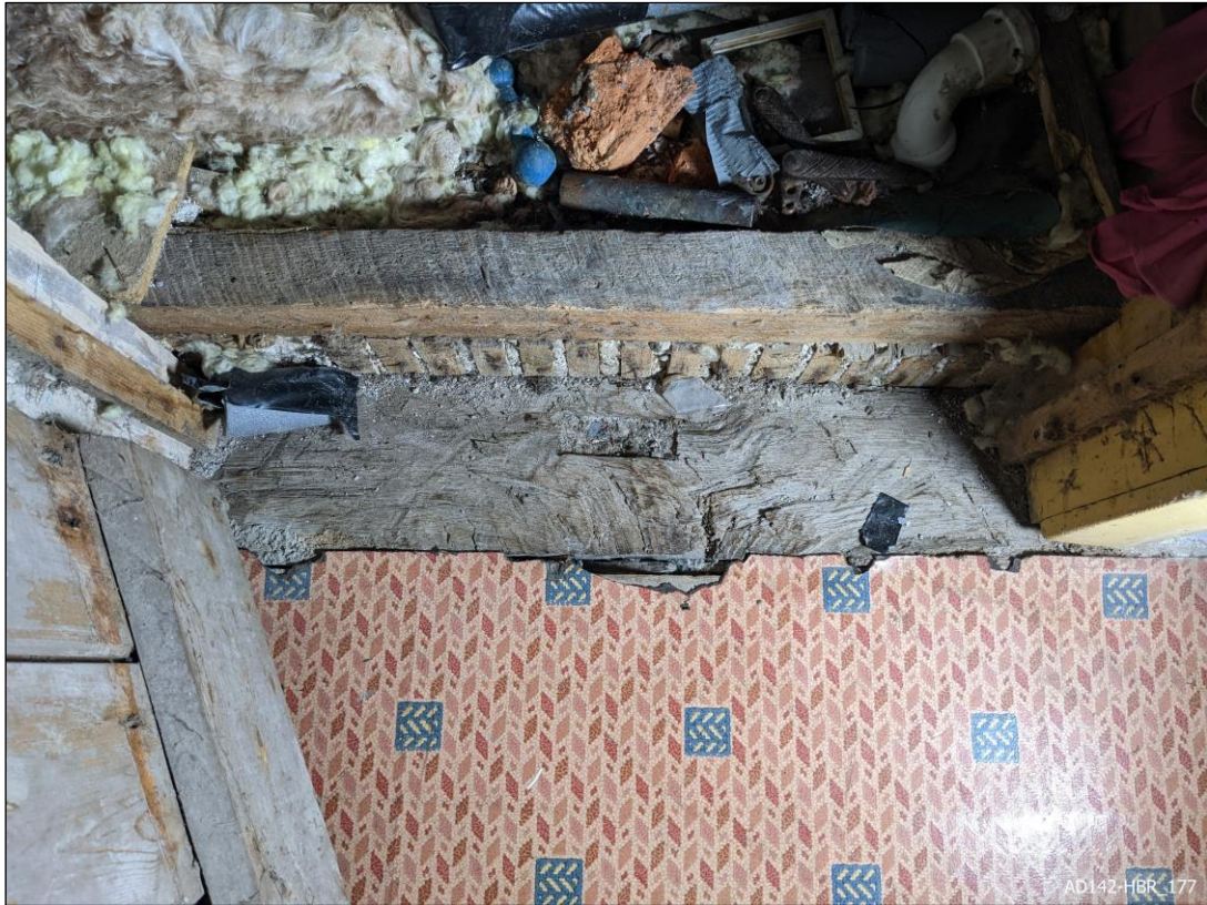
Plate 177 – View north, showing empty mortice in tie beam of Truss 4.
