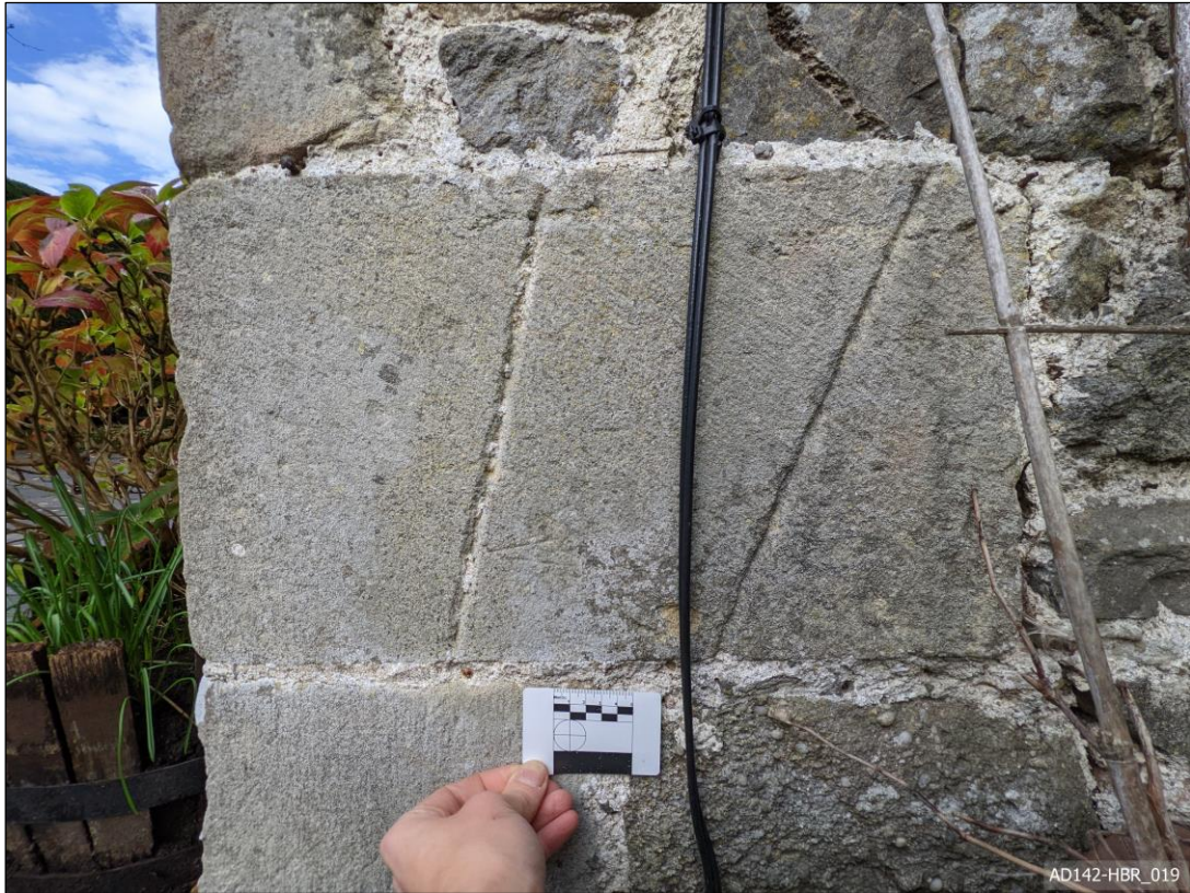
Plate 19 – View north, showing false voussoir window or doorway head reused as quoin.
