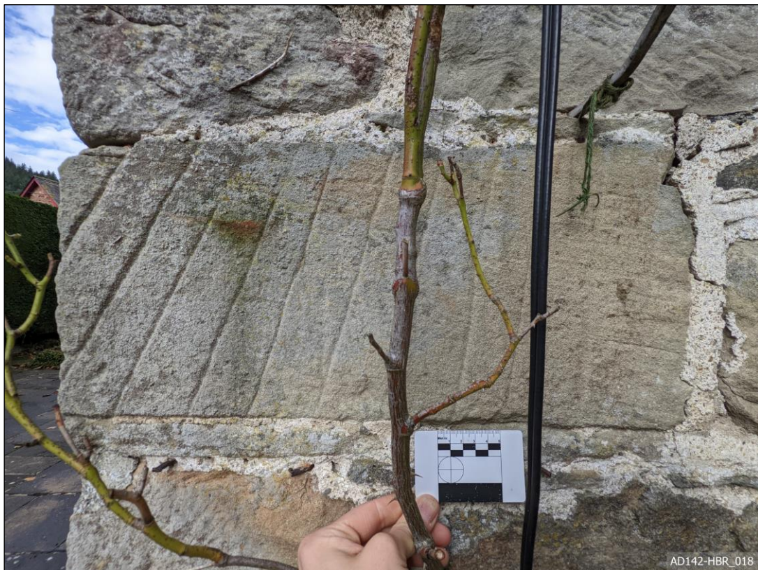
Plate 18 – View north, showing false voussoir window or doorway head reused as quoin.
