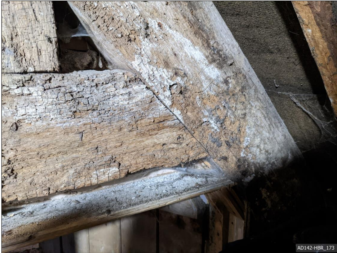
Plate 173 – View south-west, showing collar joint of Truss 4. N.B. decay.
