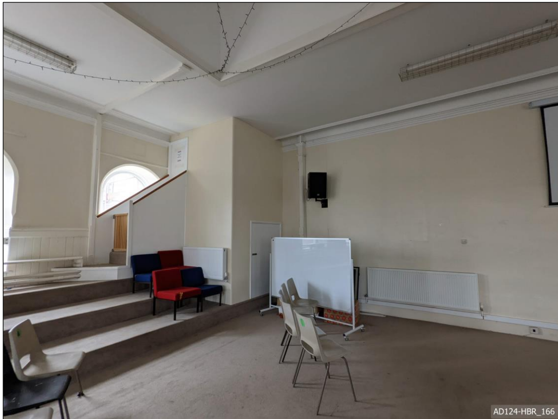
Plate 166 – View south-west, showing stair and cupboard at first floor of lecture hall.
