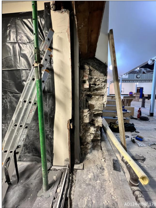
Plate 178 – View south, showing brick blocking (left) and stone of chapel wall, in lime mortar.
