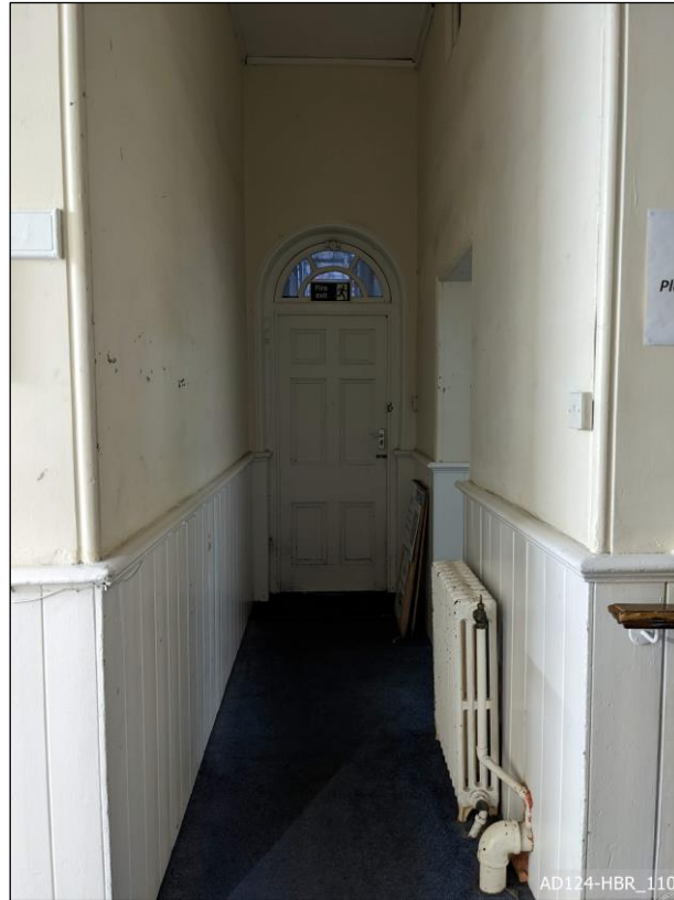
Plate 110 – View south, showing corridor between chapel and school rooms, with external doorway.
