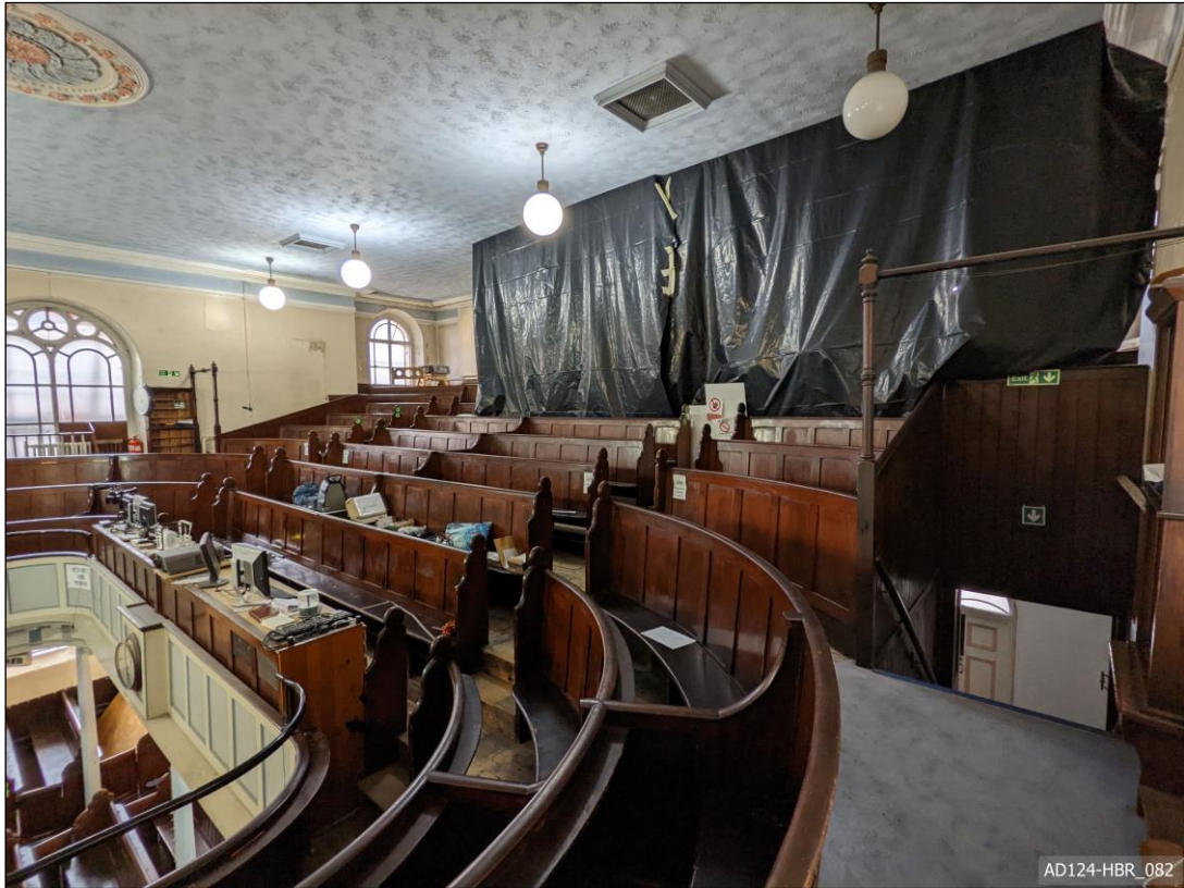
Plate 82 – View south-west, showing gallery and area of ceiling damage.
