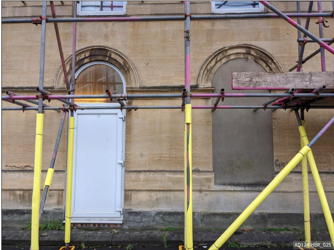
Plate 25 – View west, showing doorway and blocked window in east elevation of lecture hall.
