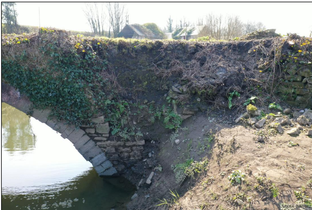
Plate 12 – Pre-works – North elevation, showing collapsed spandrel and wing wall.
