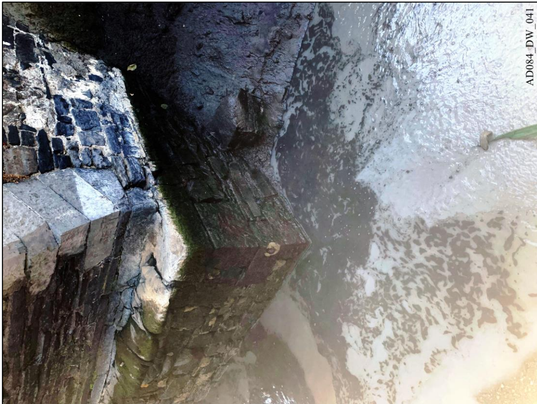
Plate 41 – During works – View east, showing east abutment and ledge of earlier abutment.
