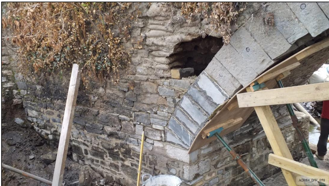
Plate 58 – During works – North elevation, showing removal of east spandrel repair and masonry rebuild.
