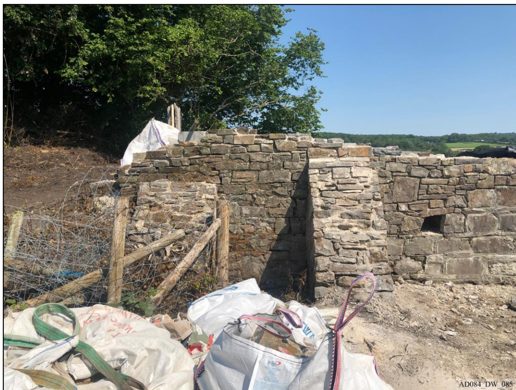
Plate 85 – During works – South elevation, showing repair of buttresses to west wing and retaining wall.
