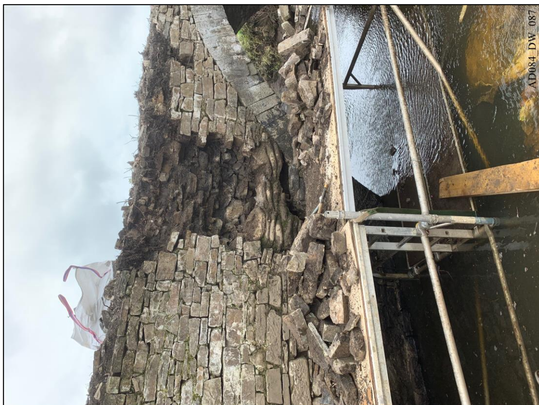
Plate 87 – During works – North elevation, showing collapse of east spandrel.
