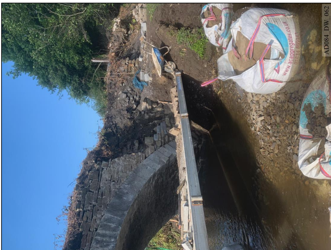
Plate 62 – During works – North elevation, showing dismantling of masonry to spandrel and wing wall.
