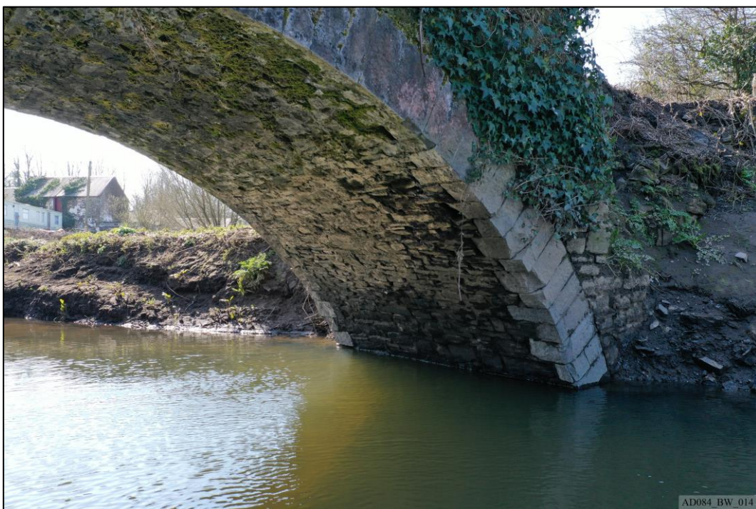
Plate 14 – Pre-works – Arch and barrel vault of west abutment, viewed from north, showing damage.
