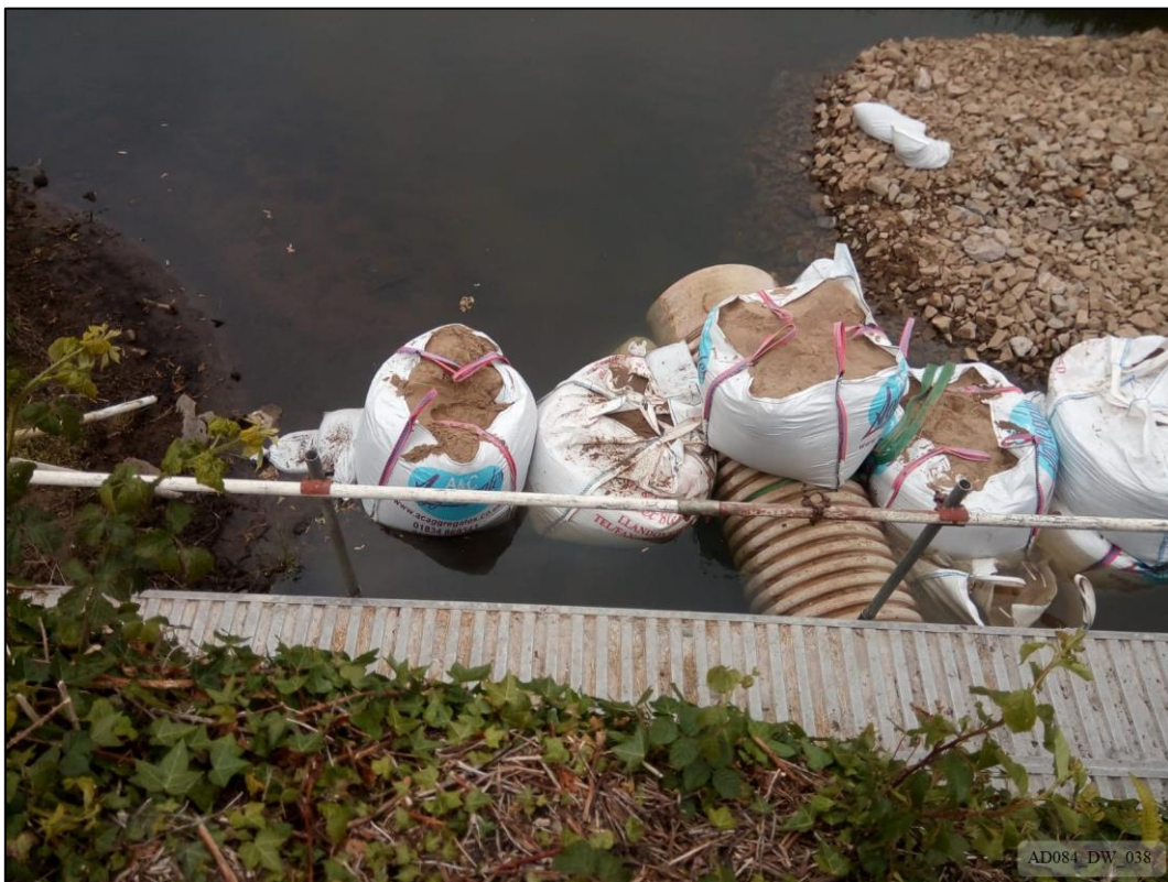
Plate 38 – During works – View down north elevation from deck, showing damming of river.
