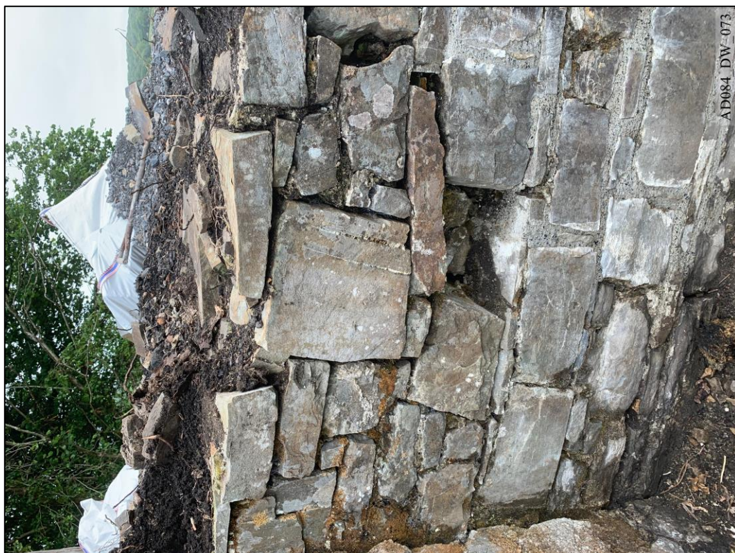
Plate 73 – During works – South elevation, showing west wing wall masonry deterioration.
