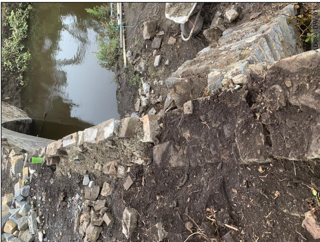
Plate 78 – During works – View east, showing top of masonry to wing and retaining wall.
