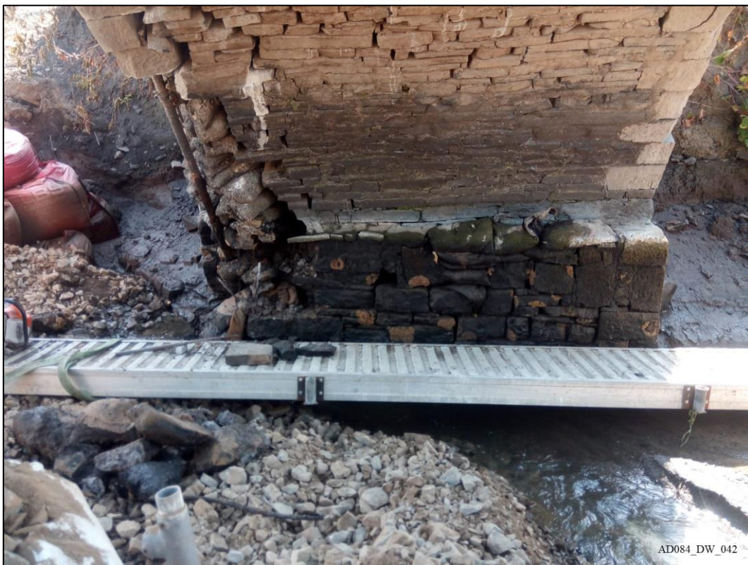
Plate 42 – During works – View east, showing east abutment and ledge of earlier abutment.
