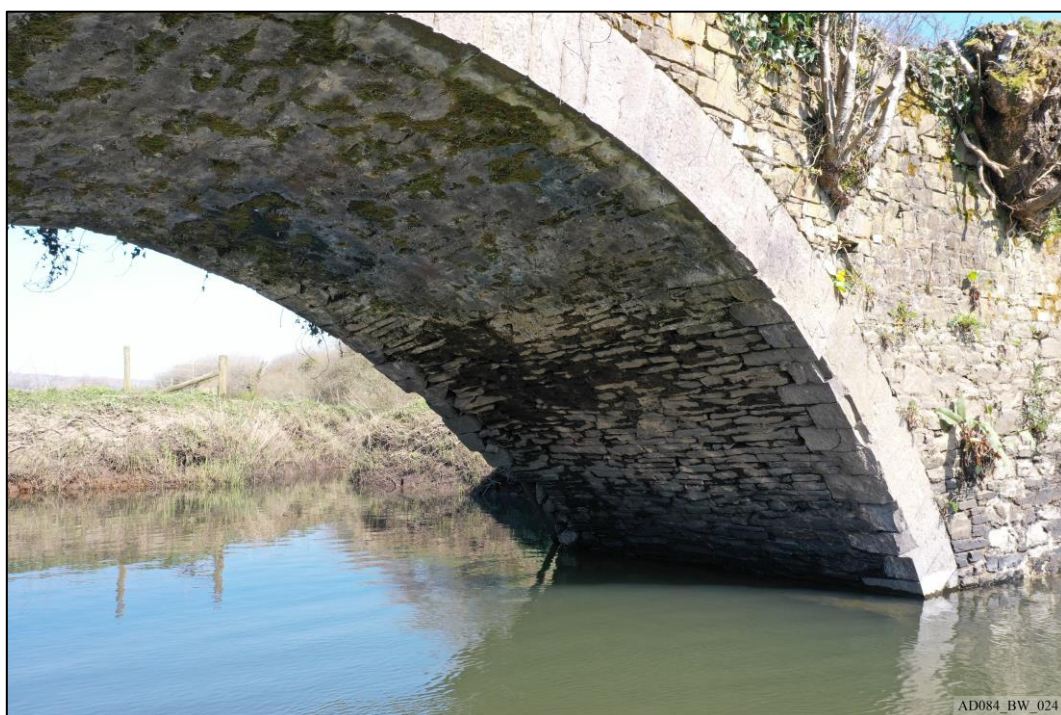
Plate 24 – Pre-works – Arch and barrel vault of west abutment, viewed from south, showing damage.
