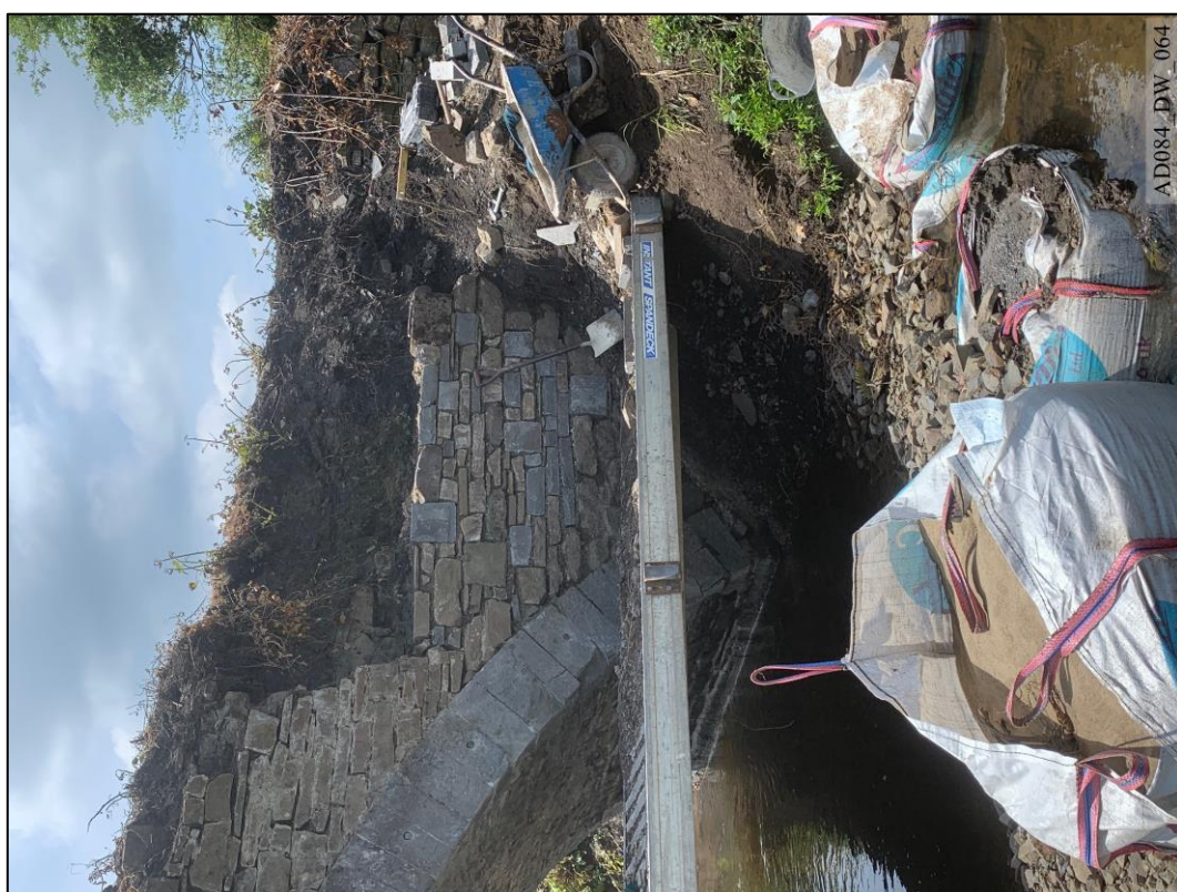
Plate 64 – During works – North elevation, showing rebuilding of west spandrel and wing wall.
