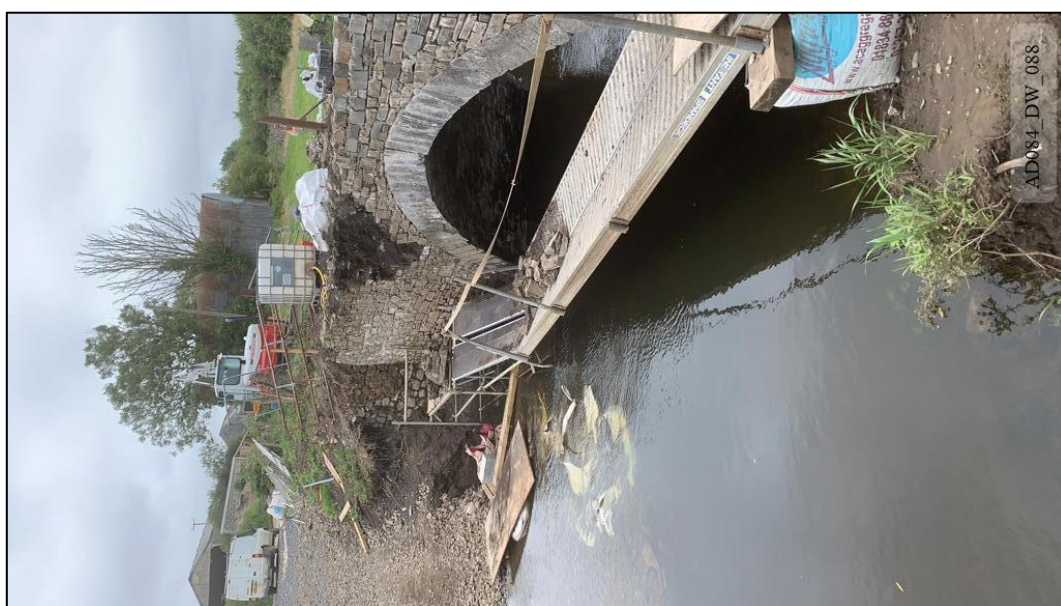
Plate 88 – During works – North elevation, showing collapse of east spandrel.
