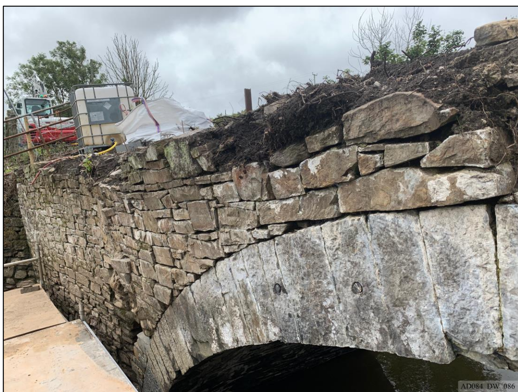
Plate 86 – During works – North elevation, showing bulge in masonry to east spandrel.
