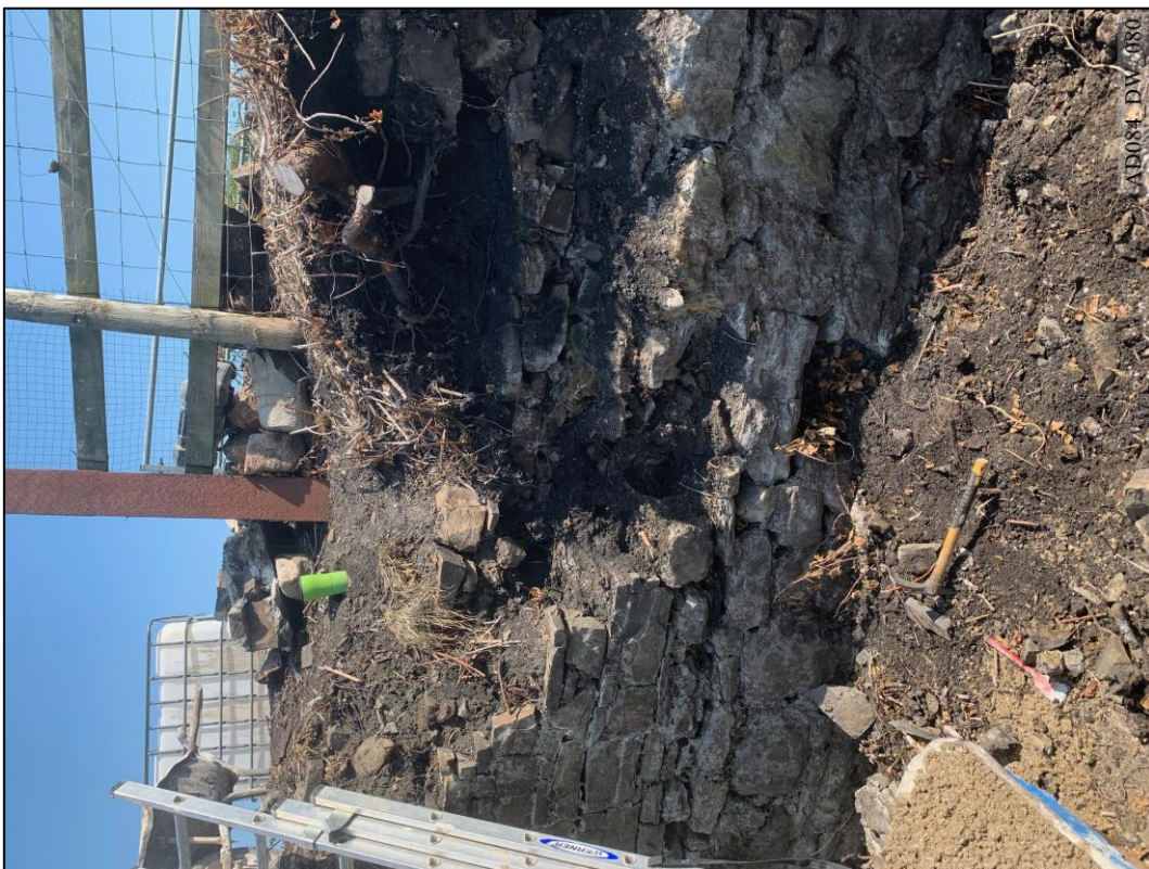
Plate 80 – During works – South elevation, showing damage to east wing wall.
