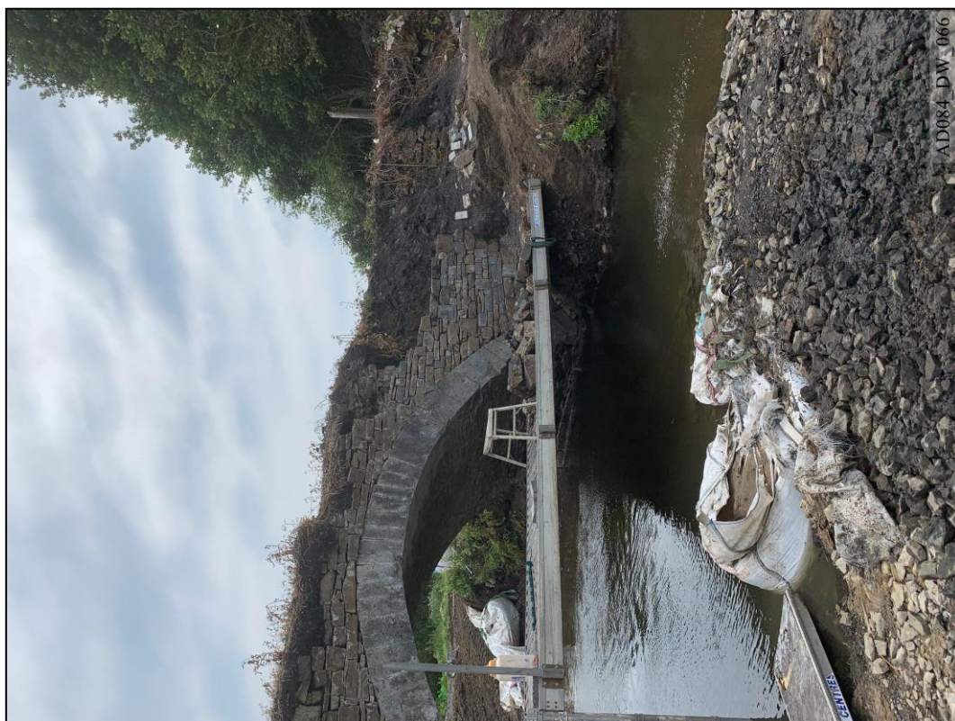
Plate 66 – During works – North elevation, showing rebuilding of west spandrel and wing wall.
