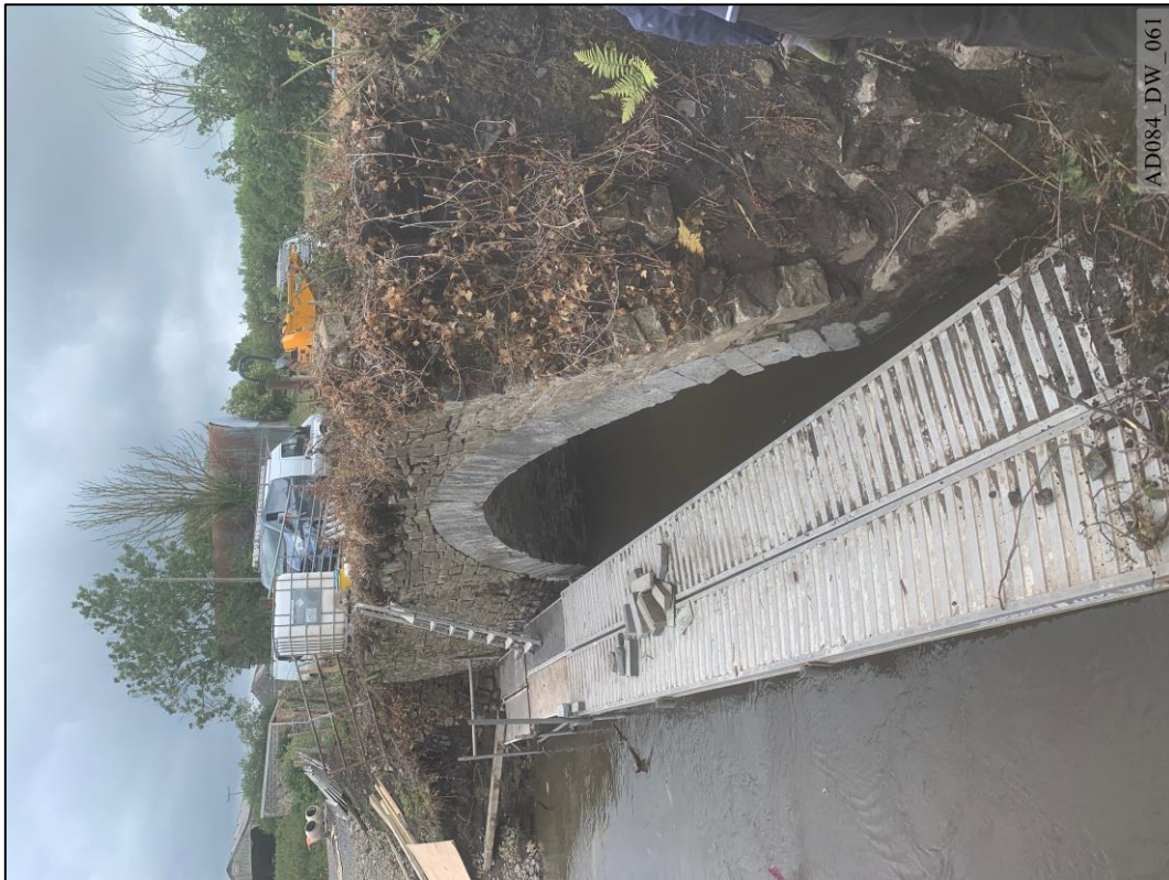
Plate 61 – During works – North elevation, showing dismantled and lean of surviving masonry.
