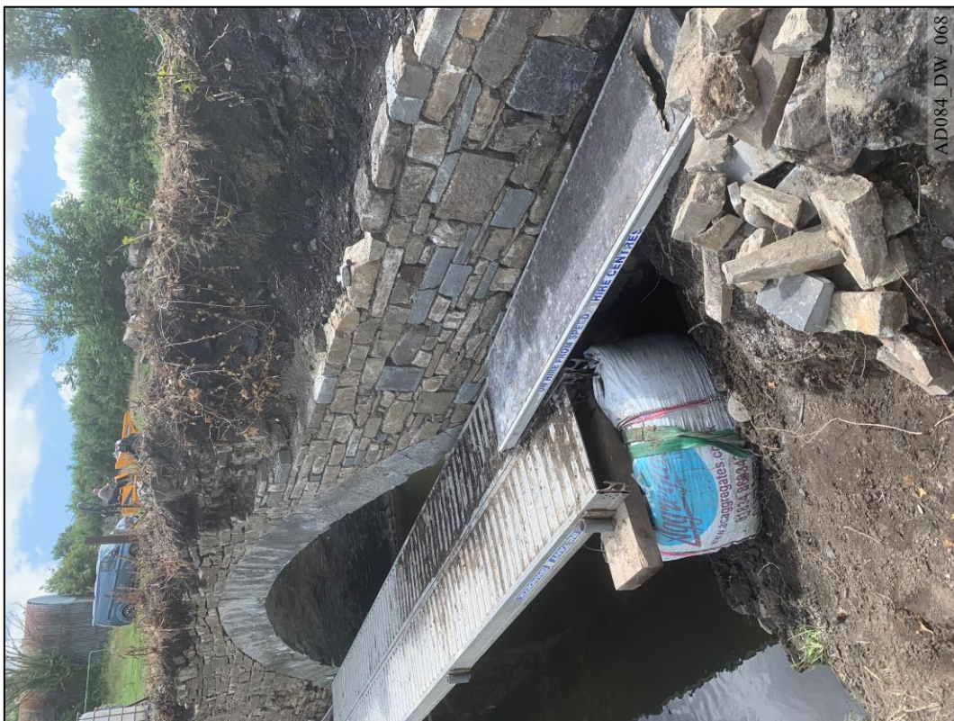
Plate 68 – During works – North elevation, showing rebuilding of masonry to spandrel and wing wall.
