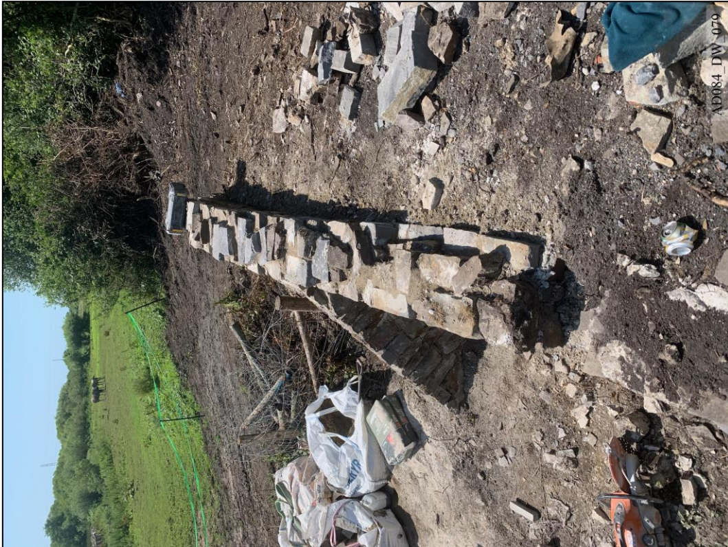
Plate 79 – During works – South elevation, view west showing rebuilt masonry of wing and retaining wall.
