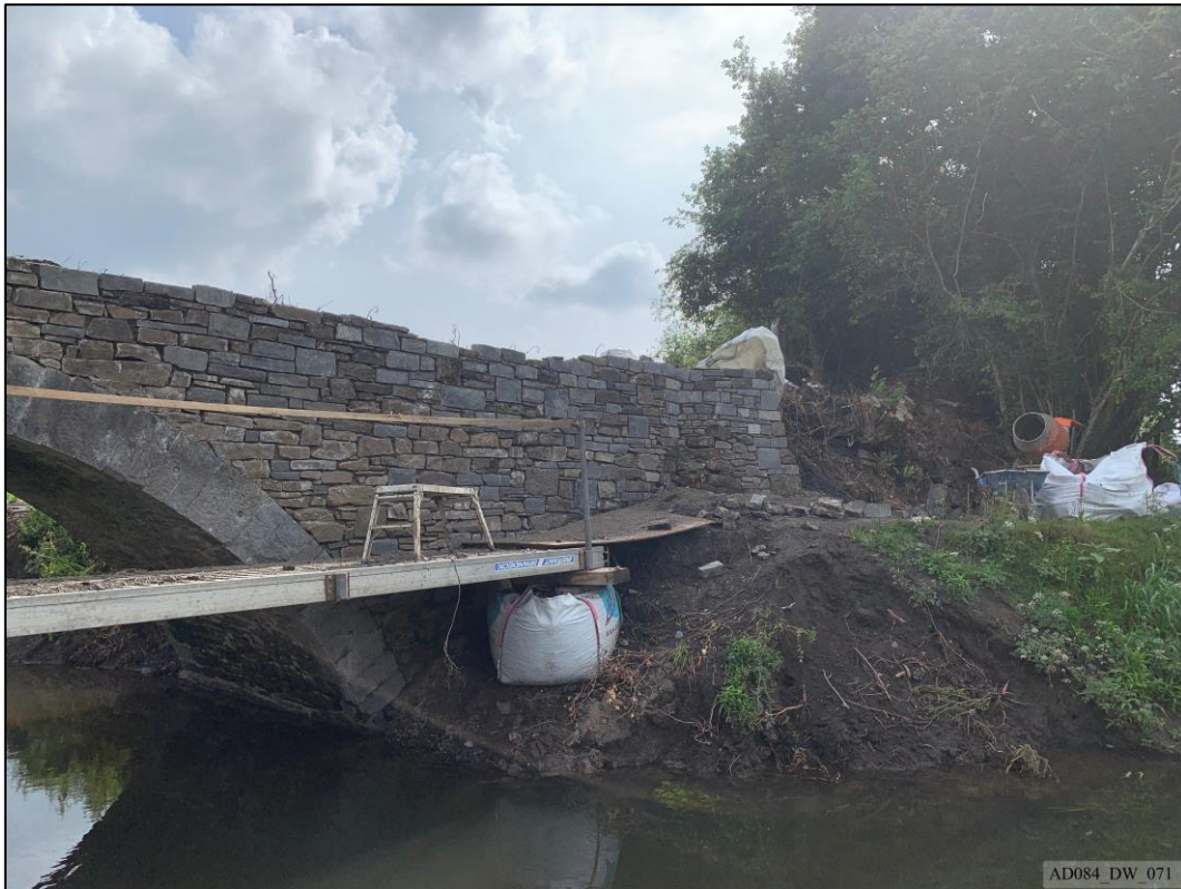
Plate 71 – During works – North elevation, showing completed west spandrel and wing wall rebuild.
