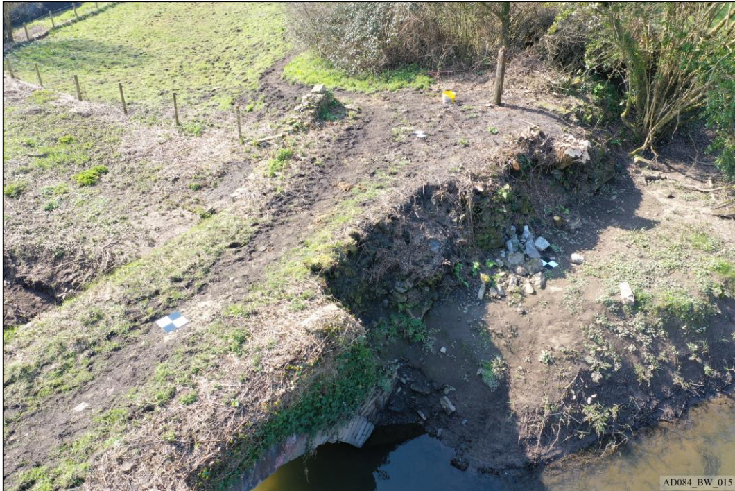
Plate 15 – Pre-works – North elevation, west spandrel and wing wall collapse.
