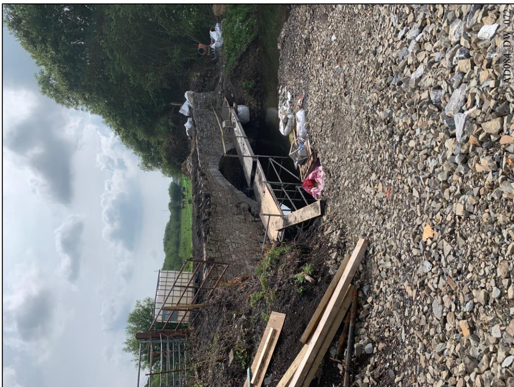
Plate 72 – During works – North elevation, showing completed west spandrel and wing wall rebuild.
