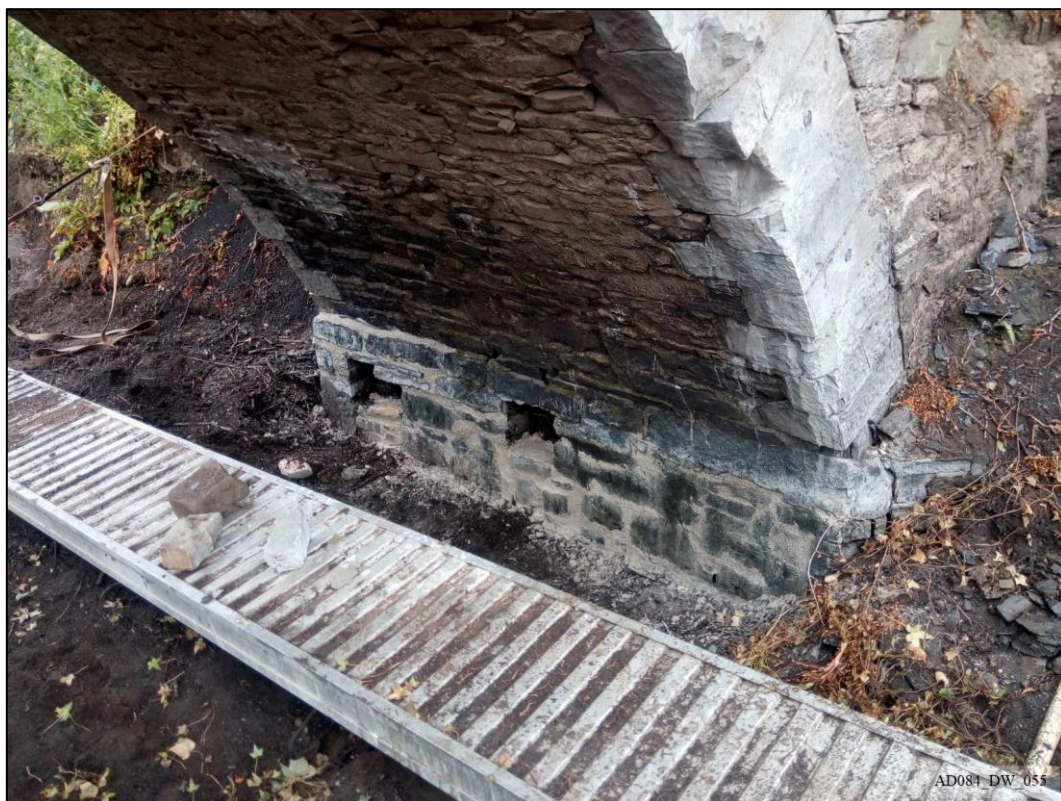
Plate 55 – During works – View west, showing earlier abutment with remains of splayed wing wall.
