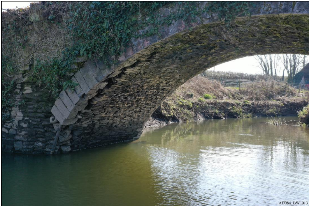
Plate 13 – Pre-works – Arch and barrel vault of east abutment, viewed from north, showing damage.
