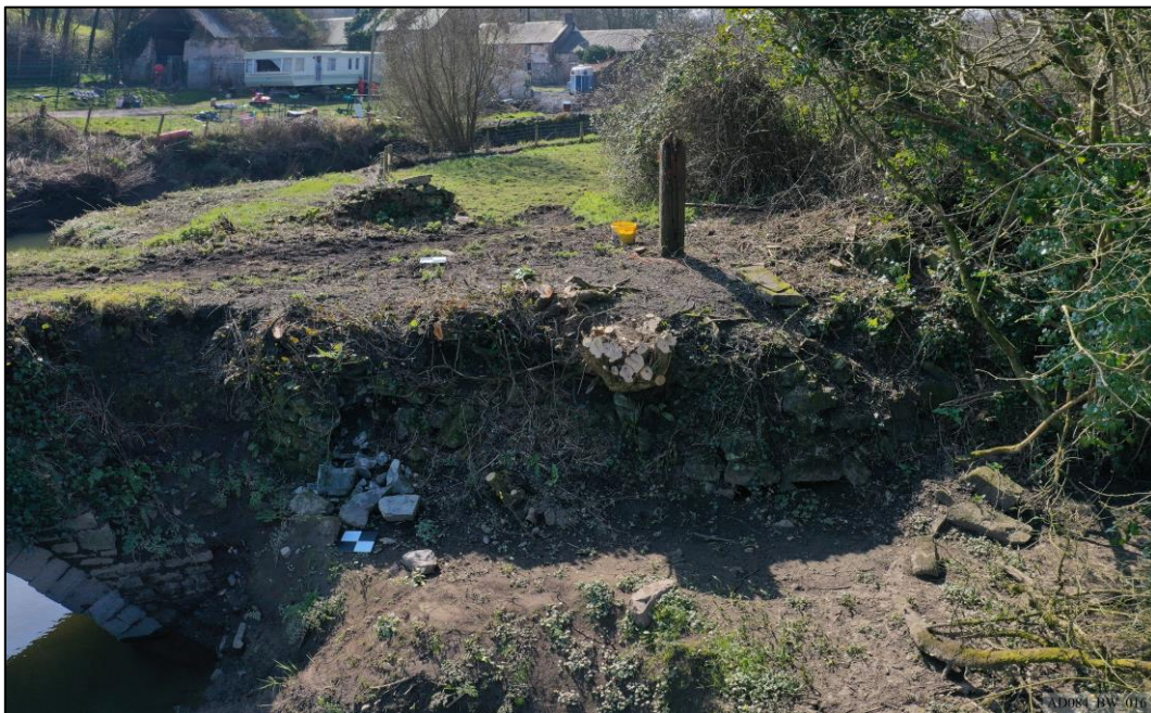
Plate 16 – Pre-works – North elevation, west spandrel and wing wall collapse.
