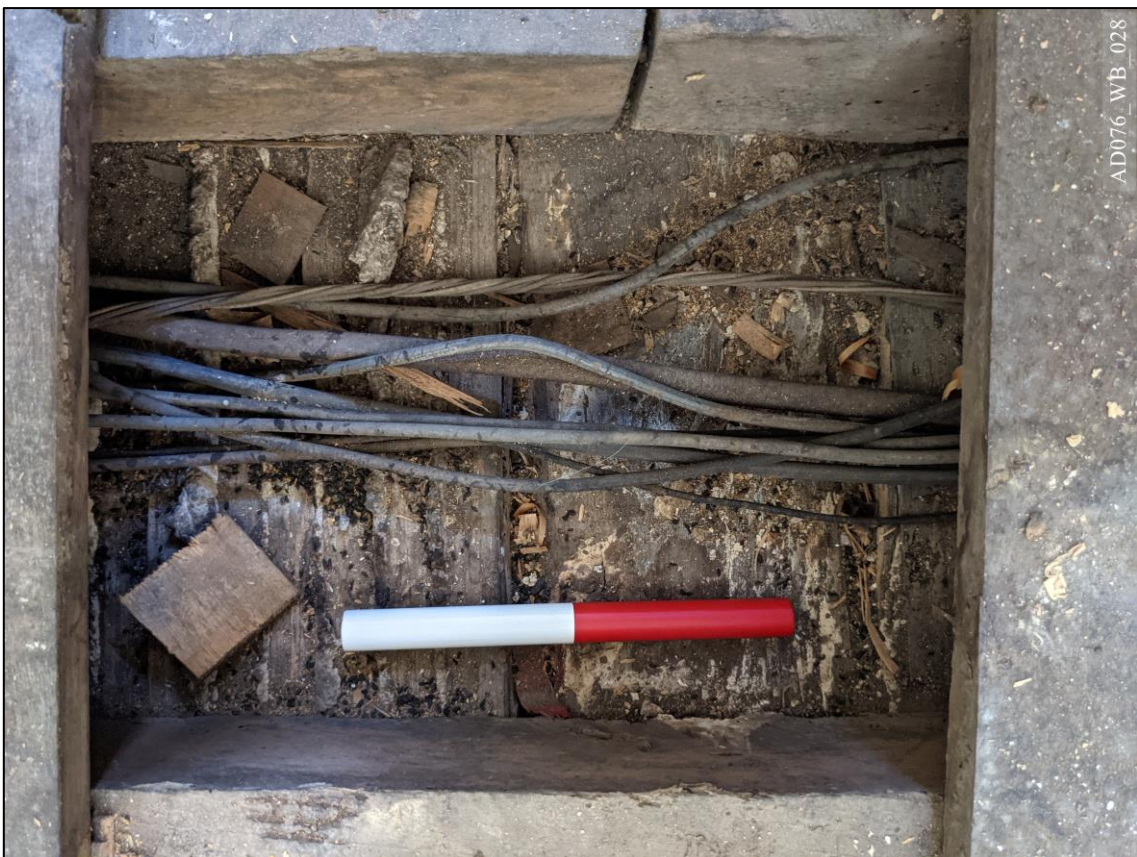
Plate 28 – 1930s lead sheathed electrical cables [FF.10].
