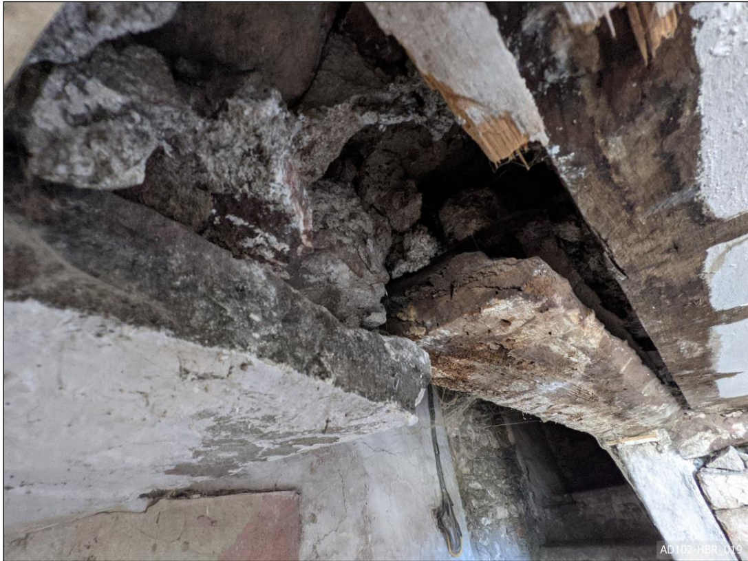
Plate 19 – Doorway B – View north, showing reused screen head as lintel in doorway from drawing room.
