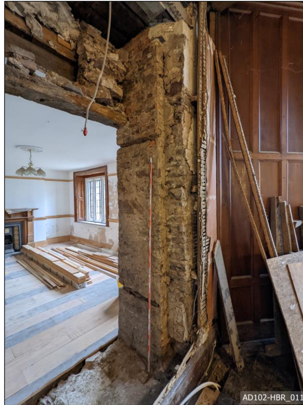
Plate 11 – Doorway A – View south, showing south reveal of doorway with brick lining.
