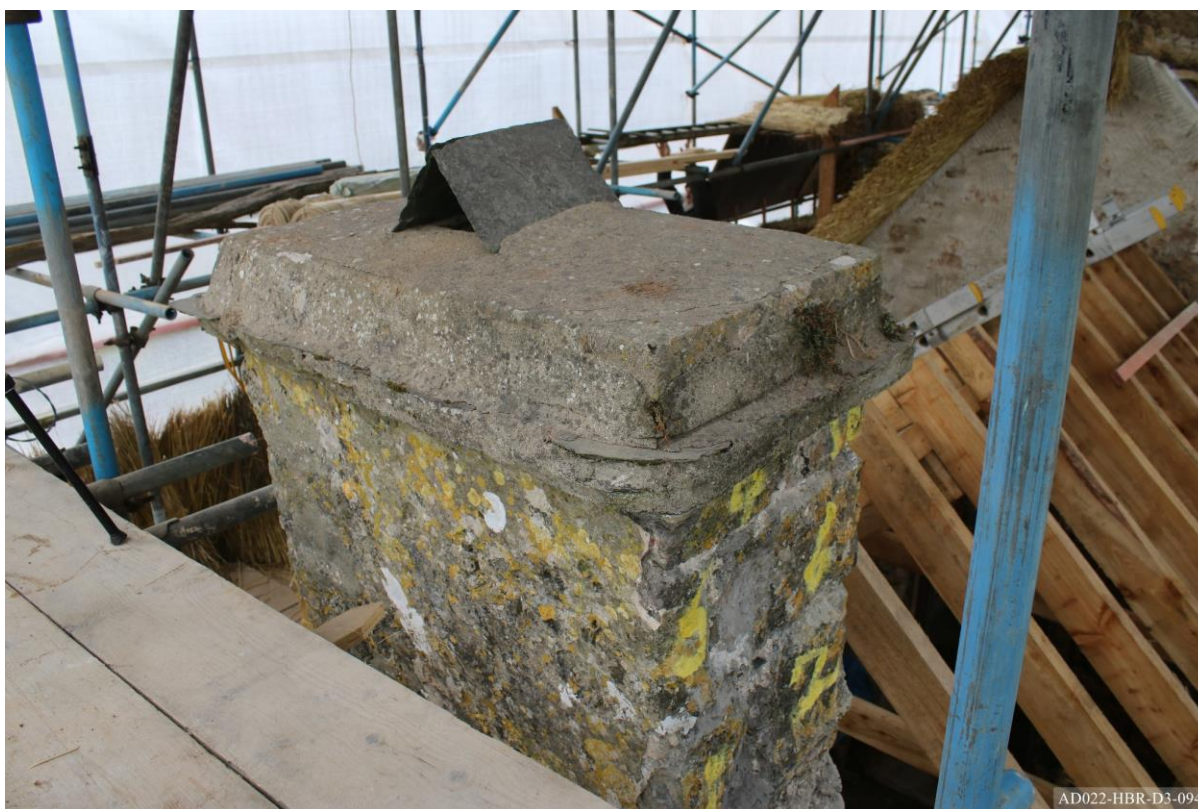
Plate 94 – View towards north-west, showing south and east elevation of chimney prior to dismantling.
