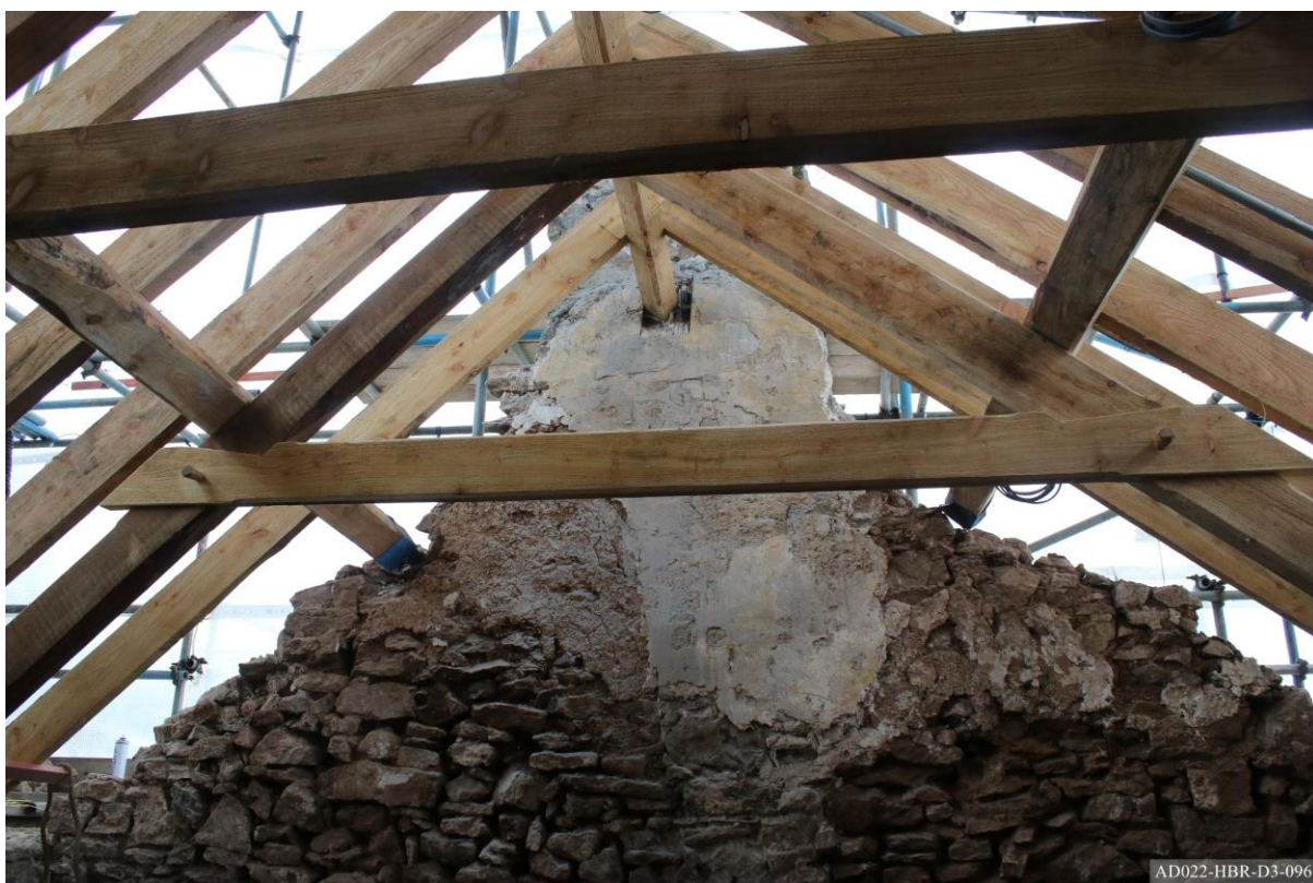
Plate 96 – View towards south of south extension, showing internal elevation of gable wall before dismantling.
