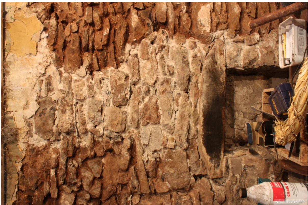
Plate 82 – View towards south of extension, showing inserted fireplace and flue, made clear by use of lime mortar.
