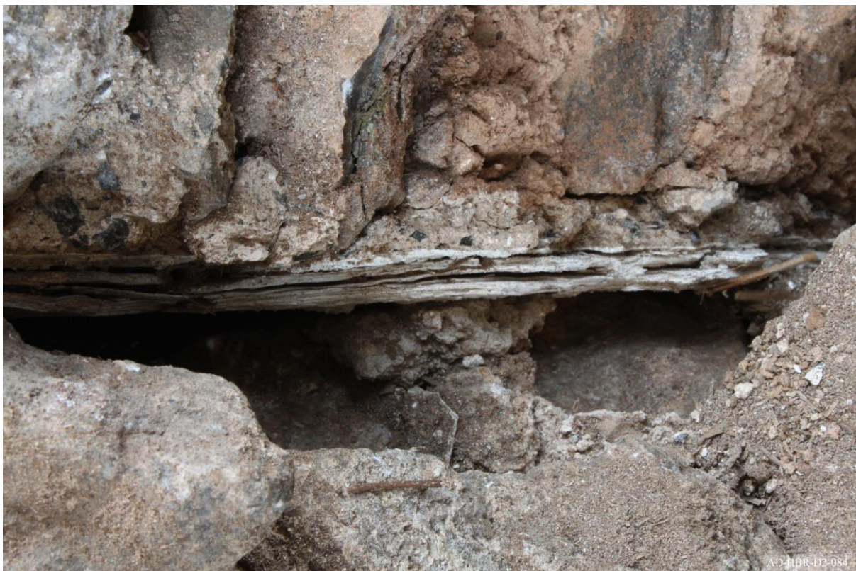
Plate 84 – View towards west of cottage, showing limewash layers in joint of wall after rebuild to outshut.
