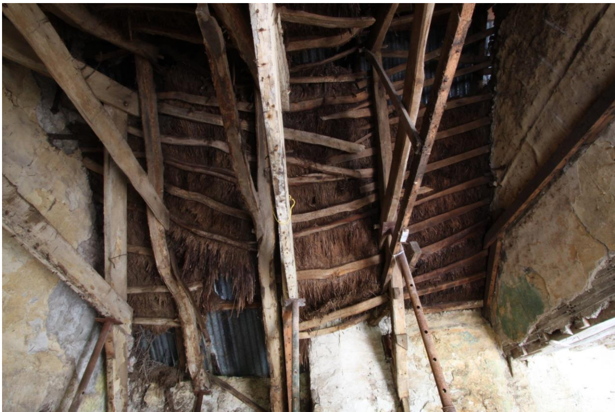
Plate 34 – View towards west of cottage, showing trusses 4-8, thatching purlins and underthatch at south end of cottage.
