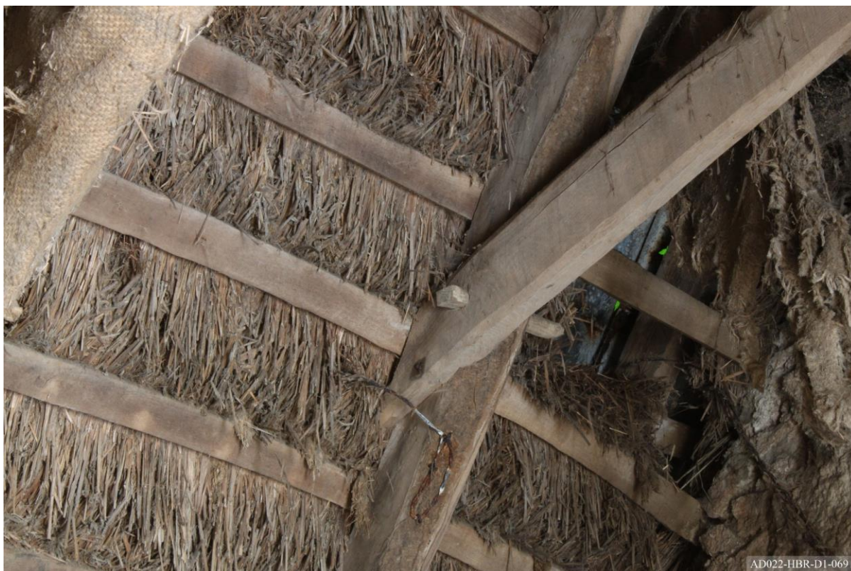
Plate 69 – View towards north of cottage, showing pegging detail to collar of truss 1.
