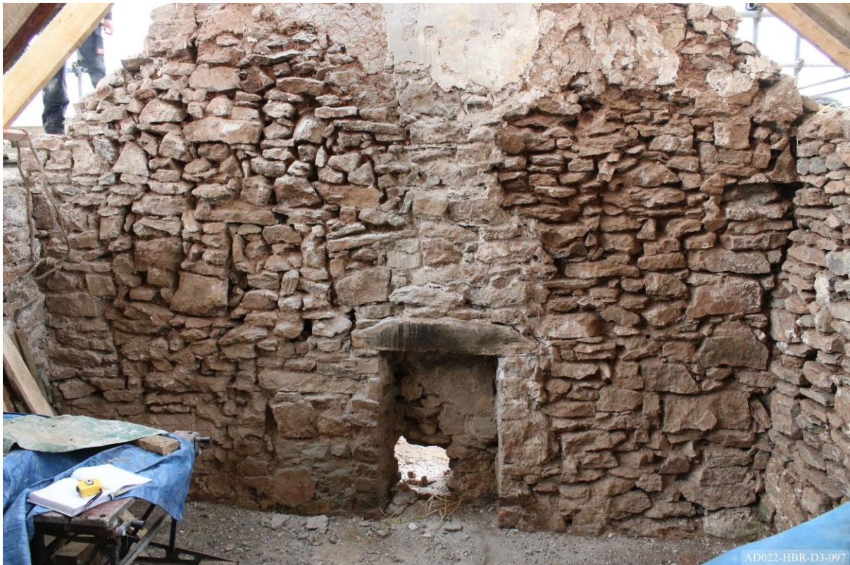
Plate 97 – View towards south of extension, showing south gable wall prior to dismantling.
