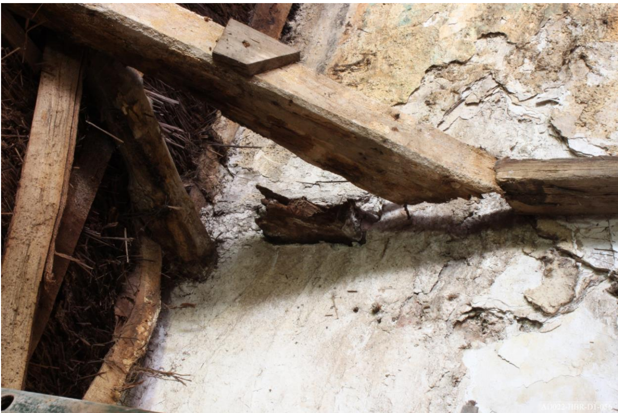
Plate 56 – View towards west of cottage, showing decayed end of west principal rafter to truss 4.
