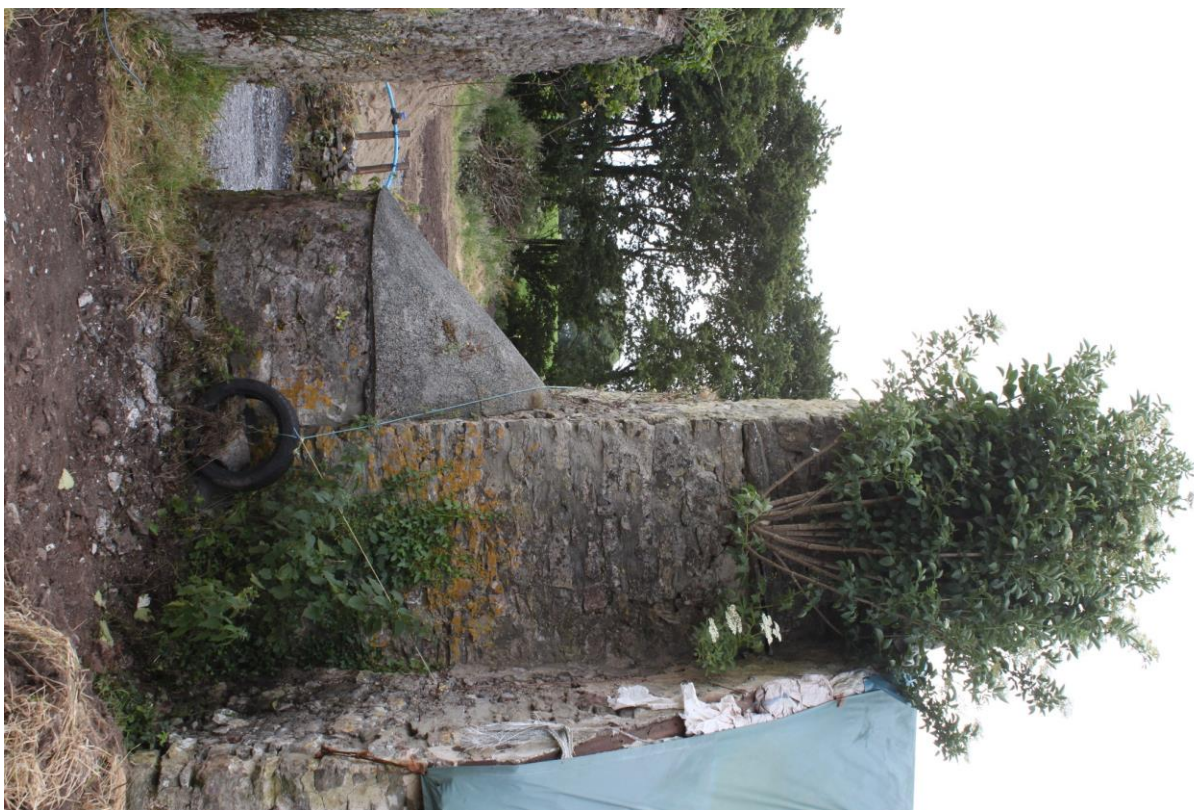
Plate 8 – View of west elevation of chimney fawr and later bread oven projecting to the north.
