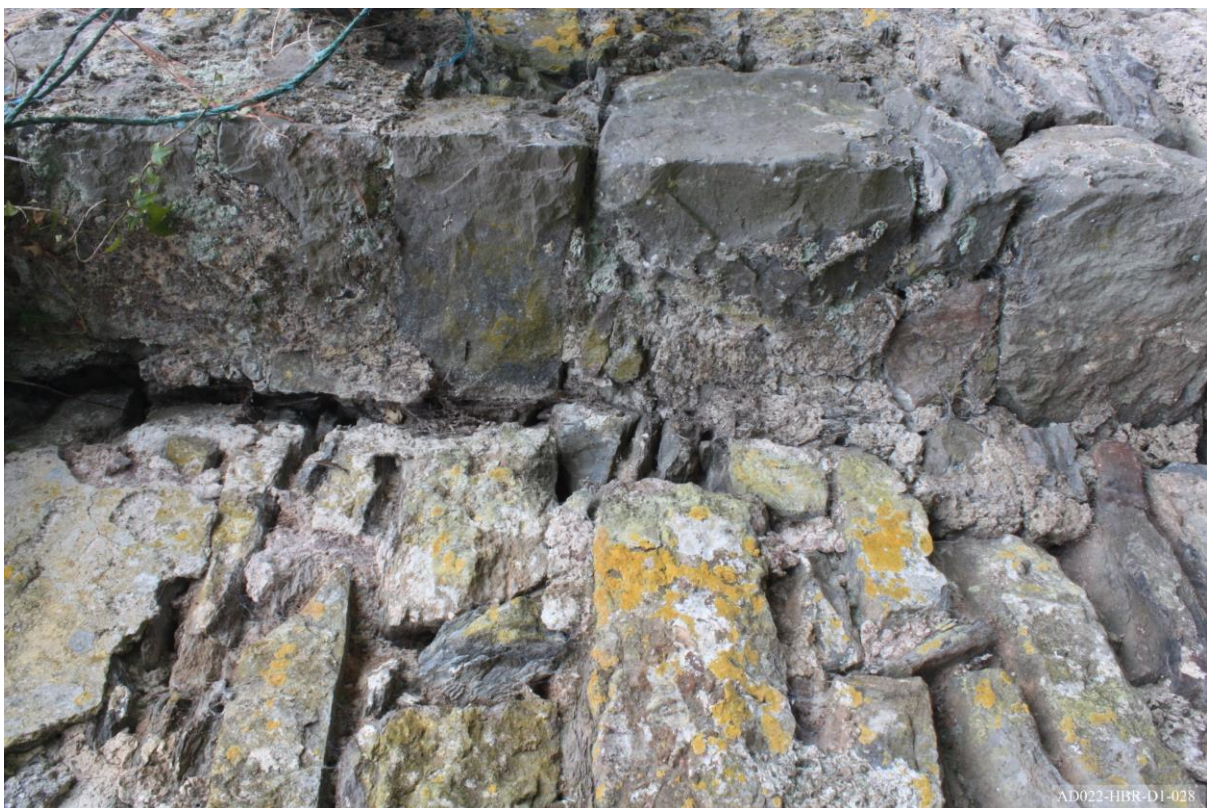
Plate 28 – View of east elevation, showing joint between lateral wall and lateral chimney.
