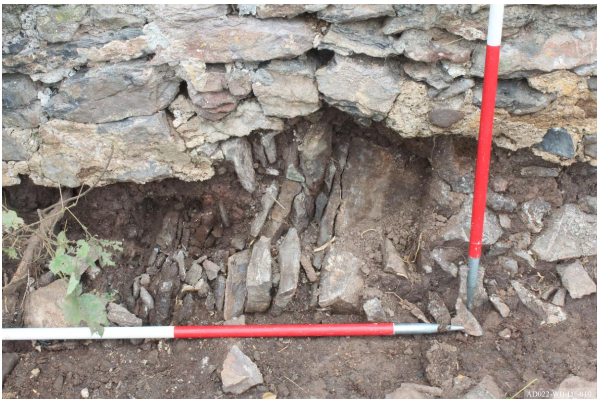
Plate 146 – Excavation to front of property (unmonitored), exposed wall of cottage built onto bedrock.
