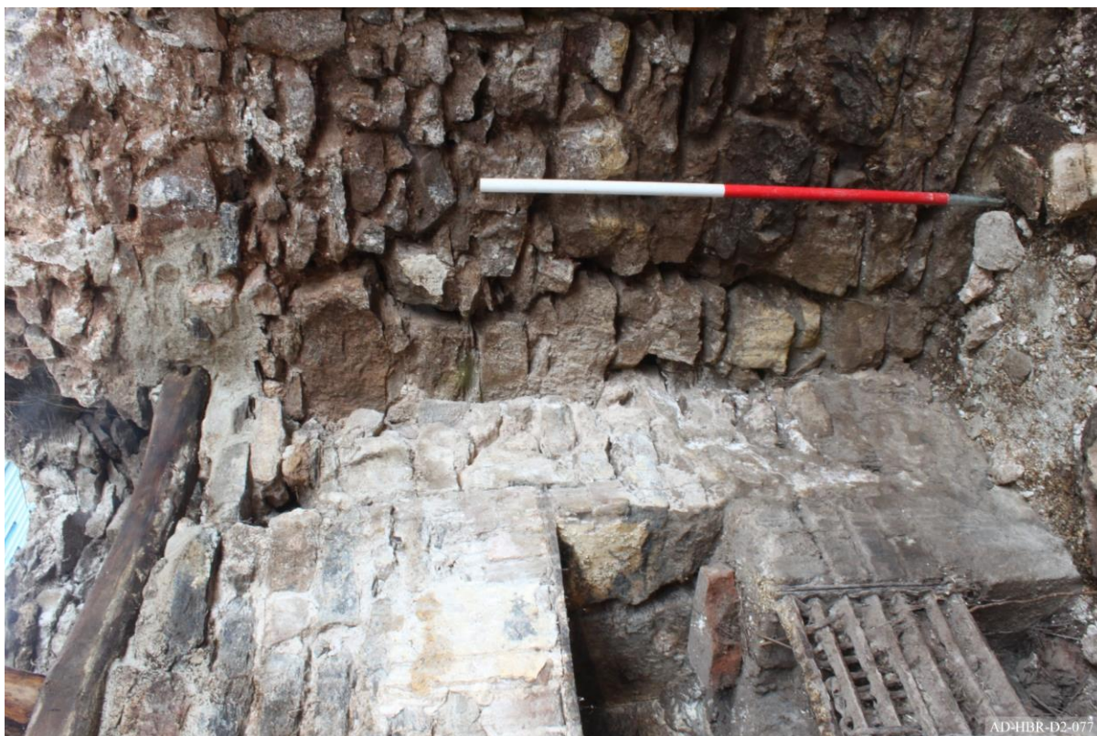
Plate 77 – View towards south-east of cottage, showing jointing between masonry of chimney and earlier wall.
