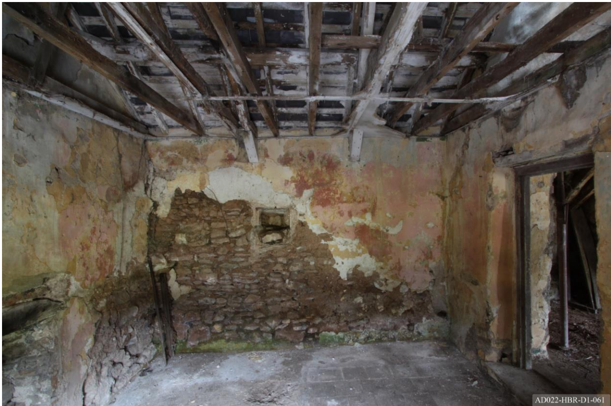
Plate 61 – View towards west of extension, showing blocked ventilation slit.
