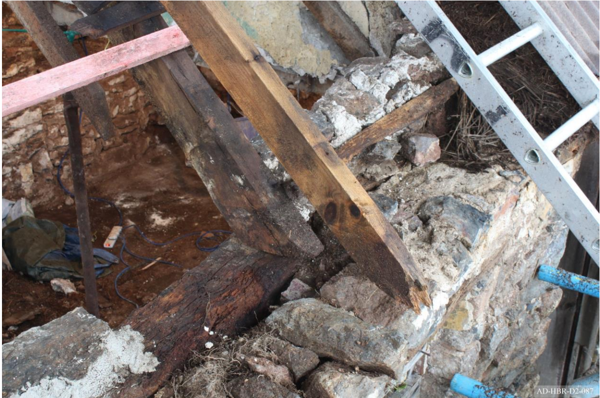
Plate 87 – View towards north-west of cottage, showing wall plate and principal rafter of truss 4.
