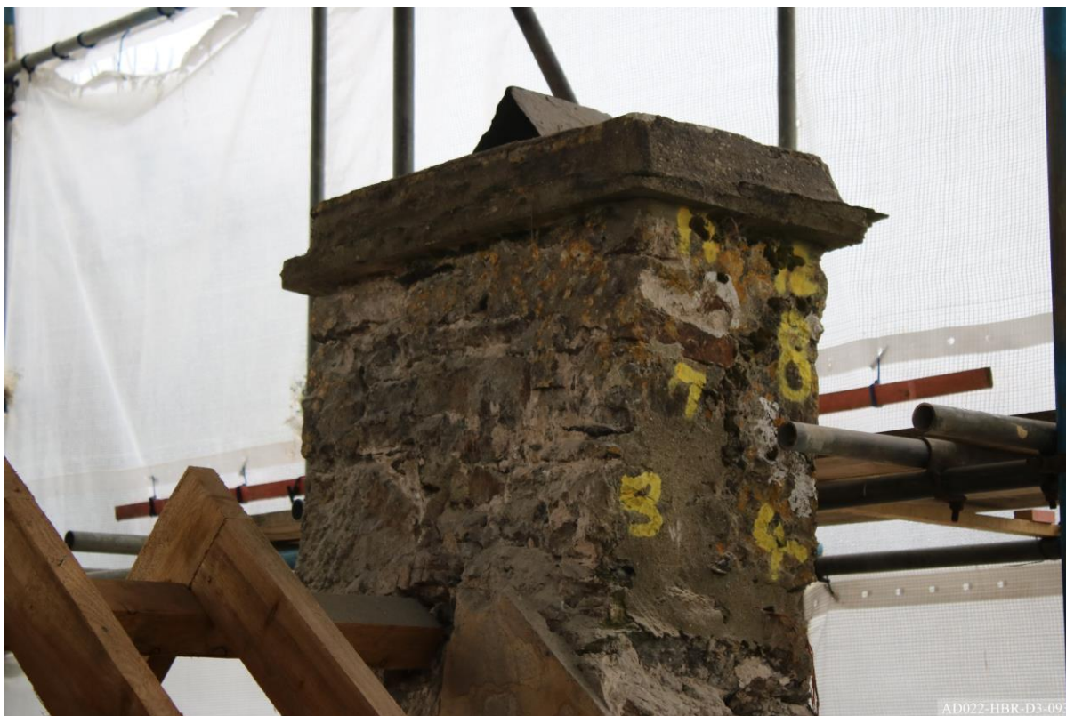
Plate 93 – View towards south-east, showing north and west elevation of chimney prior to dismantling.
