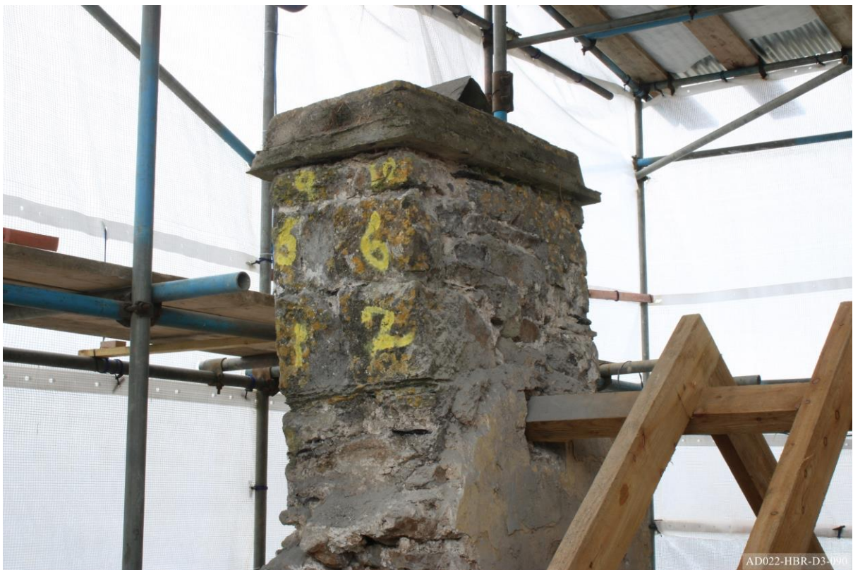
Plate 90 – View towards south-west, showing north and east elevation of chimney prior to dismantling.
