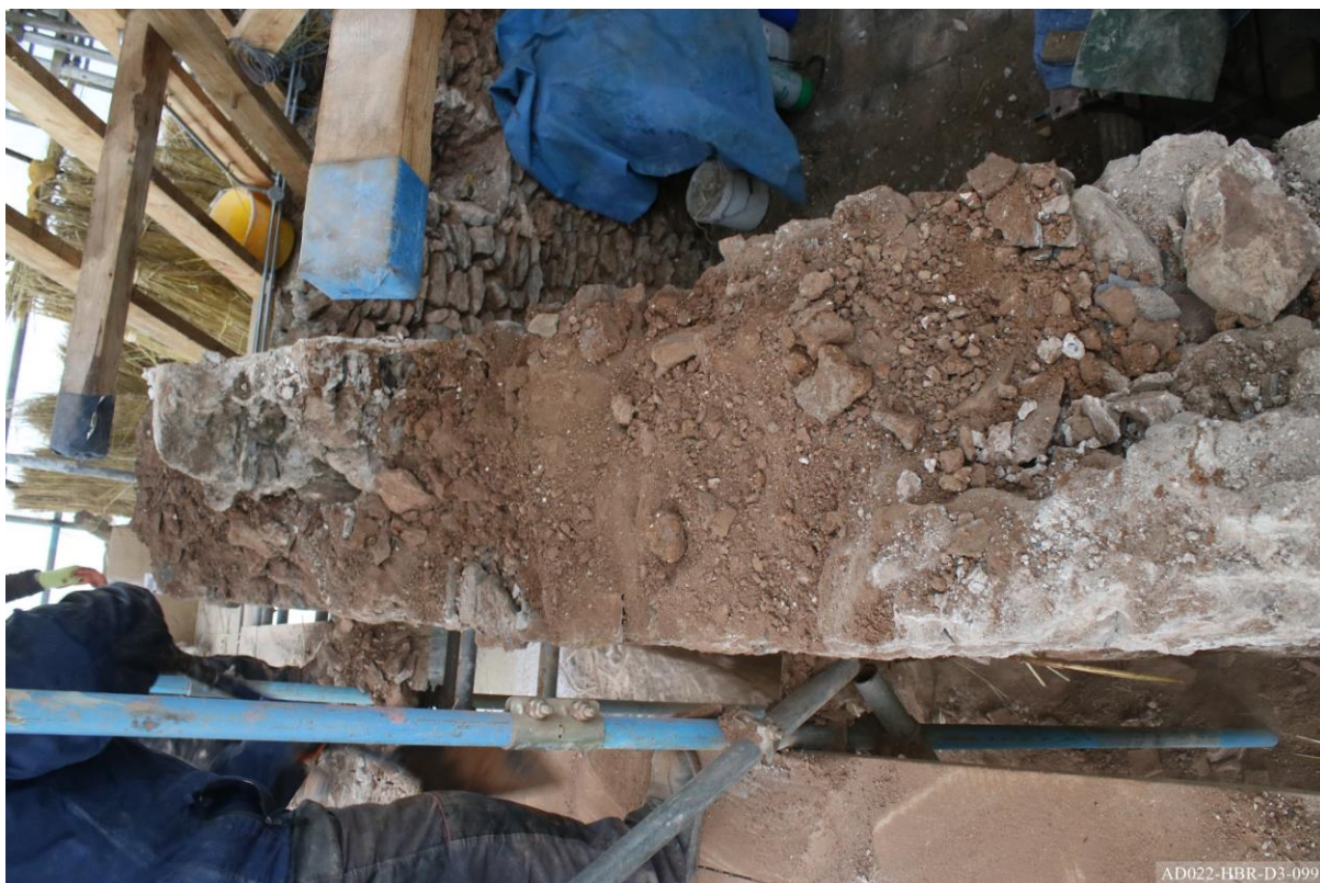
Plate 99 – View towards west, showing earth mortar and rubble fill to south gable wall.
