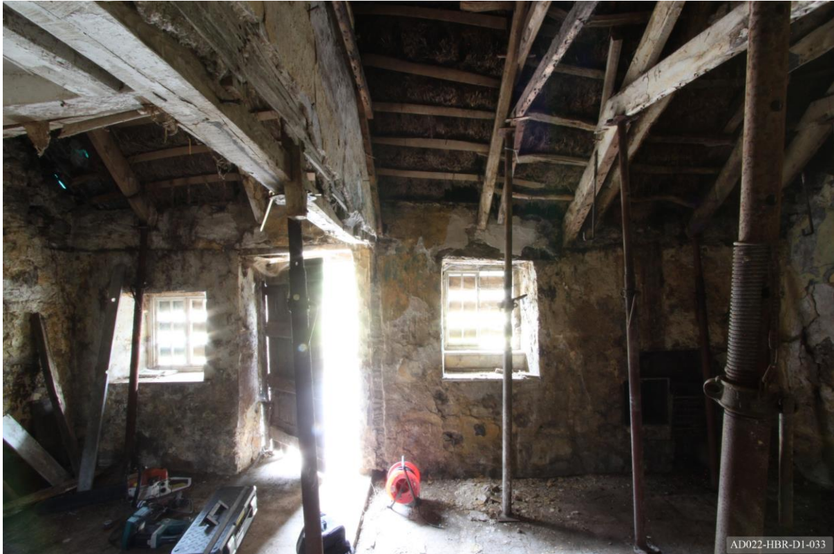
Plate 33 – View towards east of cottage, showing entrance, windows and 19 th century range.
