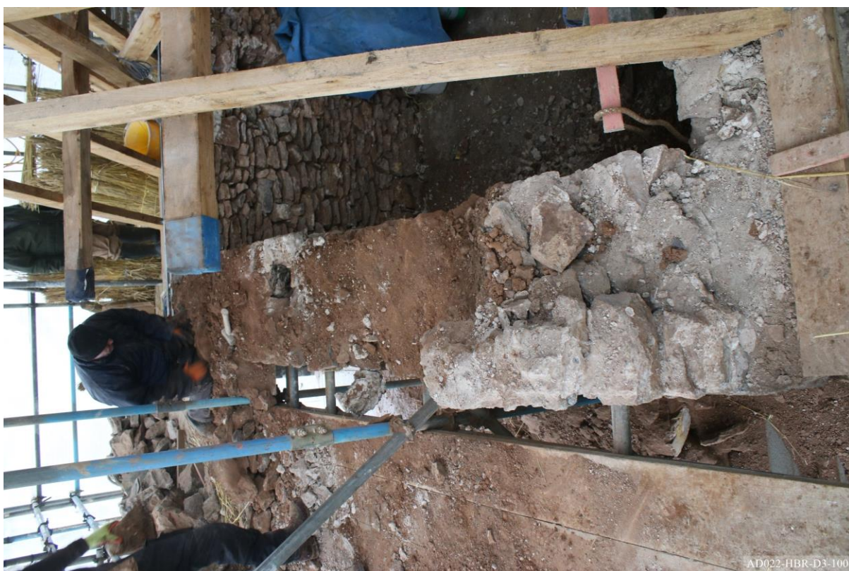
Plate 100 – View towards west, showing earth mortar and rubble fill to south gable wall.
