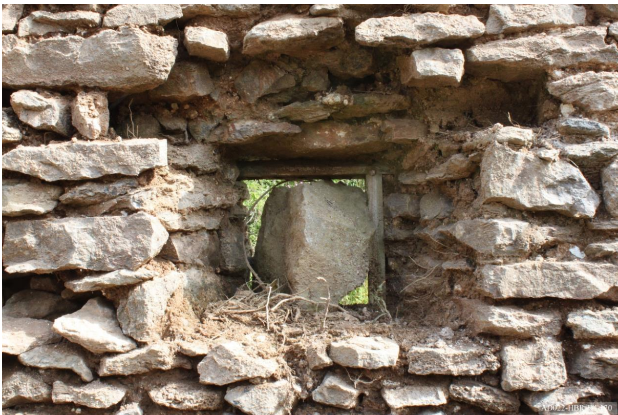
Plate 120 – View north of HB1, showing pine frame crudely blocked.
