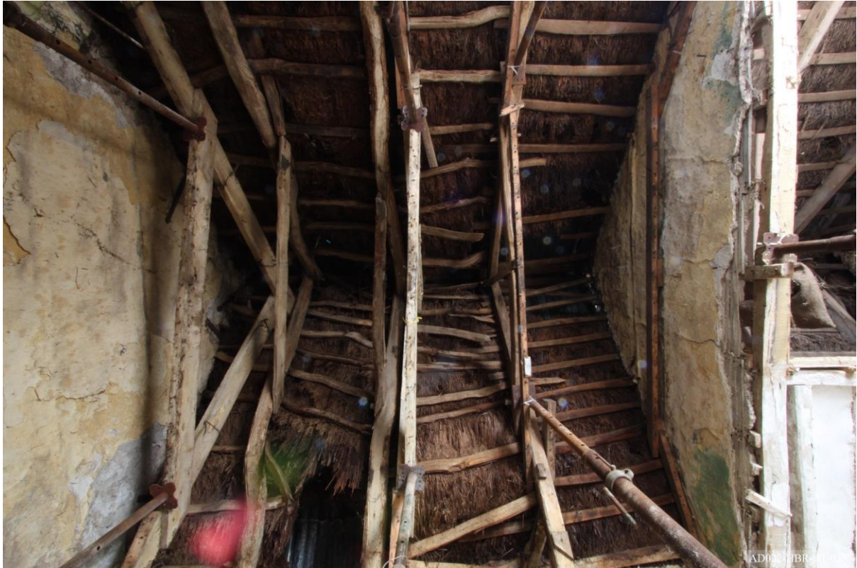
Plate 35 – View of roof structure of cottage, showing trusses 4-8, thatching purlins and underhatch at south end of cottage.
