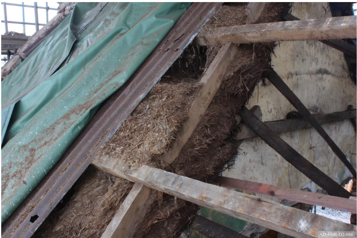
Plate 86 – View towards north of cottage, showing undercoat and weathering coats of thatch.
