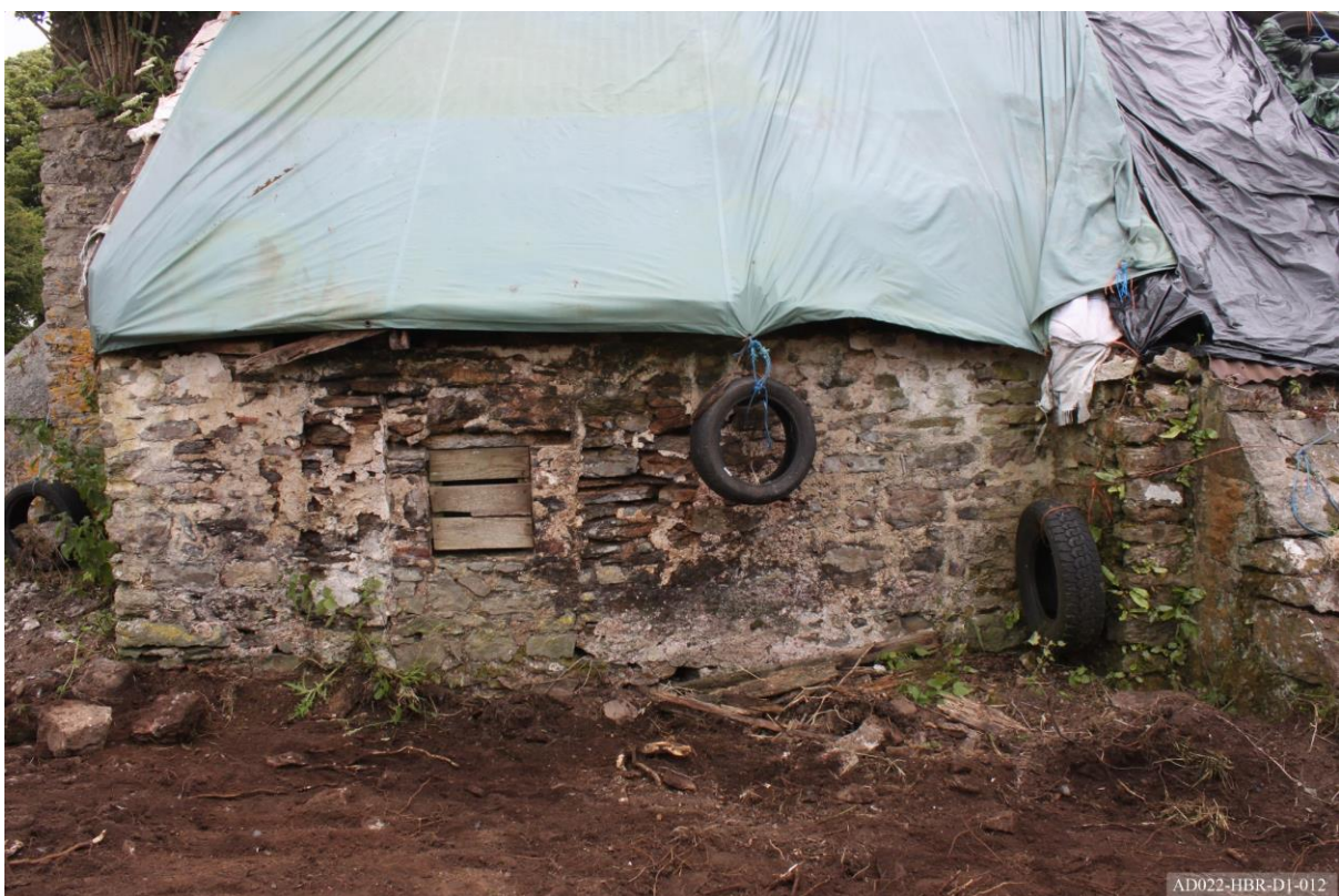
Plate 12 – View of west elevation of cottage, showing pantry window in blocked doorway.
