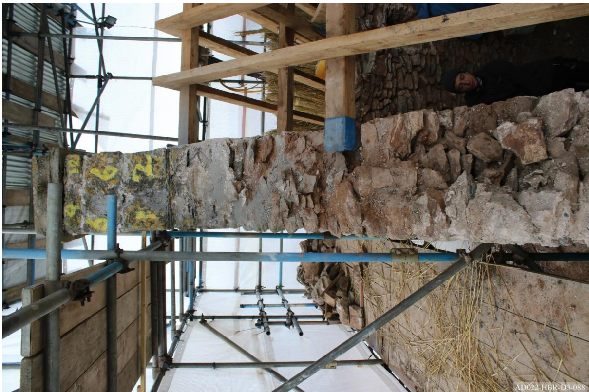
Plate 88 – View towards west, showing east elevation of chimney and south gable wall prior to dismantling.
