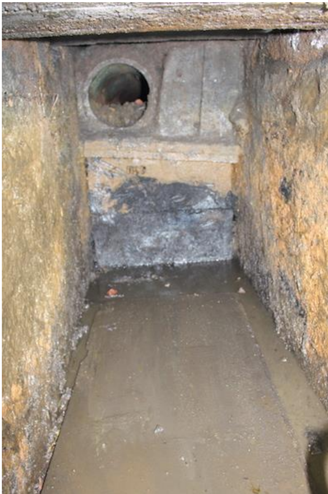
Plate 17. East-facing post-excavation photo of culvert [104], which is partially blocked with timber and laid with a land drain.
