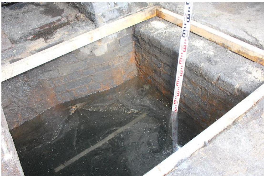
Plate 15. West facing post-excitation photo of sump [103] which was excavated to a depth of 1.6m but not bottomed. Also shows water ingress.
