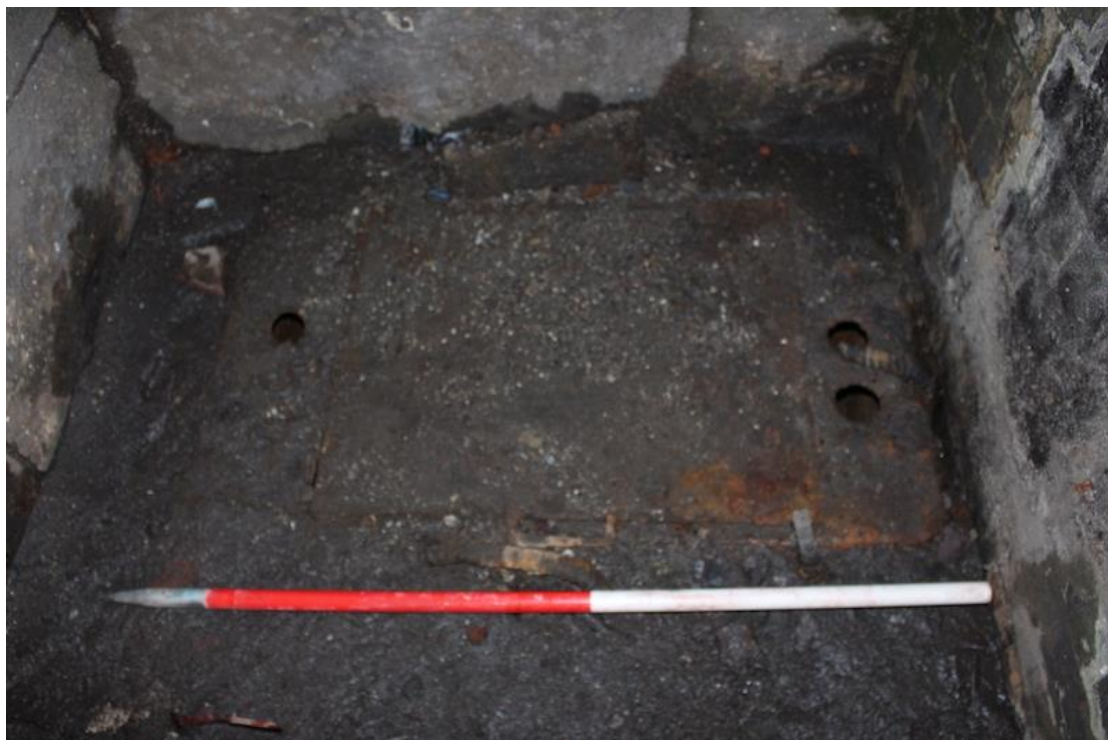
Plate 40. Detail photo showing a steel-lined sump located at the west end of main basement [105].
