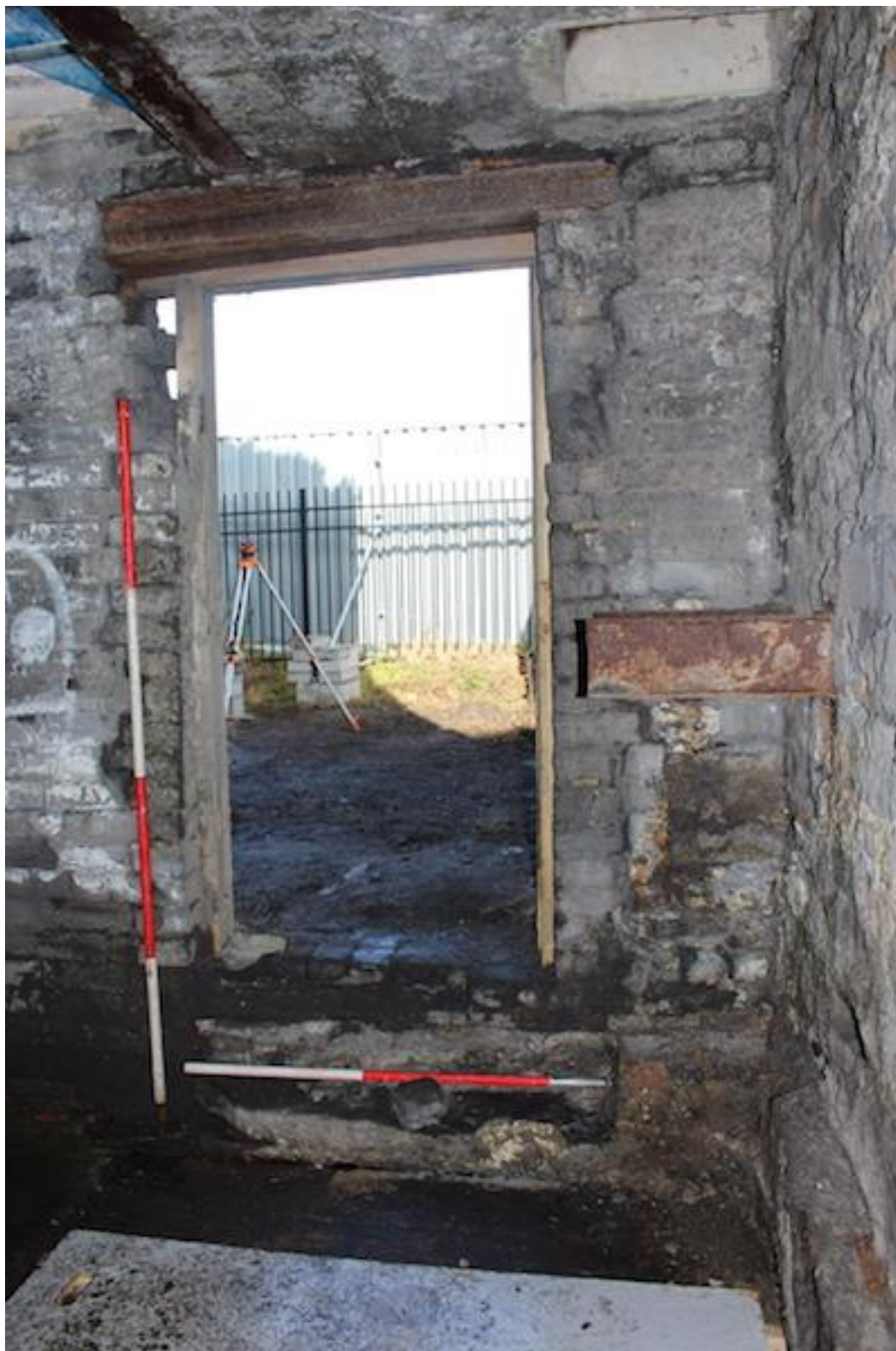
Plate 44. East-facing photo from main basement [105] showing east doorway and the pennant stone threshold stone that acts as the lintel for culvert [104].
