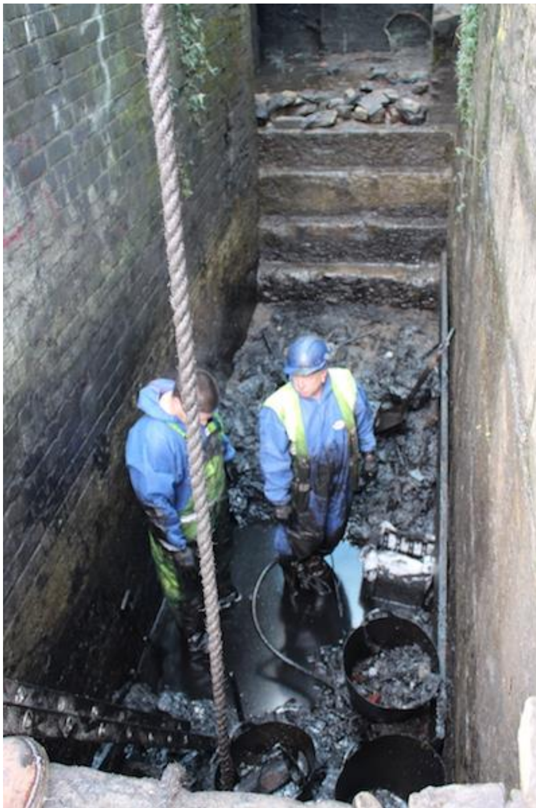
Plate 24. Working shot during excavation of wheel pit [206] showing oil contamination of lower deposit (203).
