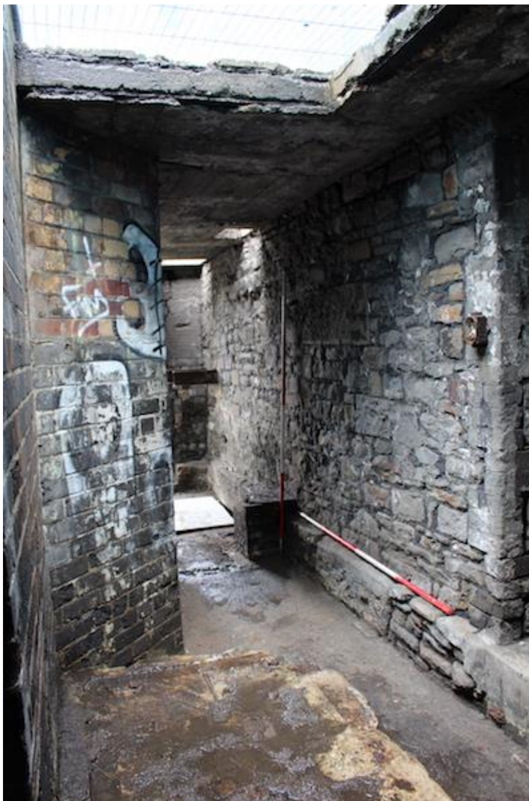
Plate 38. East-facing photo showing main basement [105] showing the south rubble stone wall and ash brick north wall with later red/ yellow brick infill.
