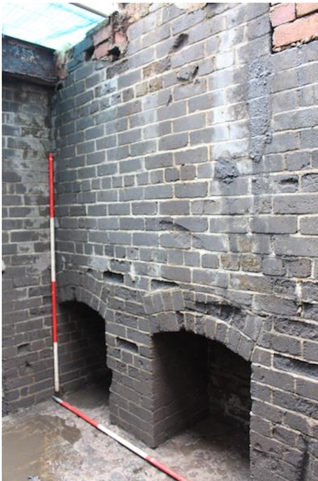
Plate 34. South-facing photo showing two of three brick arched recesses in south wall of inspection platform [207].
