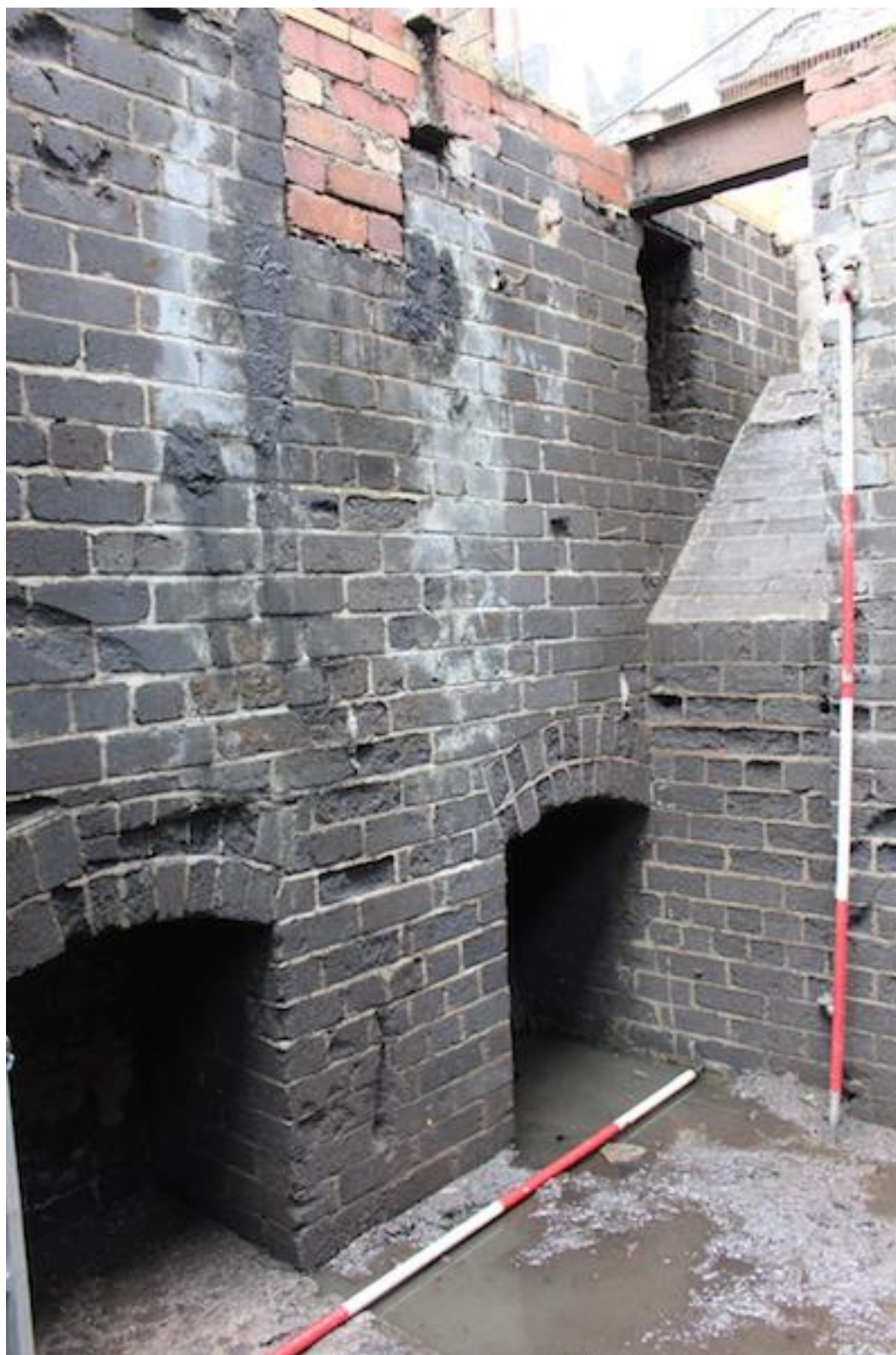
Plate 35. South-facing photo showing two of three brick arched recesses in south wall of inspection platform [207]. Also showing chute from machine floor.
