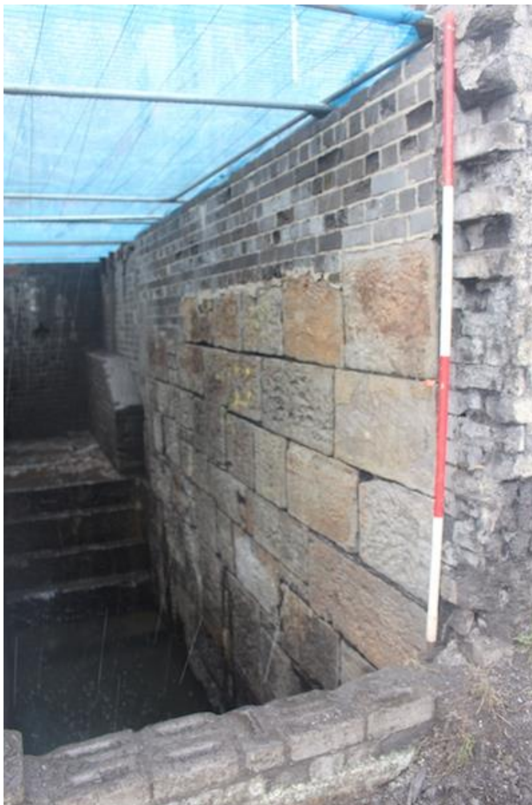
Plate 30. West-facing photo showing pennant stone north wall of wheel pit [206]. The wall is extended up to machine floor level with Vivian ash brick.
