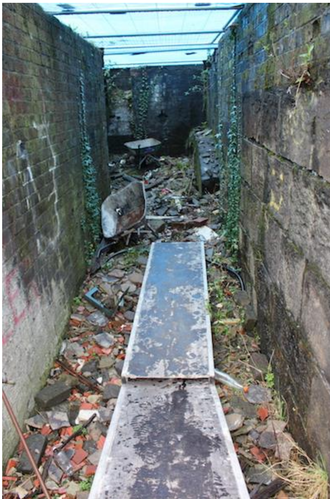
Plate 18. West facing pre-excitation photo showing deposit (201) within wheel pit [206] and inspection platform area [207] situated to the rear.
