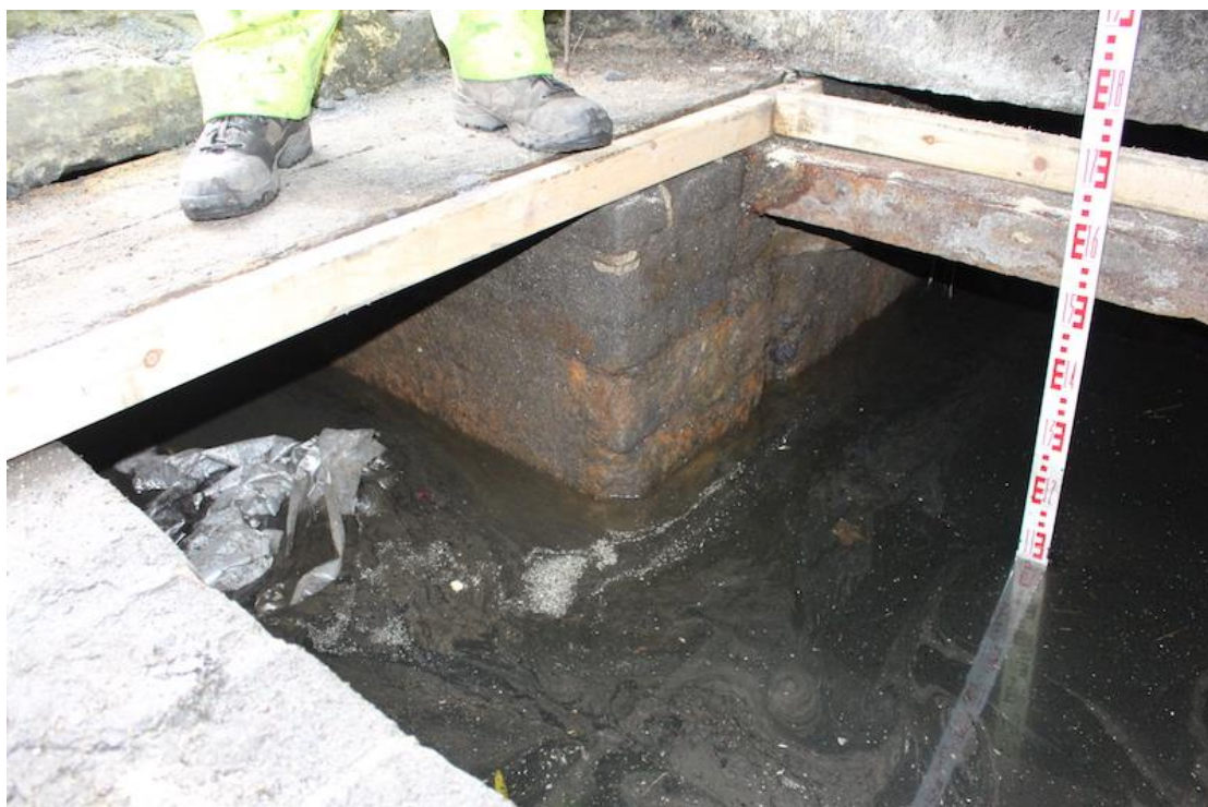
Plate 16. South facing post-excitation photo showing sump [103] to right and culvert [104] running beneath the east doorway. Also shows water ingress.
