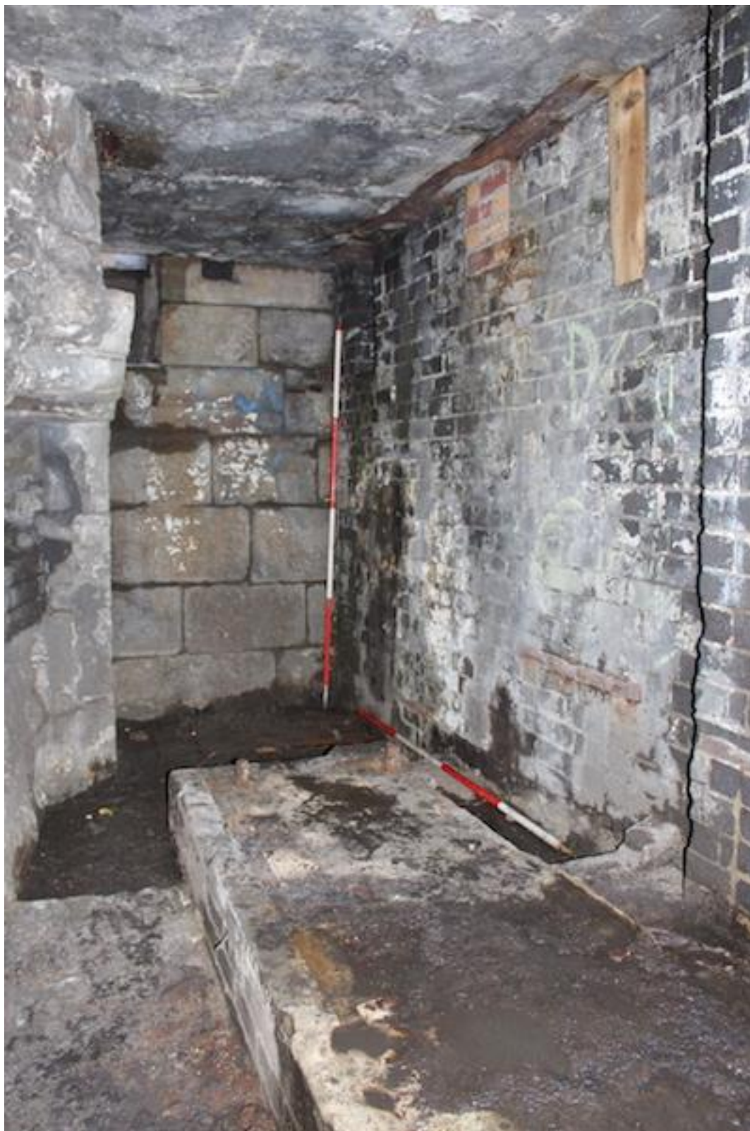
Plate 39. West-facing photo showing the pennant stone west wall of main basement [105] and ash brick north wall with later red/yellow brick infill.
