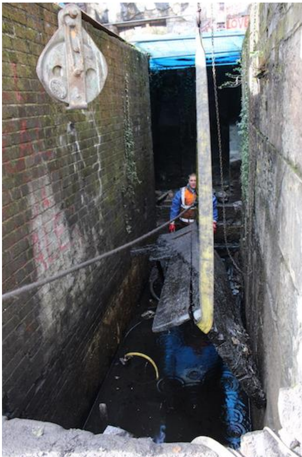
Plate 23. Working shot showing the removal of the timber leaf from wheel pit [206] using a gantry hoist.
