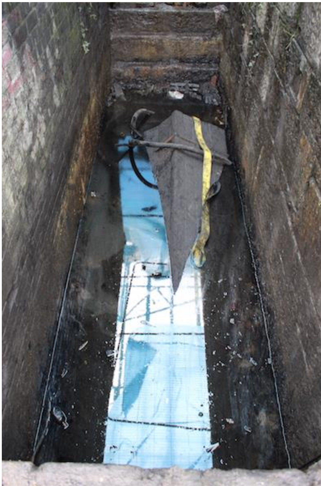
Plate 22. West-facing photo showing timber section of leat within wheel pit [206], prior to removal.
