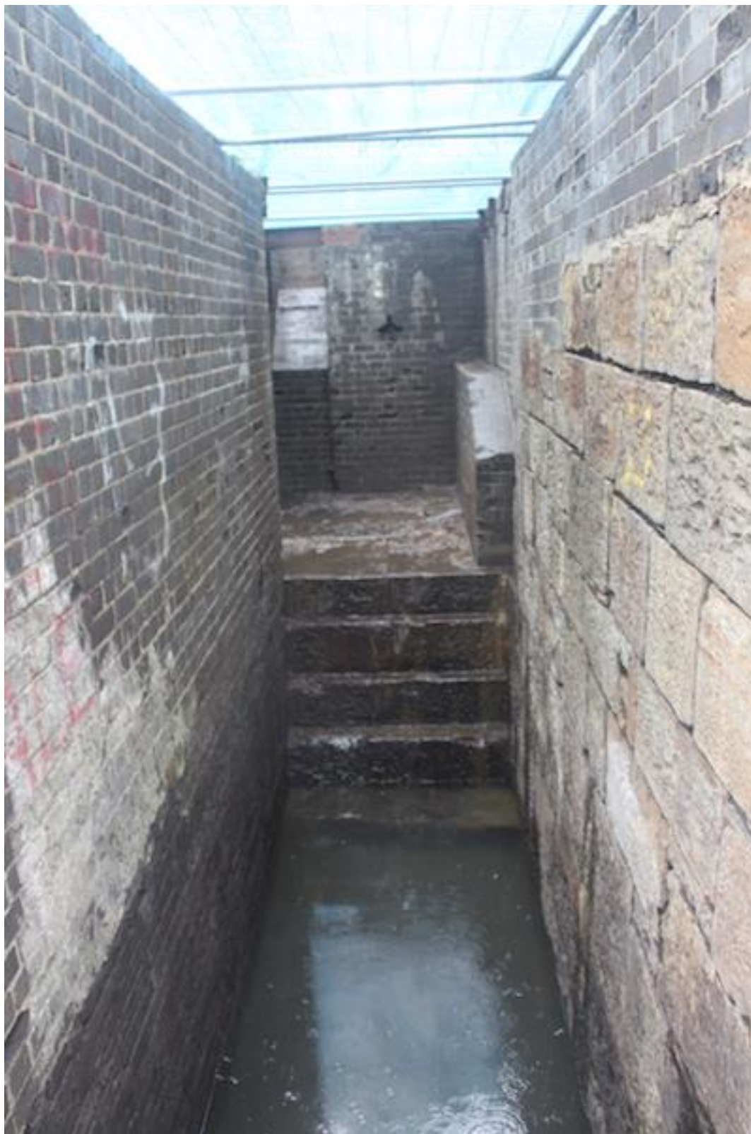
Plate 31. West-facing photo of machine pit showing wheel pit [206] and inspection platform [207] to rear. Also shows steps to the base of the wheel pit.
