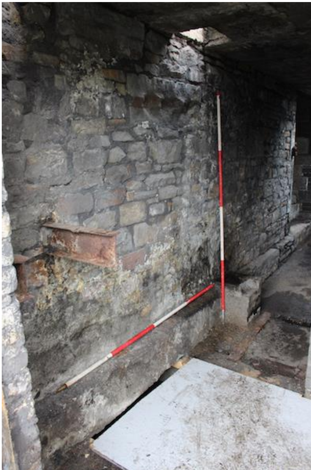
Plate 37. West-facing photo from east doorway showing the south wall of main basement [105]. The pennant stone lintel of sump [103] is visible in the foreground.
