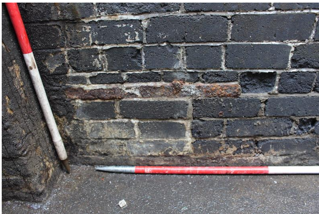
Plate 41. One of a number of blocked inspection hole/ vents. This one is located in stairwell [106].
