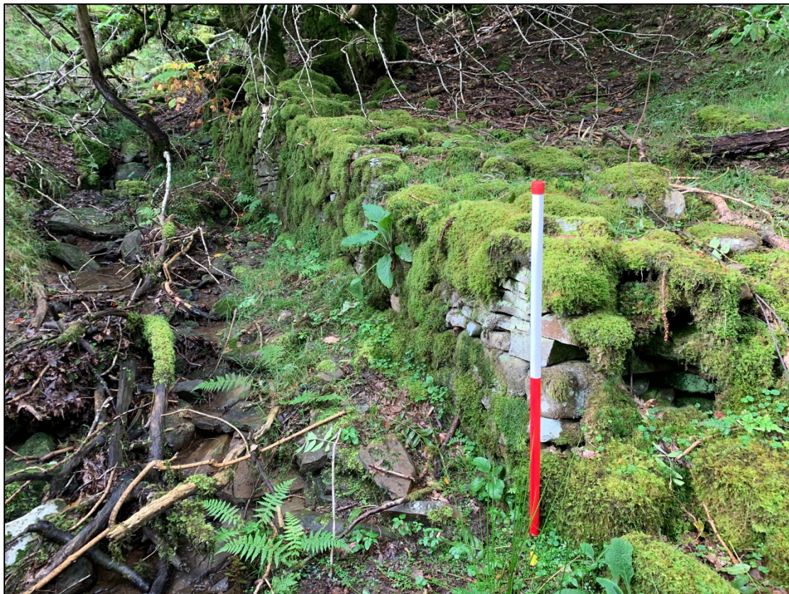
Plate 15. South west/ north east aligned wall lining the northern bank of Nant Graig within Waunwyllt Colliery.
