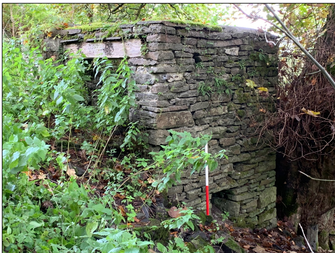
Plate 32. North west facing detail of probable Drystone Toilet (GGAT03747m) in association with Old Level (BPW02) close to Pen-y-lan Farm (GGAT03746m).
