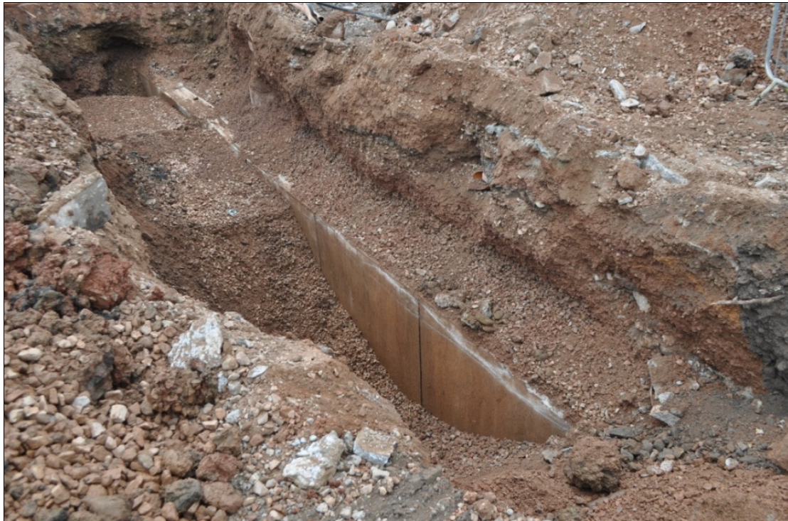
Plate 3 - Trench 2 revealing north wall of the encased Bute Feeder Canal [204]. (looking southeast)
