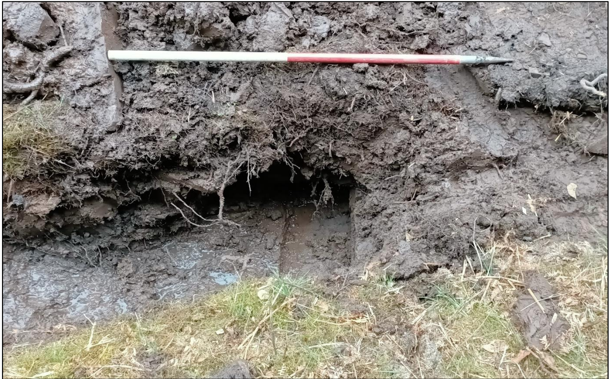
Plate 9. Inflow head [040] of Bryn Melyn Culvert I (ID30 in Appendix IV)
