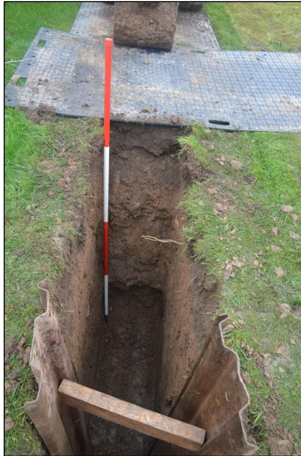
Fig. 6 View from the south-east of the trenching in the garden to the rear of No. 19. Photo CPAT 4730-034
