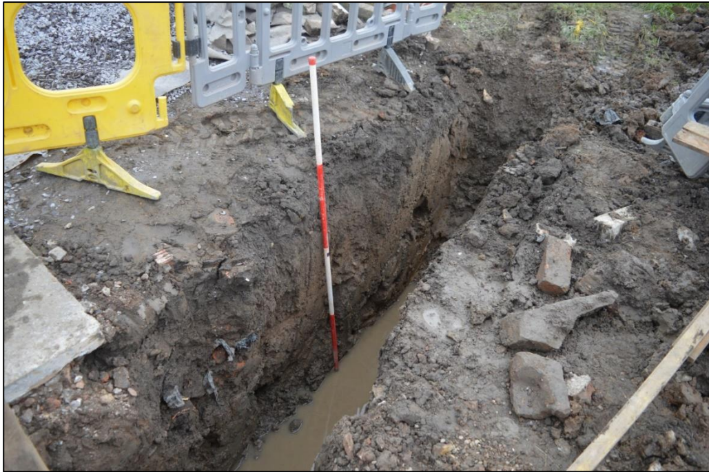
Fig. 9 View from the west of the trenching in the garden to the rear of No. 13 Photo CPAT 4730-54
