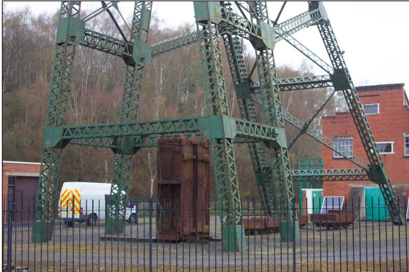
Plate 32: Base of No.2 Winding Gear with Colliery Tip in Background, Plas Grono Road, Rhostyllen, Wrexham LL14 4EG - from the east
