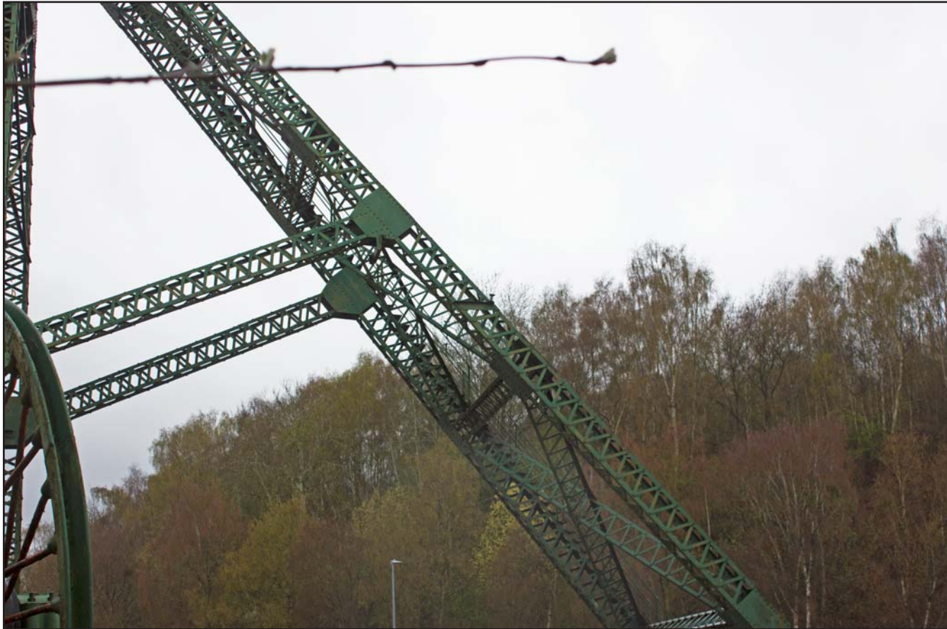
Plate 37: No.2 Winding Gear leg, with Colliery Tip in Background, Plas Grono Road, Rhostyllen, Wrexham LL14 4EG - from the east-northeast
