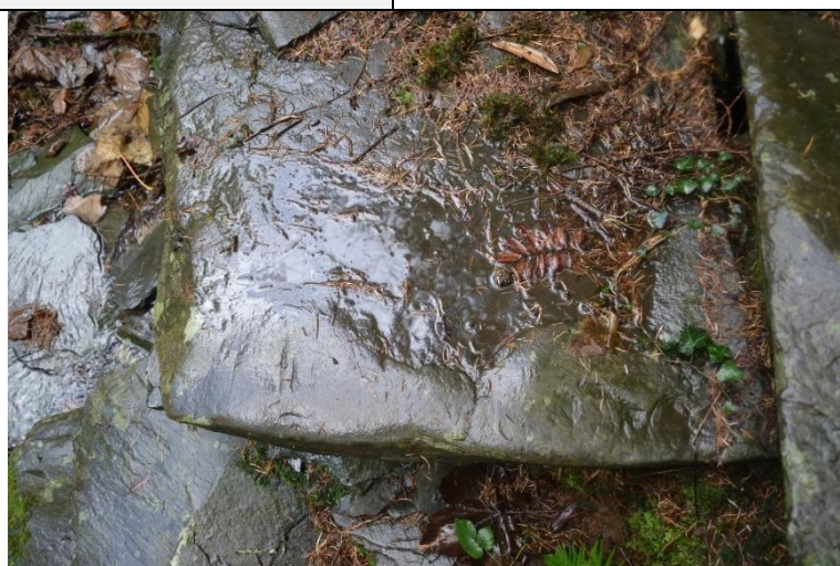
Wear on the edge of the bridge possibly from hobnail boots, from ENE (archive reference: G2754_0029)
