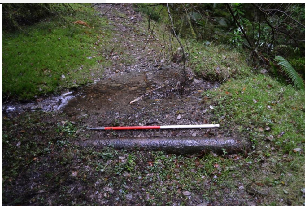
Cast iron water pipe crossing the forest track from SE (archive reference: G2754_0004)
