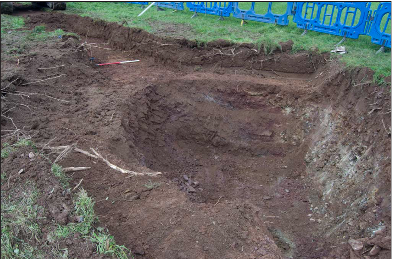
Plate 04: View of chamber area excavated to depth and pipe trench with topsoil and subsoil removed; scale: 1x1m (archive reference: G2751_016).
