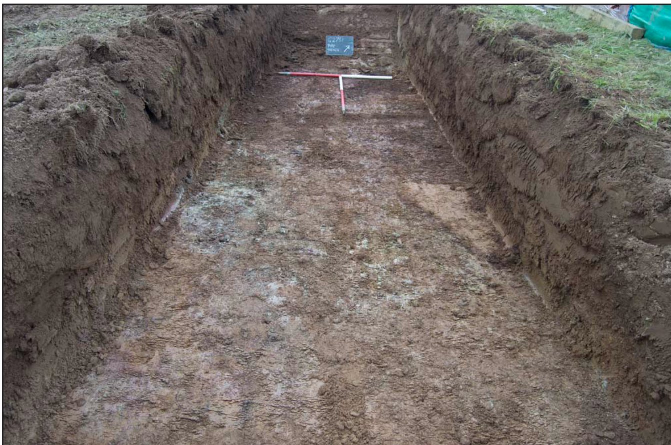
Plate 08: View from the southeast of pipe trench showing the glacial clay at the north west end of the field; scale: 2x1m (archive reference: G2557_27).
