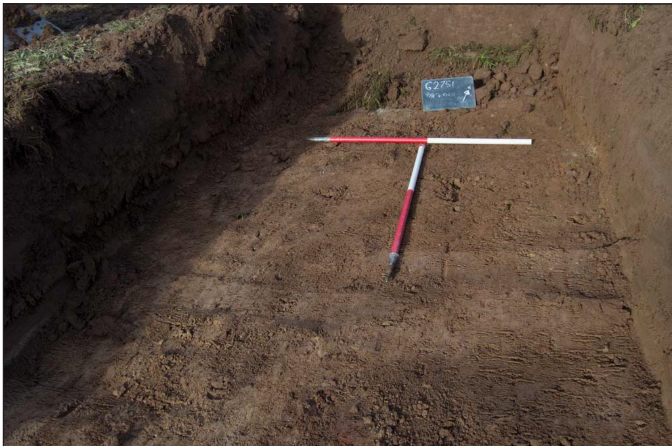
Plate 07: View from the southeast of pipe trench with topsoil and subsoil removed; scale: 2 x 1m (archive reference: G2557_21).
