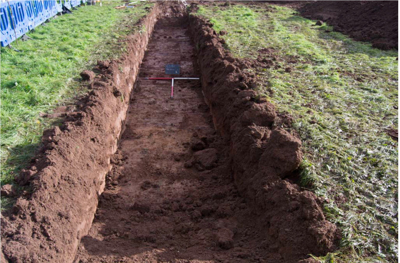
Plate 05: View of the pipe trench from the northwest; scale: 2 x1m (archive reference: G2751_17).
