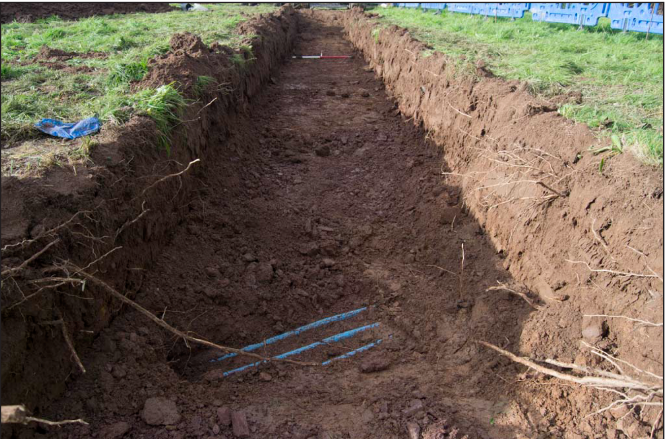
Plate 06: View of the pipe trench from the southeast showing water pipes crossing the trench; scale: 2x1m (archive reference: G2751_19).
