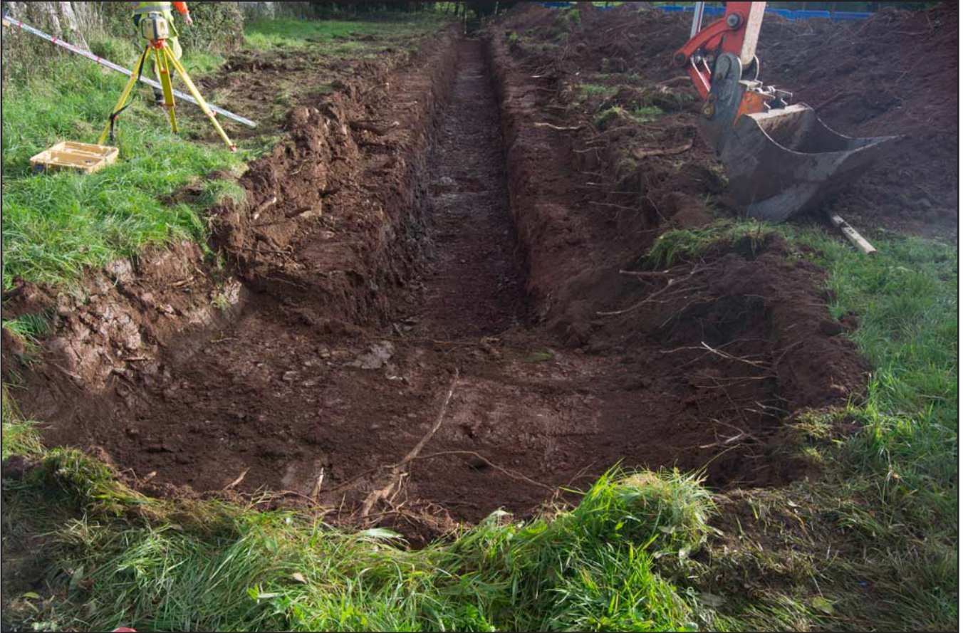
Plate 03: View of the pipe trench and chamber area with topsoil and subsoil removed to the glacial clay; (archive reference: G2751_014).
