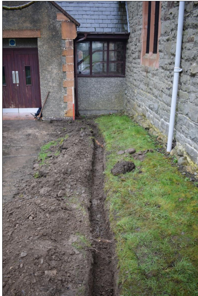
Fig. 3 The trench between the new oil tank and the church hall, viewed from the south-west. Photo CPAT 4752-0005
