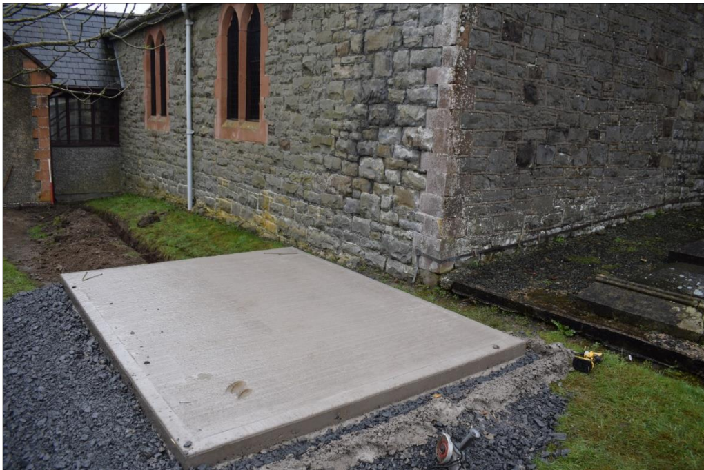
Fig. 2 The concrete base for the new oil tank, viewed from the west. Photo CPAT 4752-0005
