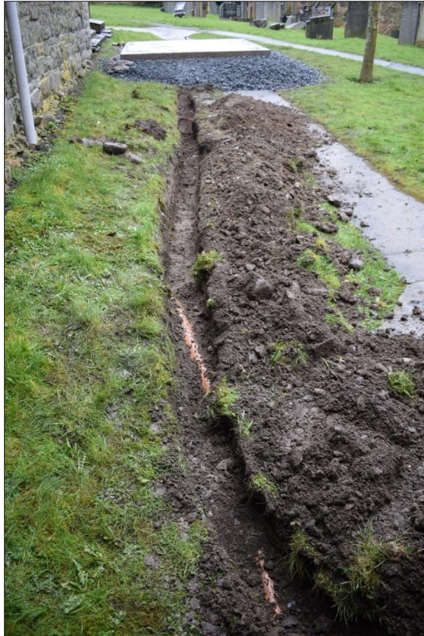
Fig. 4 trench between the new oil tank and the church hall, viewed from the north-east. Photo CPAT 4752-0006
