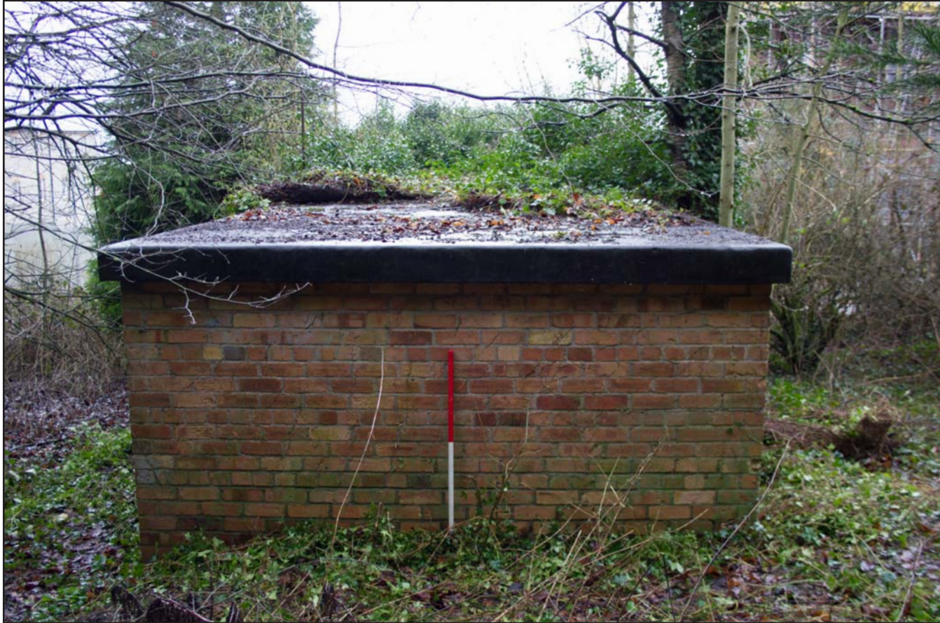
Plate 03: Air Raid Shelter 1 southwest facing external elevation, from the southwest. Scale 1.0m.
