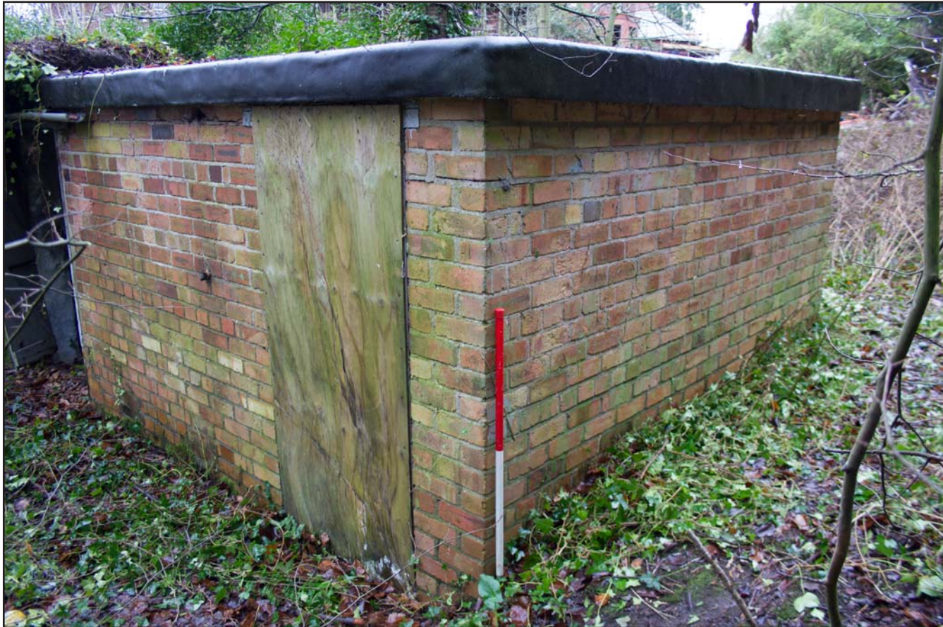
Plate 04: Air Raid Shelter 1 southwest and northwest (SW end) facing external elevations, from the west. Scale 1.0m.
