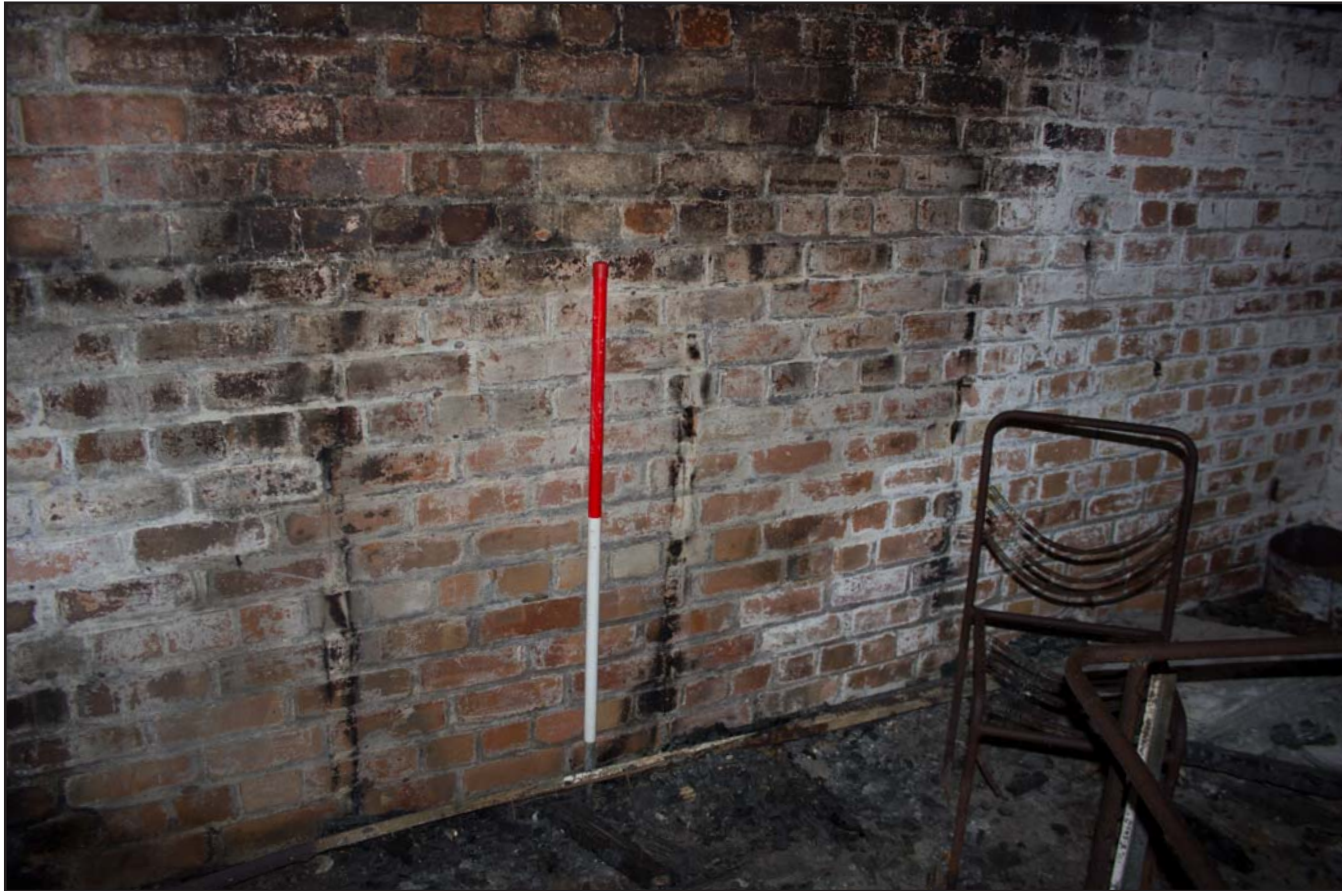
Plate 20: Air Raid Shelter 1 Main Room showing wall timber marks, from the south. Scale 1.0m.
