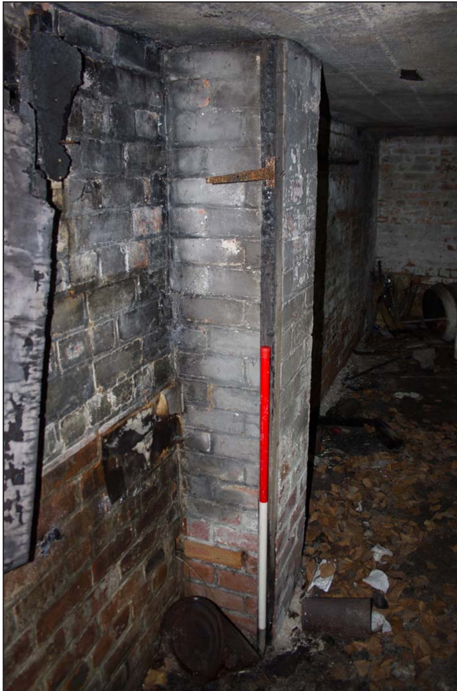
Plate 17: Air Raid Shelter 1 Main Room showing hinged timber post, from the north. Scale 1.0m.
