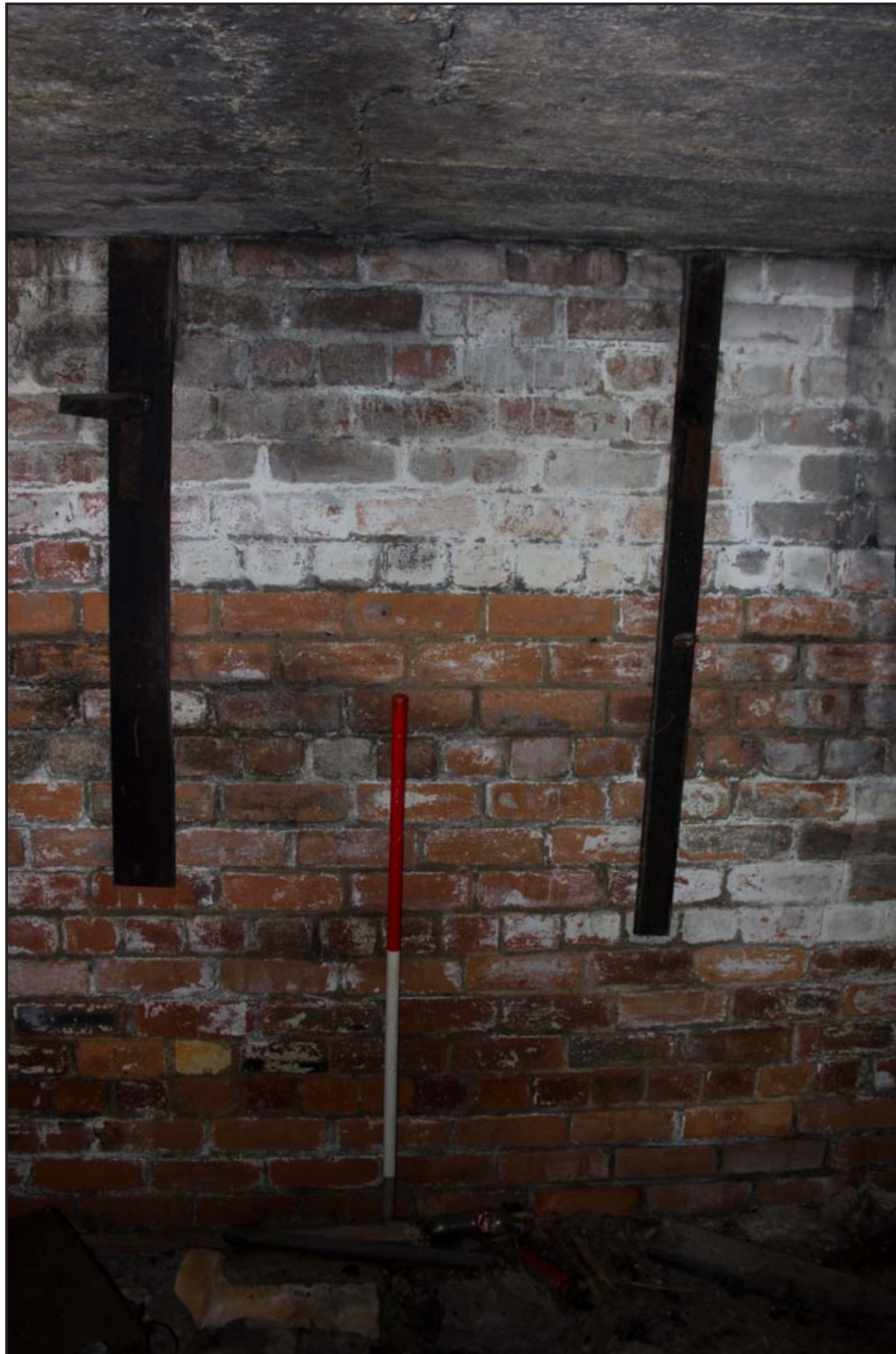
Plate 15: Air Raid Shelter 1 Main Room showing wall brackets, from the northwest. Scale 1.0m.
