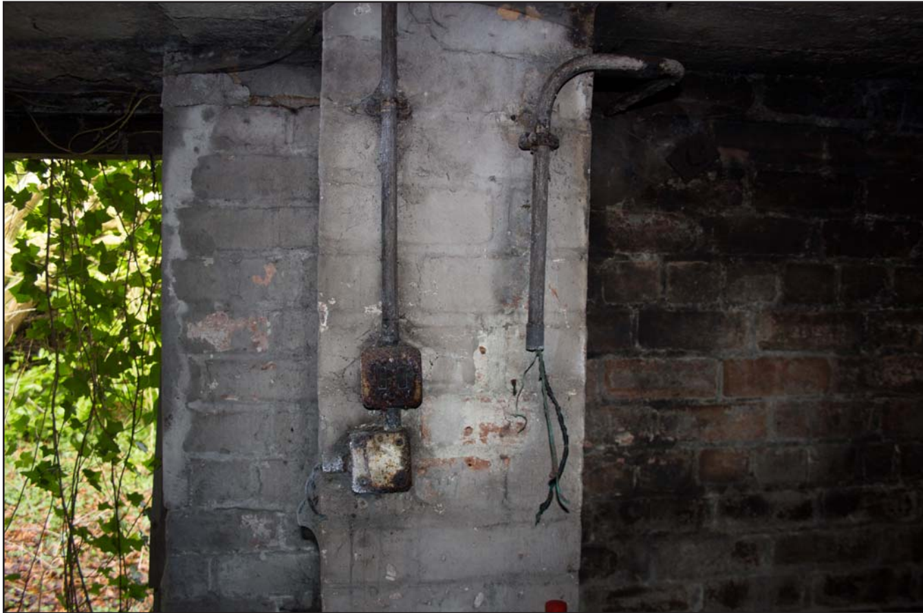
Plate 19: Air Raid Shelter 1 Main Room showing electrical light switches, from the southeast.
