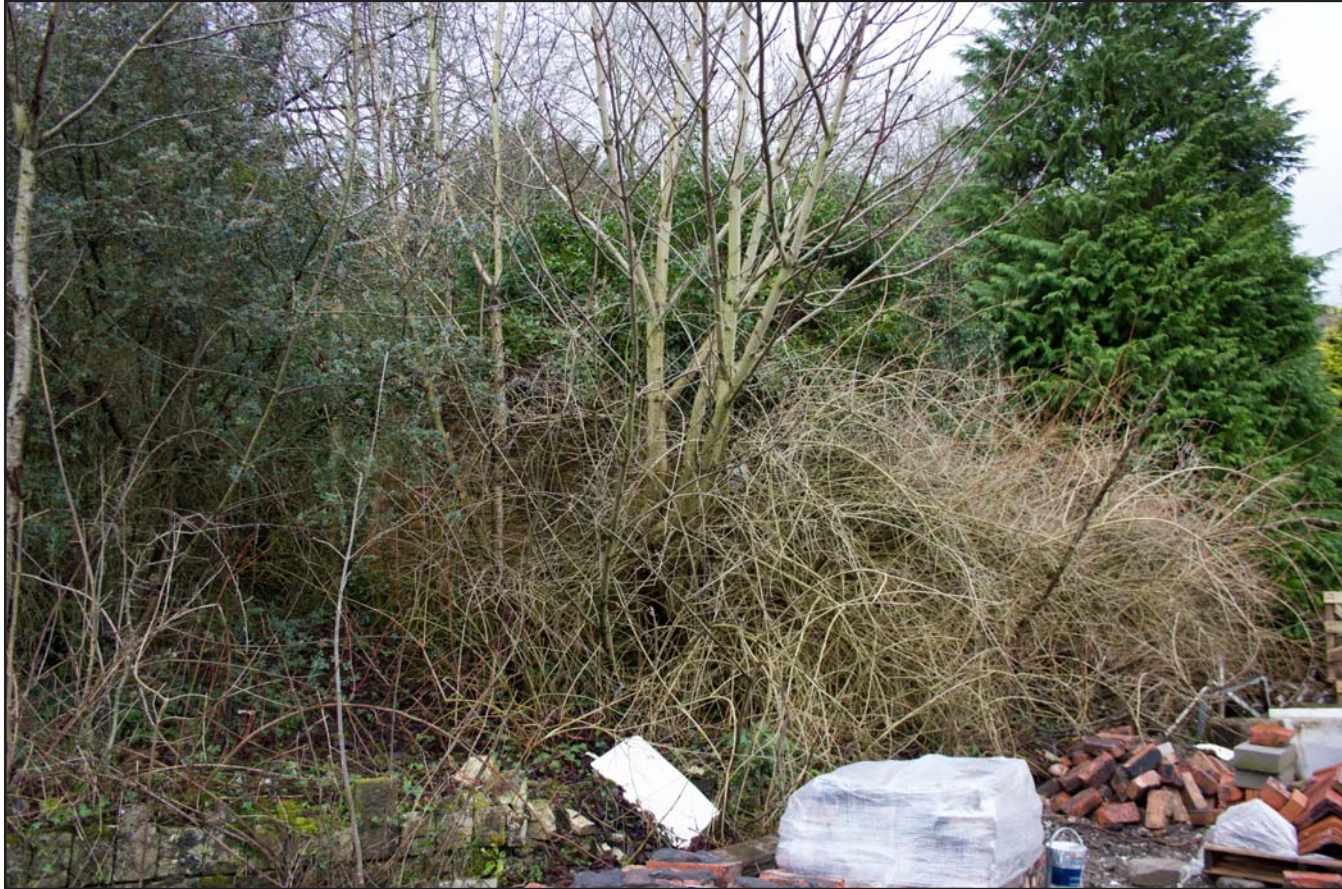
Plate 09: Air Raid Shelter 1 northeast facing external elevation (hidden behind vegetation), from the east.
