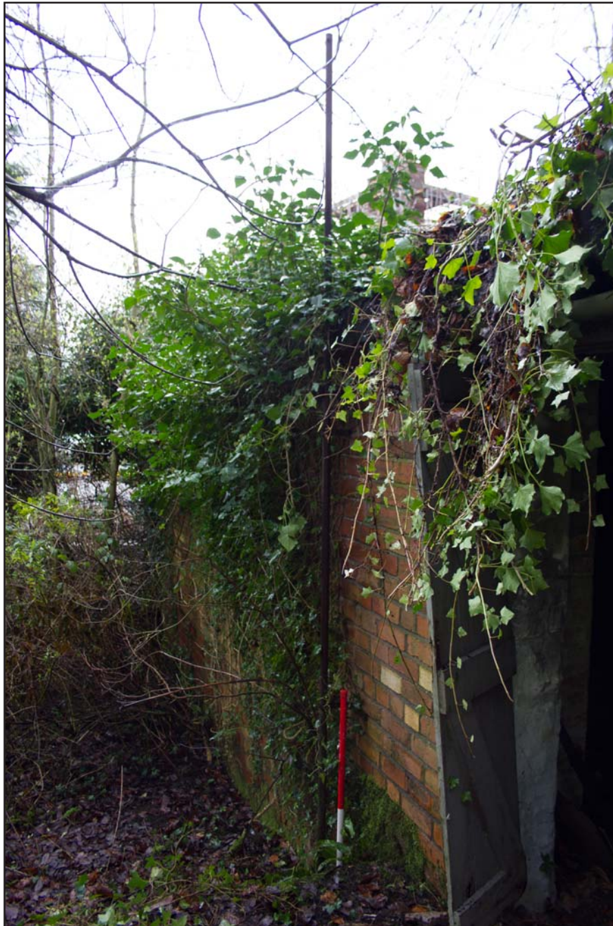
Plate 08: Air Raid Shelter 1 northwest facing external elevation showing electrical connection, from the west. Scale 1.0m.
