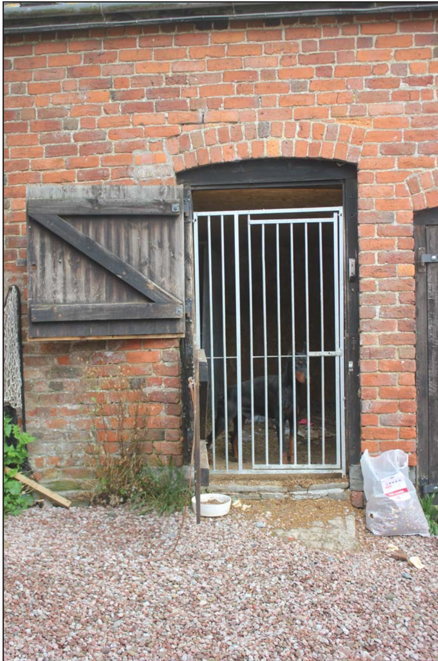
Plate 11: Southern elevation, left door of the outbuilding at The Birches, Rhos-Y-Meirch, Knighton, Powys - from the south - 2.00m scale
