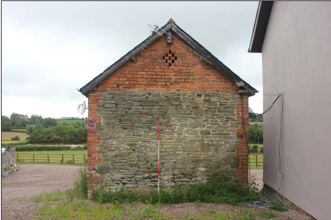
Plate 09: Western elevation of the outbuilding at The Birches, Rhos-Y-Meirch, Knighton, Powys - from the west - 2.00m scale
