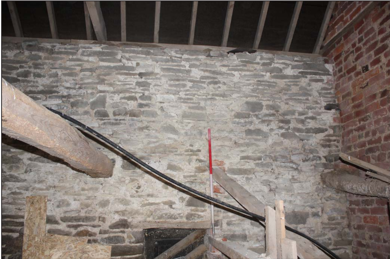
Plate 22: Northern elevation, of the eastern internal room of the outbuilding at The Birches, Rhos-Y-Meirch, Knighton, Powys - from the south - 1.00m scale
