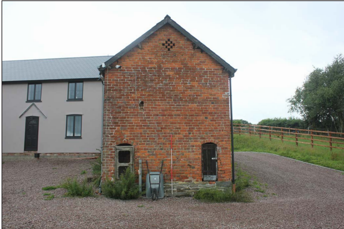
Plate 05: Eastern elevation of the outbuilding at The Birches, Rhos-Y-Meirch, Knighton, Powys - from the east - 2.00m scale
