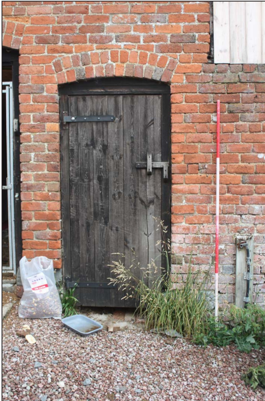
Plate 12: Southern elevation, central door of the outbuilding at The Birches, Rhos-Y-Meirch, Knighton, Powys - from the south - 2.00m scale
