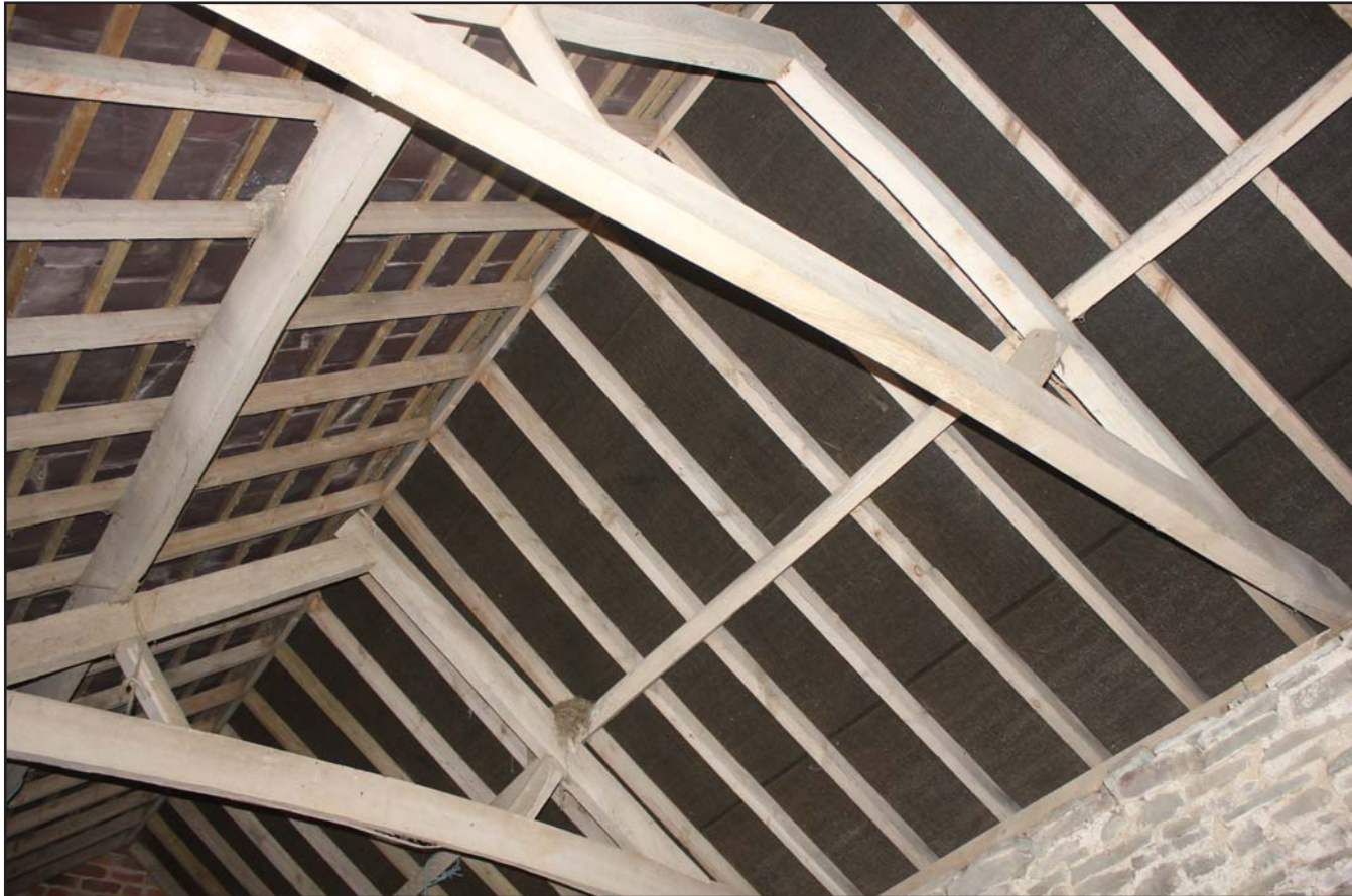
Plate 27: Sawn timber roof trusses in the outbuilding at The Birches, Rhos-Y-Meirch, Knighton, Powys - from the southeast - no scale
