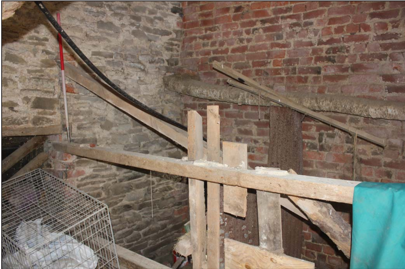
Plate 24: Pigsty construction and inserted window in the eastern room of the outbuilding at The Birches, Rhos-Y-Meirch, Knighton, Powys - from the southwest - no scale
