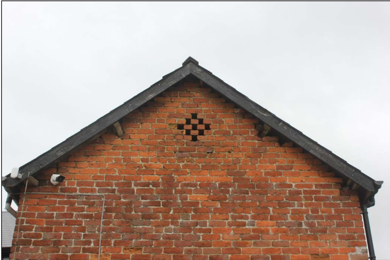
Plate 16: Eastern elevation, diaper/diamond shaped ventilation embrasure on the outbuilding at The Birches, Rhos-Y-Meirch, Knighton, Powys - from the east - no scale
