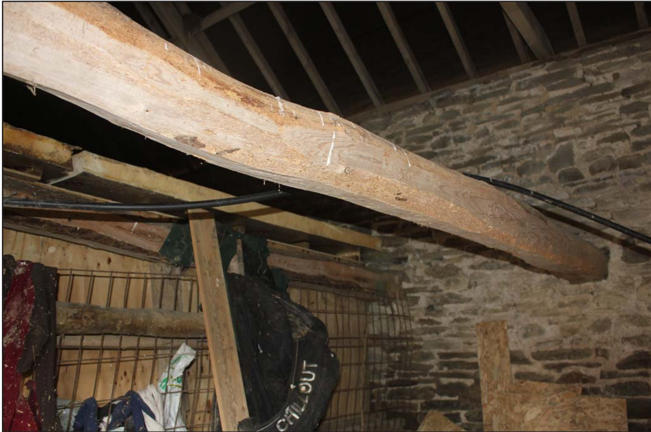
Plate 25: Handhewn beams in the eastern room of the outbuilding at The Birches, Rhos-Y-Meirch, Knighton, Powys - from the southeast - no scale
