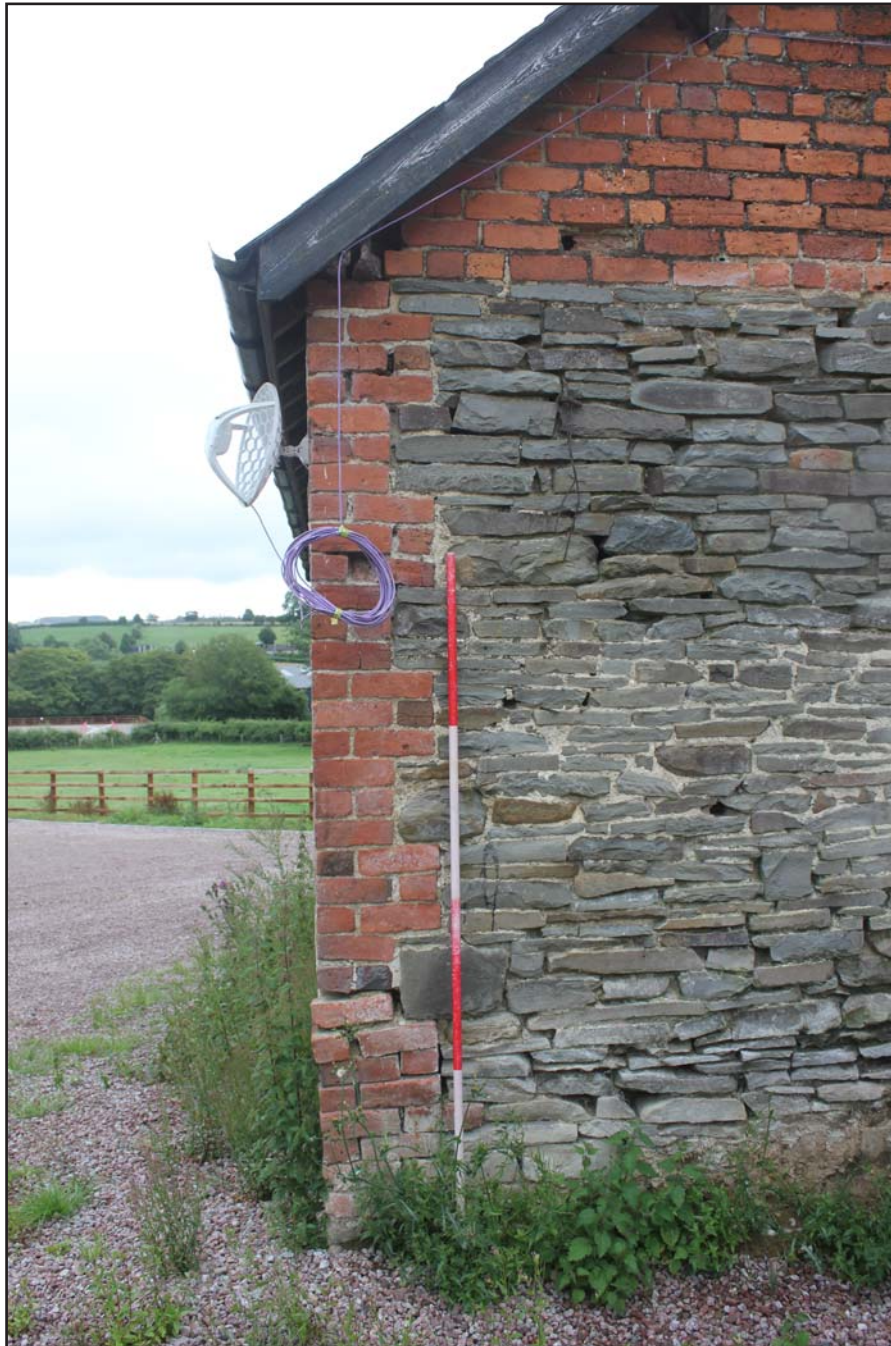
Plate 18: Brick quoin detail on western elevation of the outbuilding at The Birches, Rhos-Y-Meirch, Knighton, Powys - from the west - 2.00m scale
