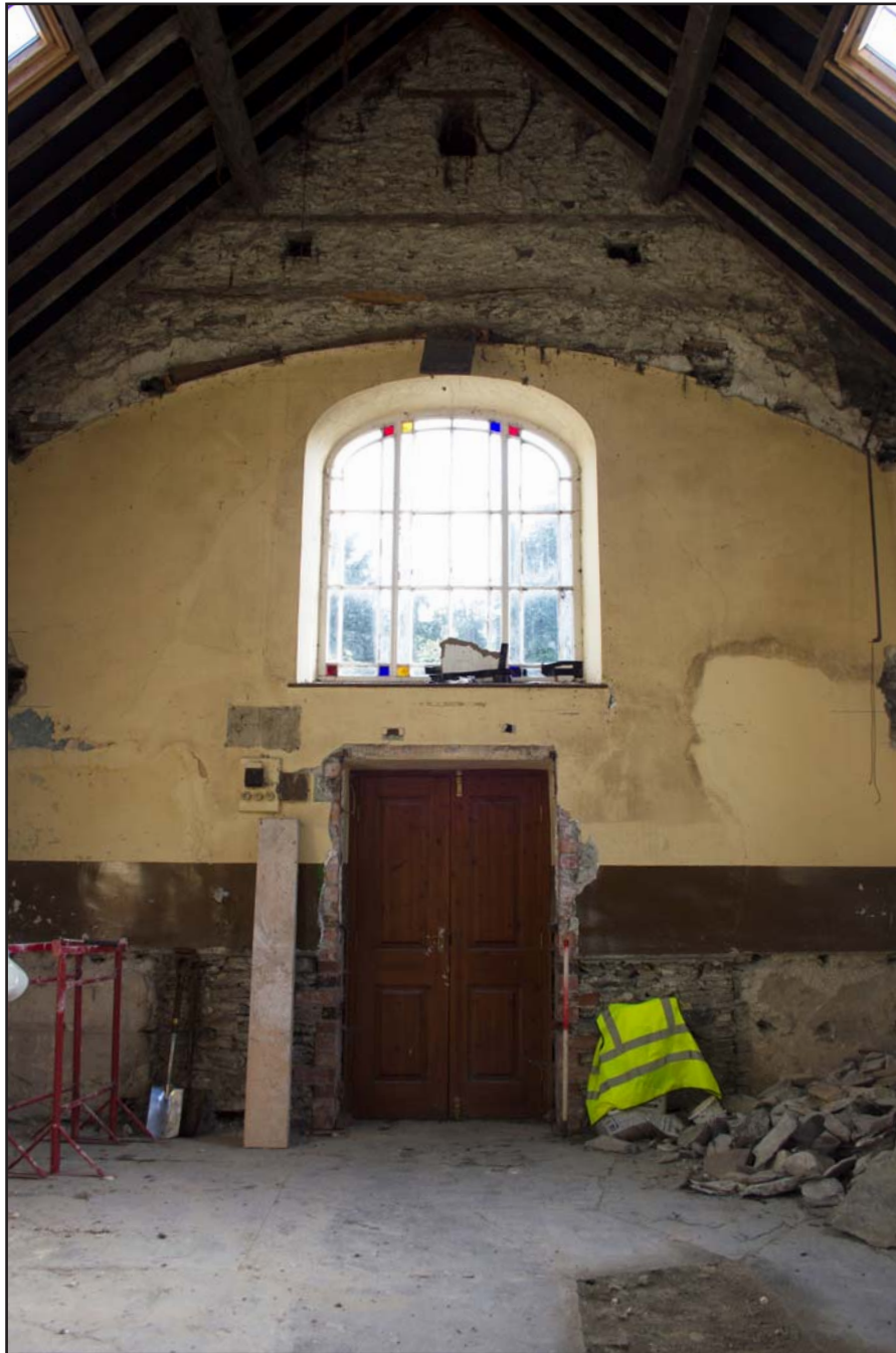
Plate 16: Framed shot of northeast internal elevation of Capel Sion, Pontfadog, Llangollen - from the southwest - 1.00m scale
