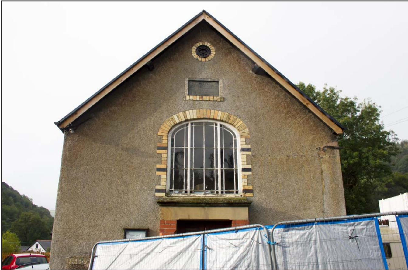
Plate 09: Framed shot of northeast external elevation of Capel Sion, Pontfadog, Llangollen - from the northeast - 1.00m scale
