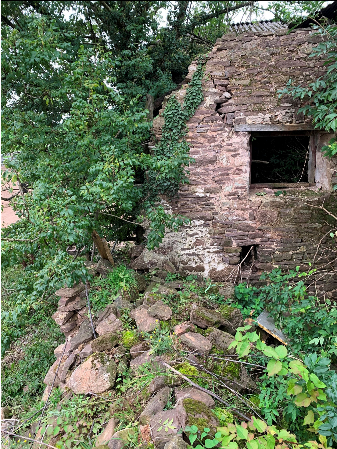
Plate 55: LLN2020_0055 - A view of the rubble marking the line of the southern gable end of the barn. This view seems to suggest that the gable wall which collapsed was not the original gable wall but was a later insert which did not bond with the lateral walls. Looking west.
