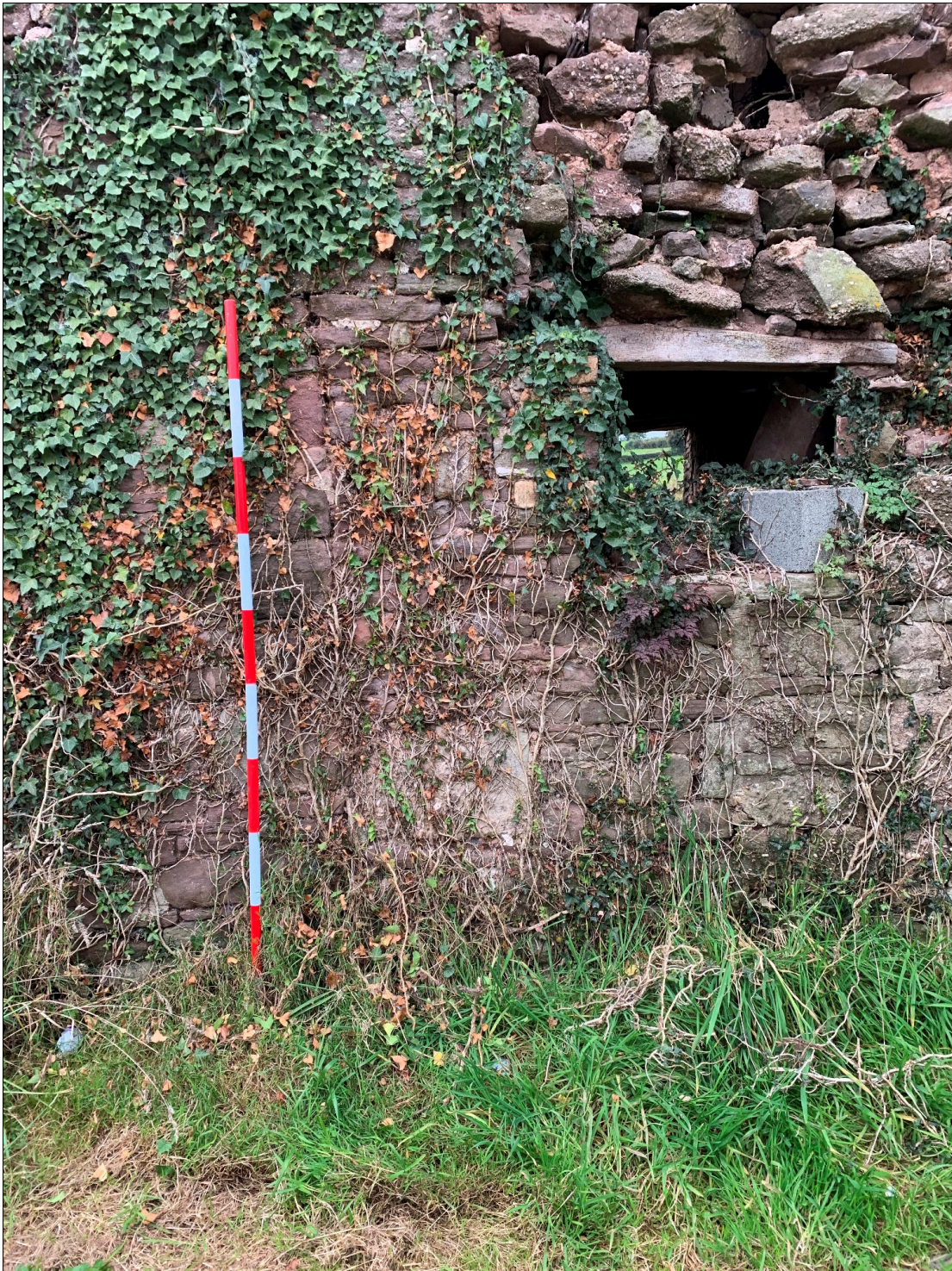
Plate 89: LLN2020_0089 - A view of the blocked-up doorway in the northern end of the eastern wall. It was blocked up before the window seen here was cut through the wall and part of the blocked-up door. Looking east.
