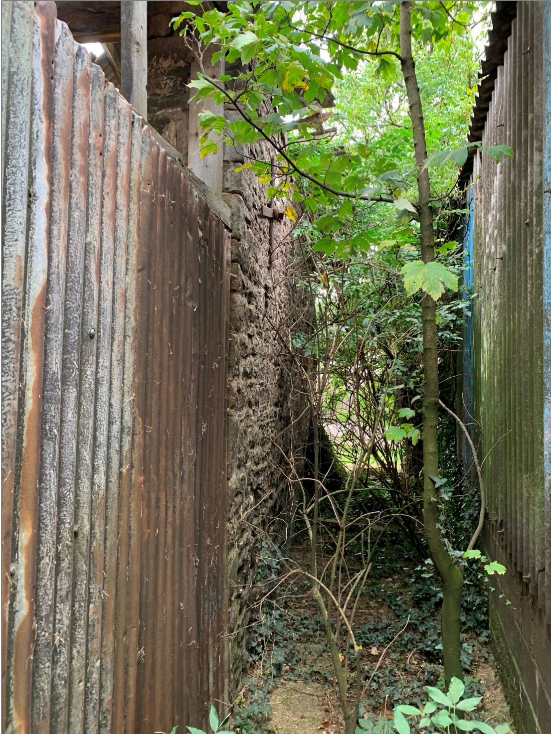
Plate 68: LLN2020_0068 - A view towards the southern end of the western wall of the barn. Note the steel tie bracket on the wall to the left of centre. Looking south.
