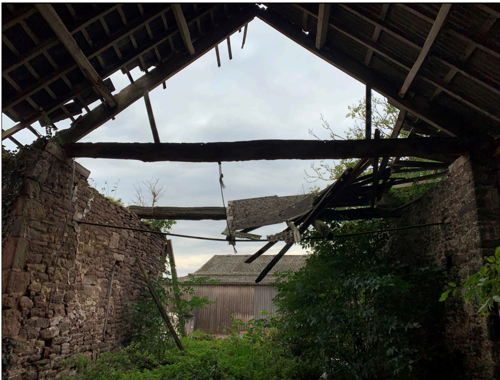
Plate 41: LLN2020_0041 - A view inside the barn, showing the collapsed southern end of the roof and an original roof truss still in place. Looking south.
