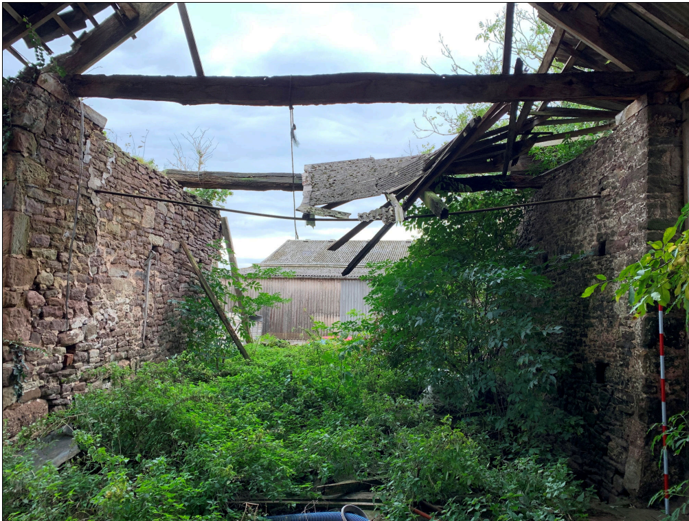
Plate 40: LLN2020_0040 - A view inside the barn, showing the collapsed southern end of the roof and the gap left by the collapse of the southern gable wall. Looking south.
