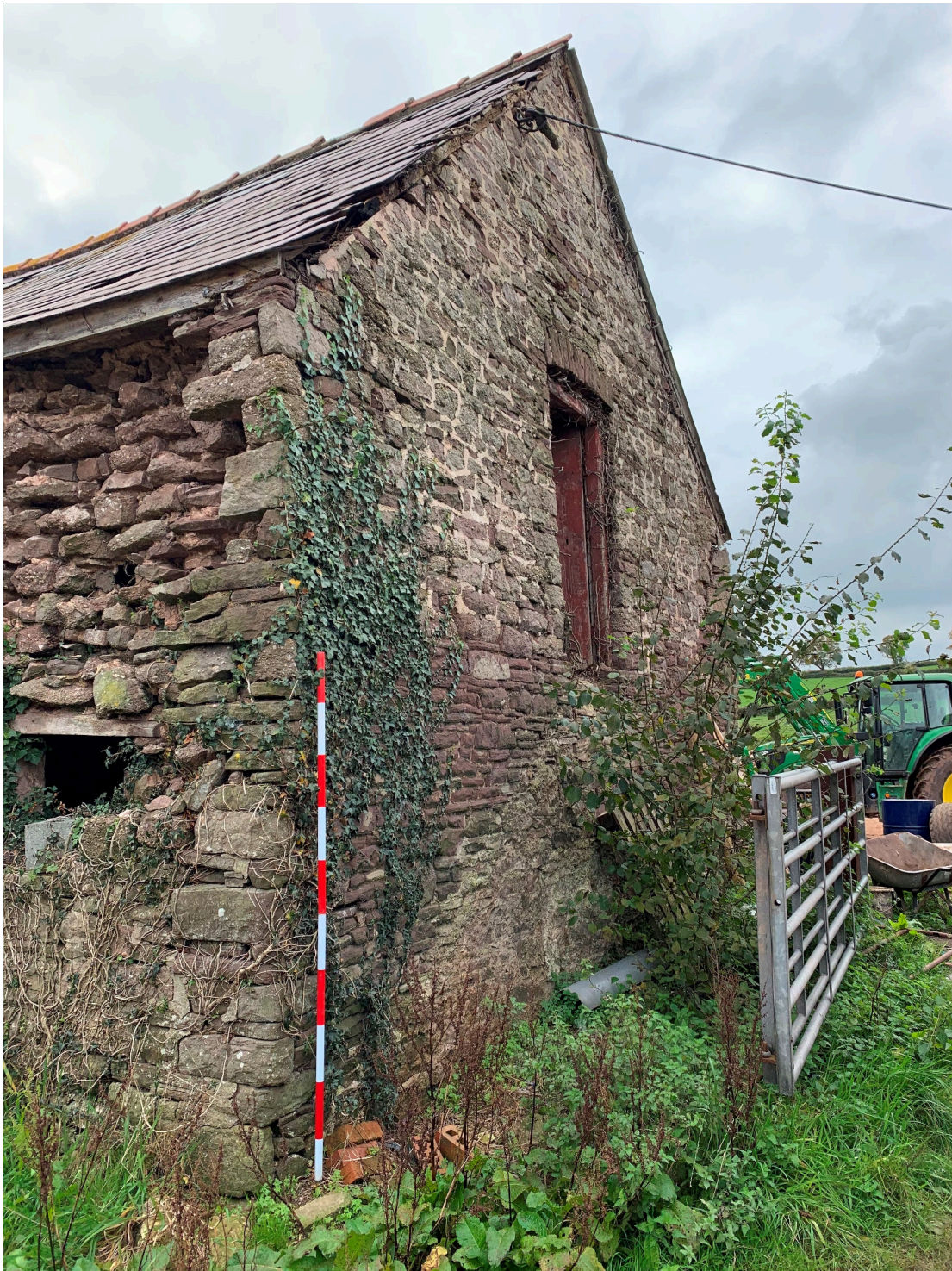
Plate 21: LLN2020_0021 - A view of the northern gable end of the cow house. The stair to the doorway in the upper floor has been removed but the scar of the structure is still visible on the wall. Looking west-southwest.
