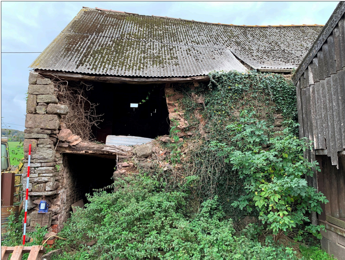
Plate 27: LLN2020_0027 - A view of the western elevation of the cow house, showing the collapsed section of wall in the upper floor above the doorway. The reveal of a window is seen to the right of the missing section. A blocked up central doorway is present on the ground floor, behind the vegetation to the right of centre. The northern end of the modern agricultural shed built alongside the barn and cow house is seen to the right of the image. Looking east.
