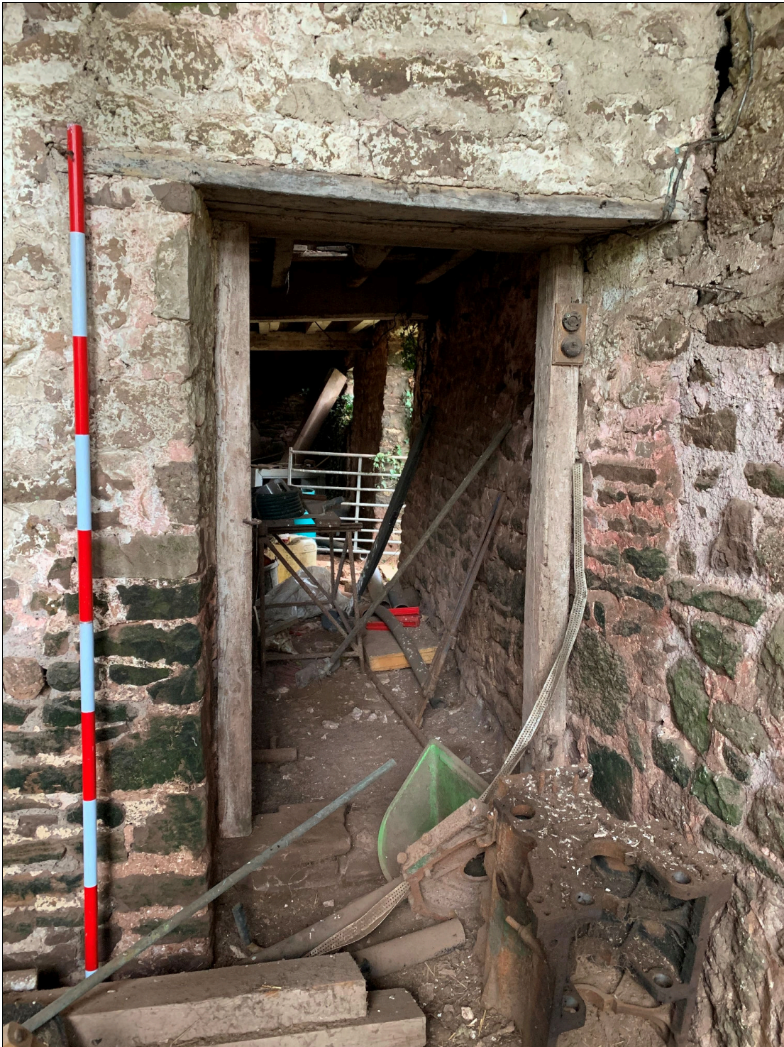
Plate 61: LLN2020_0061 - A view into the cow house through the door linking it with the barn. Looking north-northeast.
