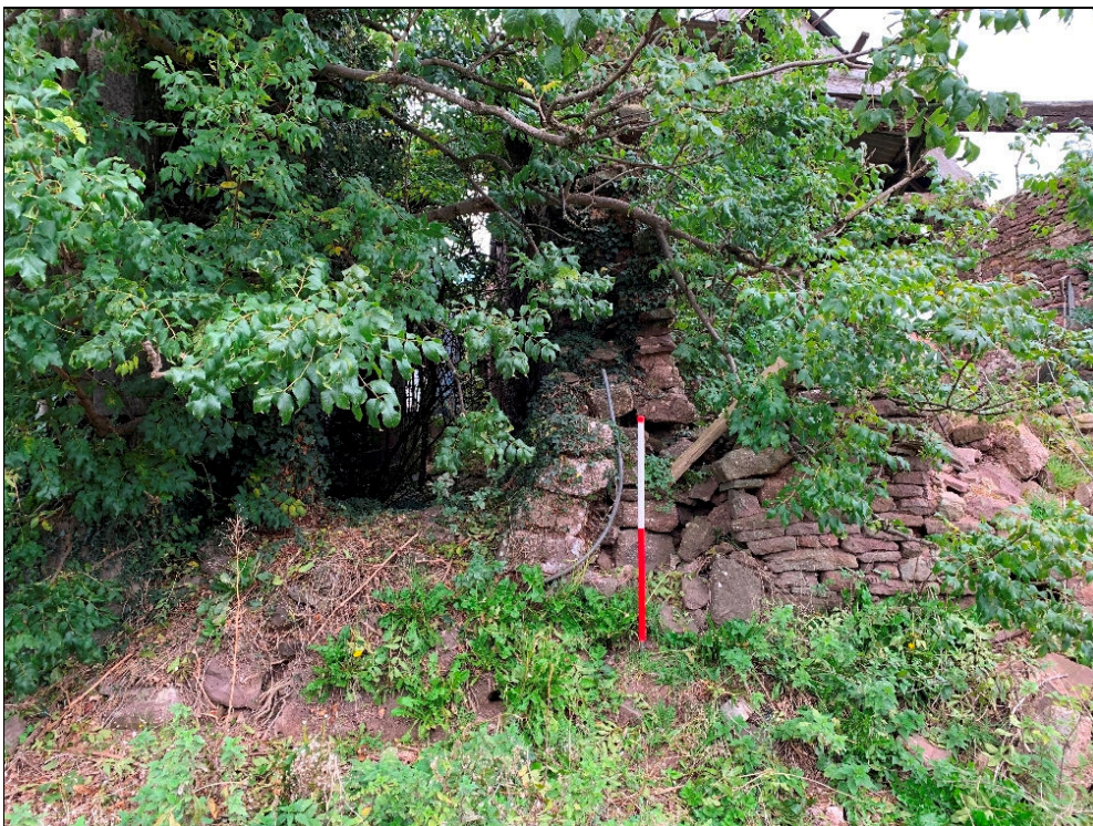
Plate 4: LLN2020_004 - A view of the southwestern corner of the barn, which seems to show that there was a rip joint where the western and southern walls met, suggesting that the original southern gable wall had been replaced at some time. Looking north.
