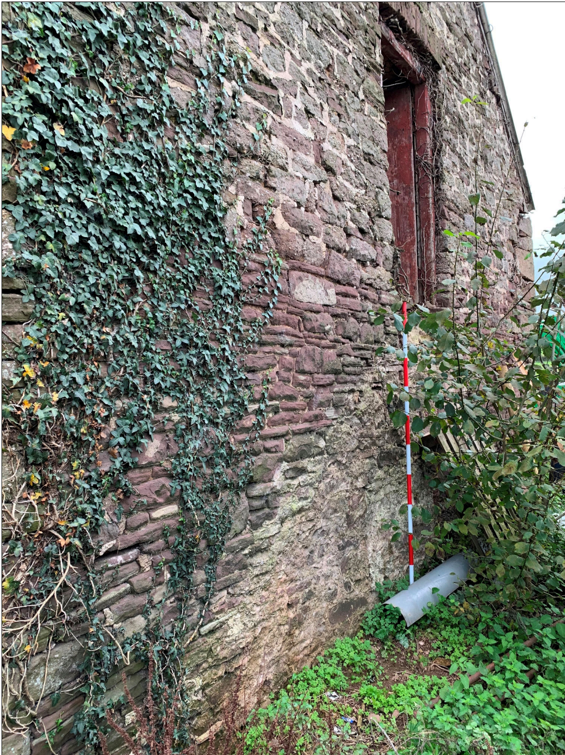
Plate 24: LLN2020_0024 - A view of the northern gable end of the cow house. The stair to the doorway in the upper floor has been removed but the scar of the structure is still visible on the wall. Looking southwest.
