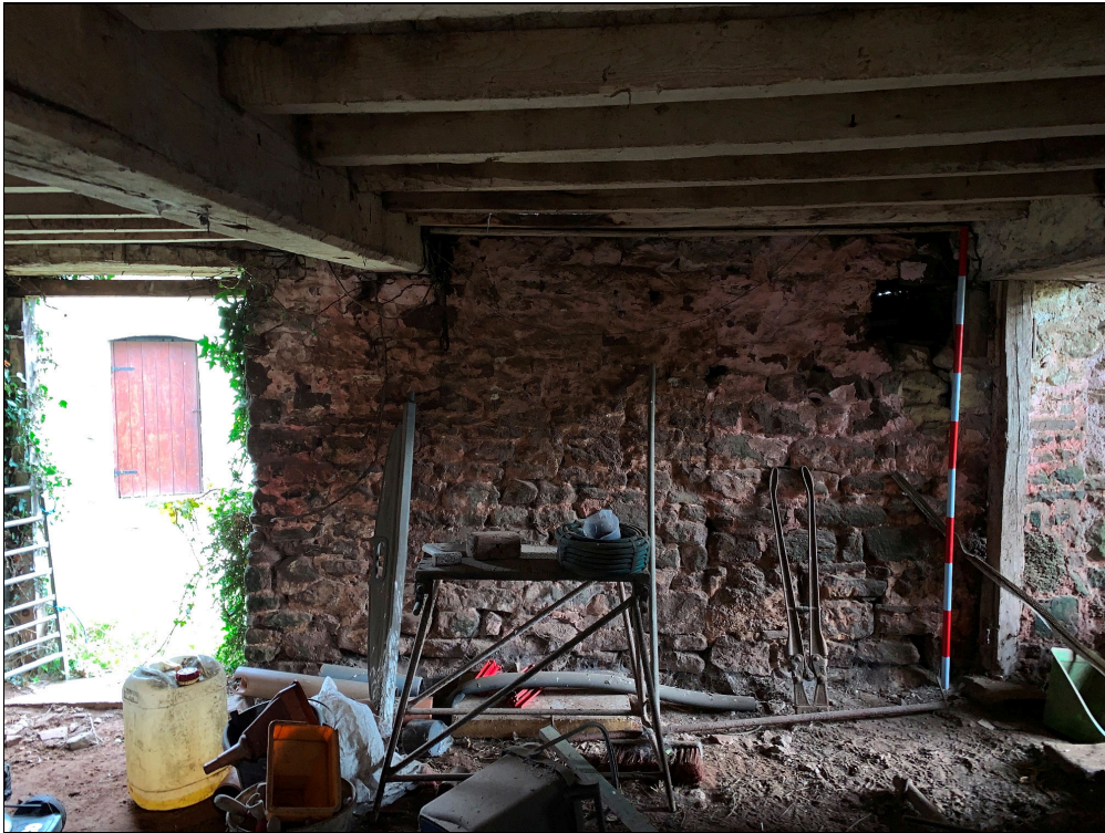
Plate 82: LLN2020_0082 - A view of the eastern wall inside the cow house. The blocked-up central door can be seen. Note the beams and joists of the floor above. Looking east.
