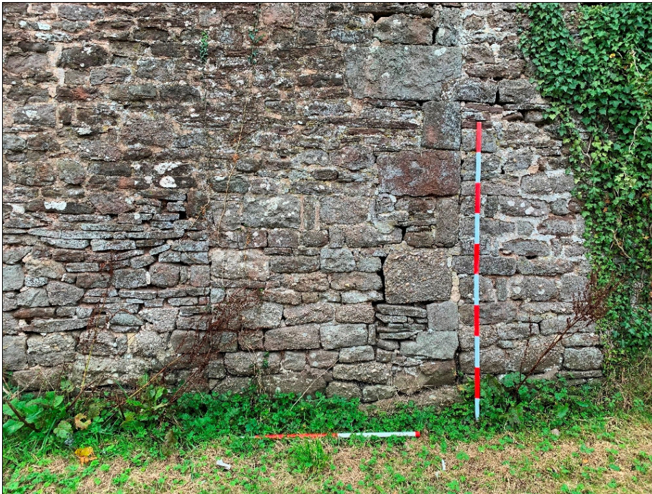
Plate 17: LLN2020_0017 - Another view of the blocked-up doorway at the northern end of the eastern wall of the barn. Looking west.
