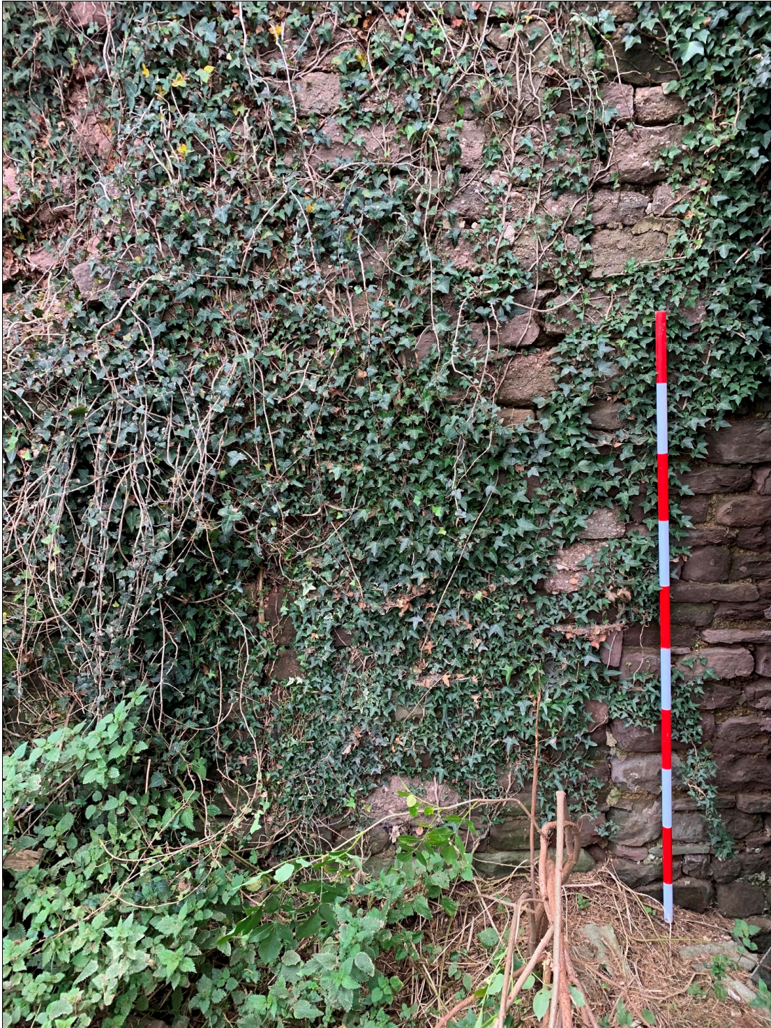
Plate 90: LLN2020_0090 - A view of a the blocked-up central doorway through the western wall of the cow house, seen through the ivy outside the building. Looking east.
