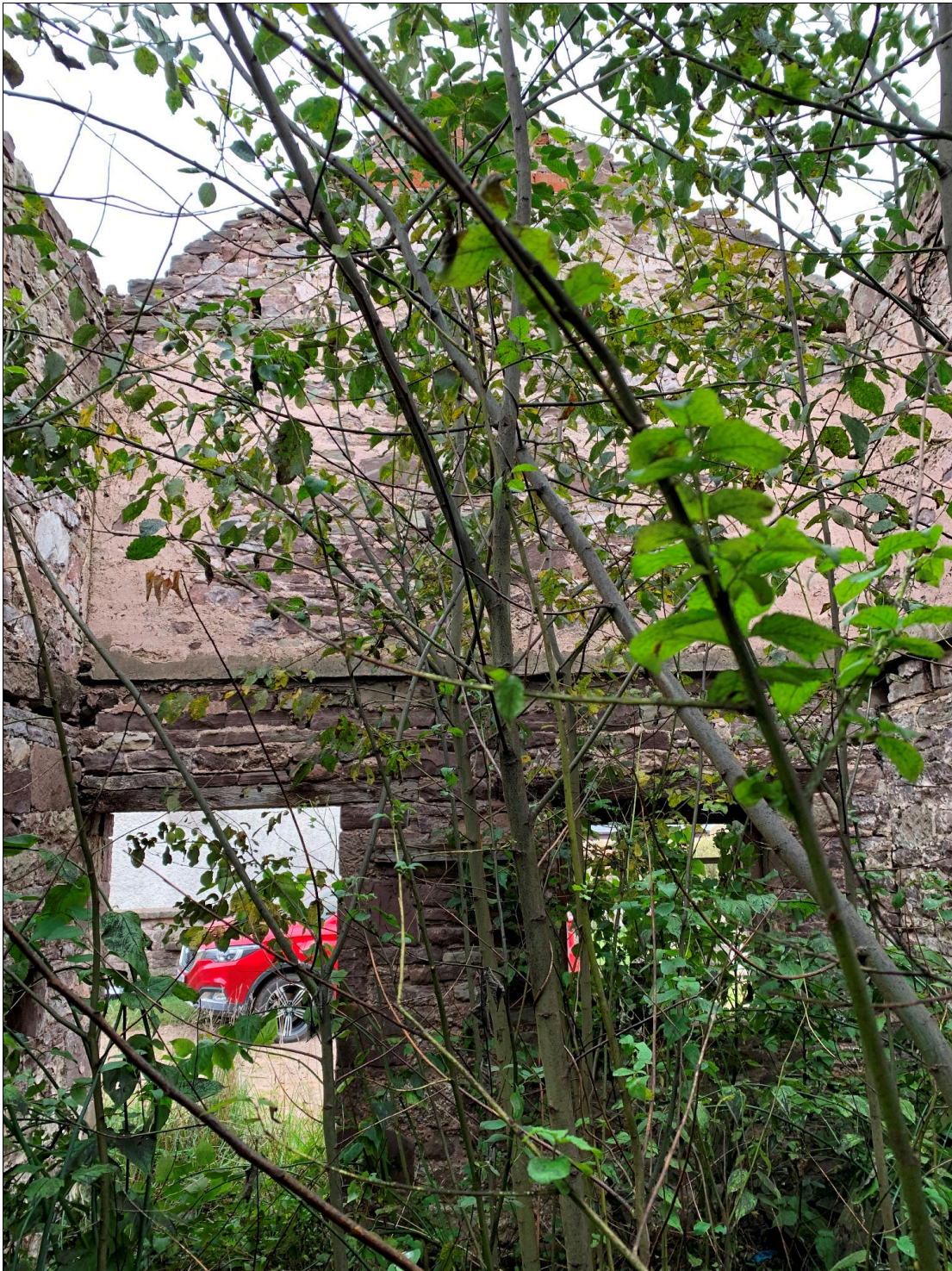
Plate 32: LLN2020_0032 - A view of the inside of the eastern gable wall of the eastern annexe. Looking east.
