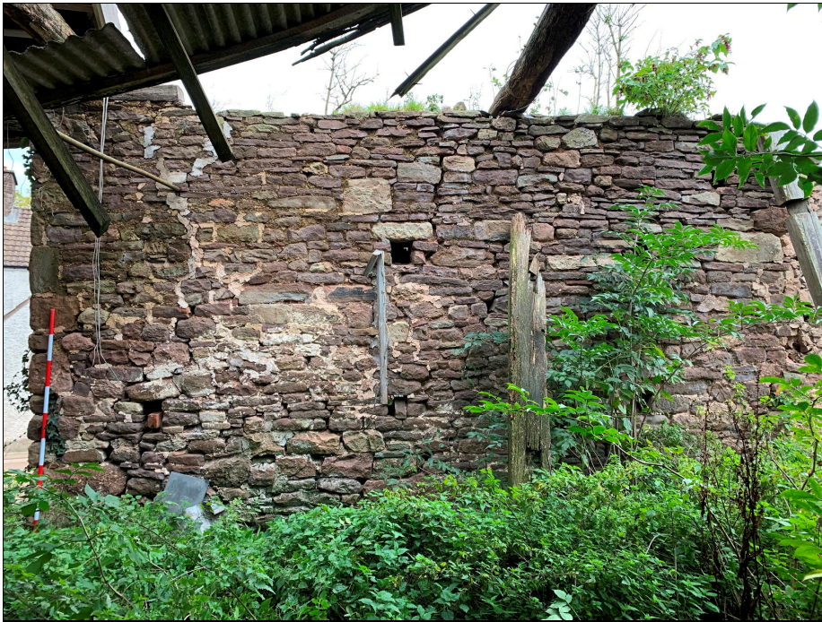
Plate 45: LLN2020_0045 - A view of the eastern wall inside the barn, showing the ventilation holes, some of which have been blocked in the past. Looking east.
