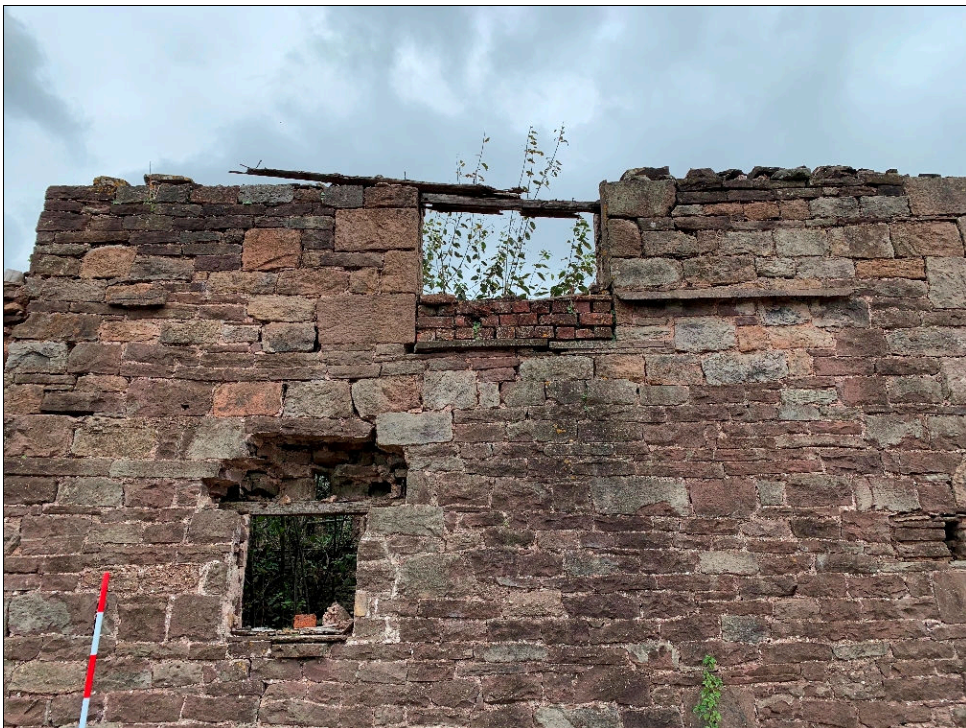
Plate 6: LLN2020_006 - A view of the windows in the southern side of the eastern annexe. The concrete line visible to the right of the upper window is thought to be the roof line of a lean-to which stood against this wall until the later 20 th century. Looking north.
