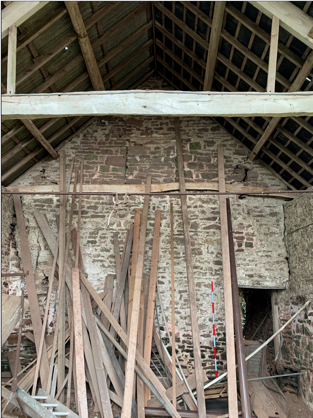
Plate 58: LLN2020_0058 - A view of the northern gable wall inside the barn. Note the blocked-up door in the centre of the upper part of the wall. The doorway to right the may original as it is a constructed feature and has not been cut through the wall. Its reveals are splayed slightly. The rip joint where the gable wall meets the eastern lateral wall to the right may be evidence of a repair or partial rebuild of the gable wall allowing for the doorway to be inserted when the adjacent cow house was added. There is also a blocked-up doorway left of centre of the wall on the ground floor, hidden by the planks stacked against the wall. Looking north.
