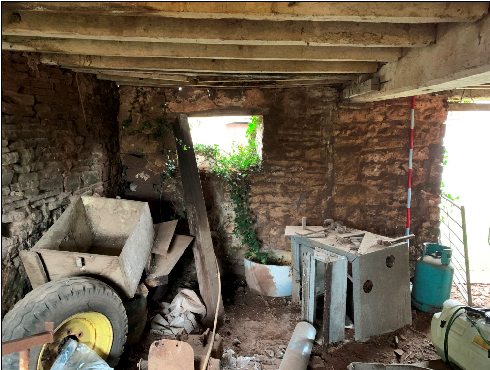
Plate 84: LLN2020_0084 - A view of the northern end of the eastern wall inside the cow house, showing the window with the straight joint of a blocked-up doorway seen to the right of the window. Looking east.
