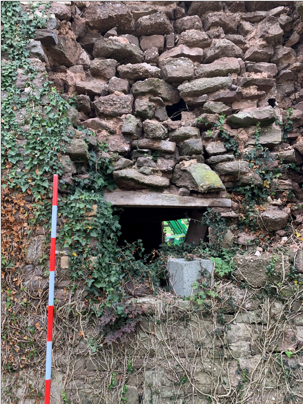
Plate 23: LLN2020_0023 - A view of the small window inserted through the eastern wall of the cow house towards its northern end. This appears to be a later feature partially cut through an earlier, blocked-up, doorway. Looking west.
