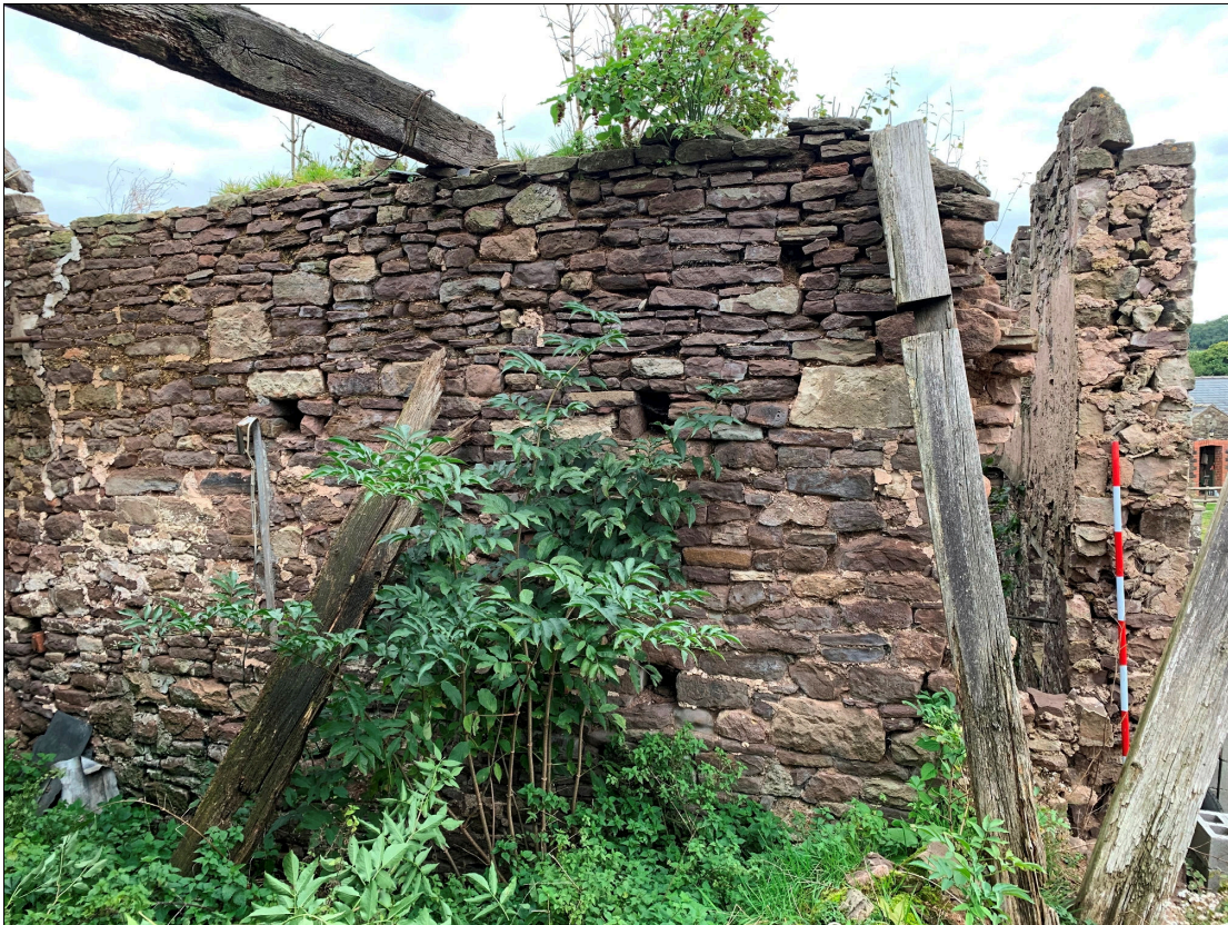
Plate 47: LLN2020_0047 - A view of the eastern wall inside the barn, showing the break in the southern end of the wall to the right, caused by the loss of the southern gable wall. This has exposed the end of the southern wall of the eastern annexe, which would have formerly been attached to the barn wall. Looking east.
