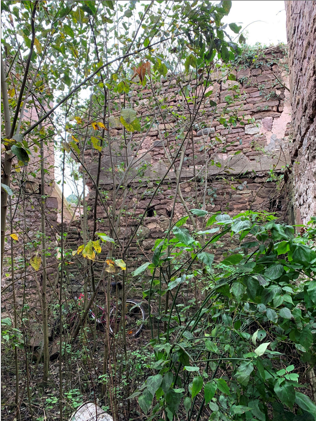
Plate 31: LLN2020_0031 - A view of the western wall inside the eastern annexe. The wall is the eastern wall of the earlier barn. The gap to the left has been caused by the collapse of the southern gable wall of the barn. Looking west-southwest.
