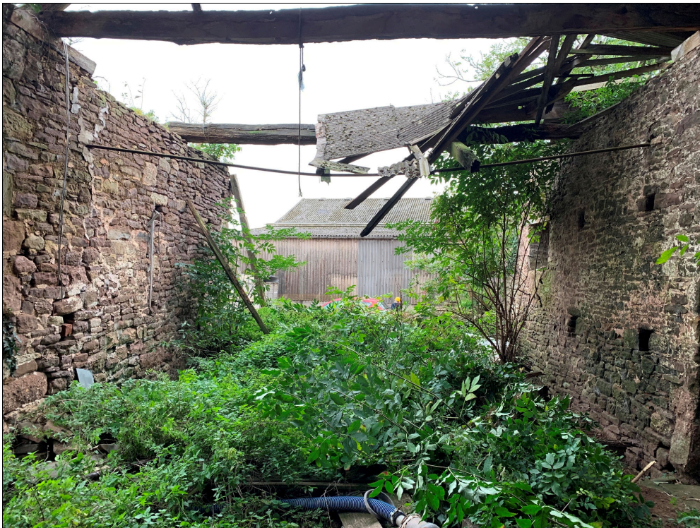
Plate 57: LLN2020_0057 - A view inside the barn showing the lateral walls mostly cleared of vegetation. Note the steel tie-bar linking the lateral walls. Looking south.
