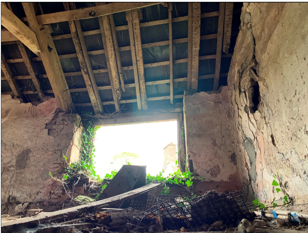
Plate 77: LLN2020_0077 - A view of the window in the eastern side of the upper floor. Looking east.
