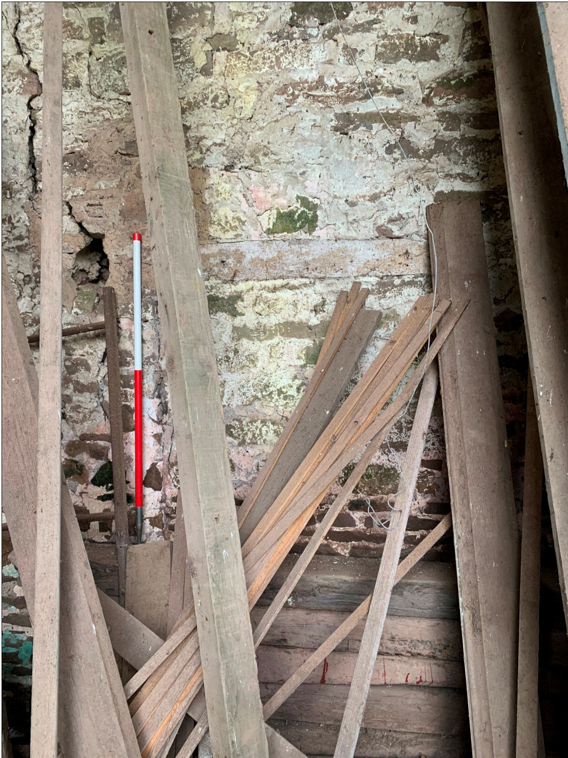
Plate 81: LLN2020_0081 - A partial view of the blocked up central doorway in the ground floor inside the barn. Looking north-northwest.
