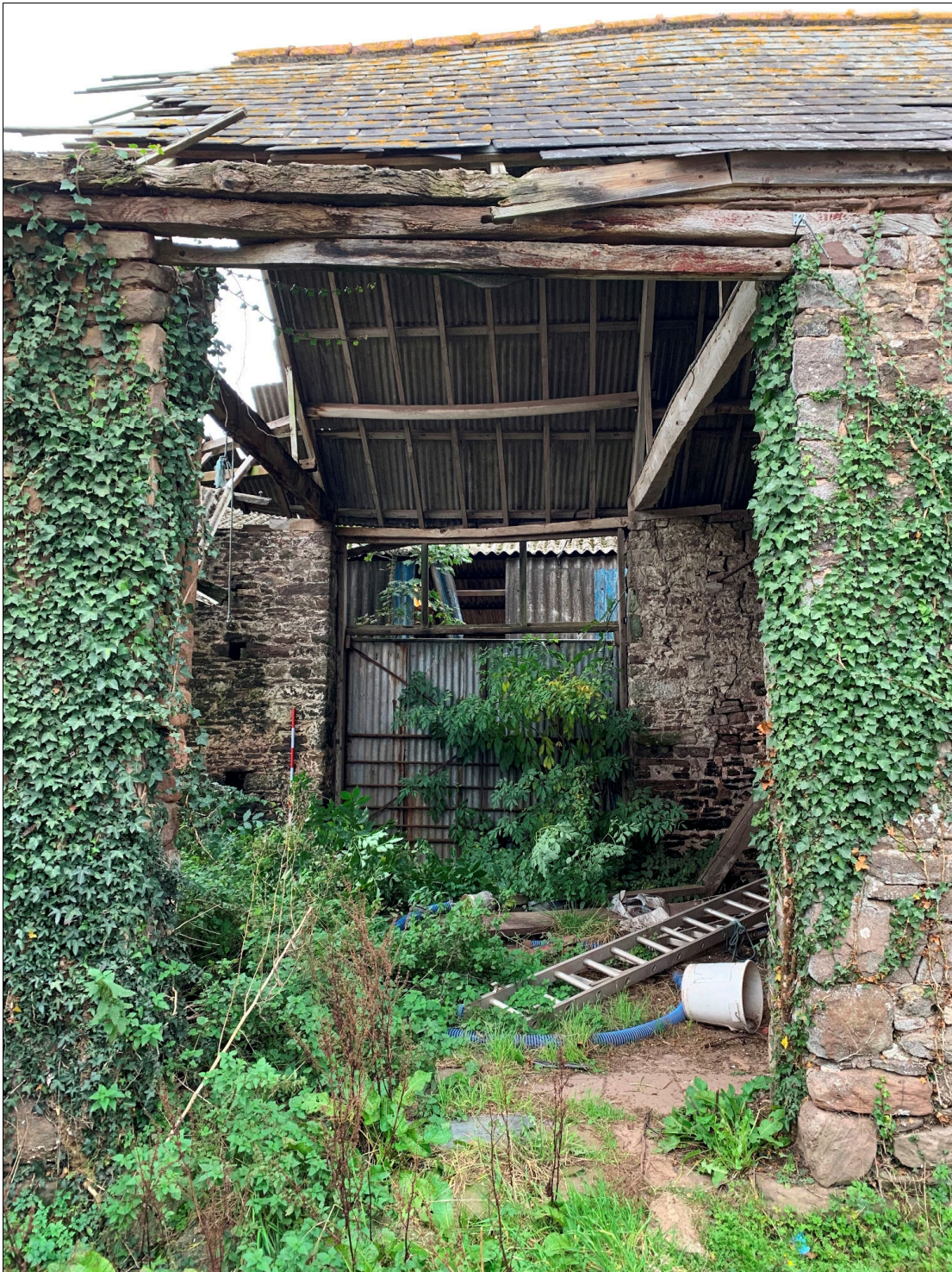
Plate 44: LLN2020_0044 - A view through the eastern door of the barn towards the opposing western door. The large, opposed doors are typical of a post-medieval threshing barn. Looking west.
