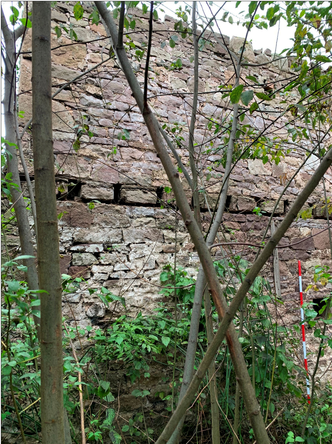
Plate 35: LLN2020_0035 - A view of the joist holes in the northern wall of the eastern annexe. Looking north-northeast.
