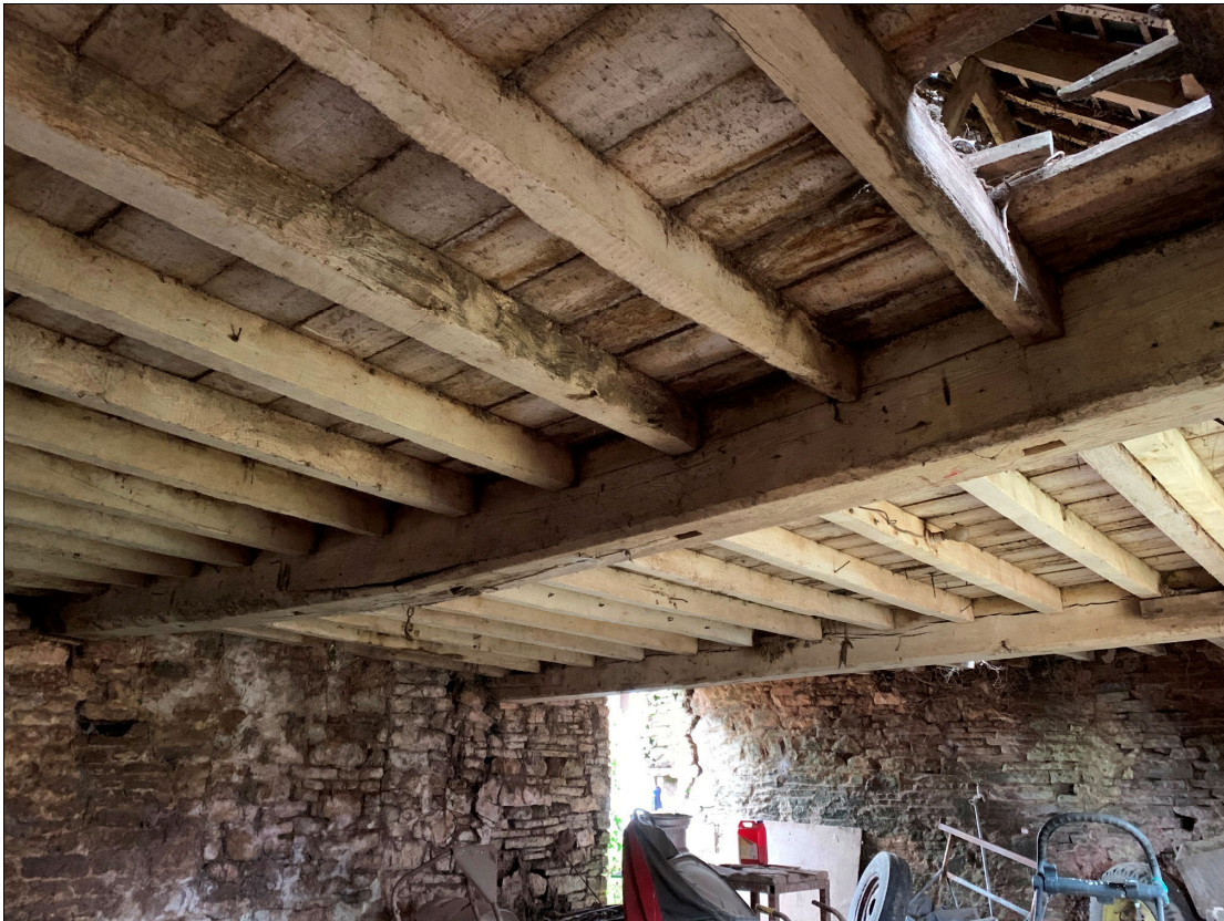
Plate 88: LLN2020_0088 - A view of the ceiling of the ground floor inside the cow house. Note the niches which would have formerly held posts for feeding stalls cut into the underside of the beam. Looking northwest.
