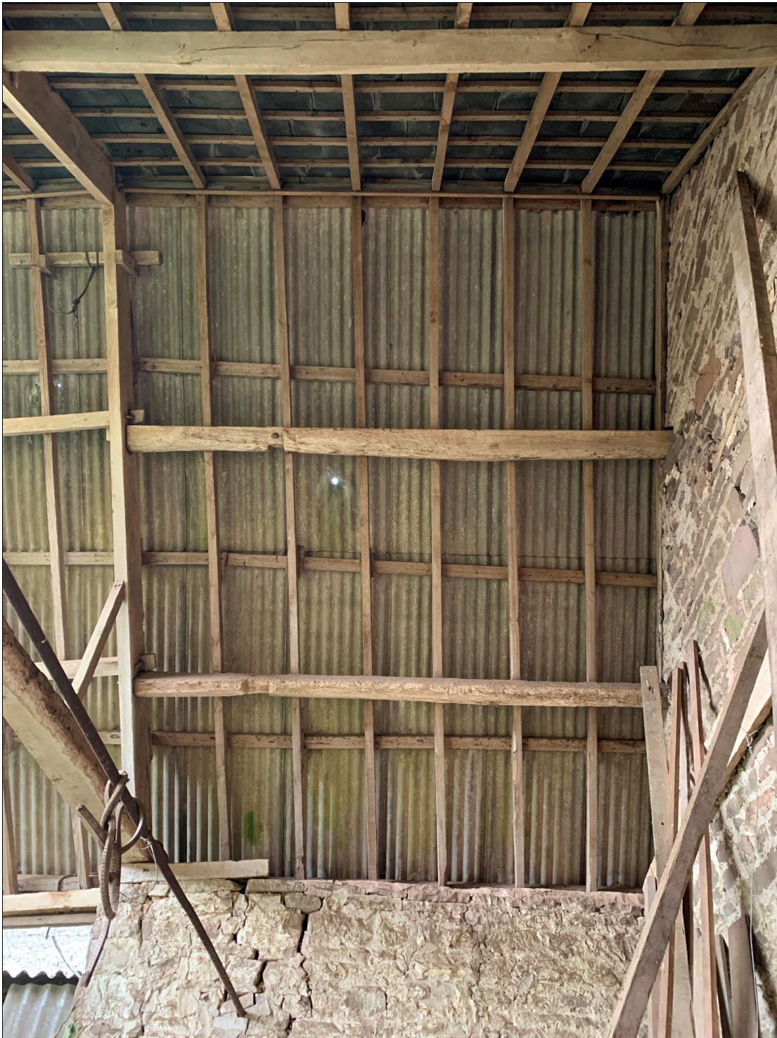
Plate 65: LLN2020_0065 - A view of the roof inside the northern end of the barn. The purlins appear machine sawn and relatively recent, but the rafters appear to be reused timbers from an earlier roof. The truss to the left appears to be machine sawn (later 19 th century) whilst the beam at its base is clearly earlier. It seems likely that a new slate roof was put across the barn when the cow house was added to its northern end. It appears that timbers were reused or replaced in the barn roof at this time. Looking west.
