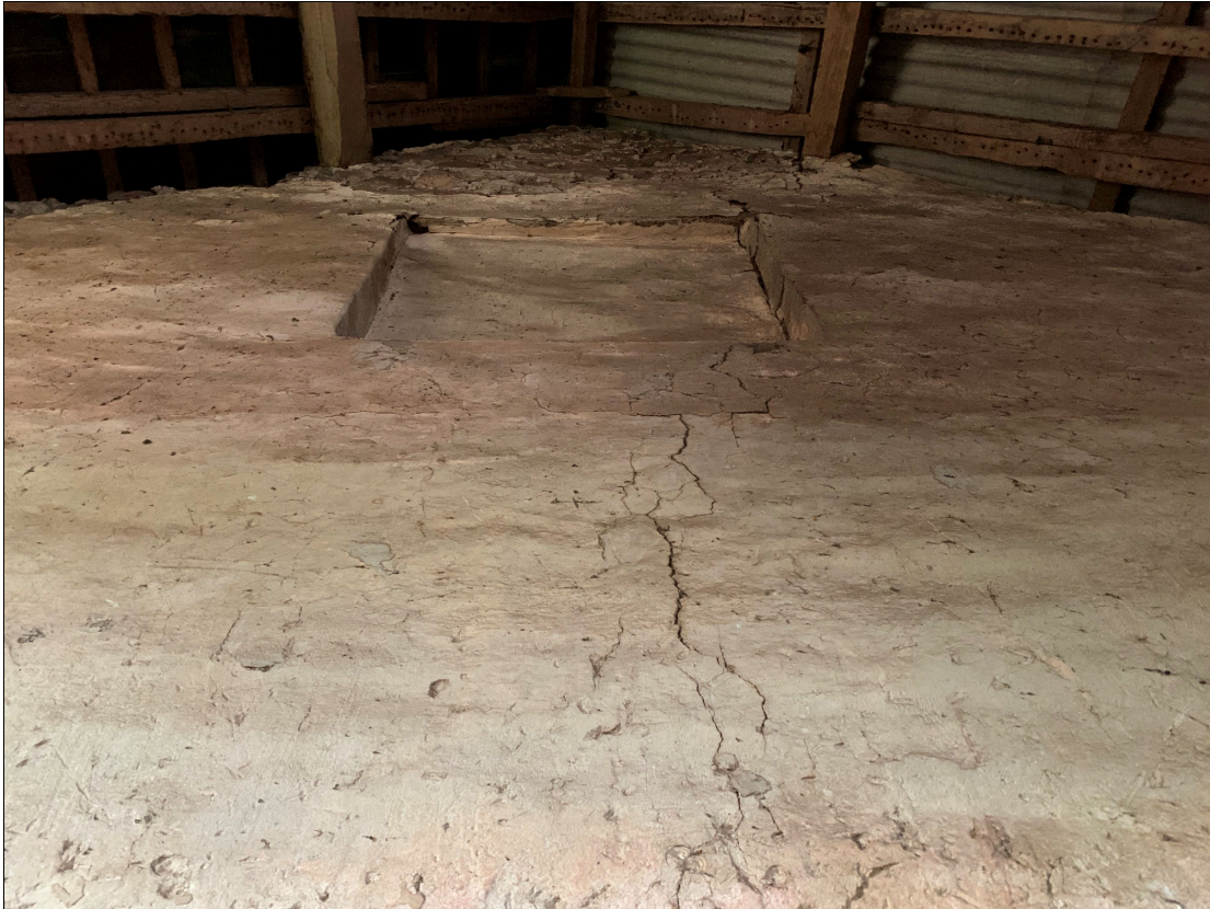
Plate 80: LLN2020_0080 - A view up the southern wall of the upper floor of the cow house, showing the blocked-up doorway high up in the peak of the gable. Looking south. The wall remains covered with a thick plaster.
