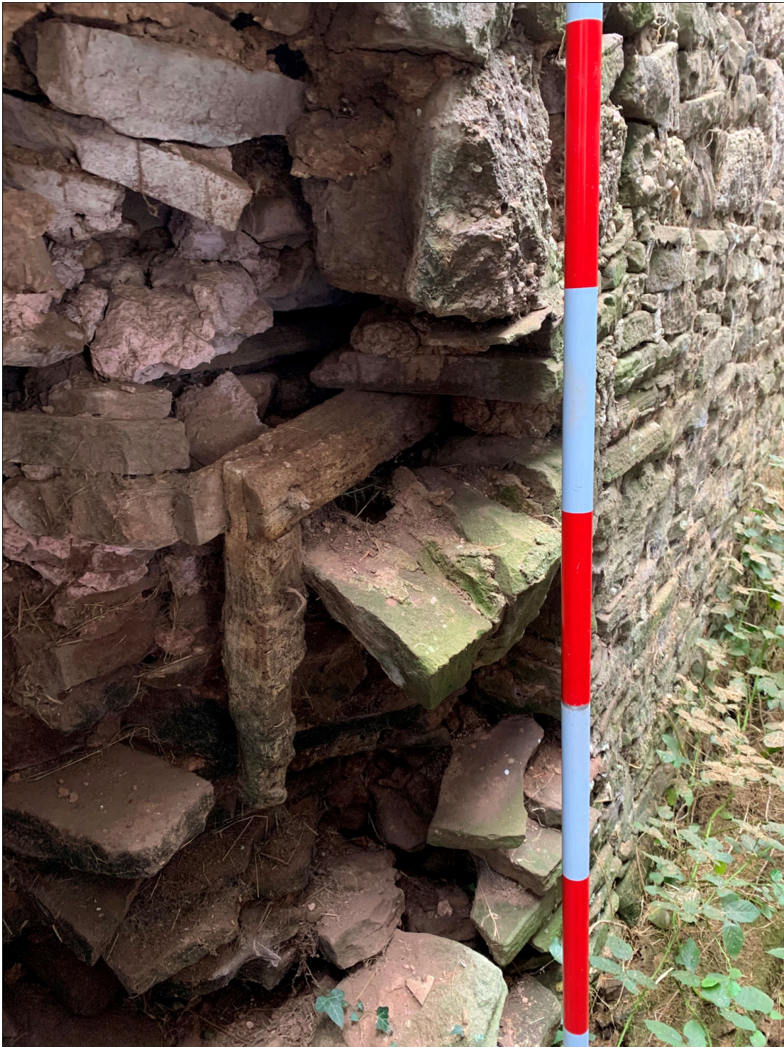
Plate 71: LLN2020_0071 - A view of the damaged wall at the northwestern corner of the barn showing a timber frame, possibly an old window frame, built into the fabric of the wall. Note that there is also lime mortar within the core of the wall. Looking southeast.
