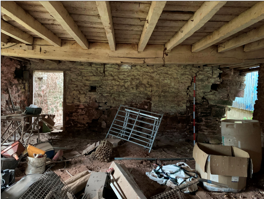
Plate 73: LLN2020_0073 - A view of the southern wall of the cow house from inside the building. The doorway into the barn is to the left, a blocked-up doorway is seen right of centre and an external doorway to the right. Note the beam, joists and floorboards of the upper floor. Looking south.
