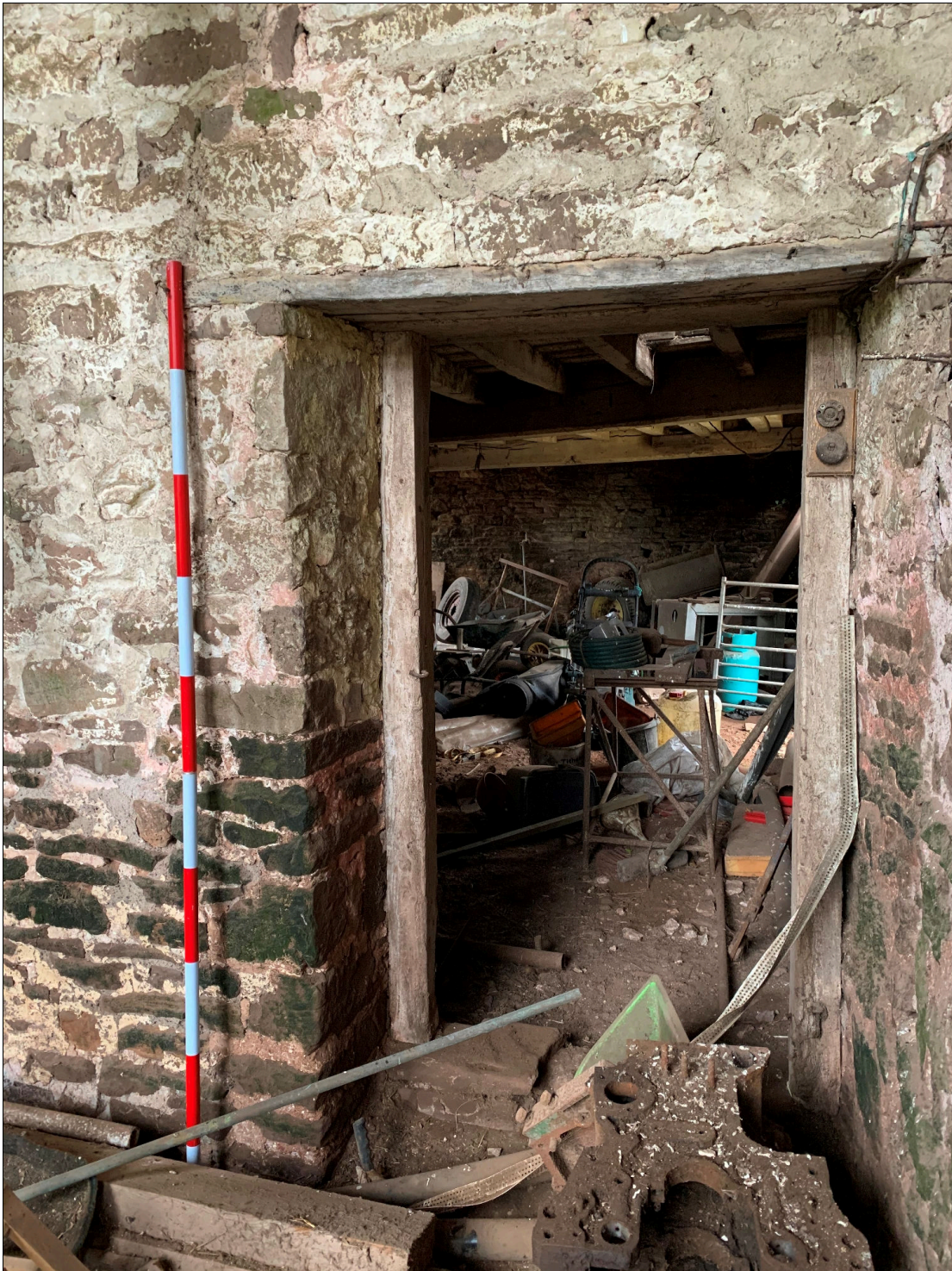
Plate 60: LLN2020_0060 - A view into the cow house through the door linking it with the barn. Looking north-northwest.
