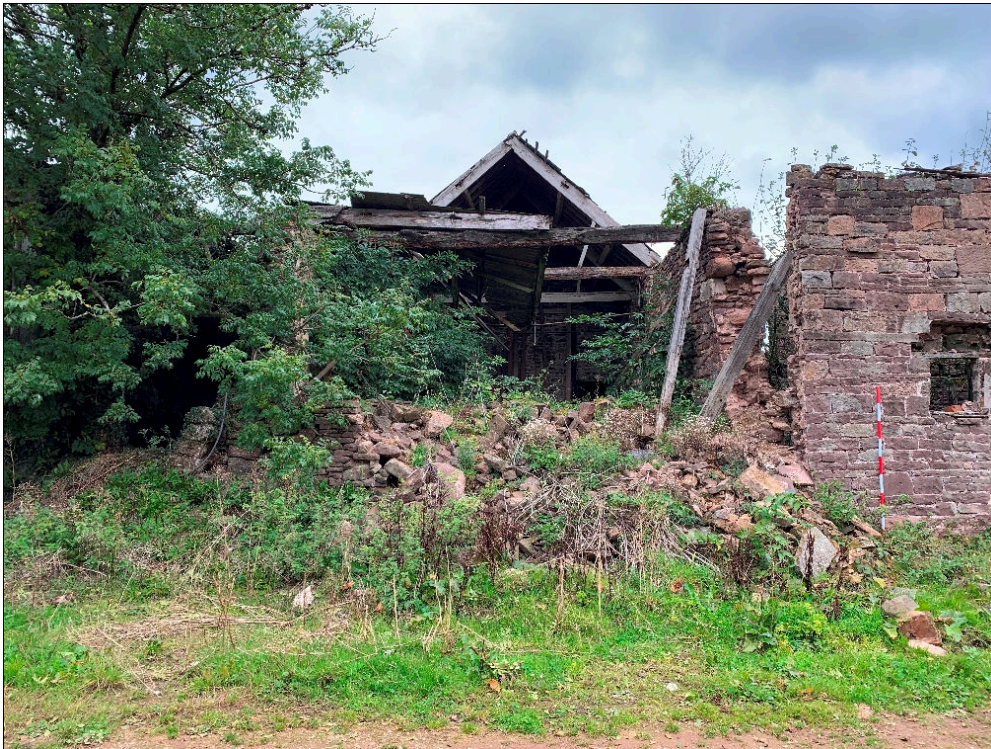
Plate 1: LLN2020_001 - A view of the now collapsed southern end of the barn at Llan y Nant. Looking north.
