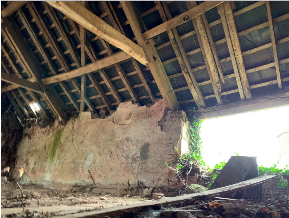
Plate 76: LLN2020_0076 - A view of the eastern side of the upper floor. Looking northeast.
