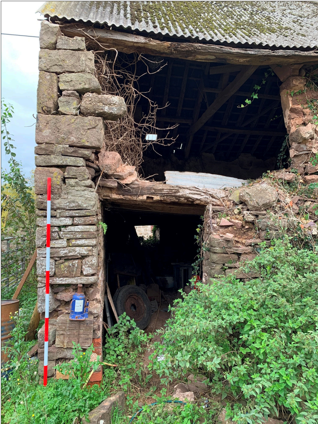
Plate 28: LLN2020_0028 - Another view of the doorway at the northern end of the western wall of the cow house. The timber lintel was probably originally hidden behind a sandstone arch – the angled stonework seen to the left of the lintel was probably shaped to allow the stones of the arch to be fitted in place. Looking east.
