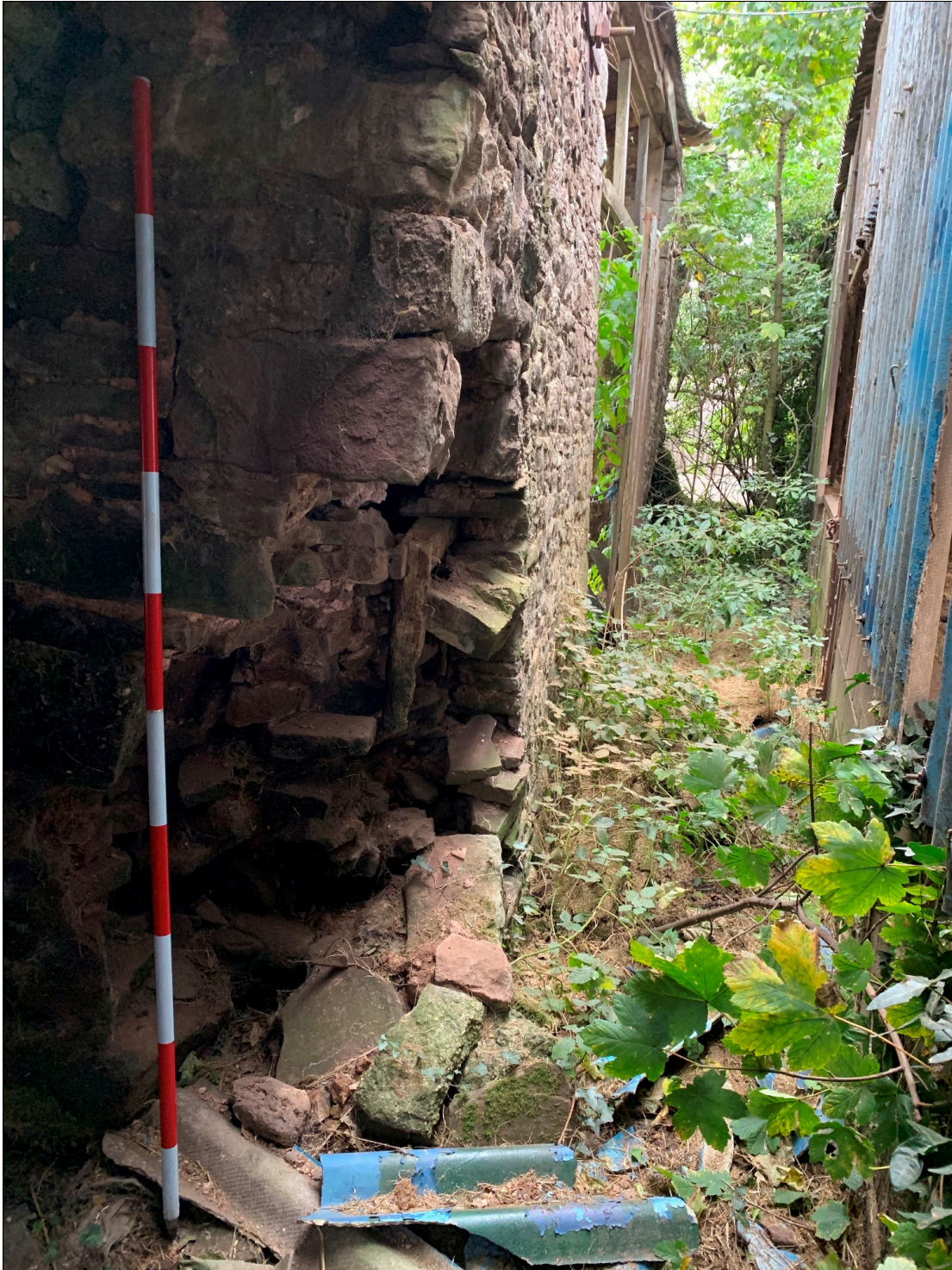
Plate 72: LLN2020_0072 - A view of the damaged wall at the northwestern corner of the barn. Looking south.
