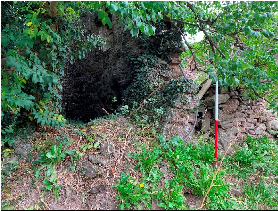
Plate 5: LLN2020_005 - Another view of the southwest corner of the barn, showing the break between the western and southern walls. Looking northeast.
