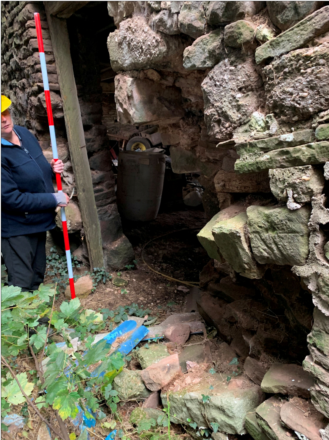
Plate 70: LLN2020_0070 - A view of the damaged wall at the northwestern corner of the barn, where it seems the lower quoin stones are missing. The cow house door is left of centre. Looking northeast.
