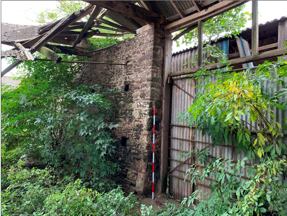
Plate 42: LLN2020_0042 - A view of the western doorway and wall inside the barn. Note the ventilation holes in the wall. Looking southwest.
