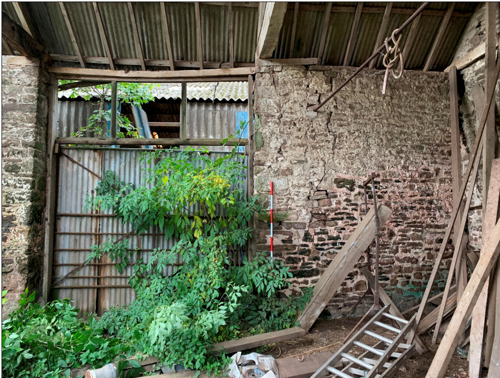
Plate 56: LLN2020_0056 - A view of the door and northern end of the western wall inside the barn. Note the corrugated steel sheeting on the western side of the roof. Looking west.
