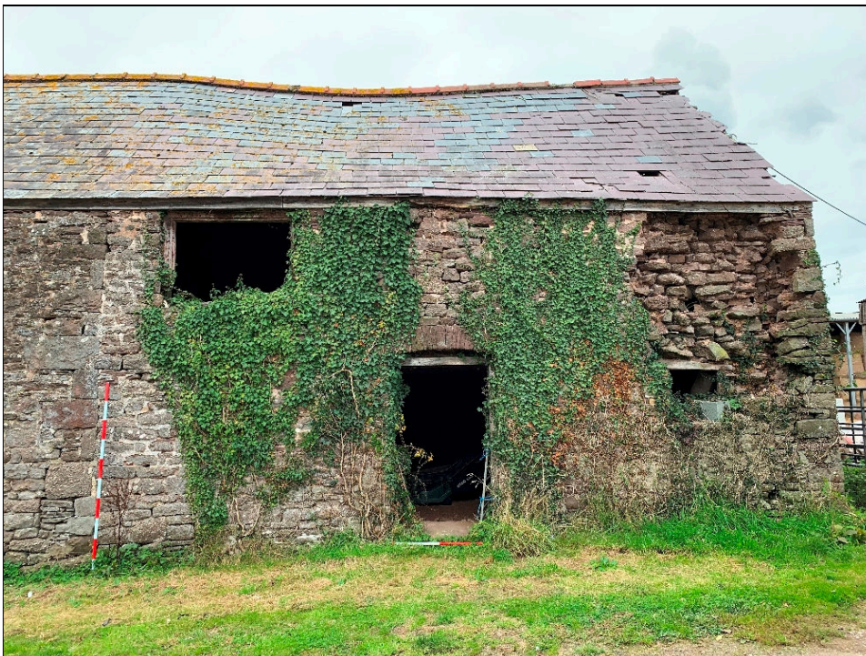
Plate 18: LLN2020_0018 - A view of the eastern wall of the cow house. Note the loss of the outer face of the wall in the upper floor at the northern end of the building. Looking west.
