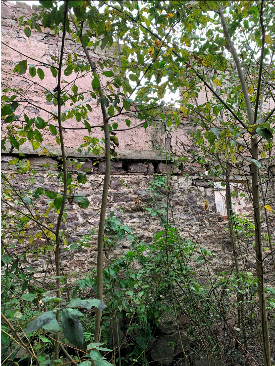
Plate 30: LLN2020_0030 - A view of the joist holes inside the southern wall of the eastern annexe. Looking southwest.
