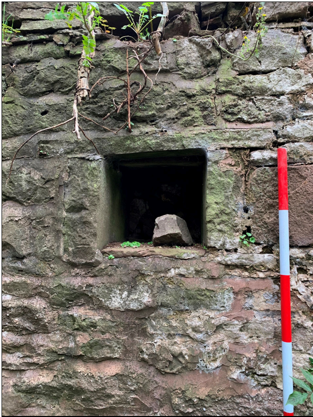
Plate 38: LLN2020_0038 - A view of the niche at the western end of the northern wall inside the eastern annexe. Looking north-northwest.
