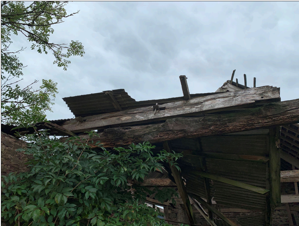
Plate 49: LLN2020_0049 - A view of the timbers of a broken roof truss at the southern end of the barn. Looking north.
