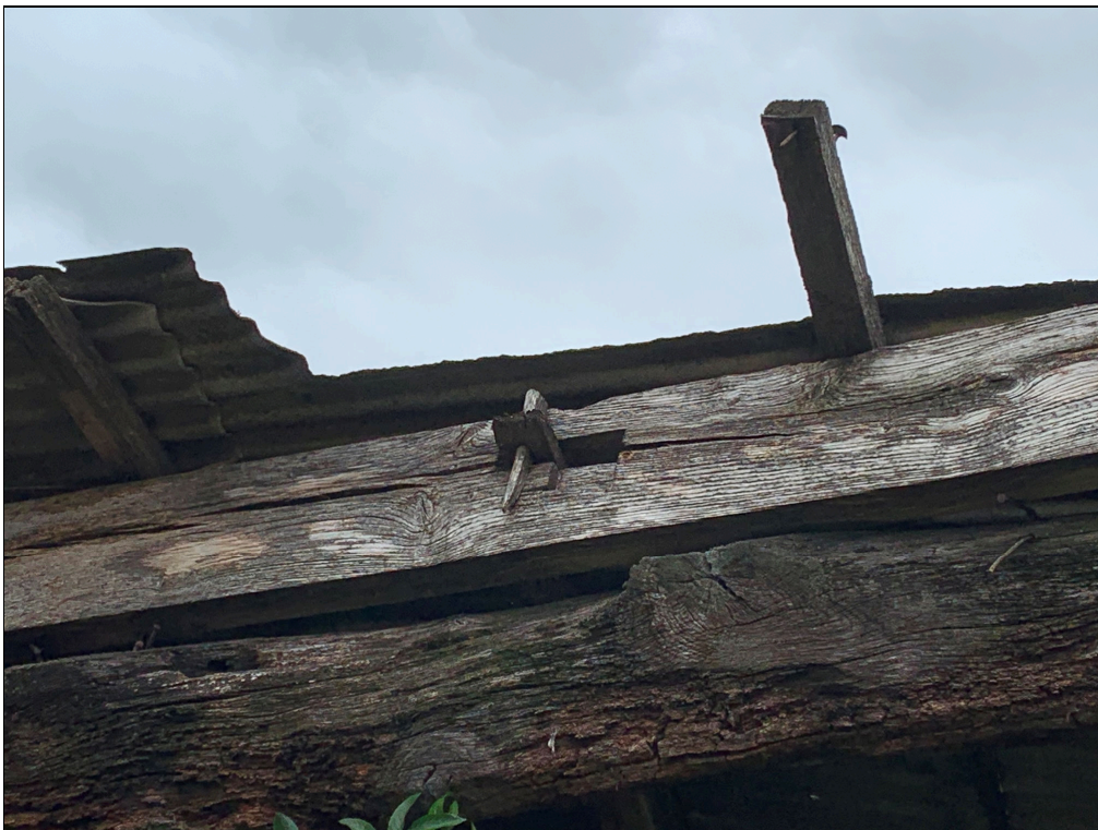
Plate 50: LLN2020_0050 - A view showing more detail of the broken roof truss, which had wooden pegs connecting the timbers. Looking north.
