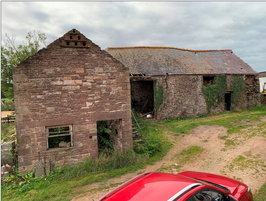
Plate 93: LLN2020_0093 - A view of the barn and cow house complex, with the eastern annexe in the foreground. Looking west-northwest.
