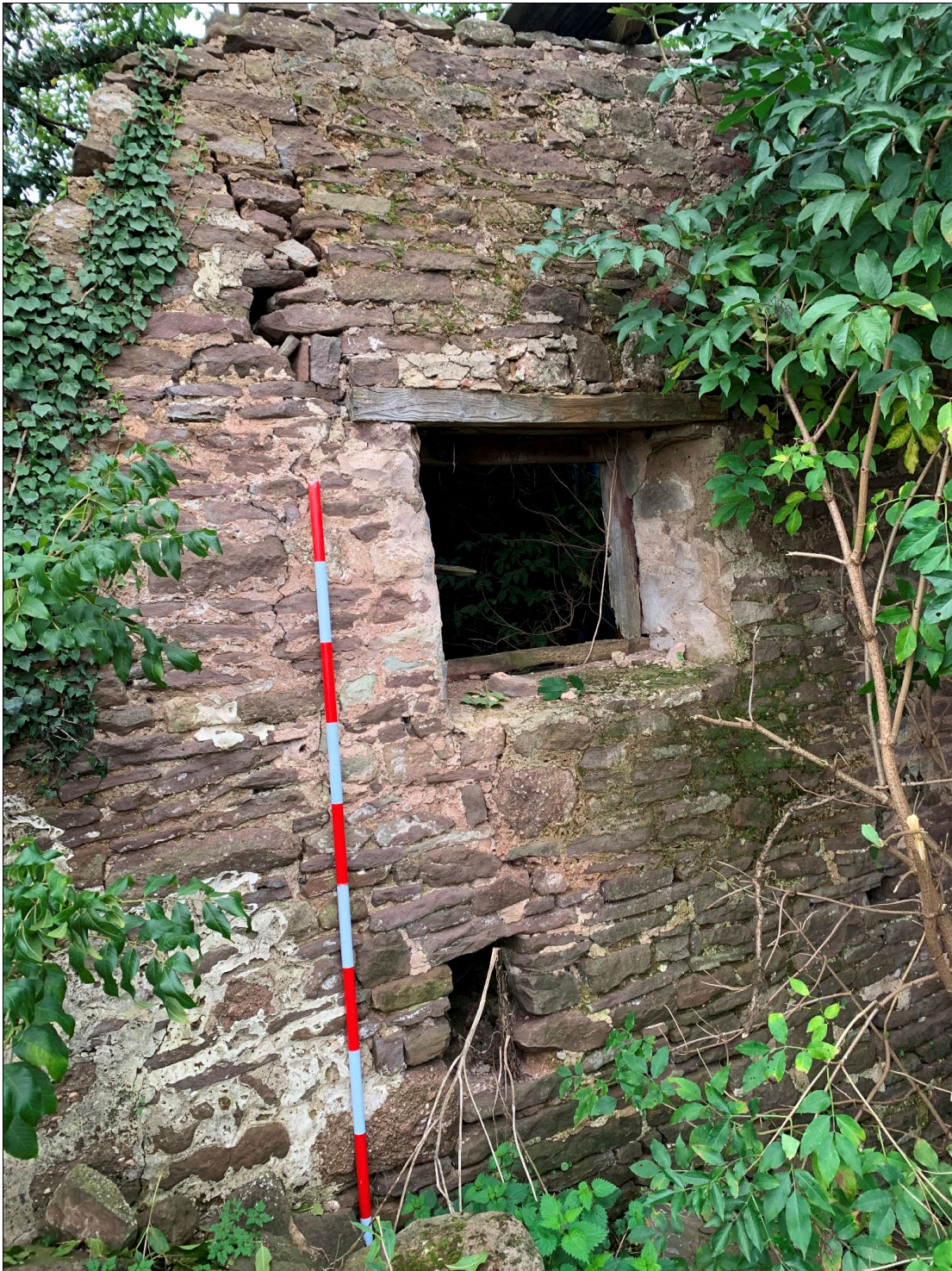
Plate 48: LLN2020_0048 - A view of the window inserted into the southern end of the western wall of the barn. A ventilation hole below is probably one of a pair, the upper vent having been lost when the window was inserted. Looking west-northwest.
