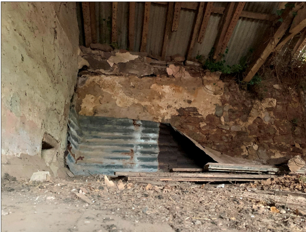
Plate 79: LLN2020_0079 - A view of the western side of the upper floor. Looking west.
