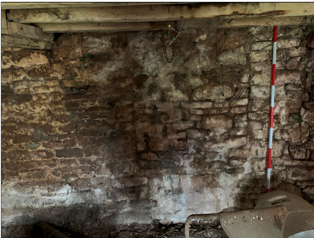
Plate 87: LLN2020_0087 - A view of the blocked-up central doorway in the western wall of the cow house. Looking west.
