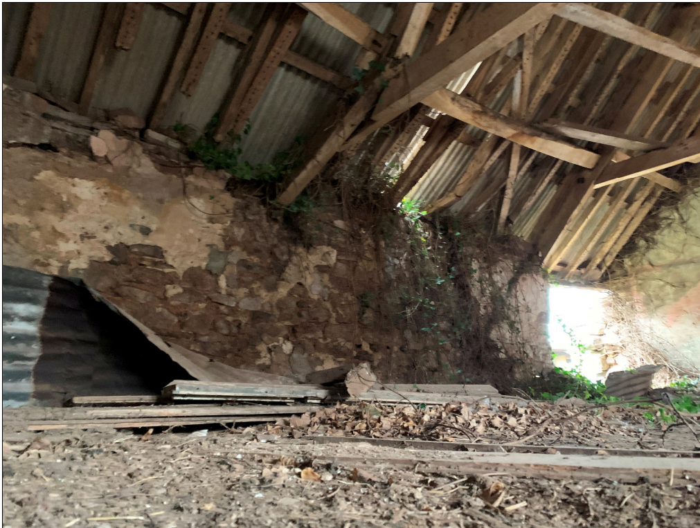
Plate 78: LLN2020_0078 - A view of the western side of the upper floor. Looking northwest.
