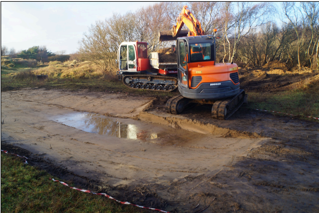
Plate 6: MMW2020_106. Sand scrape 4 during excavation, looking northwest with the spoil heap in the trees to the north.
