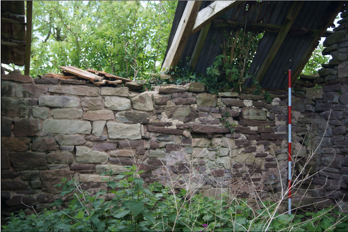
Plate 37: BGT2020_037, internal view of the western and central part of the southern wall, looking south-southwest.
