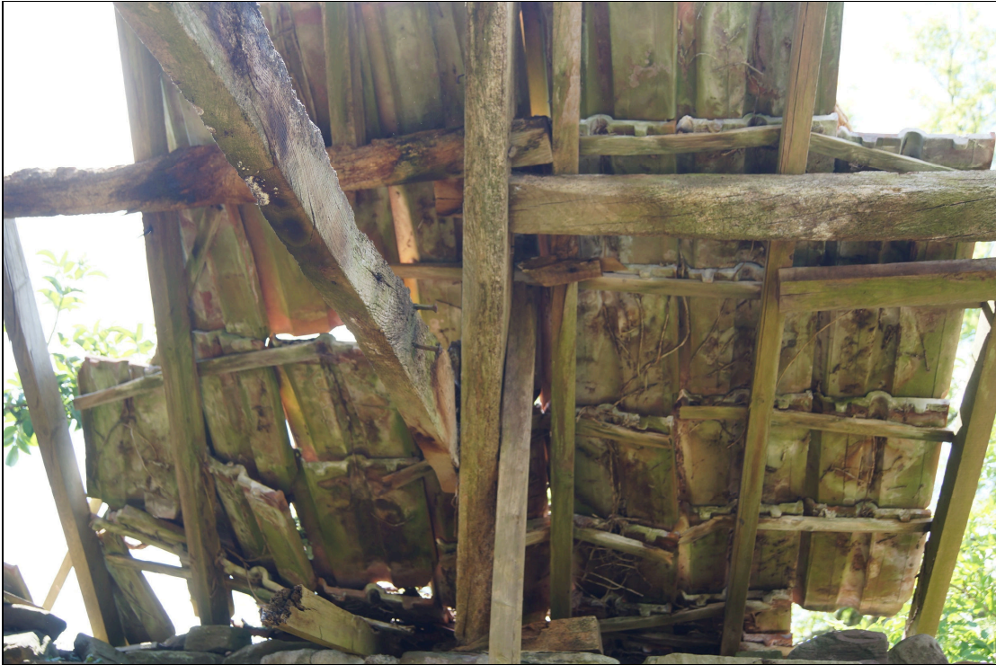
Plate 54: BGT2020_054, internal view of timbers in the middle of the roof facing south.
