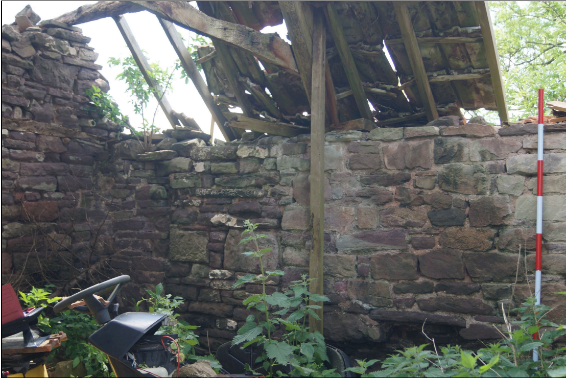
Plate 39: BGT2020_039, internal view of eastern and central part of the southern wall looking southeast.
