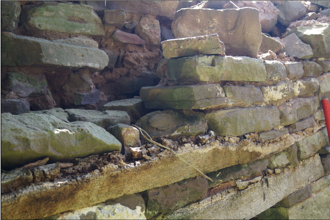
Plate 26: BGT2020_026, detail of wallplate and collapsed gable above east window looking south-east.
