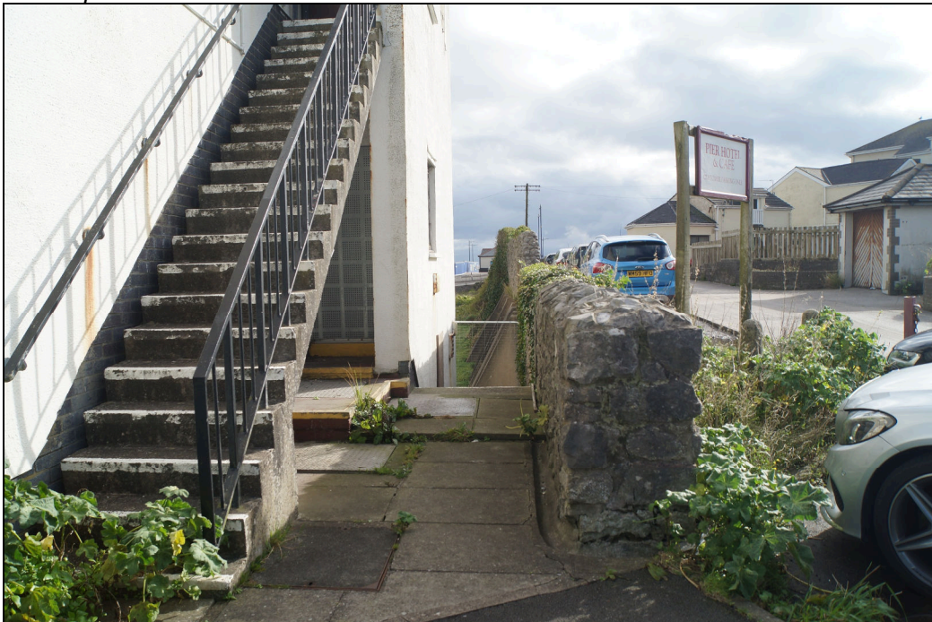
Plate 24: Looking south along the western boundary of the Glamorgan Holiday Hotel. This retaining wall is supported by more recent buttresses but the first ones were put in place when a building against the wall was removed prior to the construction of the hotel (Welsh Aerial Photography Unit 1967 and 1974)
