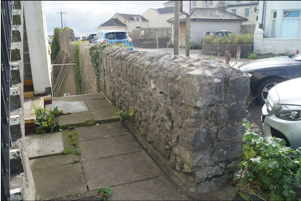
Plate 25: Looking south along the western boundary of the Glamorgan Holiday Hotel showing the stone retaining wall. The upper part of this wall may have been rebuilt but probably continues below ground to a similar level as the rest of the retaining wall which defined around this area previously
