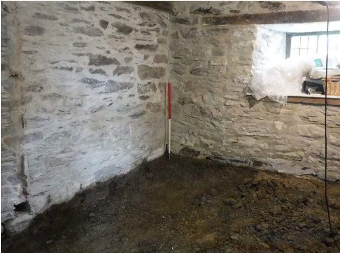
Plate 7: North-western corner of development area (study) after the lowering of the floor. 1m scale.
