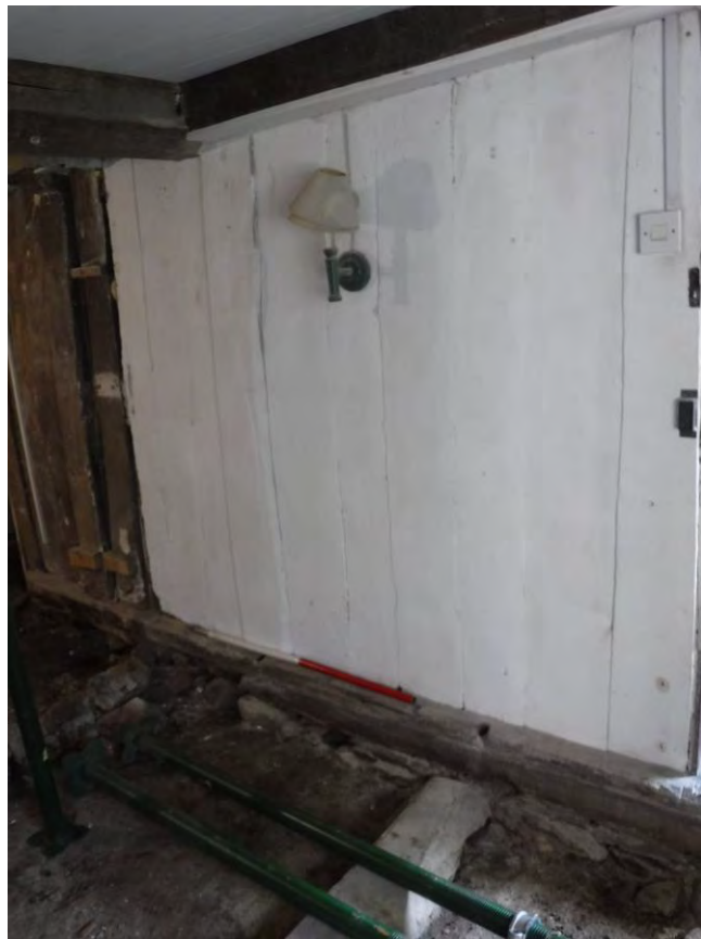
Plate 2: Post and panel partition viewed from development area (Dining Room). 1m scale.
