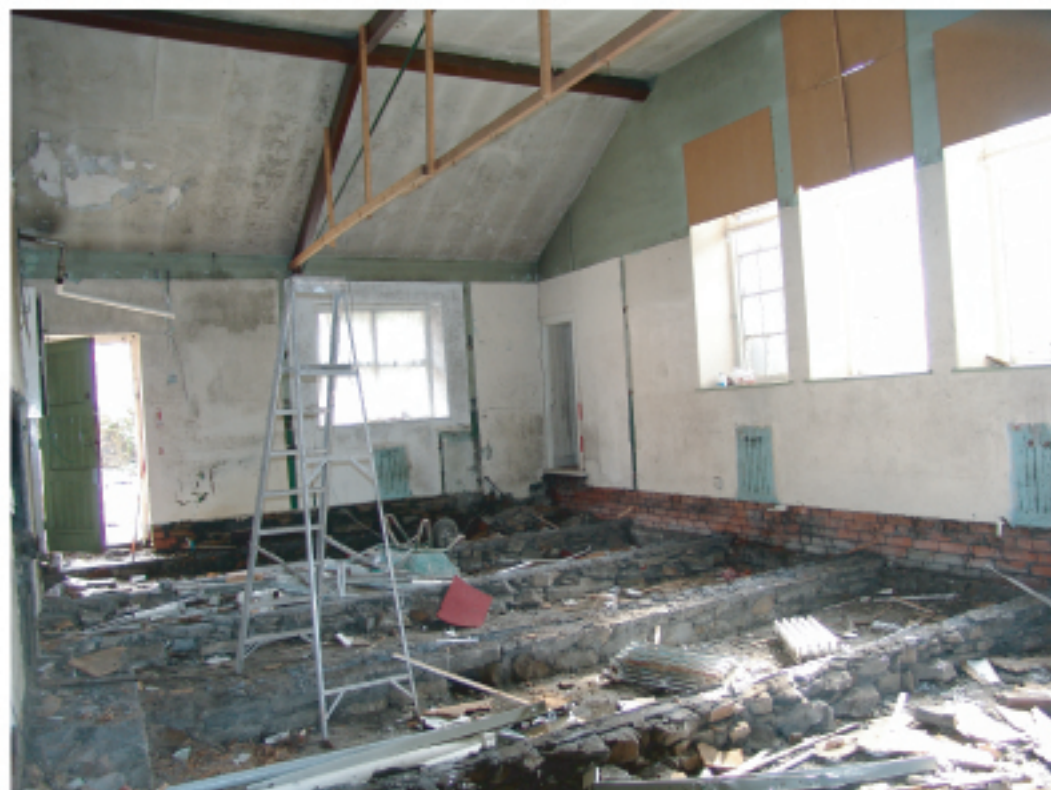
Reason for image Internal view of vestry/store area showing side entry door and internal toilet to rear.
