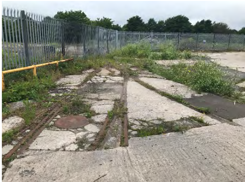
Plate 9: Railway lines at the south west of the study site, close to the location of the former foundry (looking west towards the River Taff)
