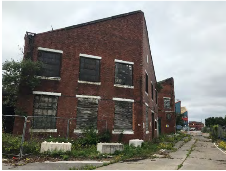
Plate 2: East elevation of mid-20 th century industrial unit associated with the Curran Engineering Works (looking north)
