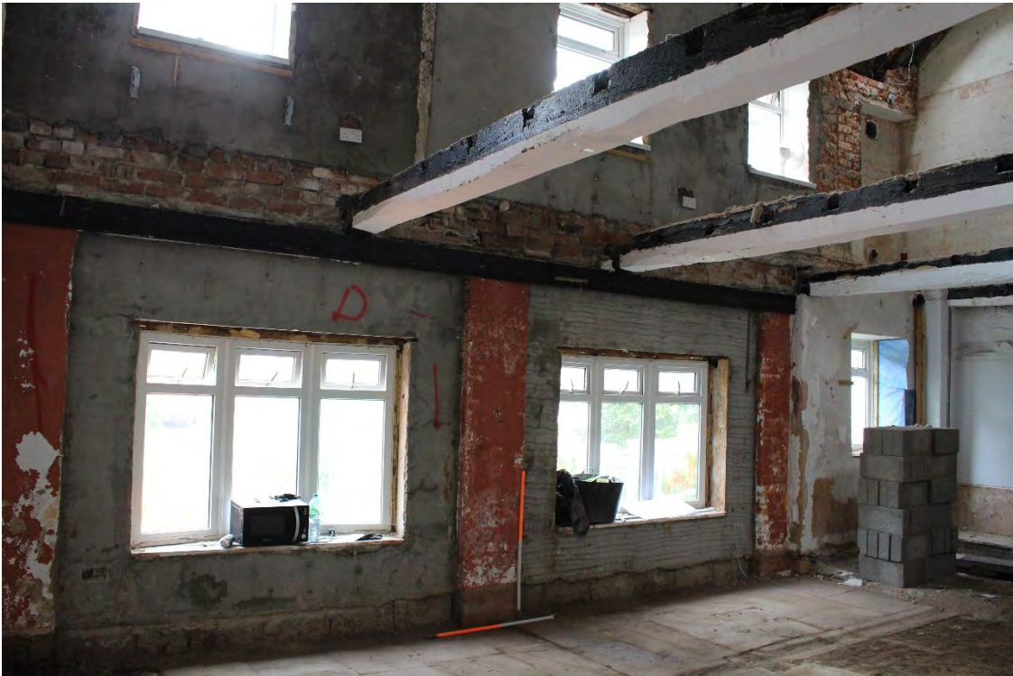
Image EDP A1.8: View of the western wall of G1, showing the blockwork infill of the former openings with windows. The floor joists of the upper floor can also be seen.
