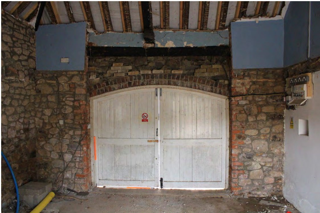
Image EDP A1.24: View of the interior of G3 (coach house) showing the inside of the former opening and infill above the brick arch.
