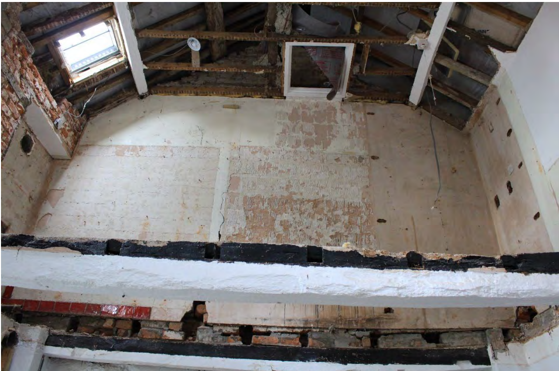
Image EDP A1.13: Upper part of the northern gable, which is rendered brickwork, looking north.
