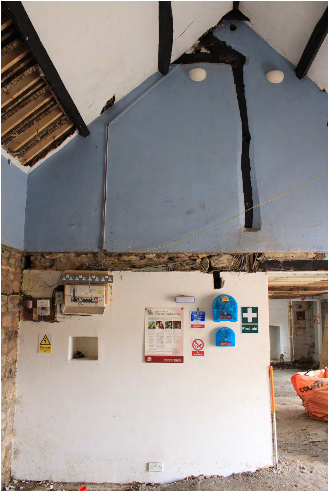
Image EDP A1.28: General view of G3 (coach house) looking north, note the exposed timber frame within the gable end indicating the roof had been raised.
