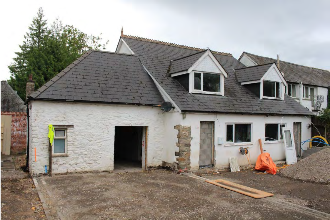
Image EDP A1.2: View of the eastern elevation of the 'Cottage', showing the main section to right and 'coach house' section to left. The majority of the fabric on the main section, shown here, is later 20 th century in date.
