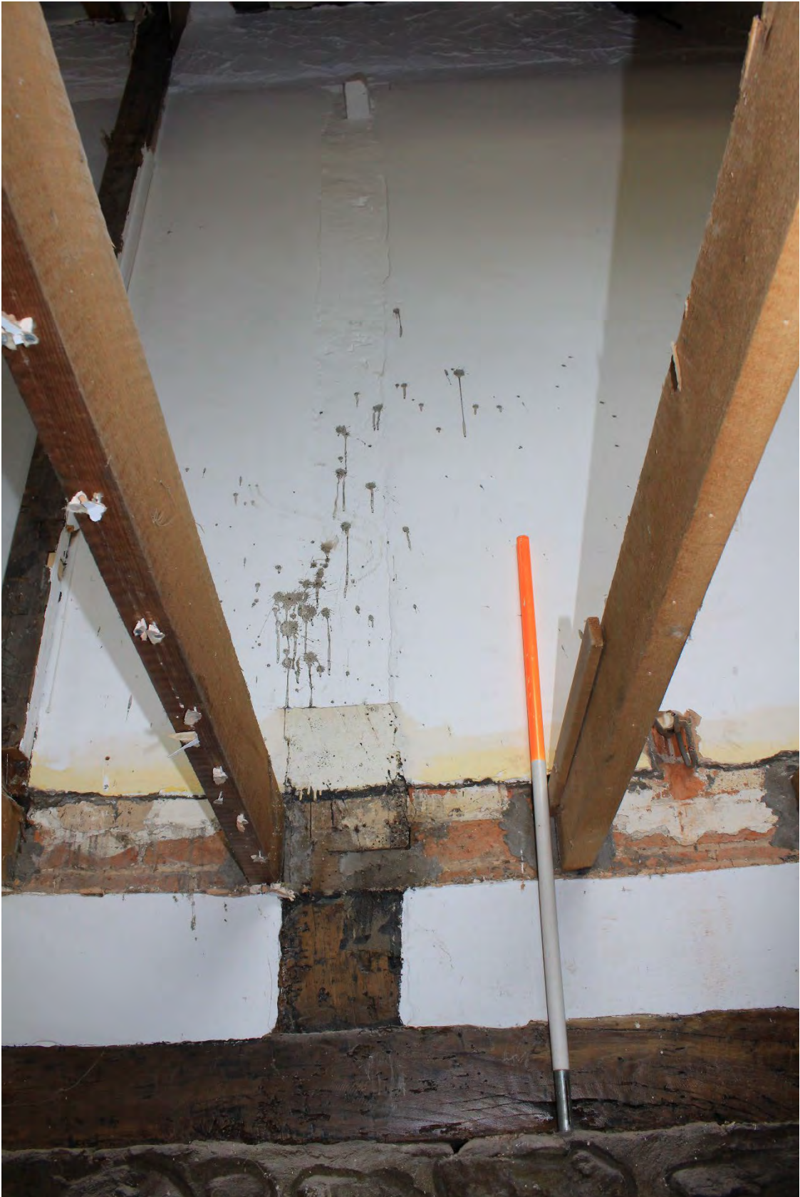
Image EDP A1.18: View of the exposed 19 th century timber upright in the upper part of the central spine wall looking west, showing the cut off timber truss.
