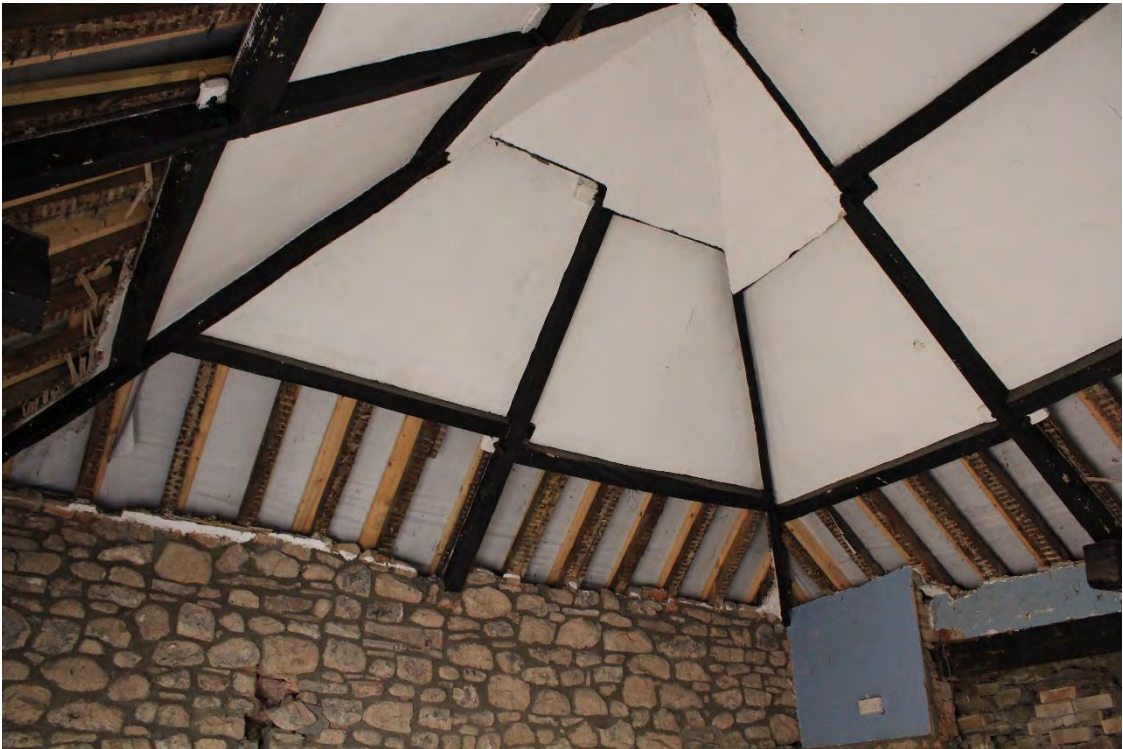
Image EDP A1.27: View of the roof structure within G3 (coach house) looking south.
