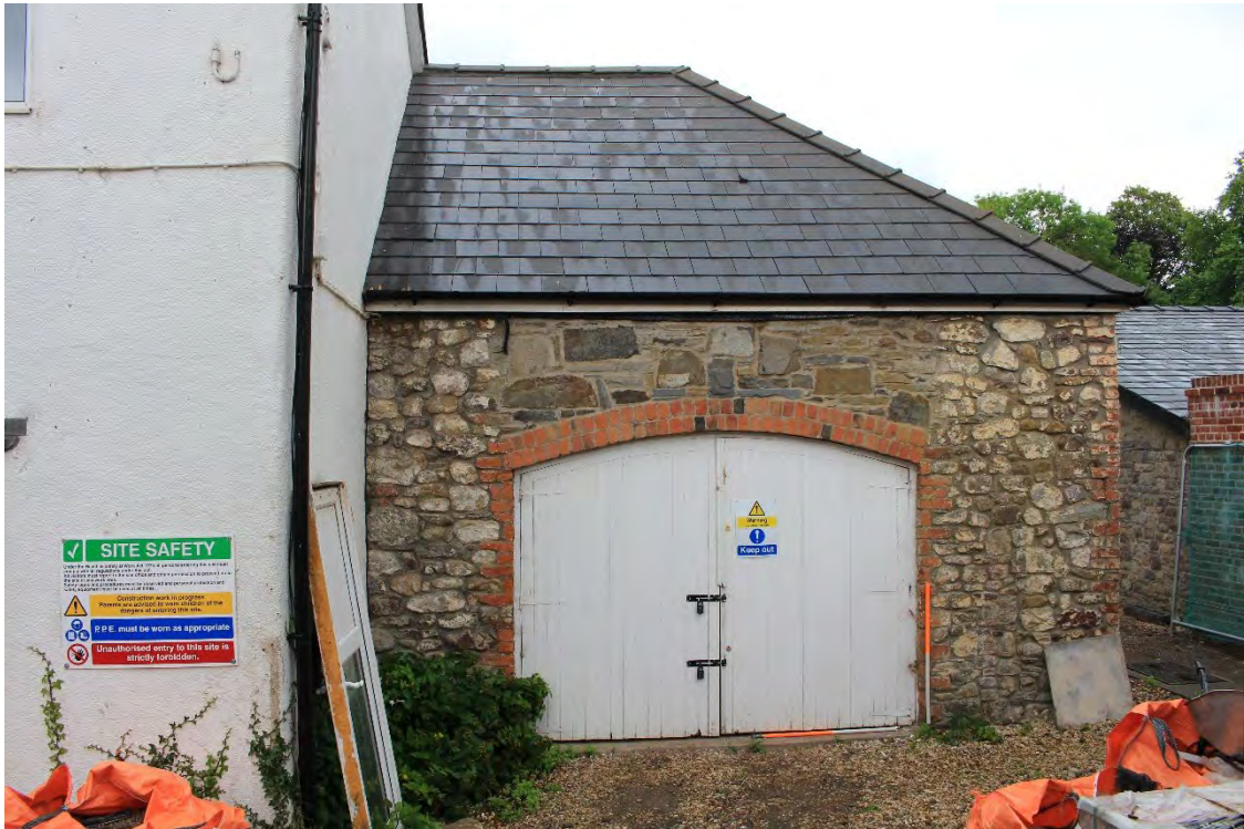
Image EDP A1.23: View of the western elevation of the 'coach house' section looking east, showing the clearly infilled section of opening above the brick arch.
