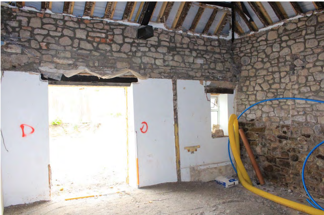
Image EDP A1.26: General view of the Interior of G3 (coach house) section, looking east.
