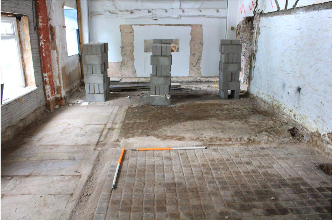
Image EDP A1.4: General view of room G1 looking north, showing the flooring.
