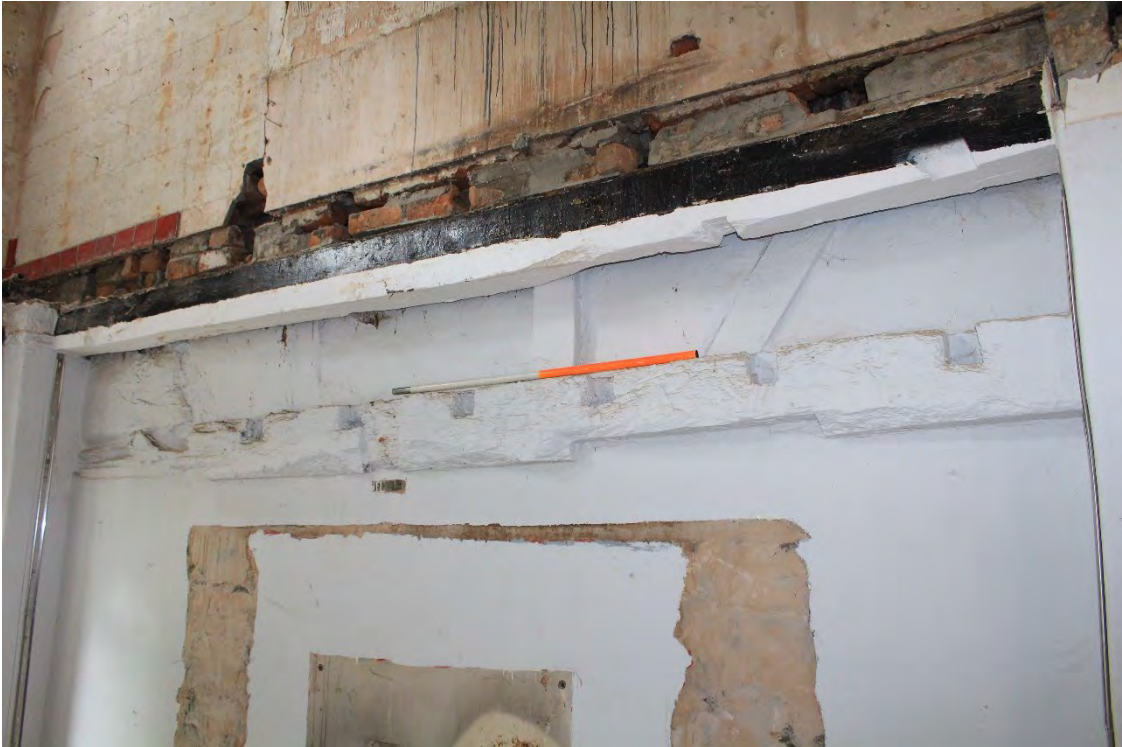
Image EDP A1.14: Detail of the timber beam looking north-west and showing the cutout recess indicating a door into the northern building. Also showing the later beam above, where the floor has clearly been raised.
