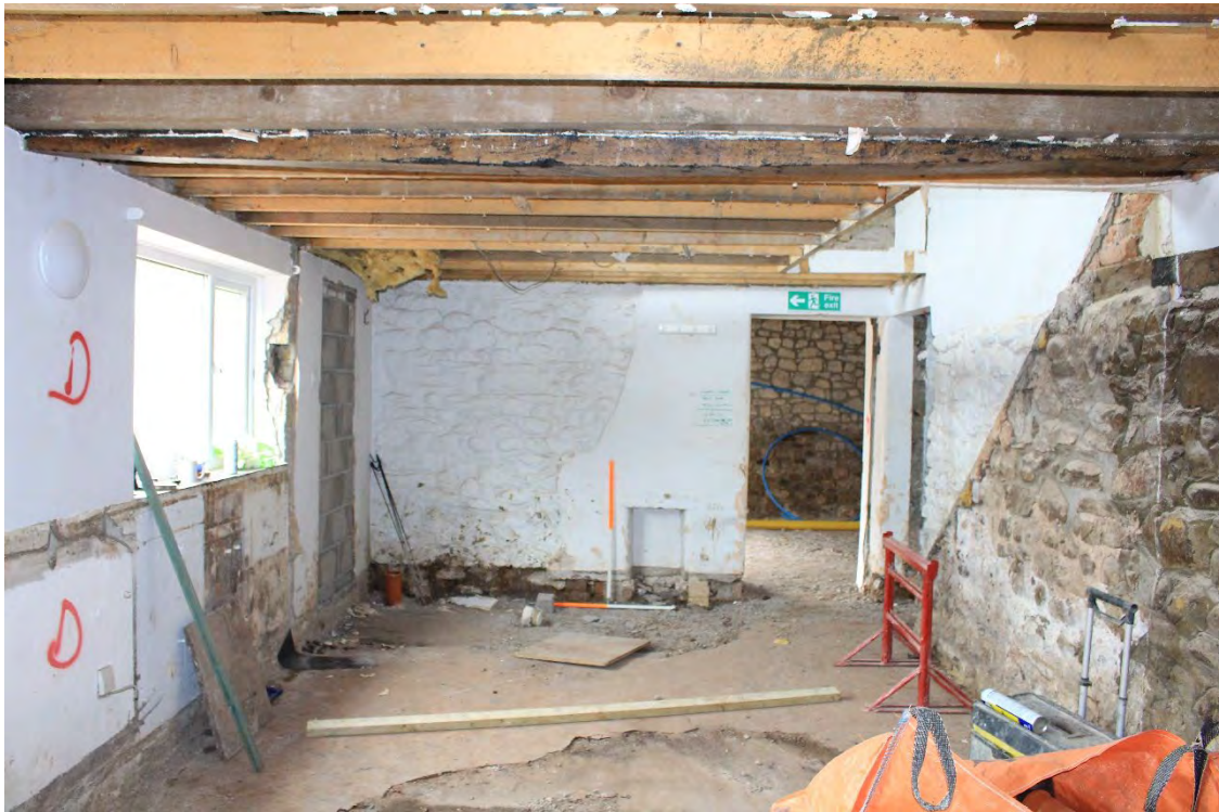
Image EDP A1.19: General view of Room G2 looking south, showing the lower part of the gable and door into the 'coach house' section G3.
