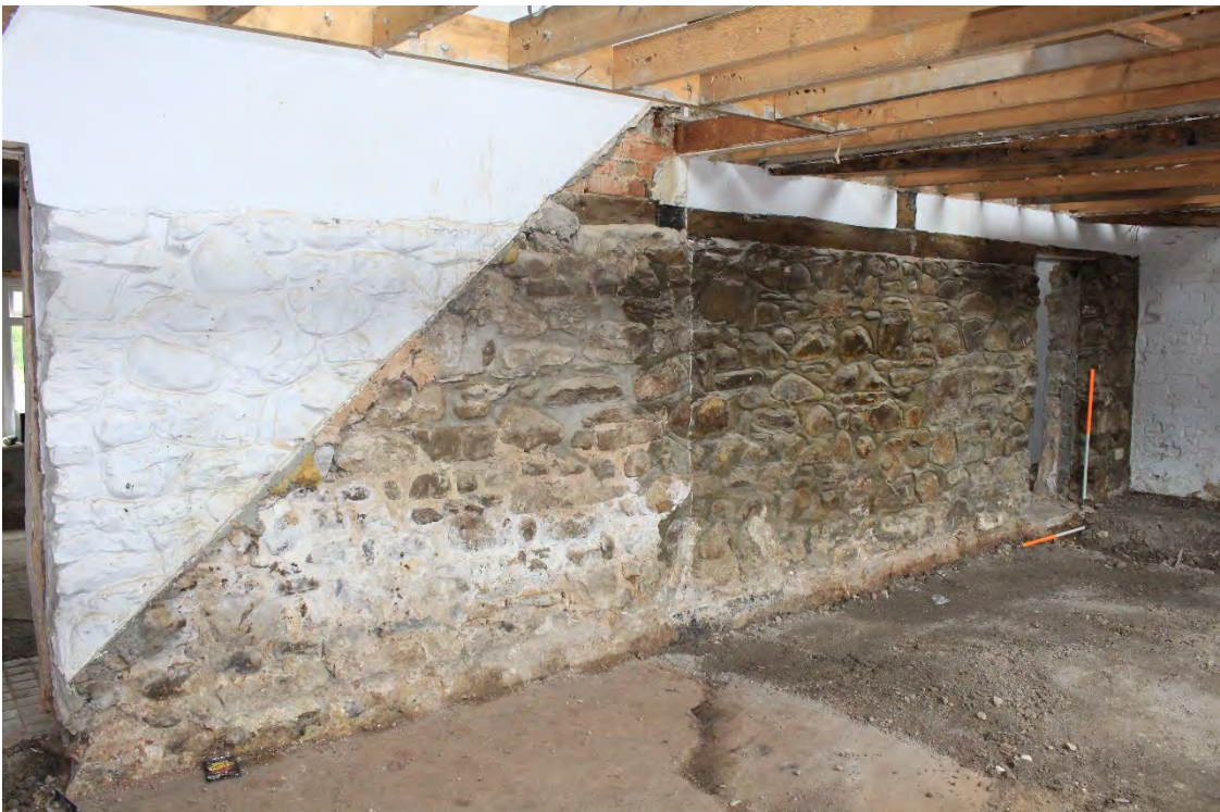
Image EDP A1.9: View of the eastern face of the main spine wall, showing stone below and timber frame above.
