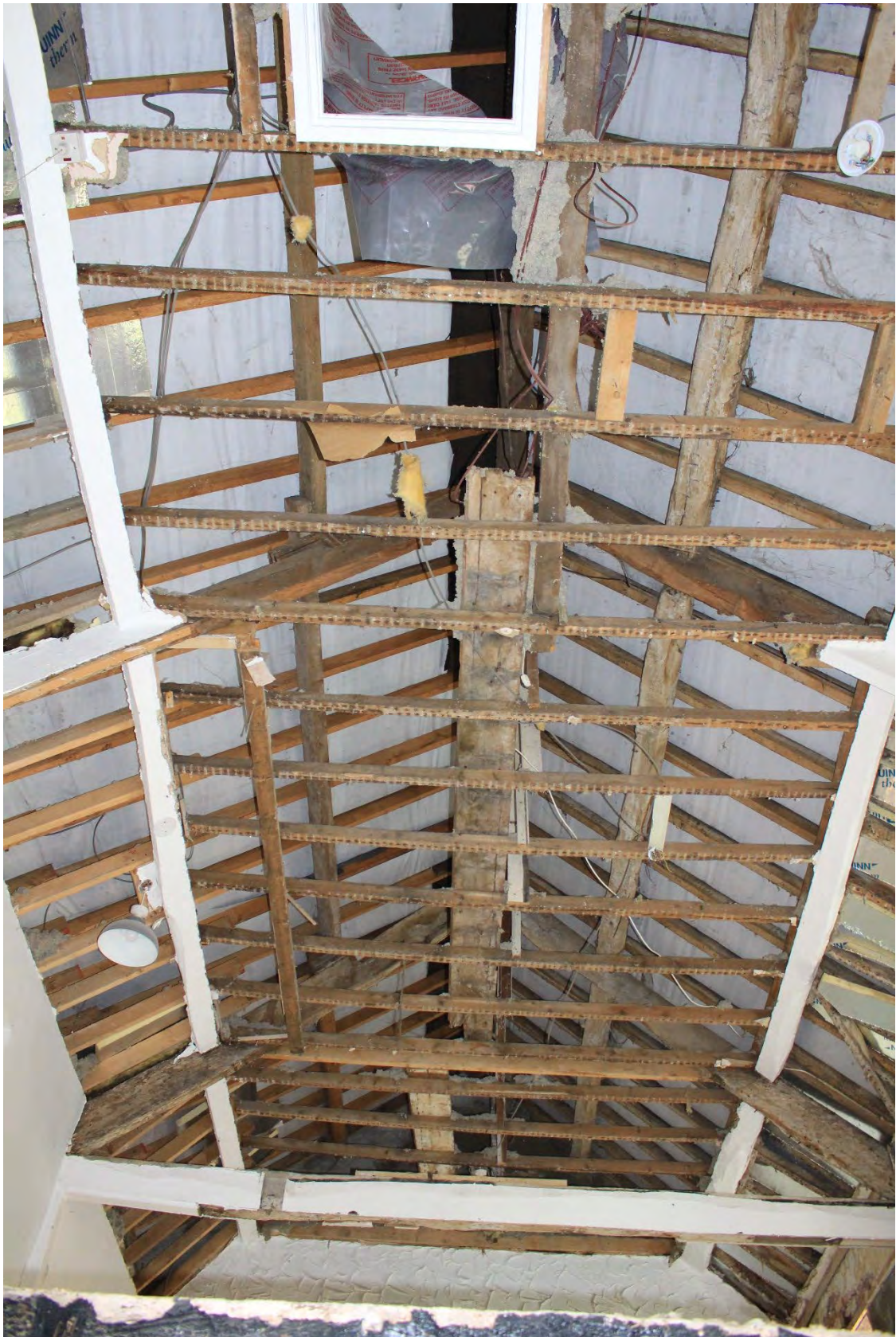
Image EDP A1.15: View of the roof structure of the main section, looking south. The east (left-hand) pitch has been completely replaced in the 20 th century.
