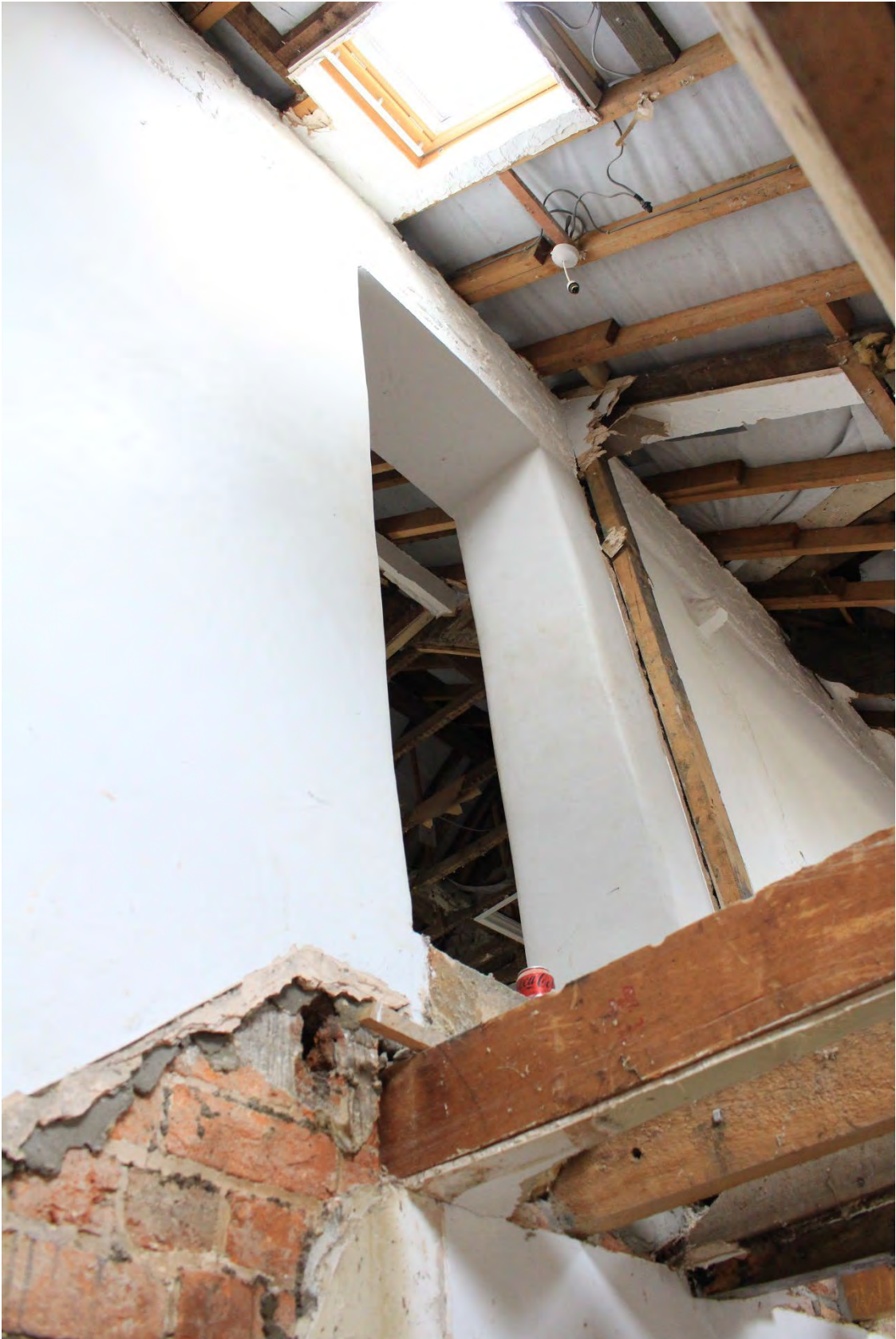
Image EDP A1.21: View of the door in the spine wall between the two upper rooms looking north-west. Also showing detail of the brickwork of the upper half of the spine wall.
