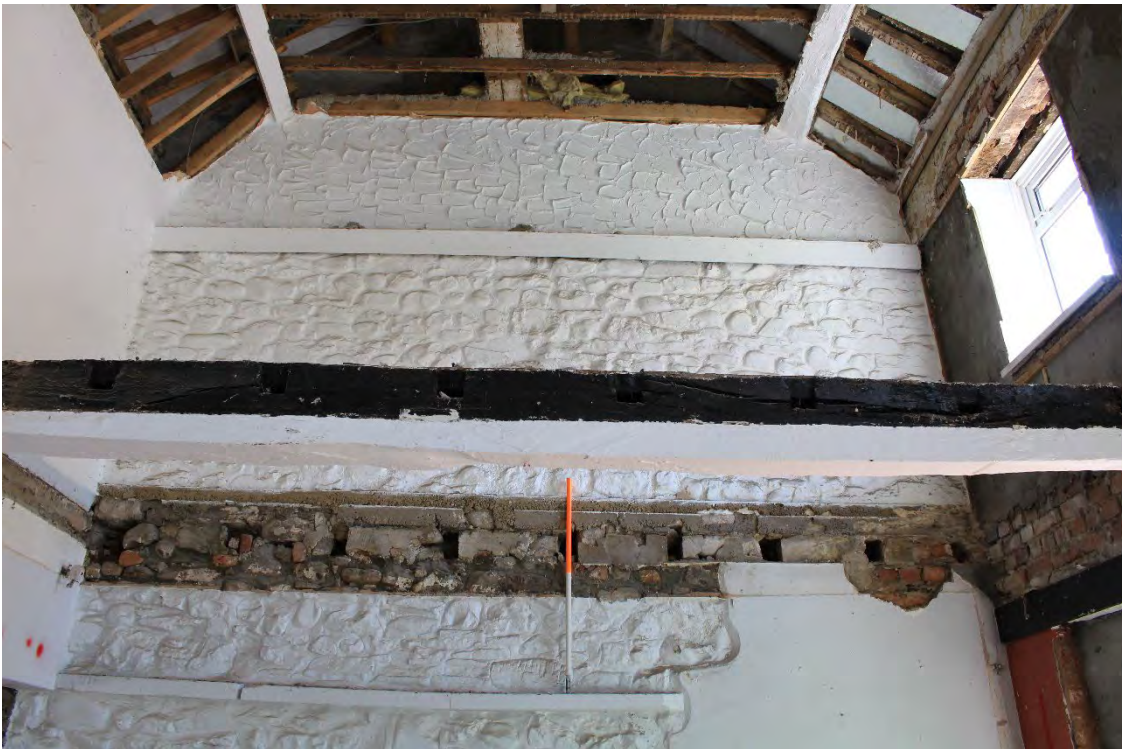
Image EDP A1.11: View of the Upper part of the southern gable in G1, showing the rendered upper portion most likely hiding brickwork, looking south.
