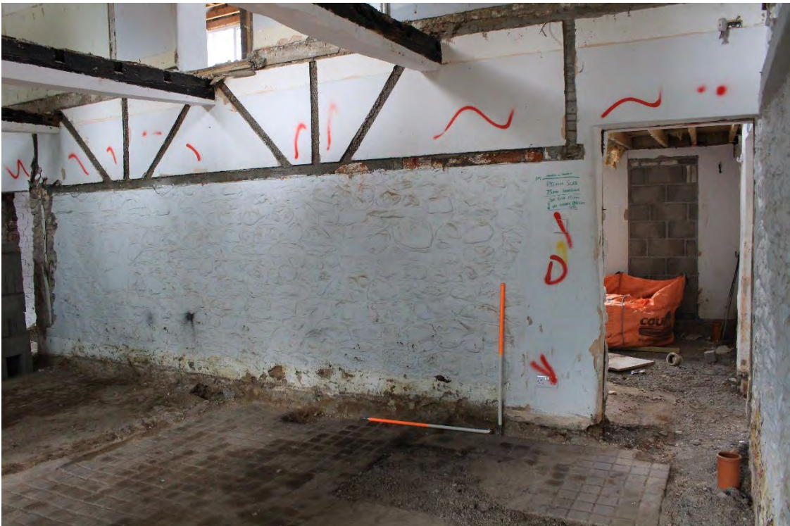
Image EDP A1.3: View of the stone spine wall dividing G1 and G2, with brick on the upper part of the wall.
