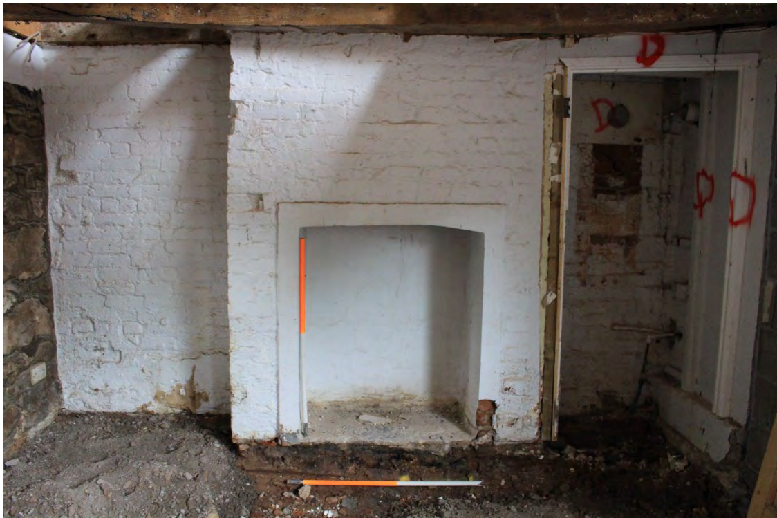
Image EDP A1.17: View of the fireplace and adjacent cupboard in the northern elevation of G2, looking north.
