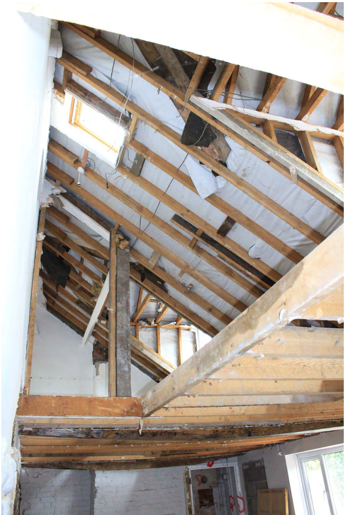
Image EDP A1.22: View into the upper floor above G2 looking north, showing the completely 20 th century floor and roof structure.
