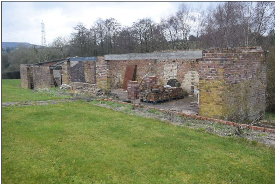
Fig. 5 Outbuilding viewed from the north-east showing the large later opening in the east elevation Photo CPAT 5040_006
