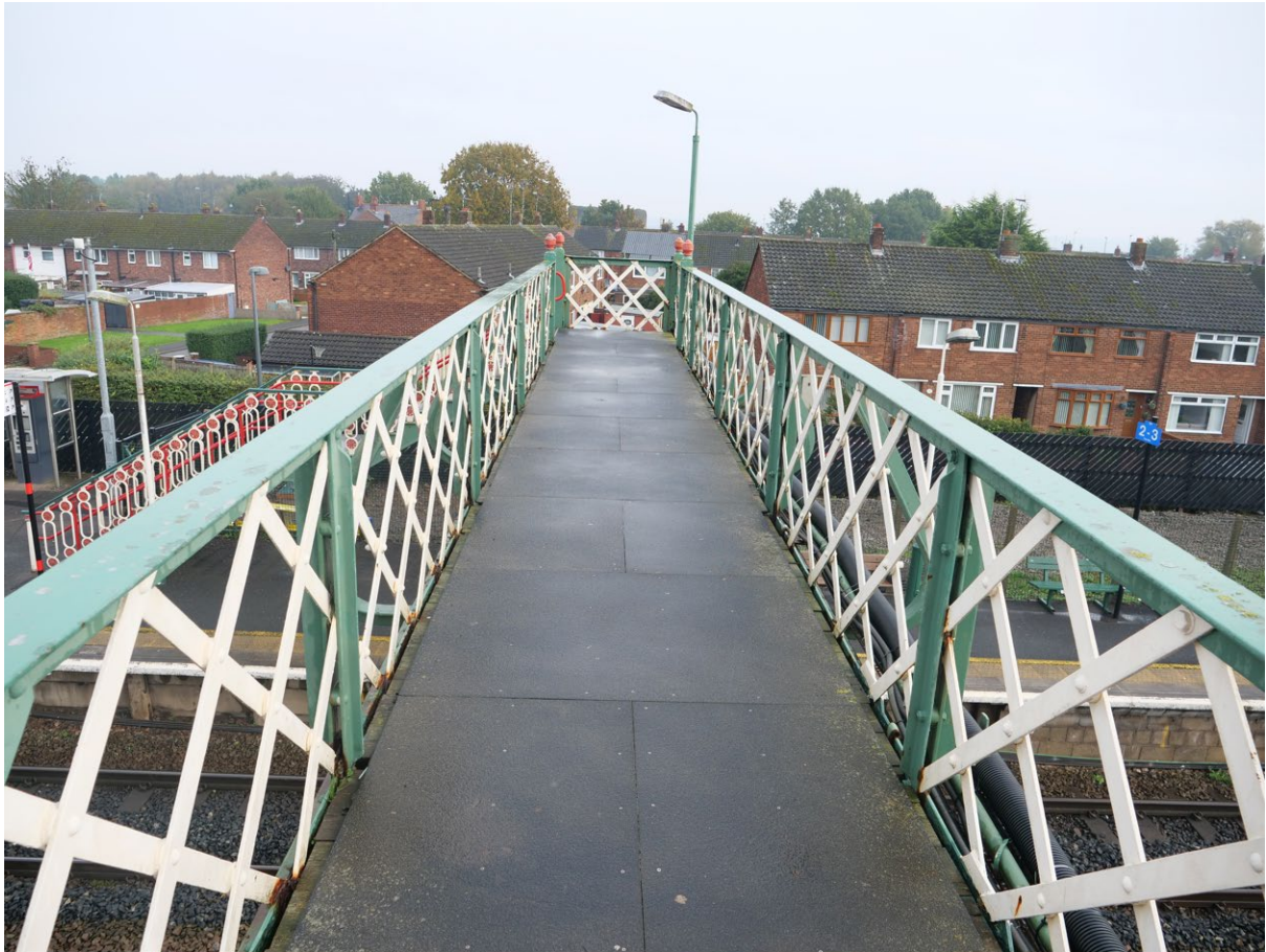
Plate 12: Another view of the deck, looking northeast, showing modern services carried along the south side of the footbridge
