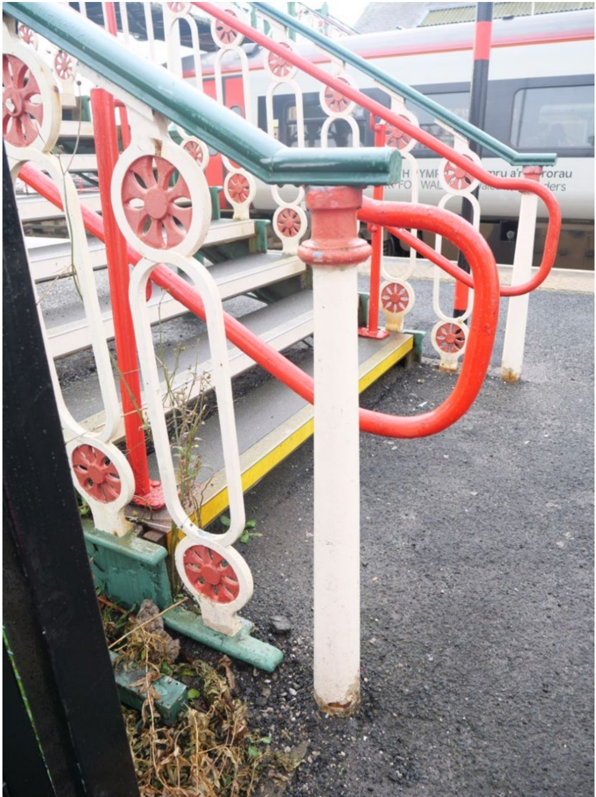
Plate 23: Cast iron newel post and balusters at foot of northeast staircase (Platform 1), looking south
