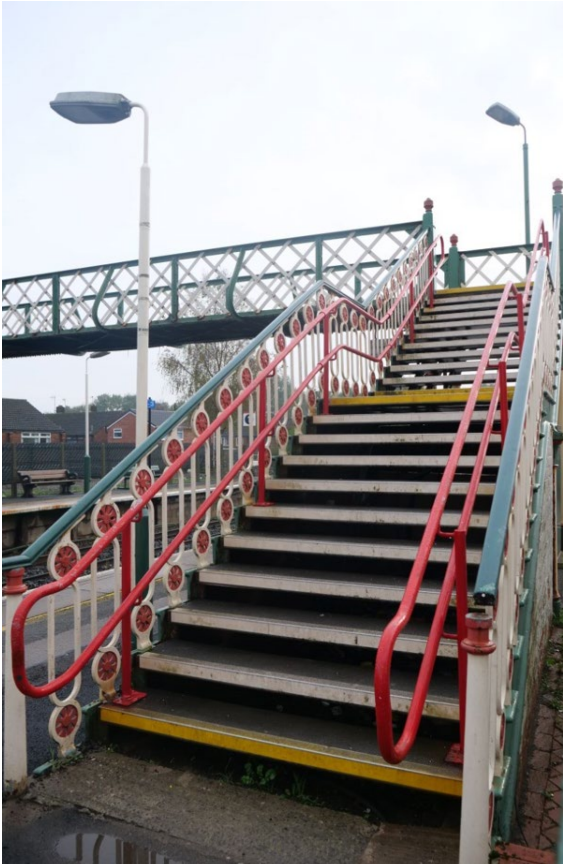
Plate 24: View of southwest staircase (Platform 2), showing method of attachment of modern safety handrails to steps, looking southeast
