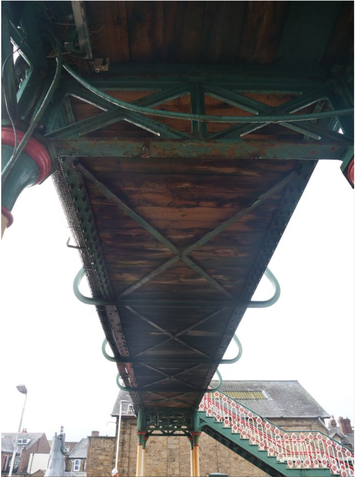
Plate 10: The underside of the bridge deck, showing longitudinal girders and diagonal braces, looking southwest from Platform 1
