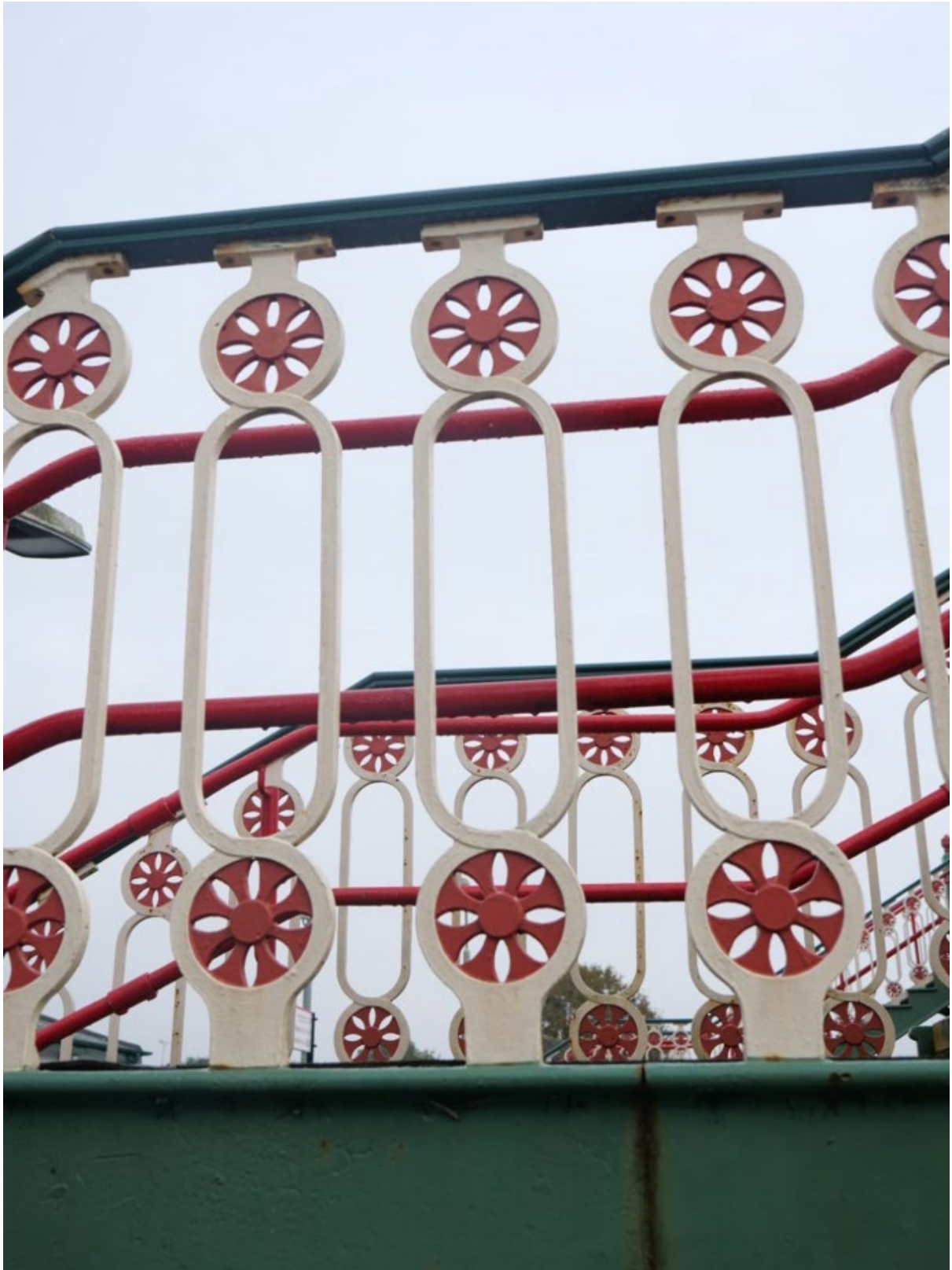
Plate 22: Detail of decorated cast iron balusters on landing of southwest staircase (Platform 2), looking northeast
