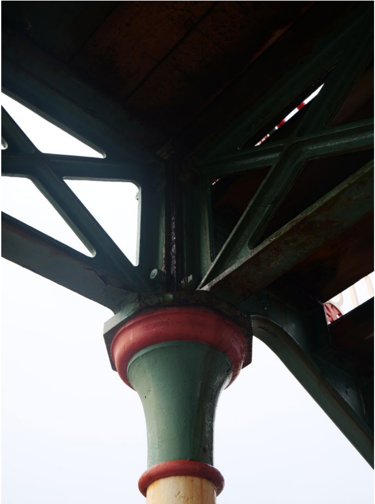
Plate 8: Detail view of southwest bridge pier/tower (Platform 2), showing cross girders bolted into vertical iron stanchions
