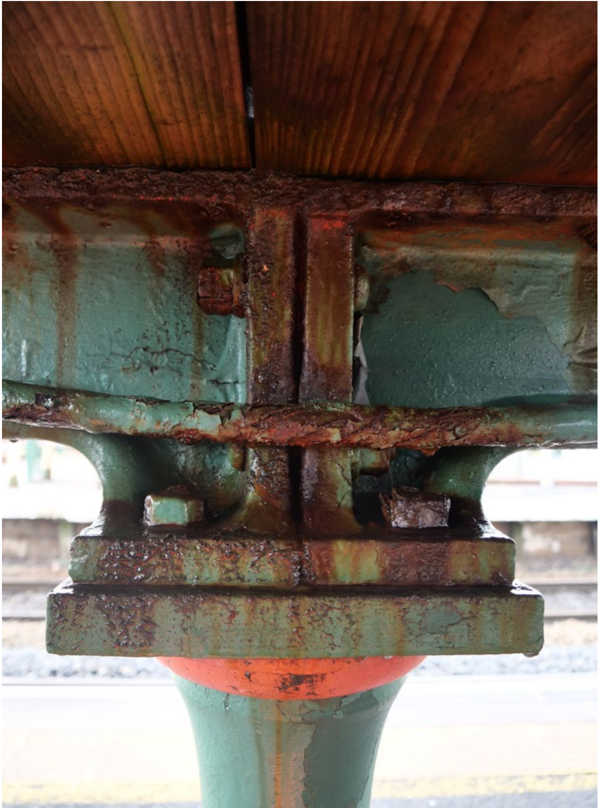
Plate 20: Expansion joint connecting upper and lower stringers on the northeast staircase (Platform 1), looking west
