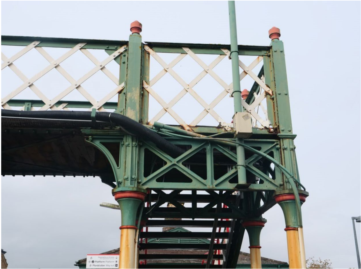
Plate 7: The northeast bridge pier/tower (Platform 1), showing cross girders and bracket supporting the bridge deck. Looking northwest
