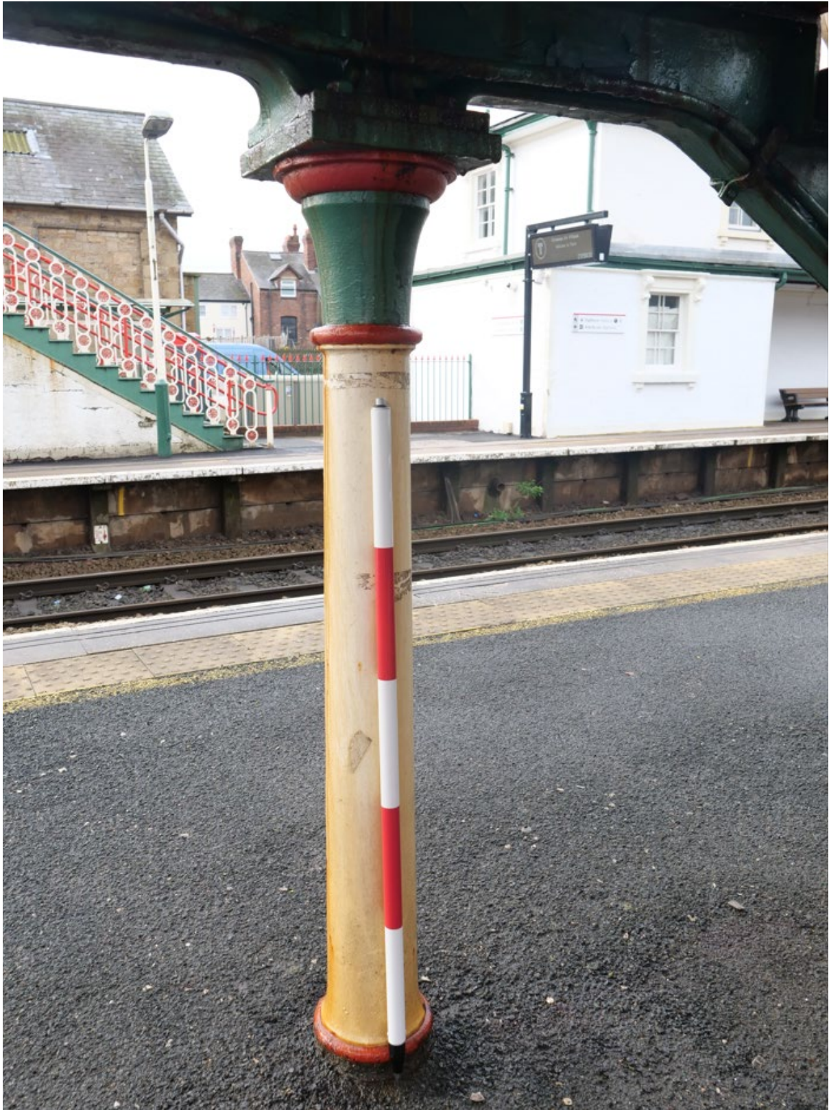
Plate 18: Cast iron column supporting the central landing of the northeast staircase (Platform 1), looking west
