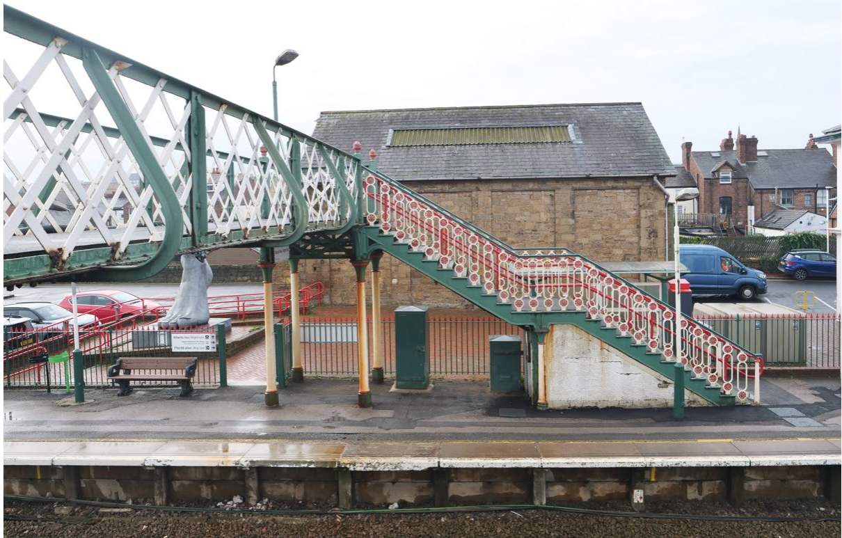
Plate 16: North elevation of footbridge, showing wind struts and southwest staircase (Platform 2), looking southwest
