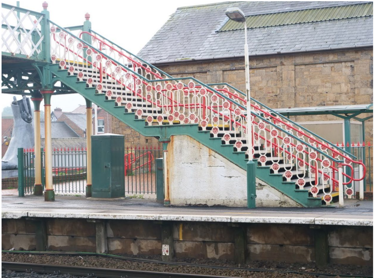
Plate 3: The southwest staircase, looking southwest from Platform 1. The former Goods Shed is in the background
