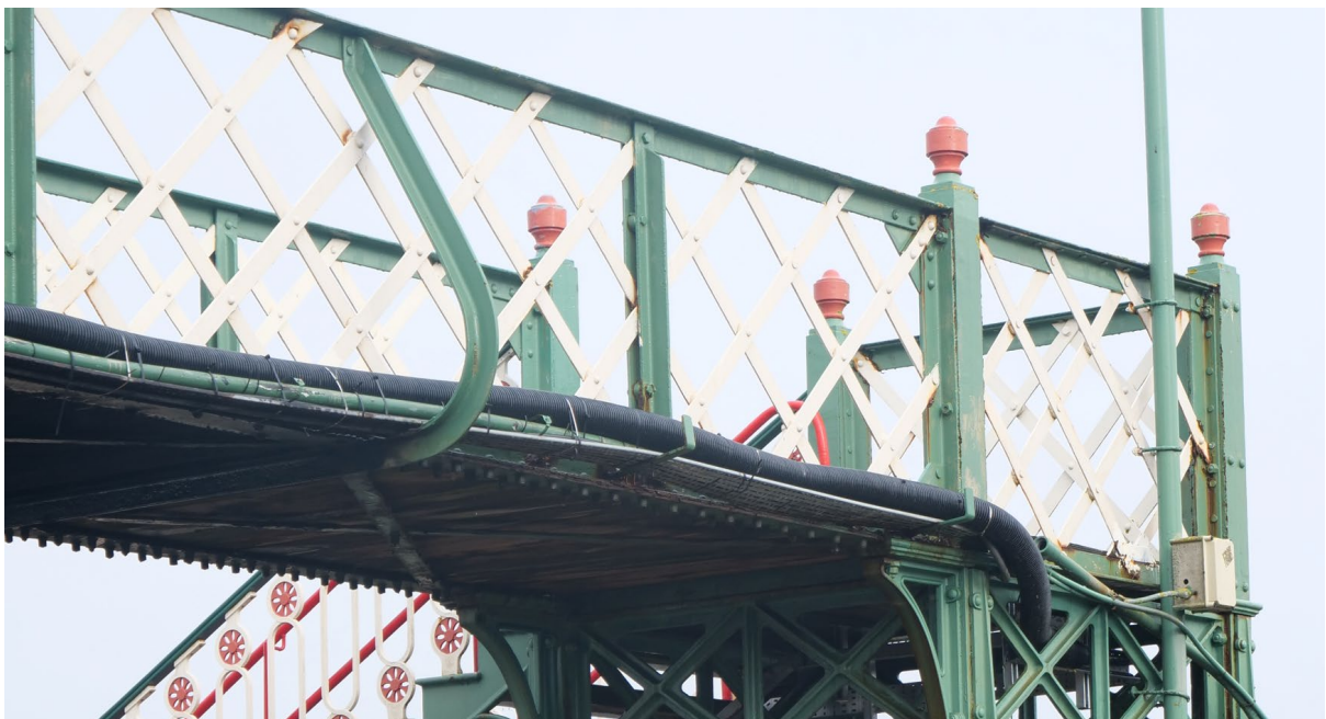
Plate 13: Detail view of south face of footbridge, showing wind strut (left) and attached brackets and pipes to carry services across the tracks, looking north from Platform 2
