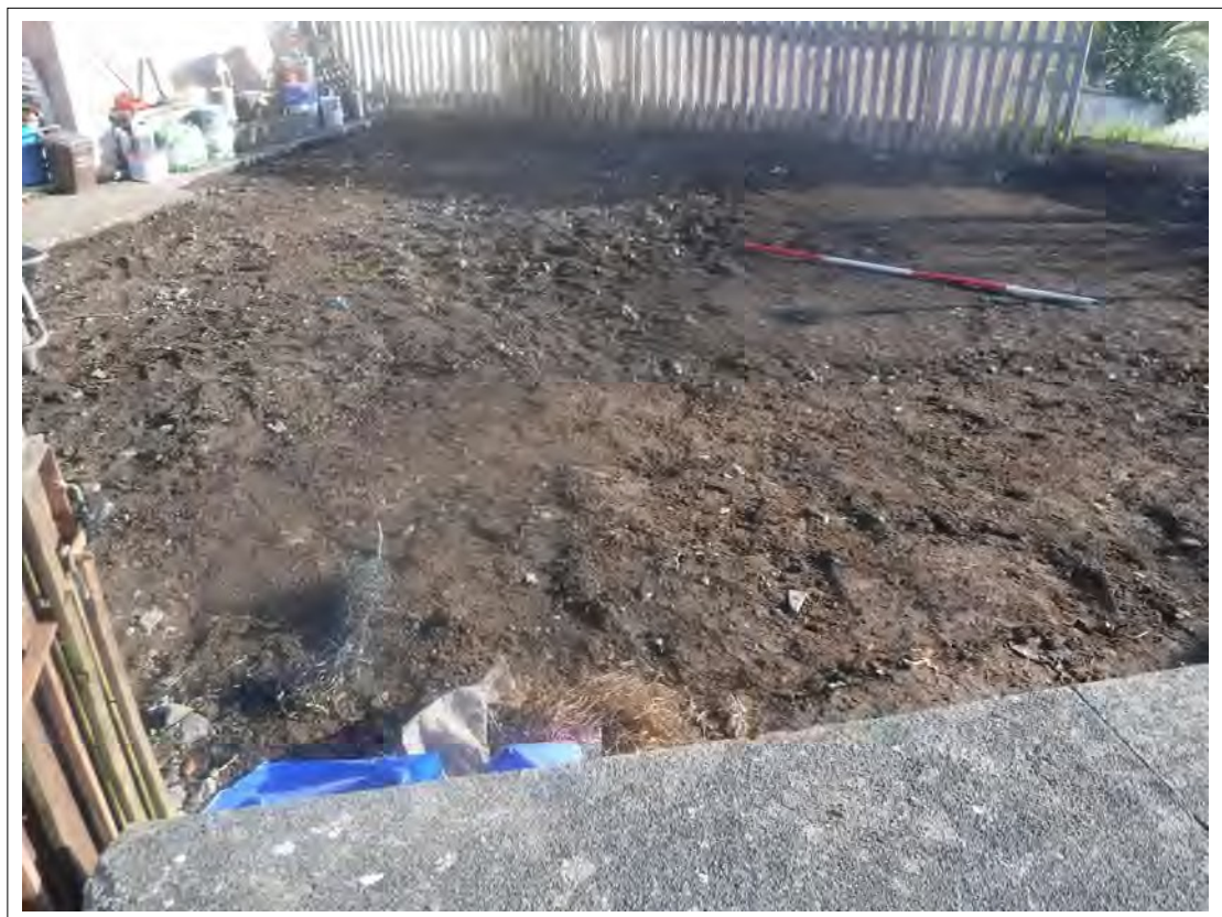
Plate 26. Deposit of silty loam mixed with cobbles (103/004) viewed from the north-east. Scale 2m
