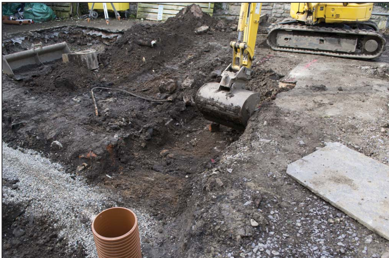
Plate 45: View from northeast of foundation trench (northern end) detailing modern drainage cut; scale not used; view from SE (archive reference: G2766_096).
