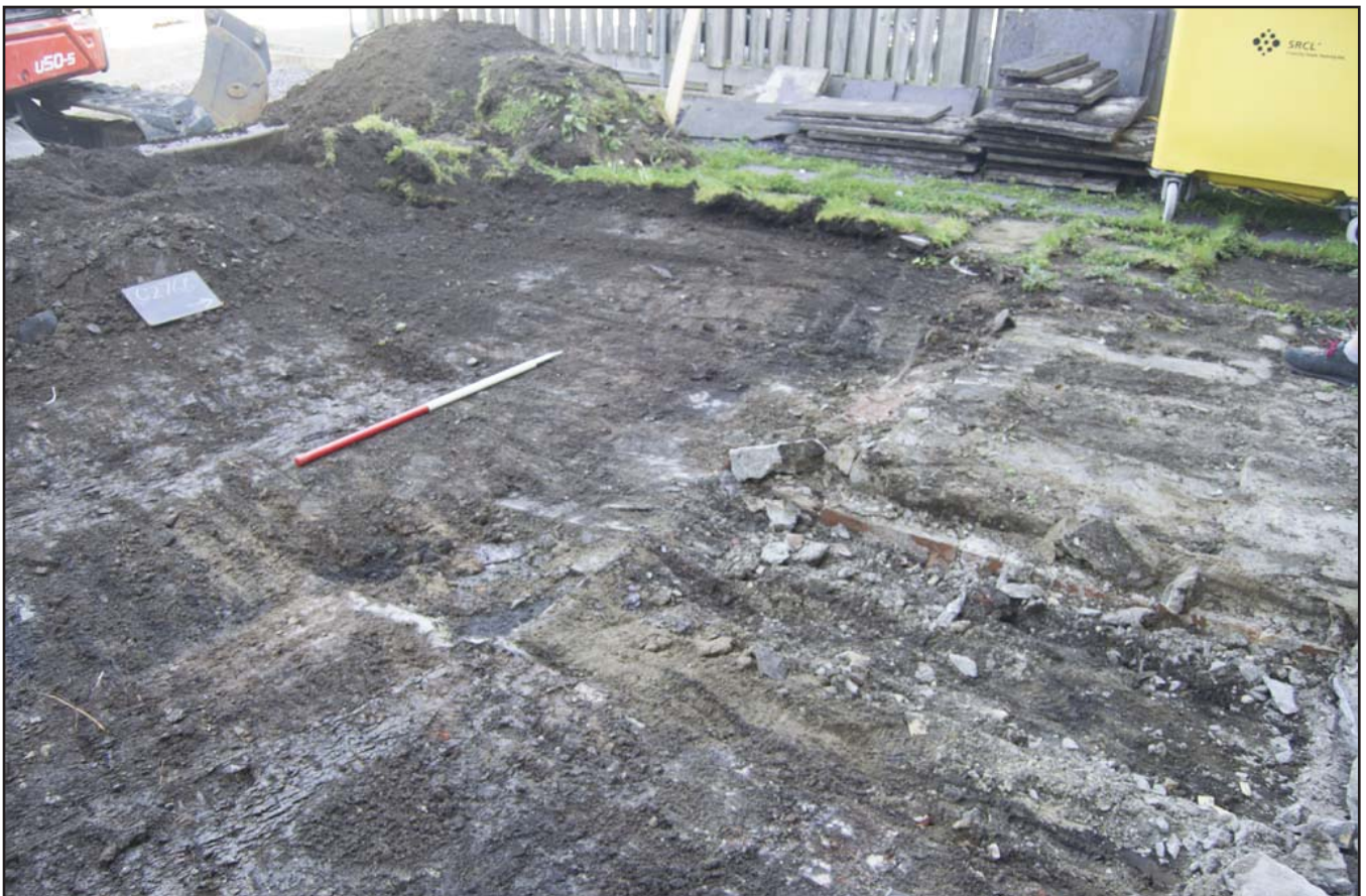
Plate 4: Stripped area with concrete pad and bricks in the NE of extension area (mid-excavation); scale 1x1m; view from SE (archive reference: G2766_004).
