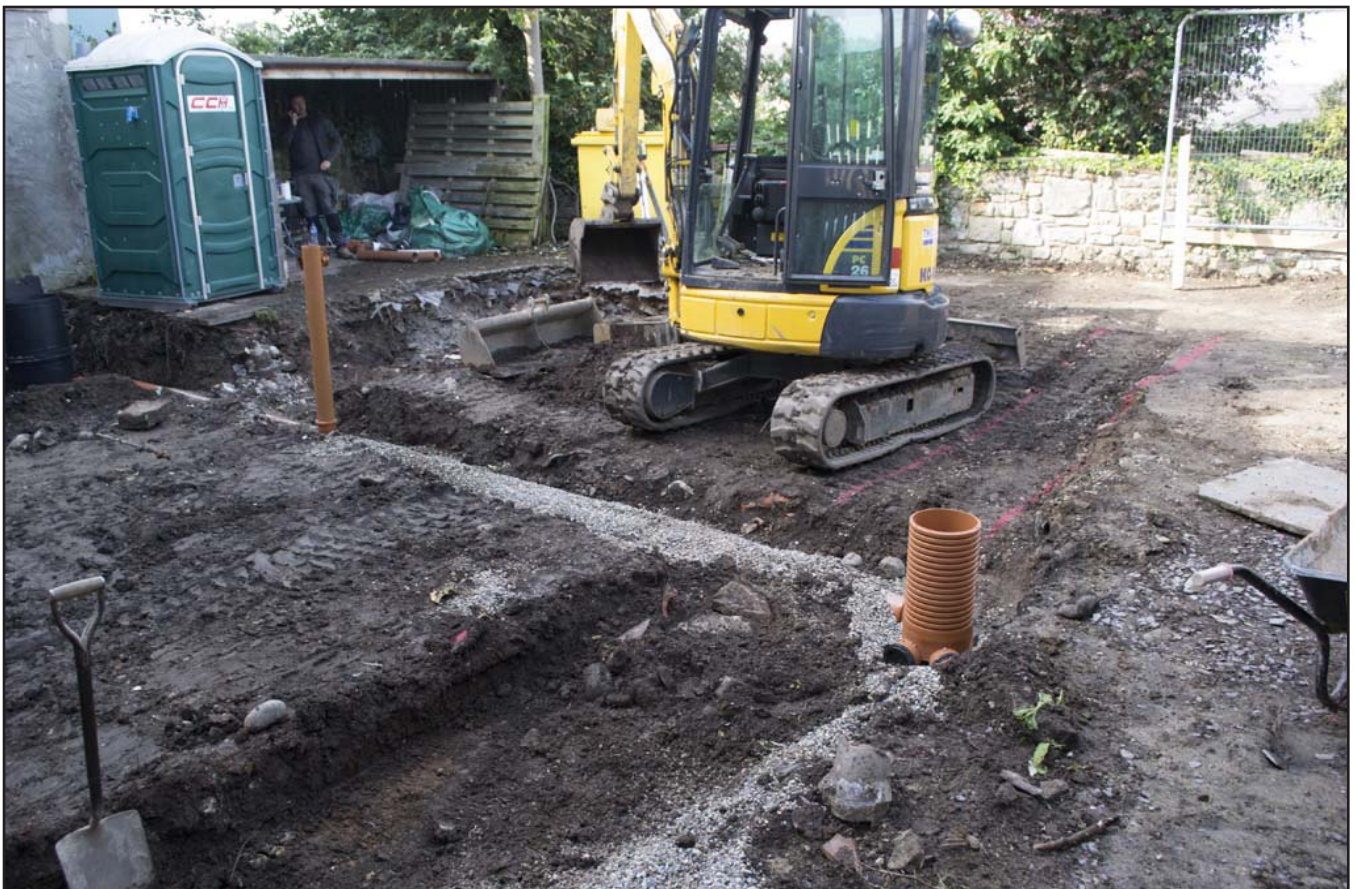
Plate 44: View from northeast of foundation trench (northern end) showing in-situ irregular shaped stones; not structural; scale not used; view from NE (archive reference: G2766_093).
