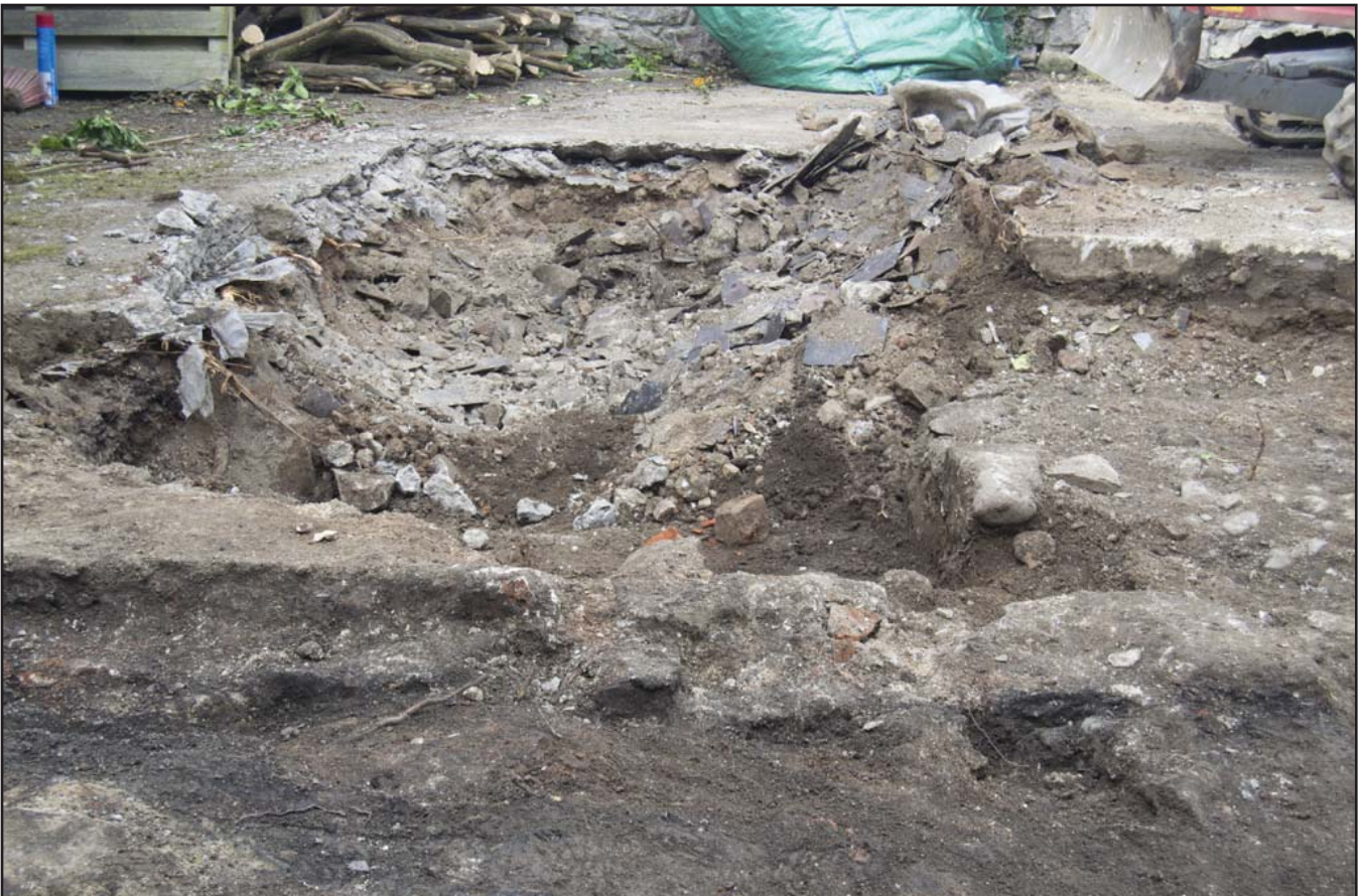
Plate 12: Working shot of removal of demolition debris to west end of extension area; scale not used; view from NE (archive reference: G2766_018).
