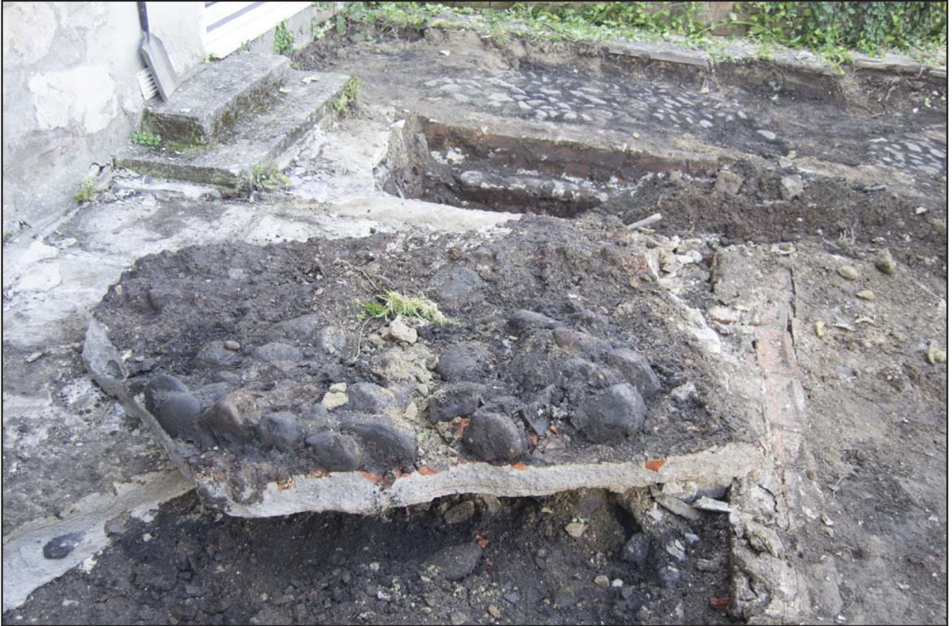
Plate 9: Shot of yard cobbles attached to the underside of removed concrete pad; scale not used; view from N/A (archive reference: G2766_012).
