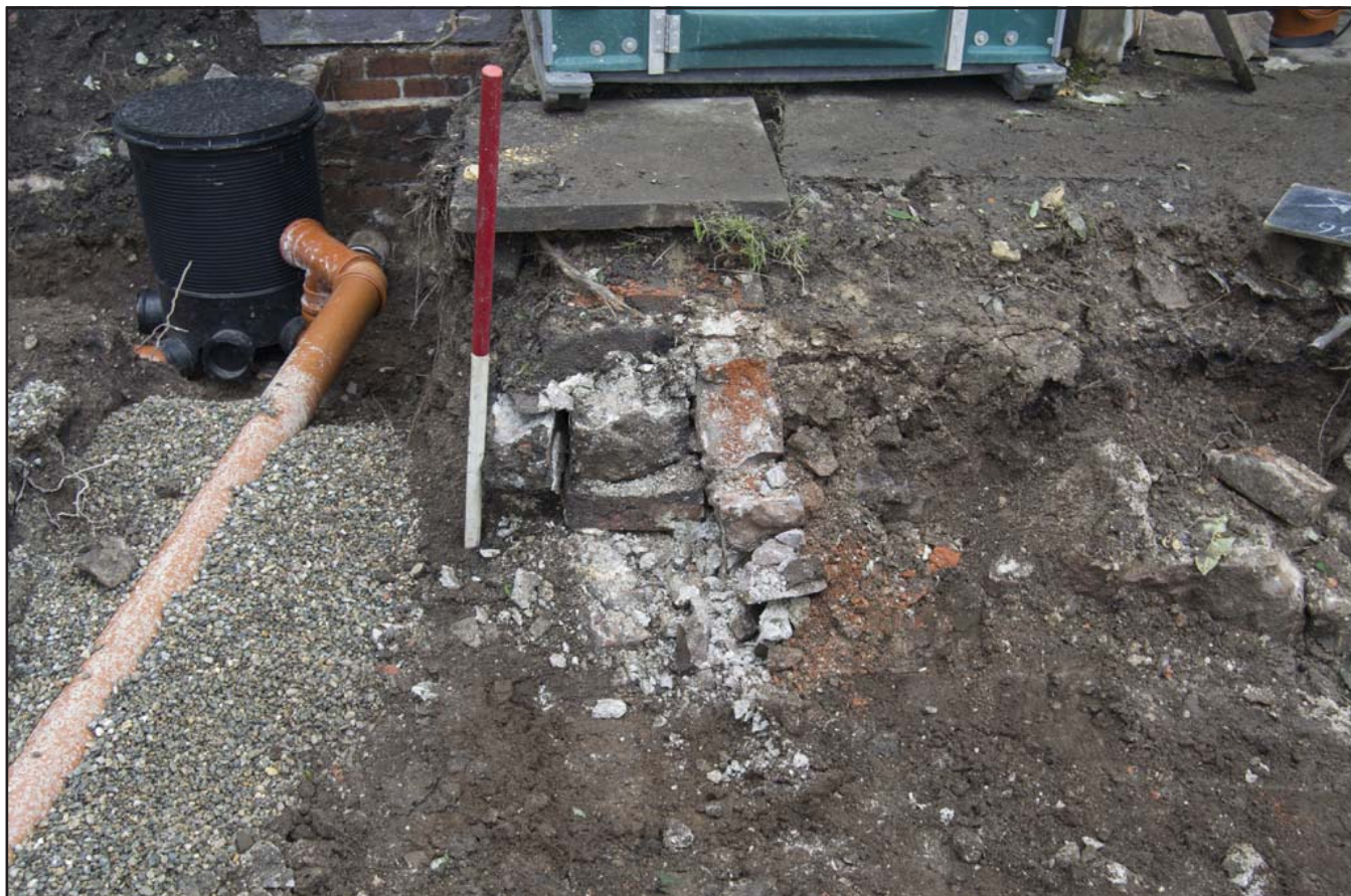
Plate 41: North facing elevation of 106 partially removed; scale 1x1m; view from N (archive reference: G2766_084).
