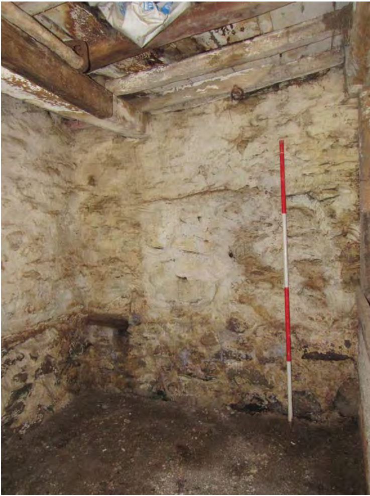
Plate 45. Interior of Room 3 of main range, possible blocked window, SW corner, view SW. 2m scale
