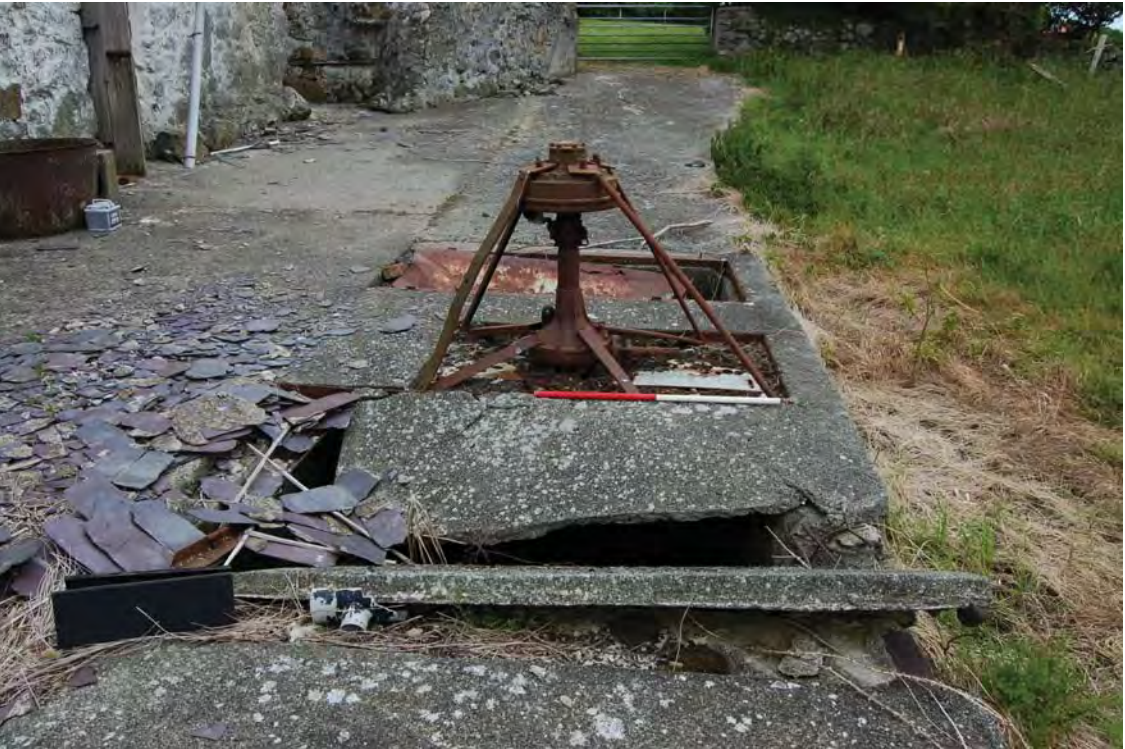
Plate 26. Industrial remains in yard to E of main range, iron tank, view NW. 1m scale
