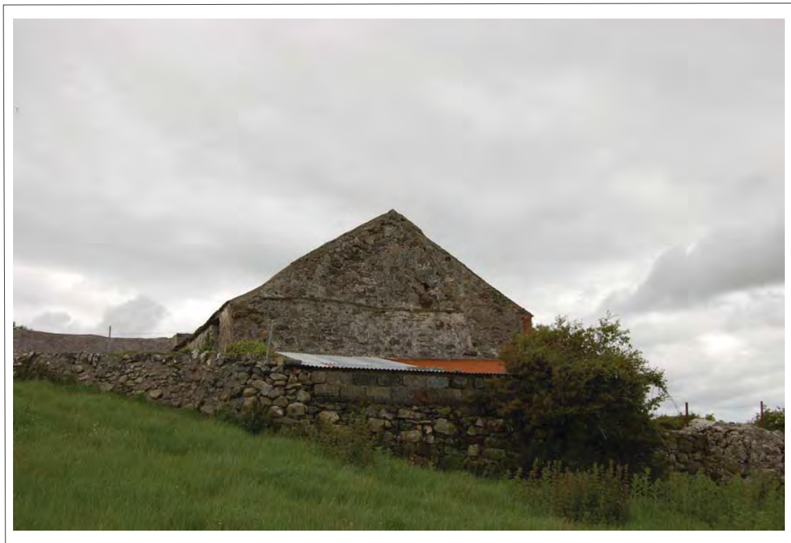
Plate 69. Main Range SE gable end, with boundary wall and extension. View NW
