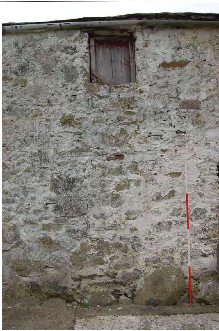
Plate 21. Main Range SE end hatch and blocked window, view SW. 2m scale
