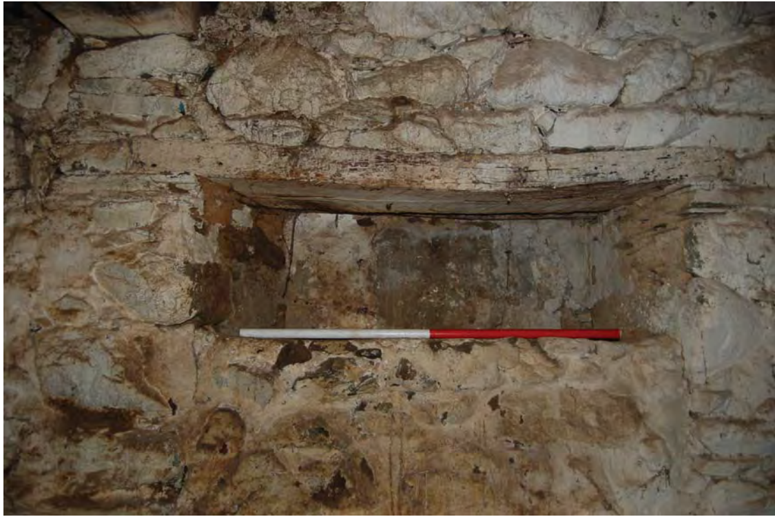
Plate 33. Interior of Room 2 of main range, filled window, view NE. 1m scale
