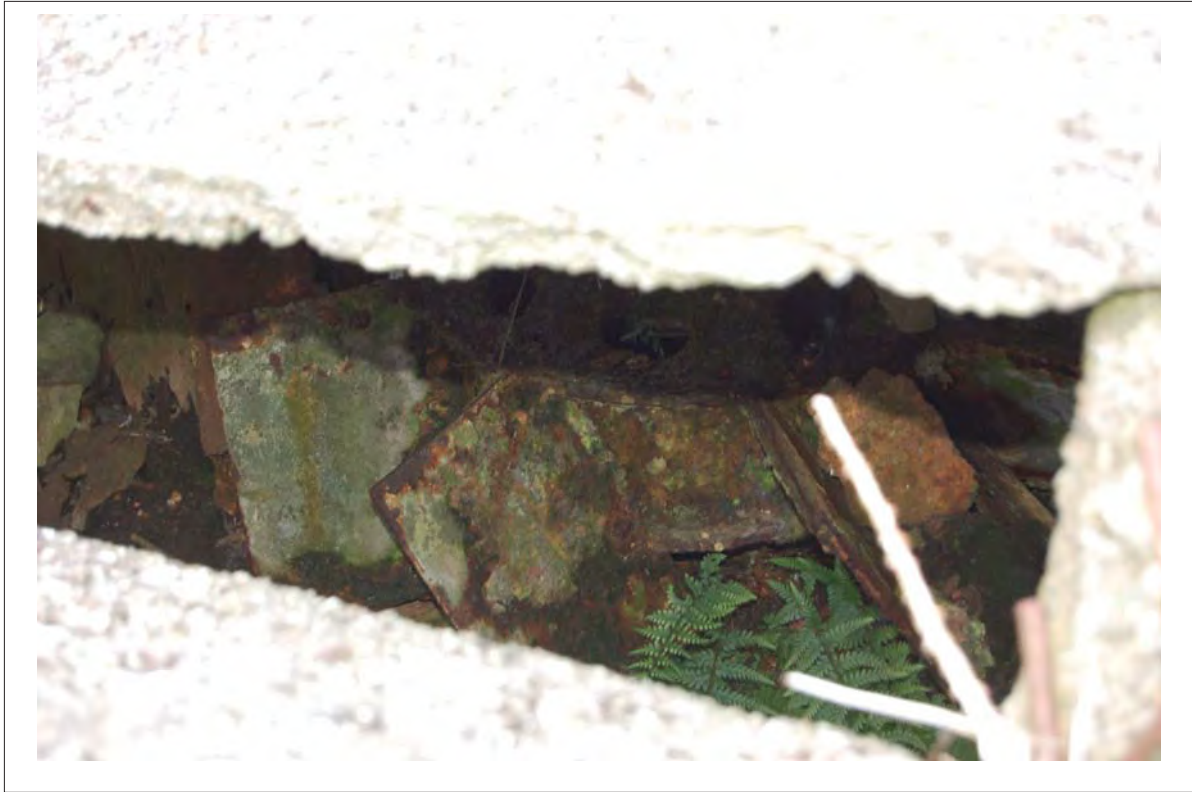
Plate 27. Industrial remains in yard to E of main range, flywheel in tank, view NW.
