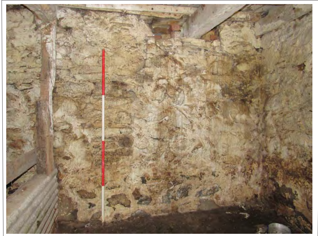
Plate 46. Room 3 of main range, possible blocked window, NW corner, view SW. 2m scale
