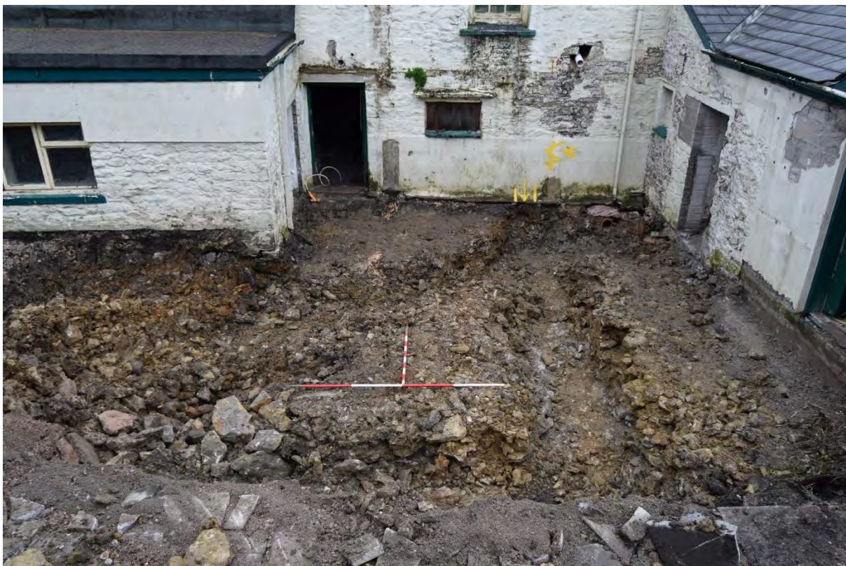
Plate 20: Phase 3 exterior (rear), showing the area subsequent to excavations, revealing the fragmented bedrock (202) throughout. View south, 2m & 1m scale.
