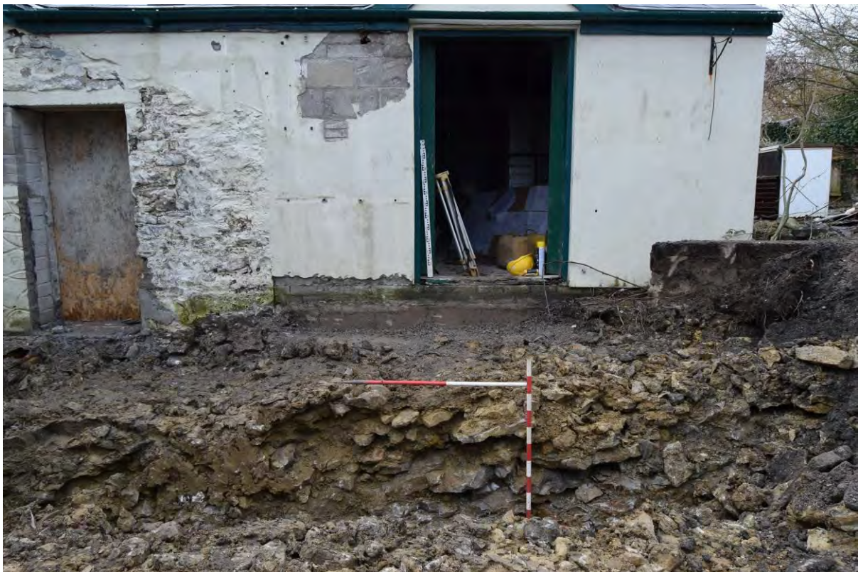
Plate 22: Phase 3 exterior (rear), showing representative section and relative levels of excavated area. View west, 1m scales.
