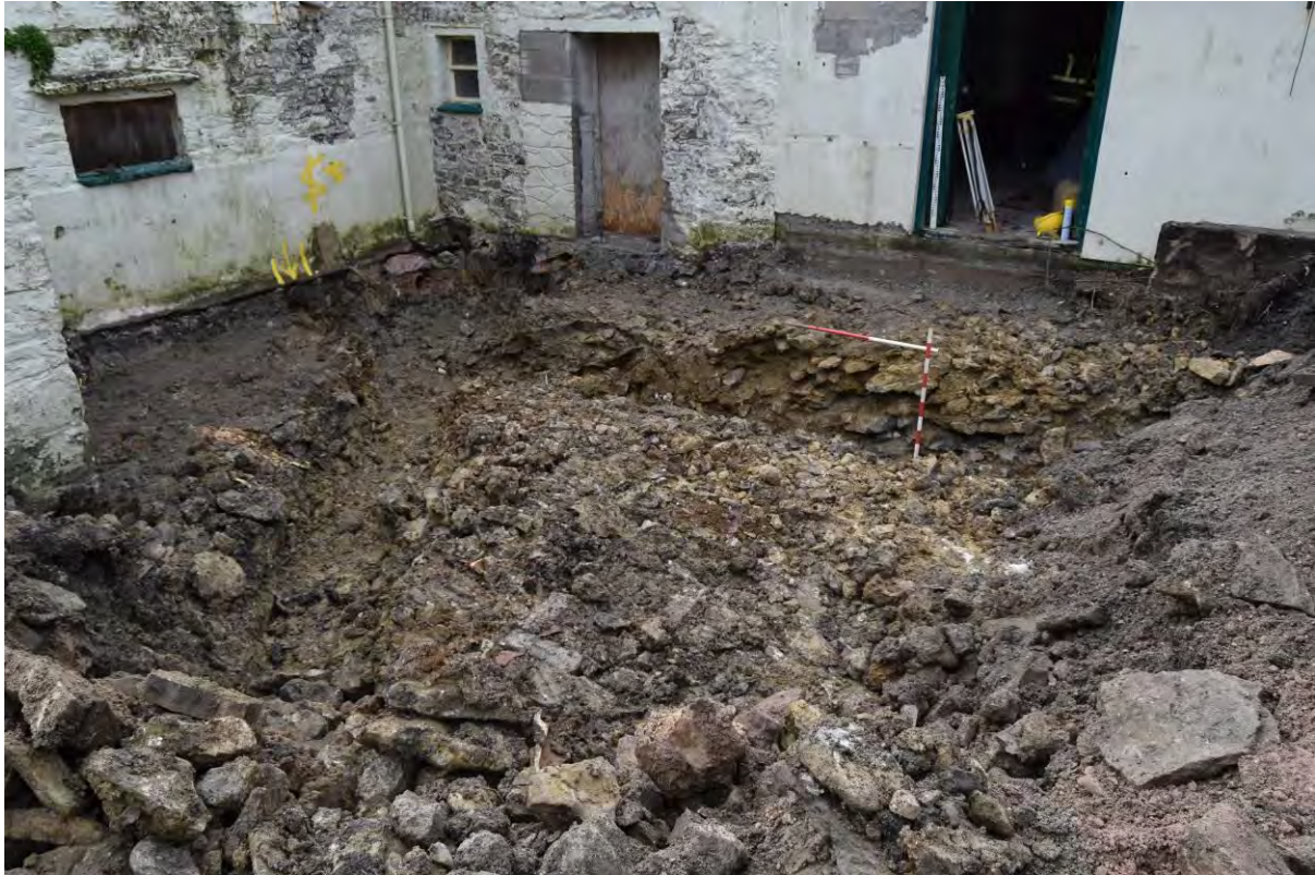
Plate 21: Phase 3 exterior (rear), showing the area during excavations, with fragmented bedrock (202) exposed throughout. View southwest, 1m scales.
