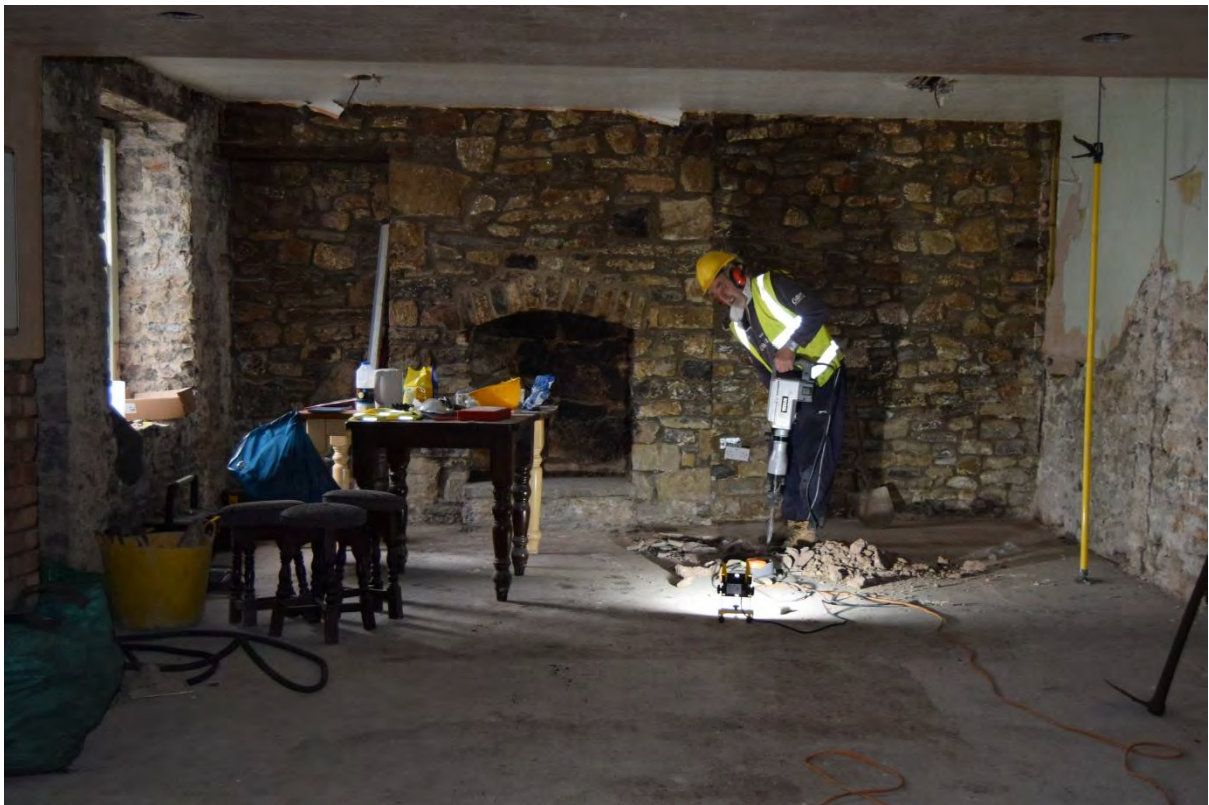
Plate 2: Phase 1 works within the building, showing excavation of test pits in progress and the fireplace against the western wall. Looking west.
