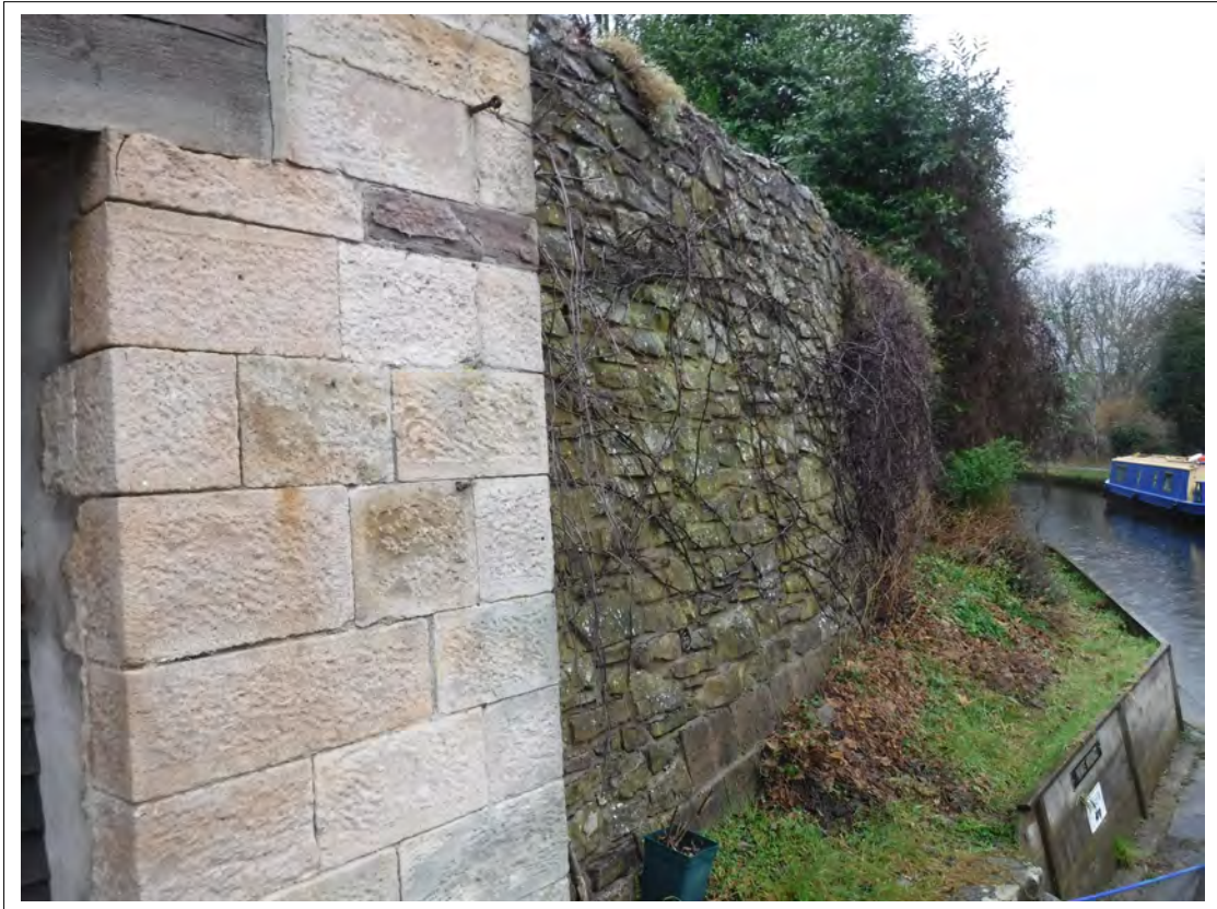
Plate 17. Retaining wall to the north of The Boathouse, looking north from the wharf
