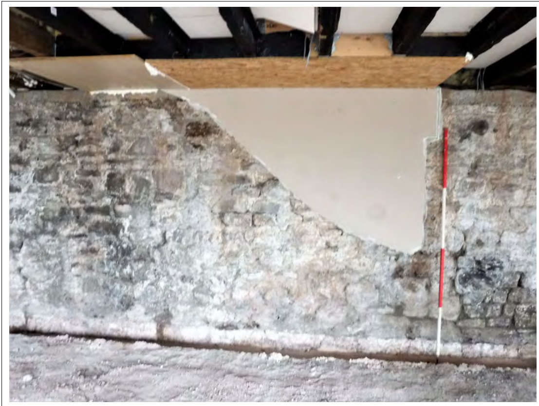
Plate 37. Plaster board on western wall where a modern staircase has been removed, looking west
