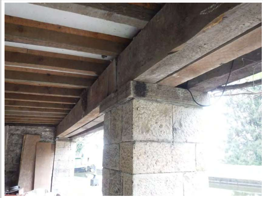
Plate 15. Detail of the top of a pillar showing modern mortar, looking north-east
