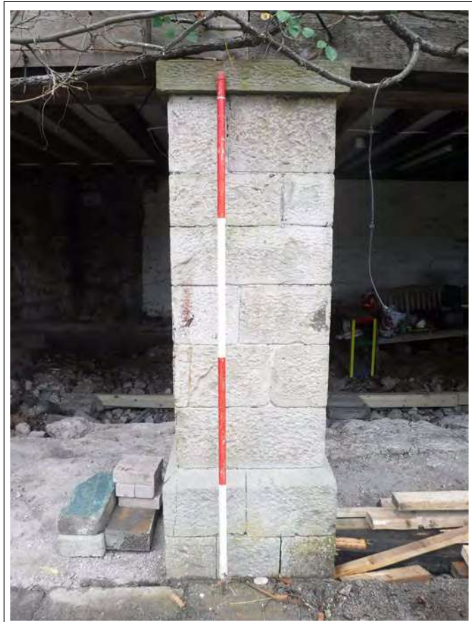
Plate 14. Limestone pillar to the north of the east elevation, looking west. Scale 2m
