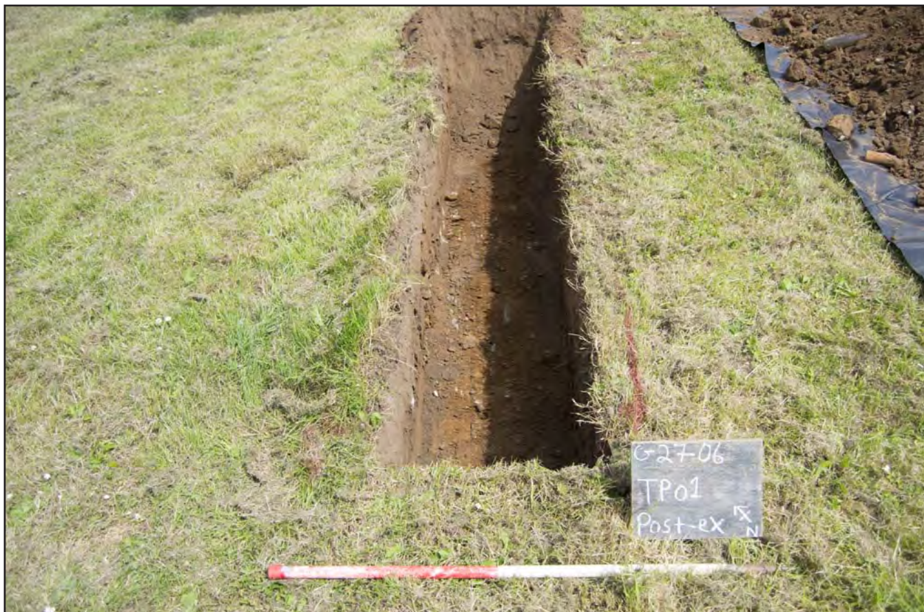
Plate 1: Post-excitation view of TP01 down to natural horizon; View from: SW; Scale: 1x1m (archive reference: G2706_002).
