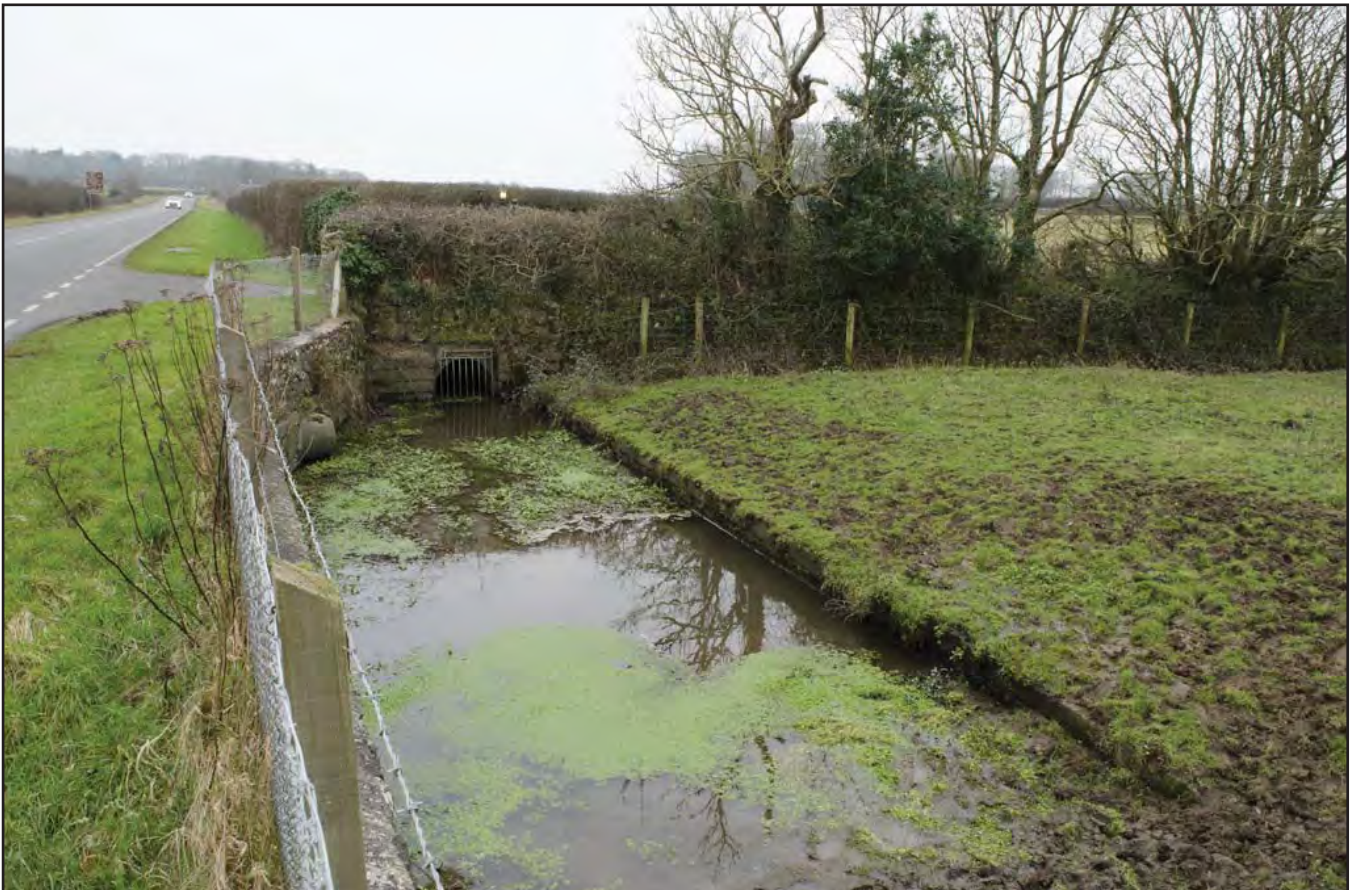
Plate 10: Culvert for Afon Rhyd y Valley at entrance to Maen Hir (archive reference: G2706_006).
