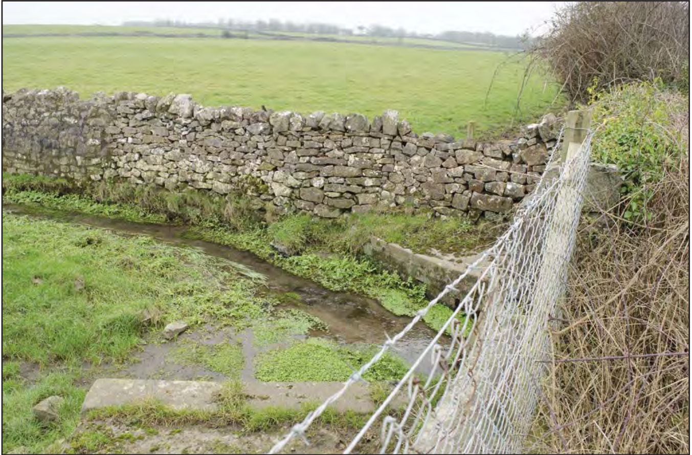
Plate 09: Culvert for Afon Rhyd y Valley as it passes beneath A4080 (archive reference: G2706_005).
