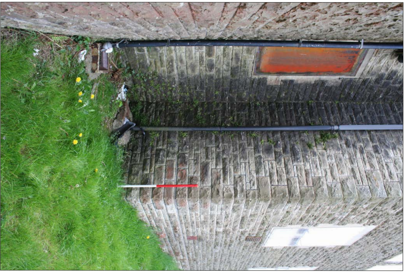
Plate 35. Window to SE-facing elevation connecting section to rear projecting element, looking W
