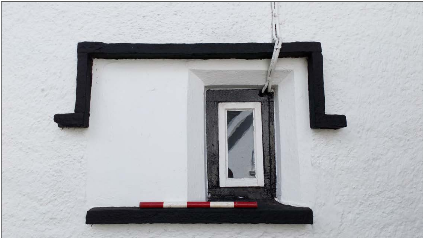
Plate 6. Detail of window alteration.
