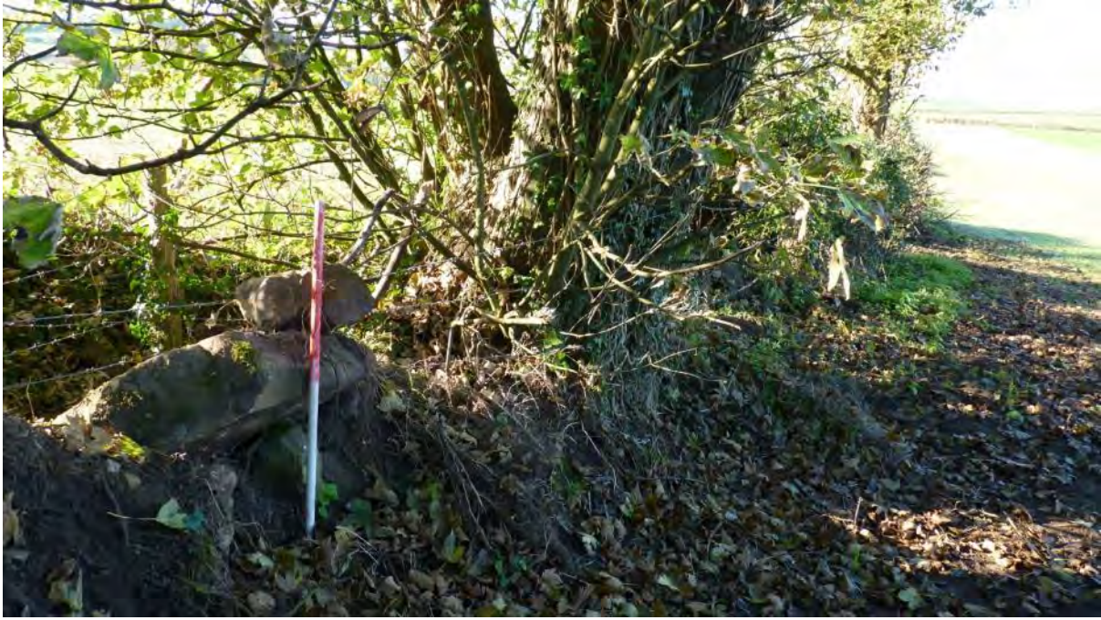
Photo 5: the southern field boundary of A1, comprising largely hedgerow with post-and-wire fencing, but in the SE corner incorporating the remains of stone walling. 1m scale. Looking SW.
