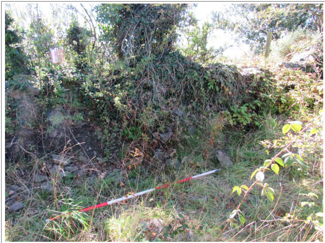
Plate 21. Southern dry stone boundary wall with scar of a wall return. View SW. 2m scale.
