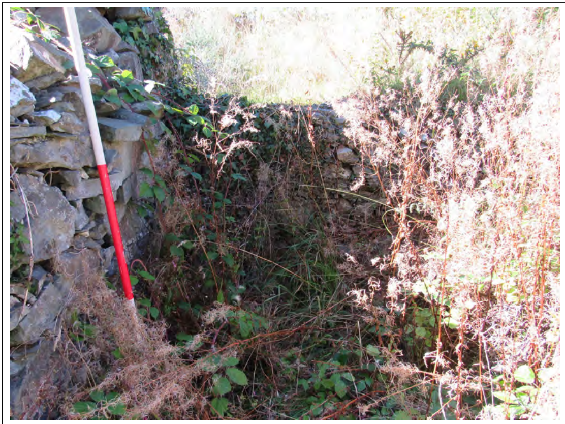
Plate 9. Join of northern wall of house ruins and western boundary wall. View W. 2m scale.
