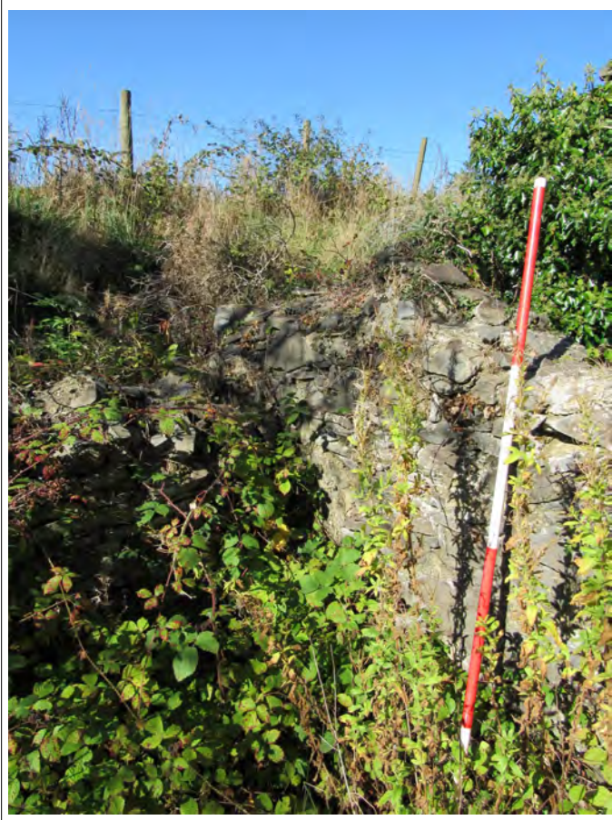
Plate 7. Join of southern wall of house ruins and western boundary wall. View NW. 2m scale.
