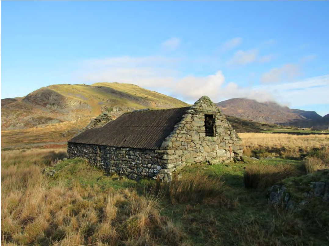
Photo 21: View of barn HW03, with blocked doorway visible in the side wall, and missing roof sections to the north. View northeast. 1m scale.
