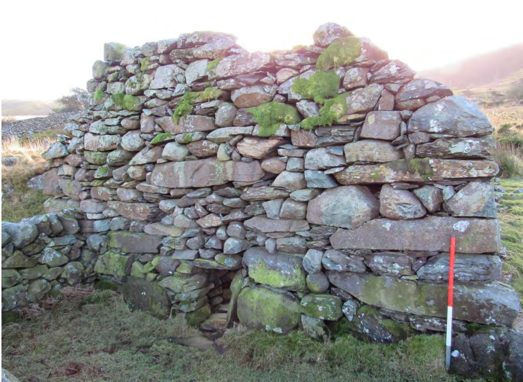
Photo 16: External face of northern gable wall of Cow Barn HW02. The central blocked doorway and sheep access visible. View south. 1m scale.
