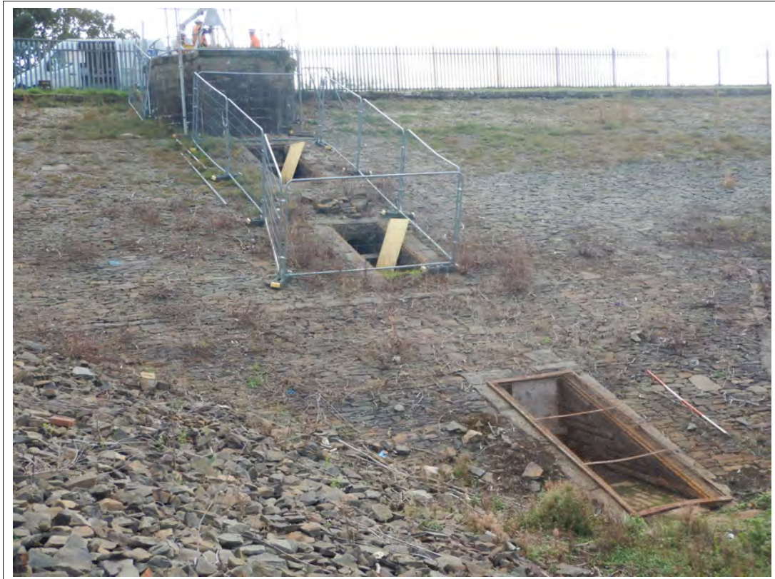
Plate 15. The outflow control valve platform and associated inlets below, looking south-west. Scale 2m.
