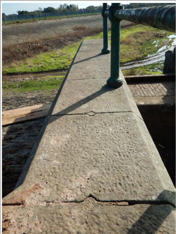
Plate 68. Coping stones on the top of the Inlet Gauge Chamber walls, showing the mortar plug joints and cast iron fence.
