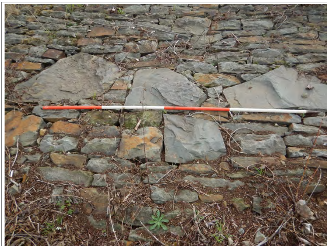
Plate 6. Detail of the interior of the pitched stone embankment, showing several unusually large stones which appear to be more recent additions. Scale 2m.
