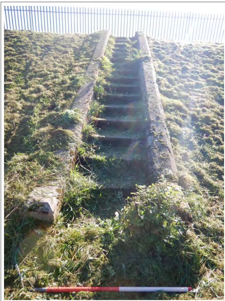
Plate 54. Concrete steps on western side of the reservoir, looking east. Scale 1m.
