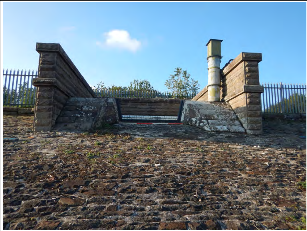
Plate 39. Cipoletti Weir, taken from the interior of the reservoir, looking west. Scale 2m
