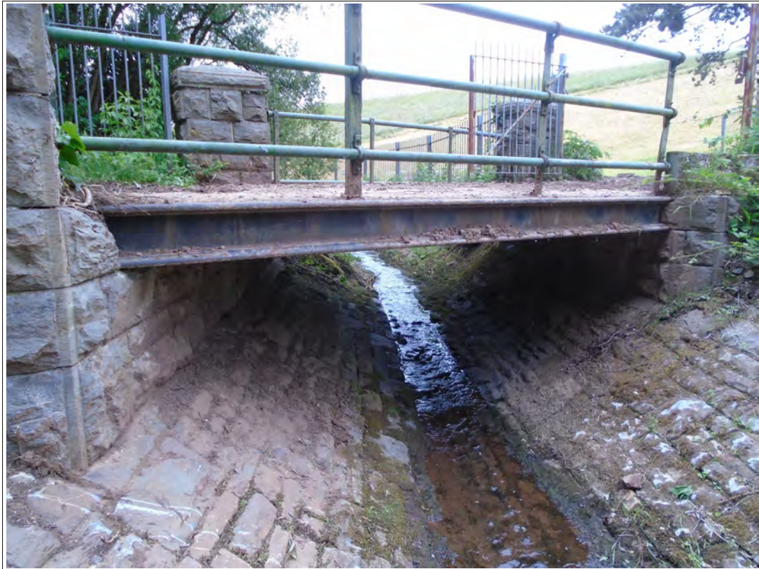
Plate 27. 'SEMD' bridge showing the cast iron edge beam resting on the stone abutments, looking north-west.
