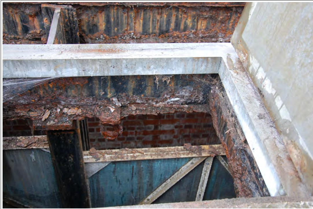
Plate 51. Interior of the screening chamber from an access hatch, showing an iron hook attached below the hatch.
