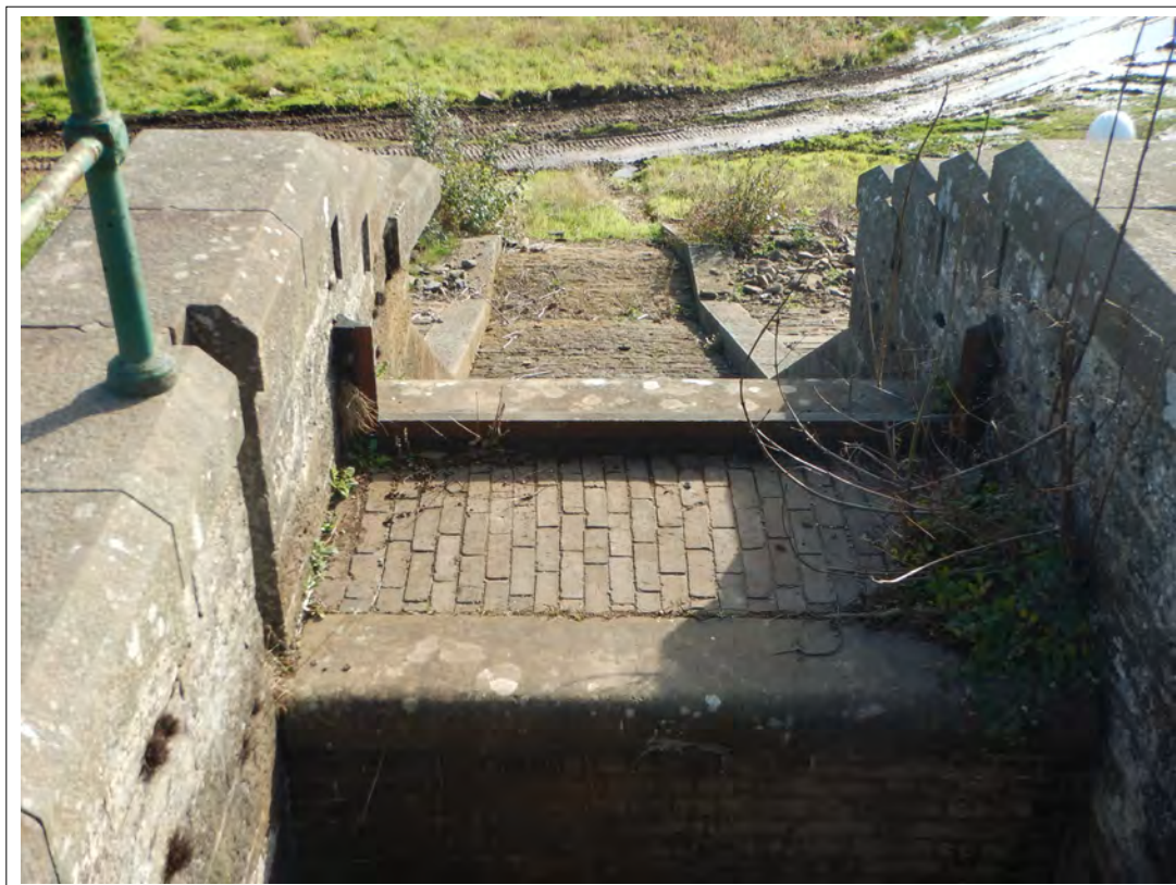
Plate 70. South-east wall of the Inlet Gauge Chamber, looking south-east down the outlet flow channel into the reservoir.
