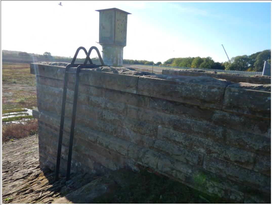
Plate 47. Northern exterior wall of the Cipoletti Weir showing the water meter case and ladder, looking south.
