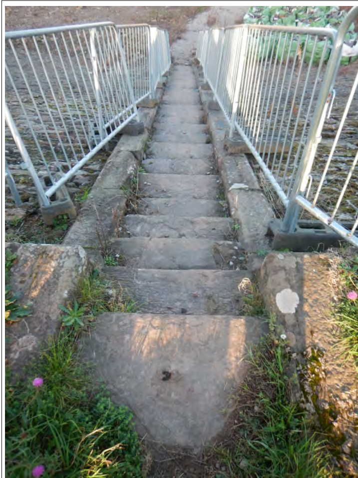
Plate 12. Access steps to the interior of the reservoir from the south-east corner.
