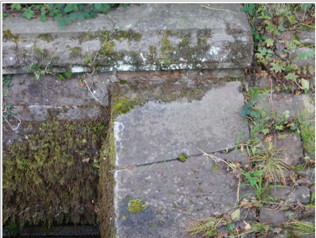
Plate 34. Detail of the stonework showing a notch in the stonework which probably held an in-wash screen.
