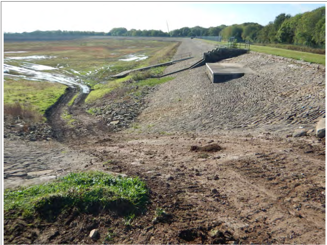
Plate 66. View south-west from the north-west corner of the reservoir, showing the Inlet Gauge Chamber, Jetty, and in the foreground the Slipway.
