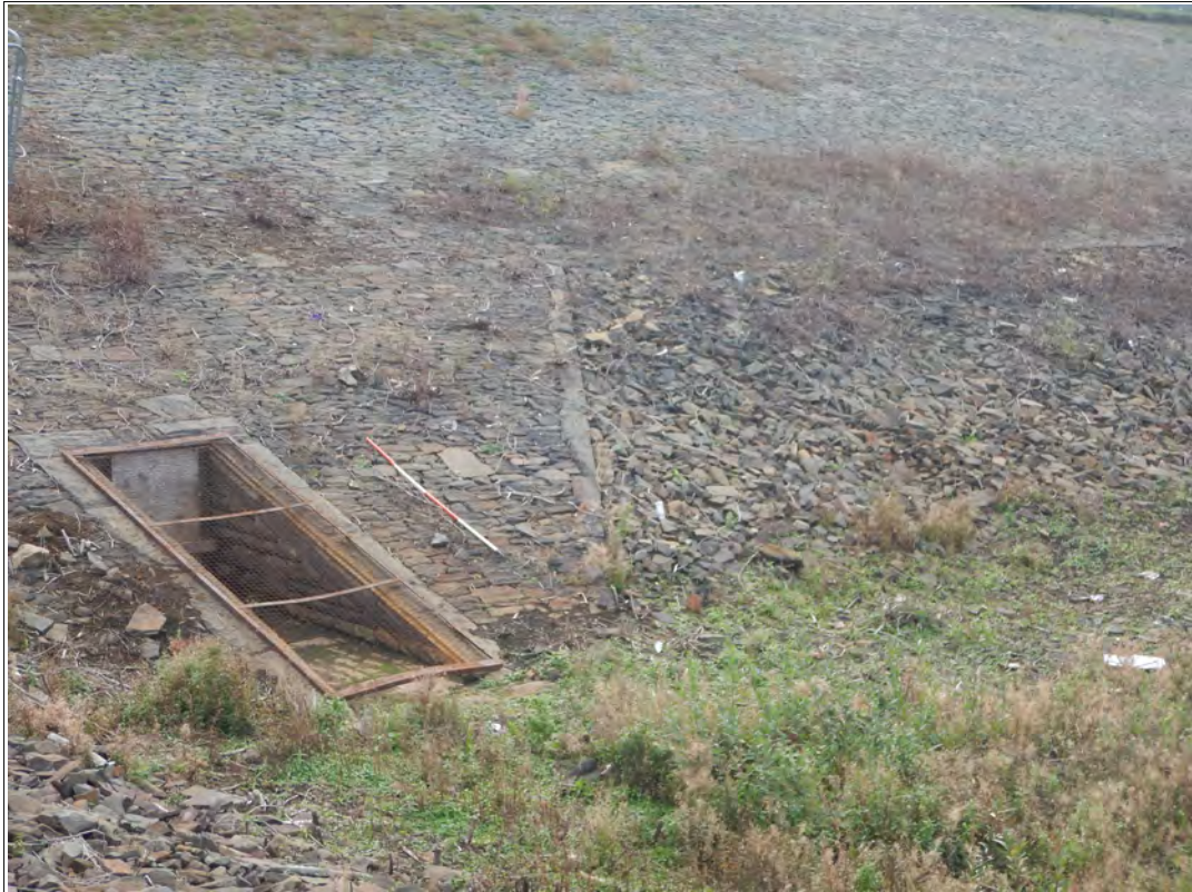
Plate 17. Extension of the pitched stone around the lower outflow control valve platform inlet, looking south-west.
