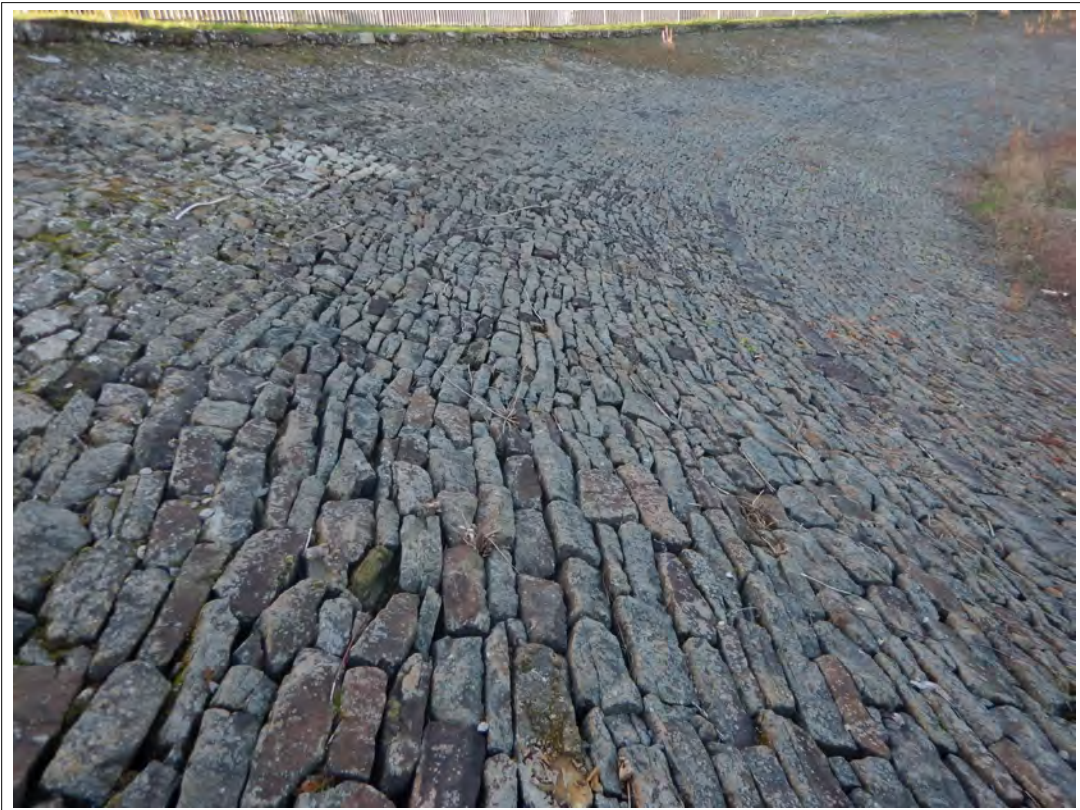
Plate 7. Interior of the pitched stone embankment in the south-east corner of the reservoir, looking south-west.
