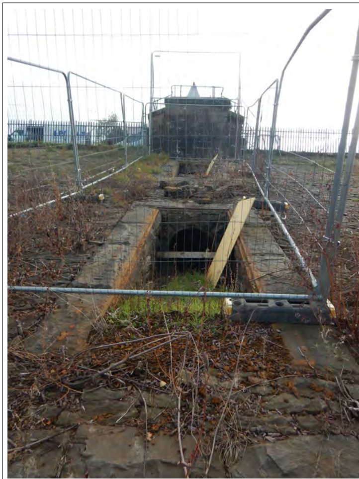
Plate 16. The outflow control valve platform, looking south.
