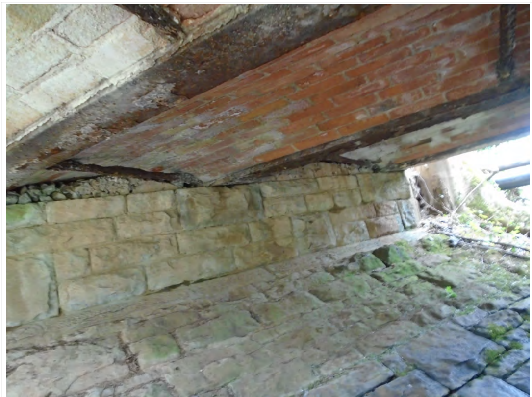
Plate 28. The underside of the 'SEMD' bridge, showing the brick jackarches with supporting cast iron rails.
