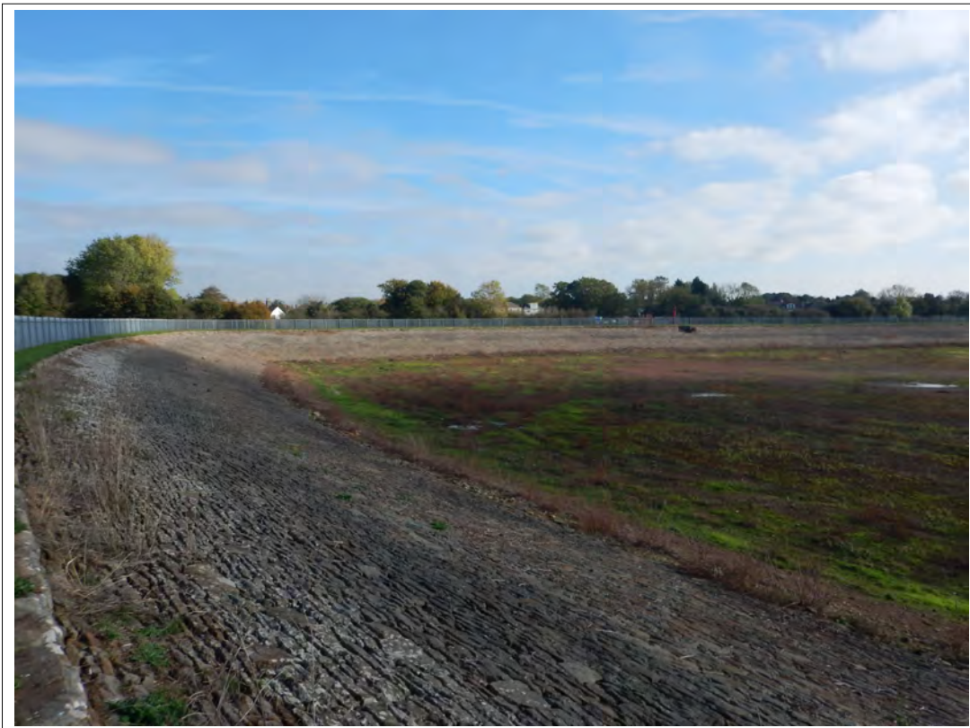
Plate 76. North-east bank of the reservoir, with a pipe penetration visible on the far bank, looking south-east.
