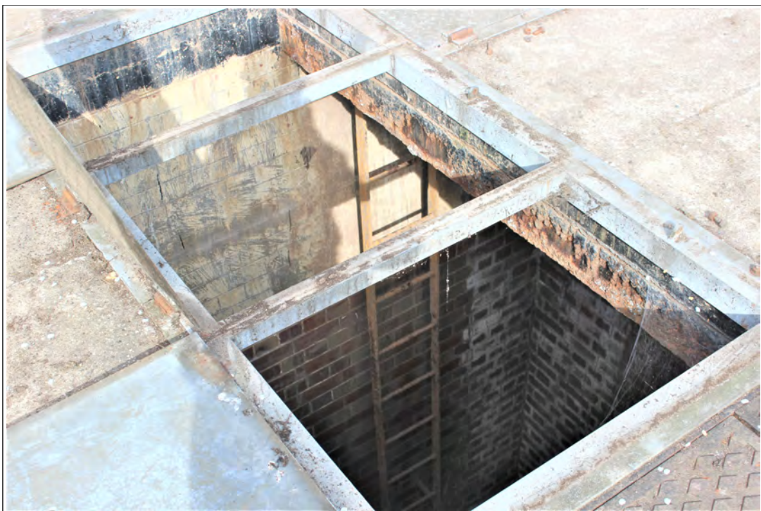
Plate 50. Looking into the interior of the screening chamber, showing the interior brickwork and access ladder.
