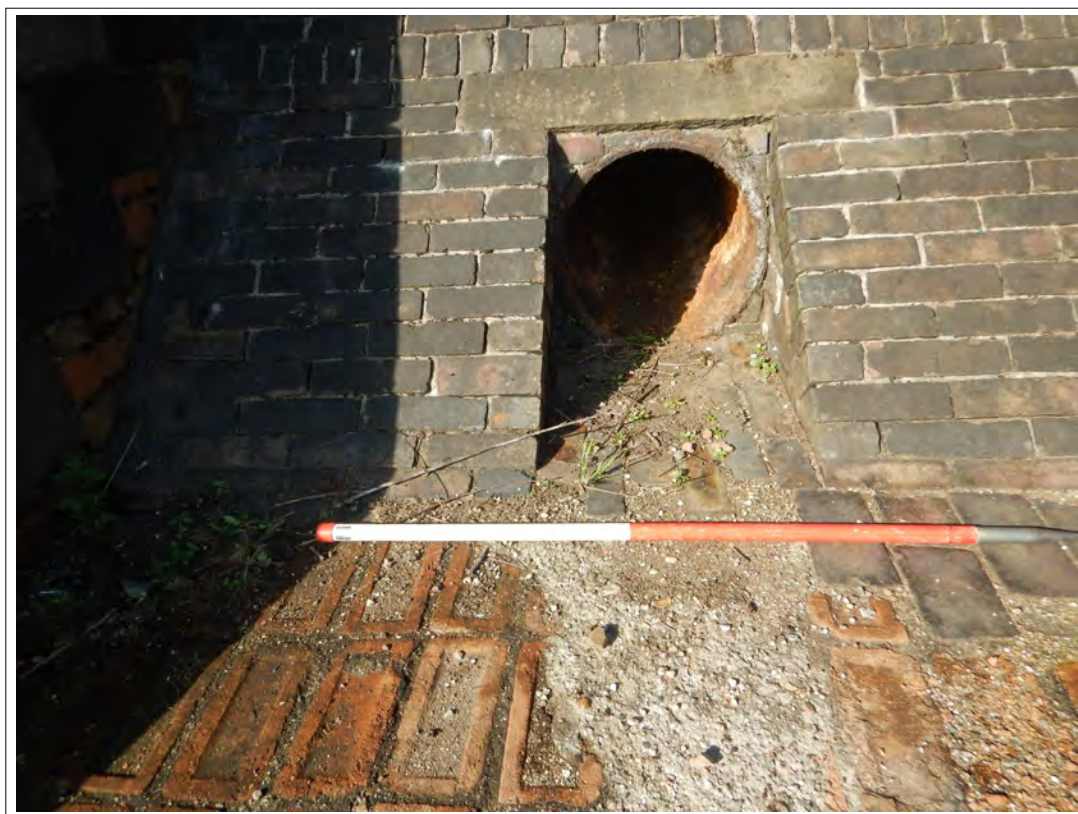
Plate 72. Close-up of the outlet pipe on the Inlet Gauge Chamber, looking north-west. Scale 1m.
