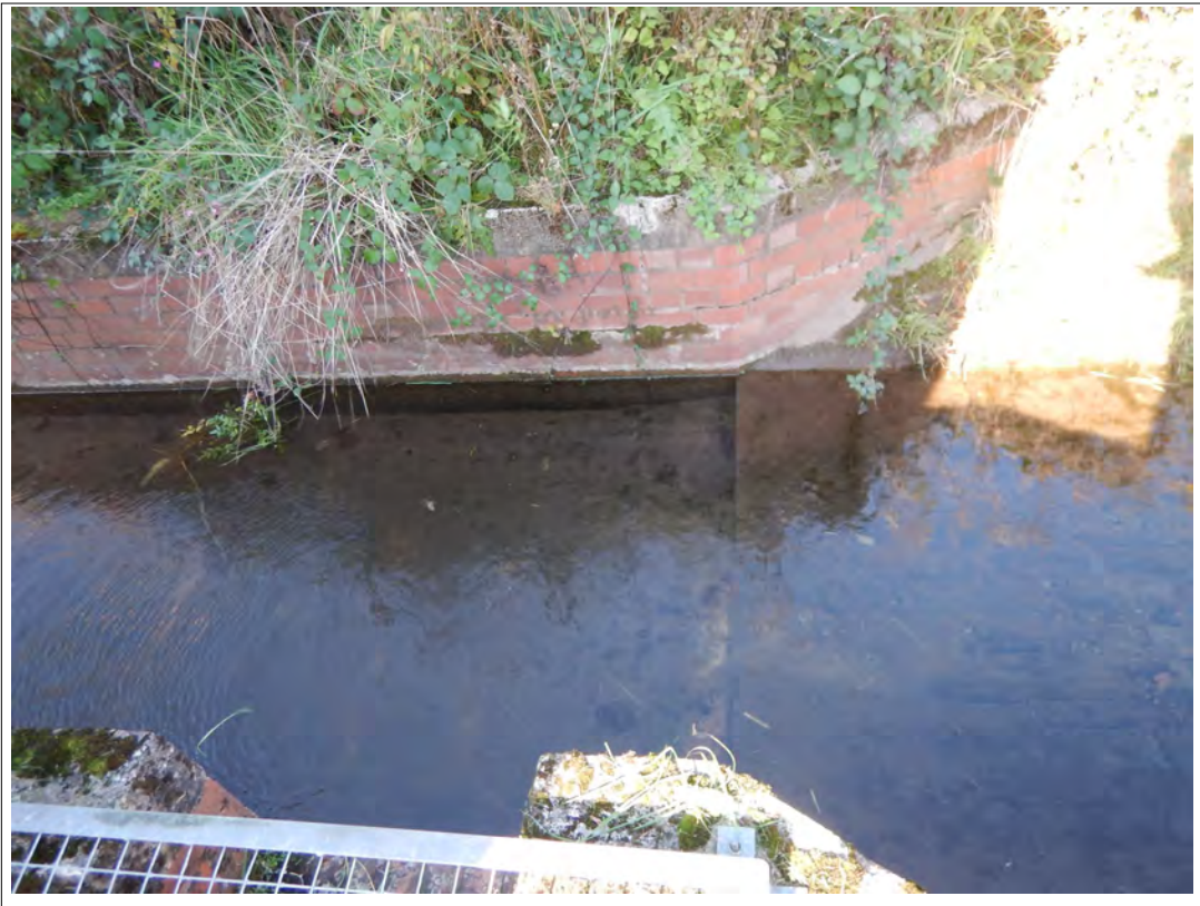
Plate 63. Modified section of the by-wash channel to the rear of the Gauging Station building, looking west.
