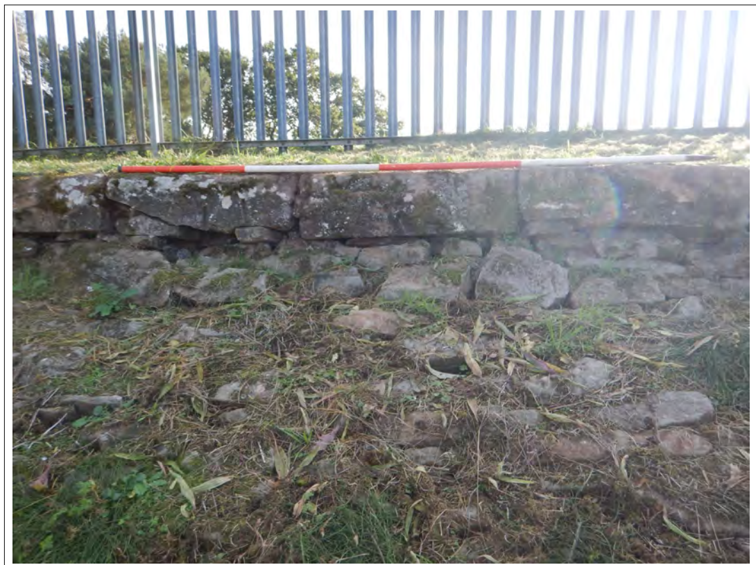
Plate 8. Edging stones to the top of the pitched stone embankment interior, looking south. Scale 2m.
