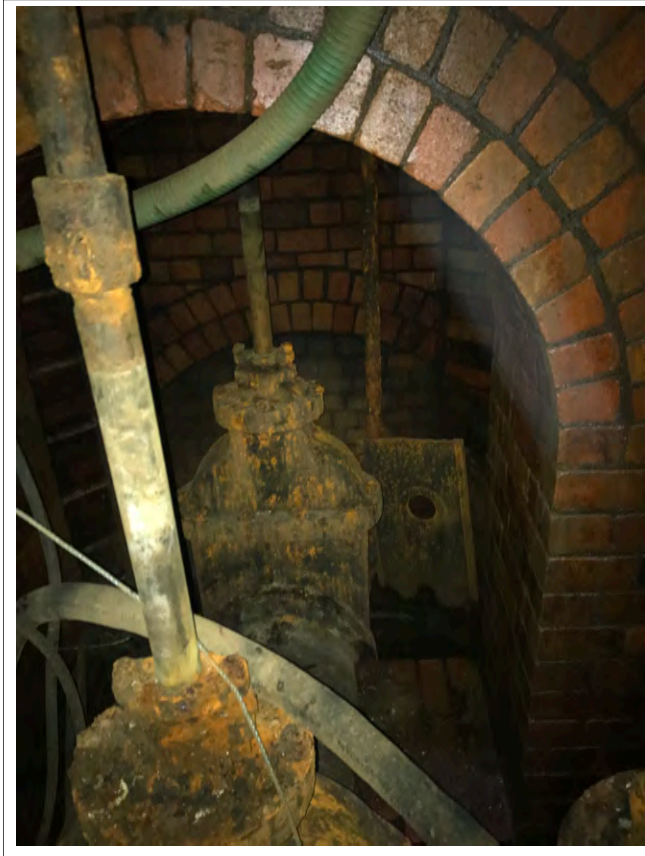
Plate 21. Brick arches at base of the valve tower, showing pipes and valve mechanism.
