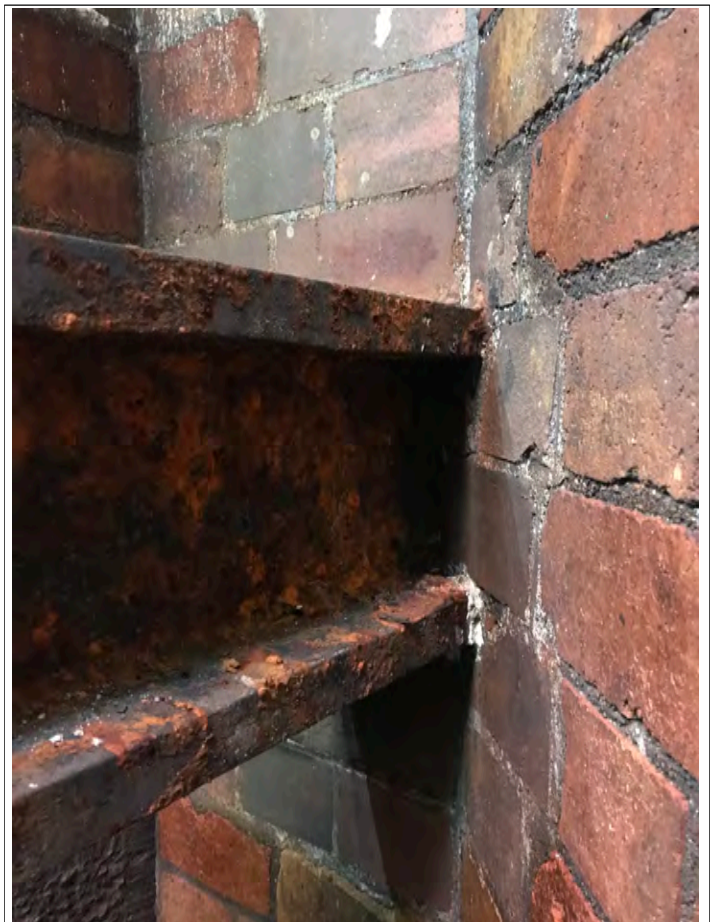
Plate 20. A later addition girder, probably part of the 1929 alterations to the valve tower, with replacement brickwork.
