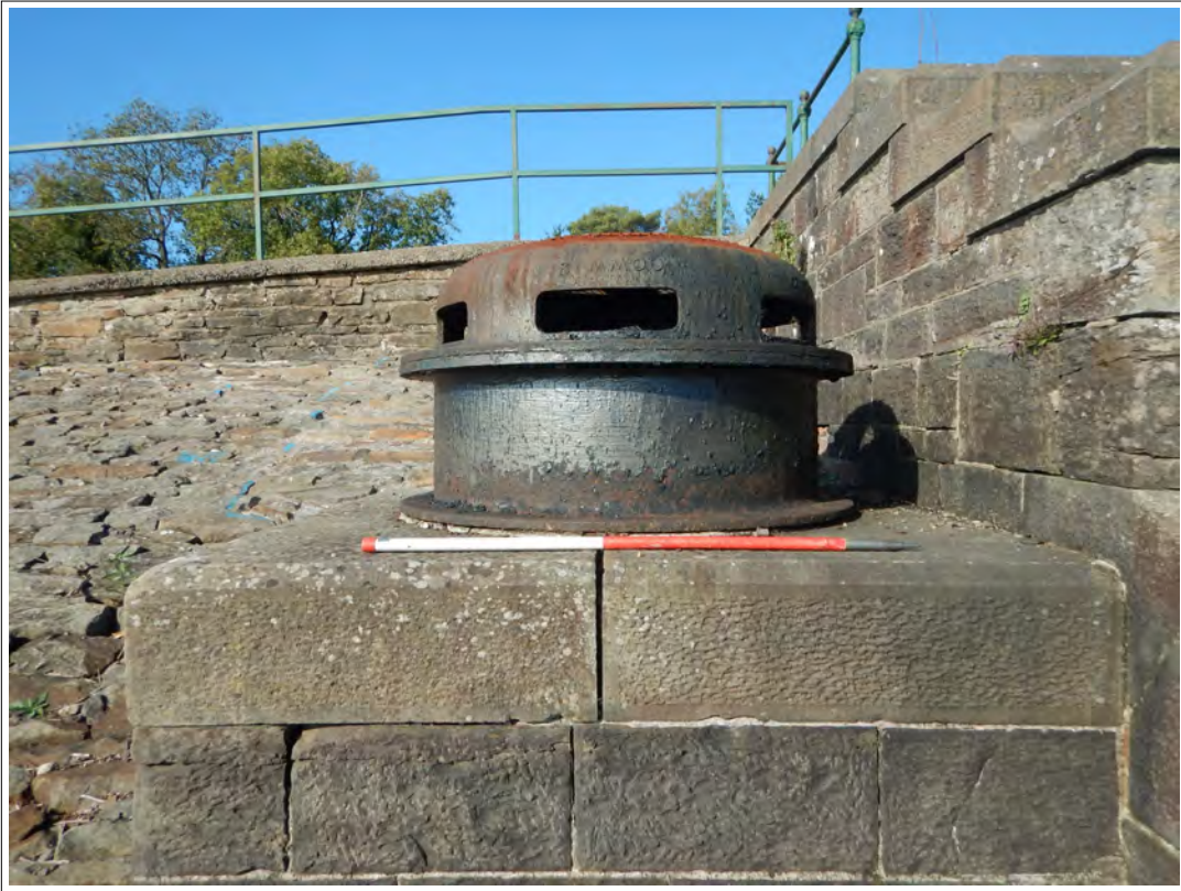
Plate 67. Overflow valve to the south-west of the Inlet Gauge Chamber, and the south-western wall. Scale 1m.
