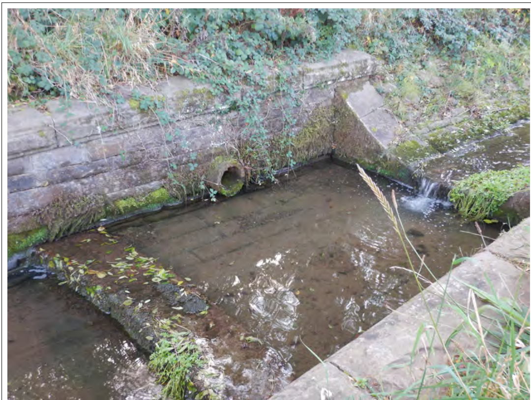
Plate 31. Detail of the stepped weir showing the inflow from the by-wash channel.
