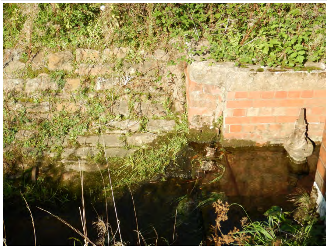
Plate 64. South-west of the modified section of the by-wash channel by the Gauging station building showing small stone step weir, looking west.
