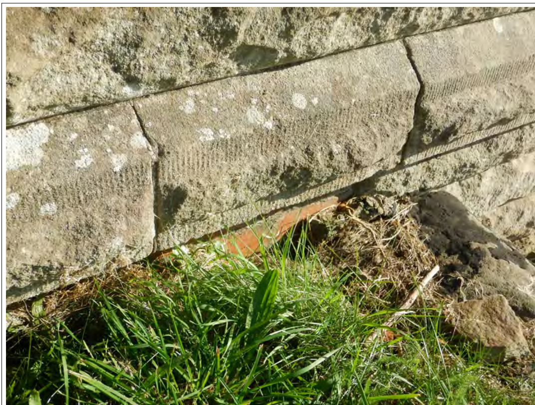
Plate 42. Detail of southern exterior wall of the Cipoletti Weir, showing exposed bricks at the base.
