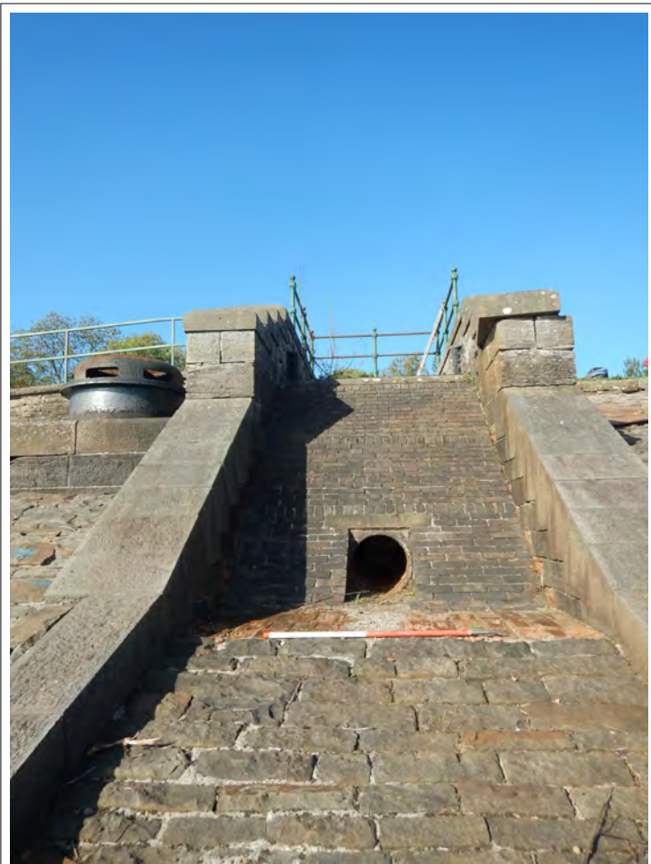
Plate 71. South-east elevation of the Inlet Gauge Chamber showing the outlet pipe, looking north-west. Scale 1m.
