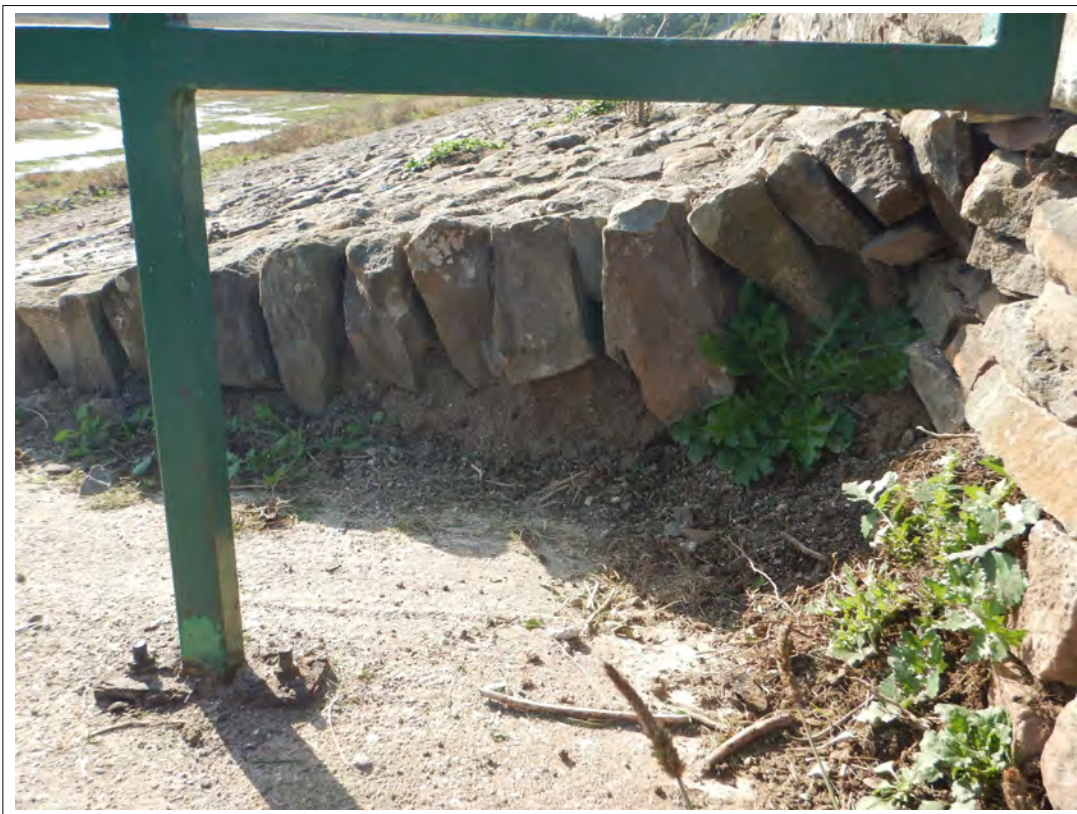
Plate 3. Section into the pitched stones of the embankment interior where the Jetty was constructed, showing the pitched stone construction, looking south-west.
