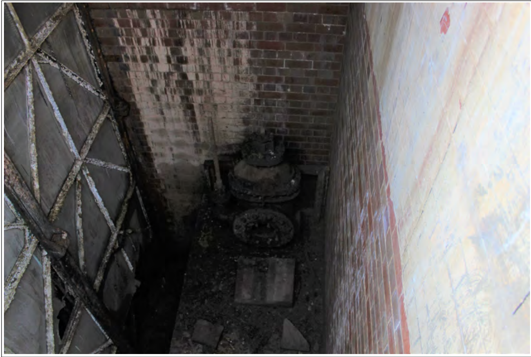
Plate 53. Interior of the Old Screening Chamber, showing some of the original pipe work and the screen.
