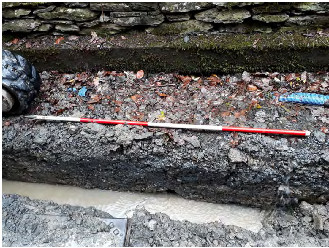
Plate 30. Drainage run to the NE (rear) of the house, clay in section. View NE. 2m scale
