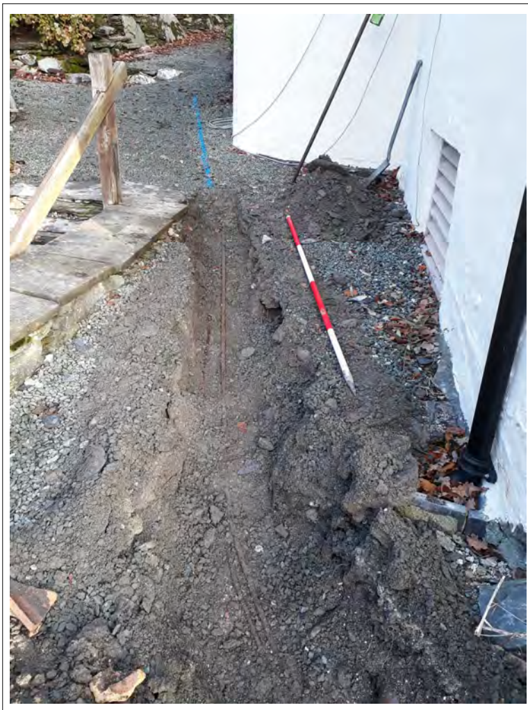
Plate 16. Drainage run to the NW of the house, revealing disused iron pipes. View NE. 2m scale
