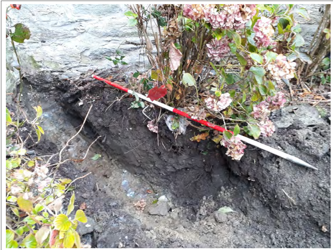
Plate 35. Drainage run to the SE of the house. View NE. 2m scale
