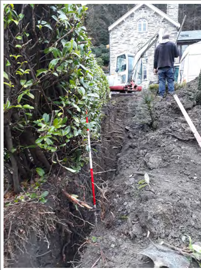
Plate 11. Drainage run in the front garden to SW of house. View NE. 2m scale
