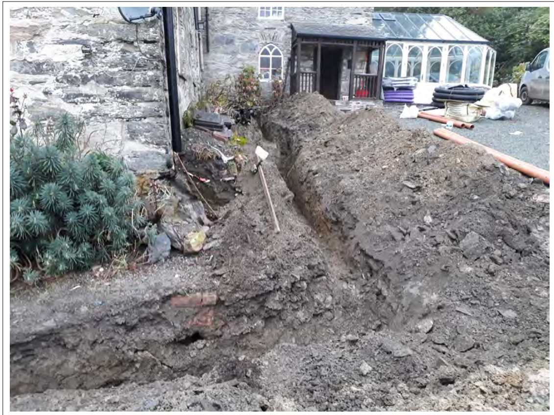
Plate 39. Drainage run to the SE of the house. View NE. 2m scale
