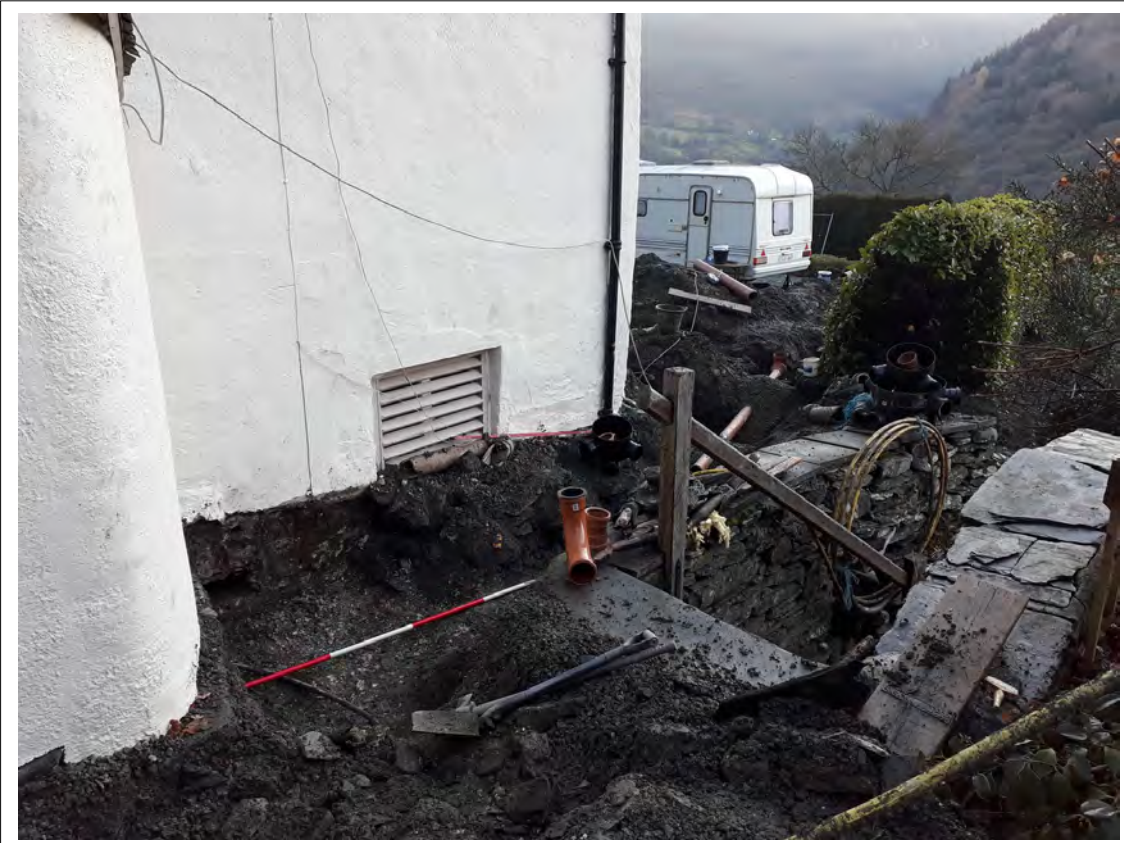
Plate 20. Drainage run to the NW of the house, with entrance for boiler services. View SE. 2m scale
