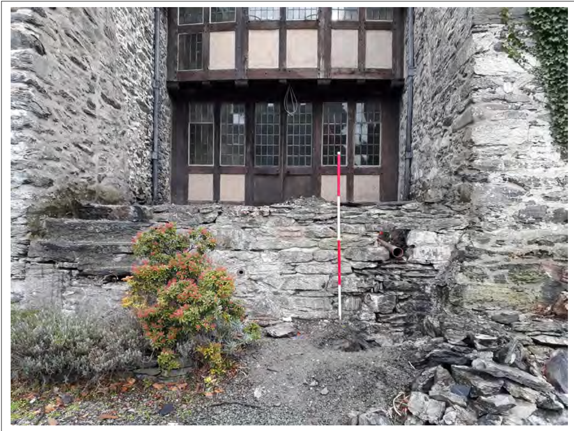
Plate 3. The front of the house (SW) with drainage works. View NE. 2m scale
