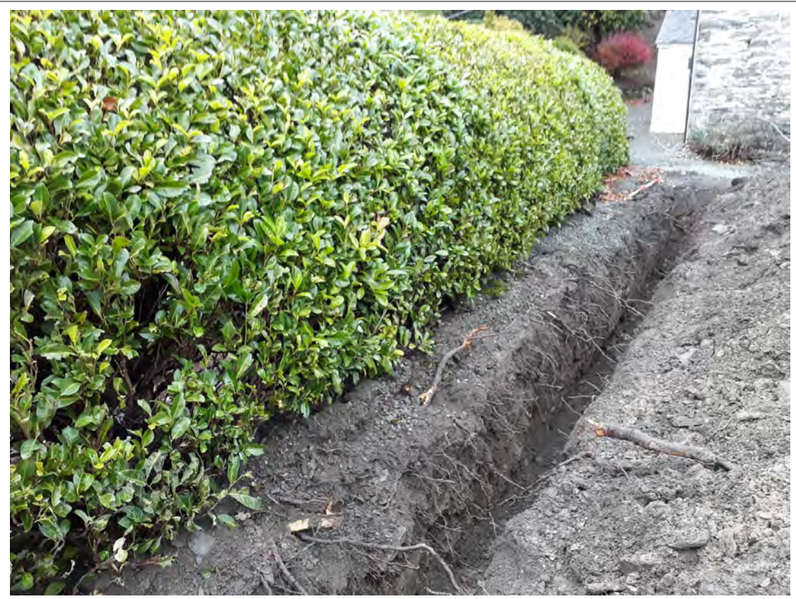
Plate 13. Drainage run in the front garden to SW of house. View NE.
