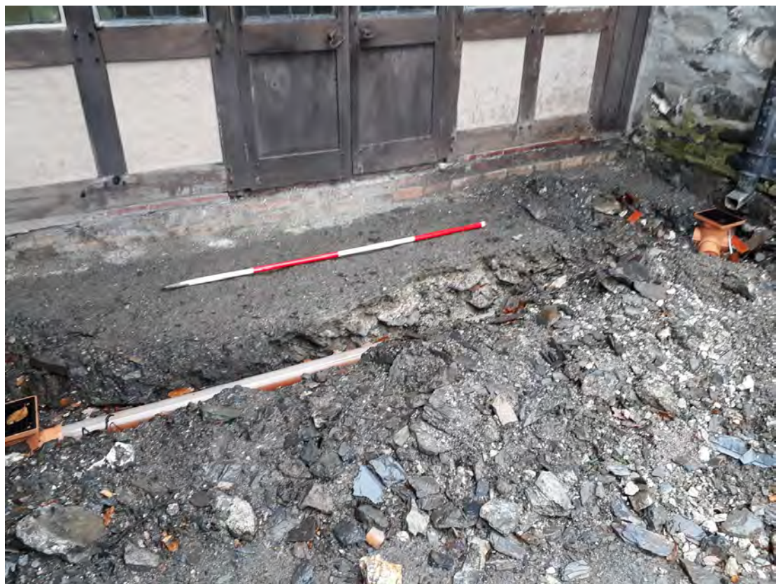
Plate 5. The front of the house (SW) with drainage works, showing rubble hard-core below entrance. View NE. 2m scale
