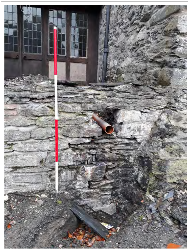
Plate 4. The front of the house (SW) with drainage works. View NE. 2m scale
