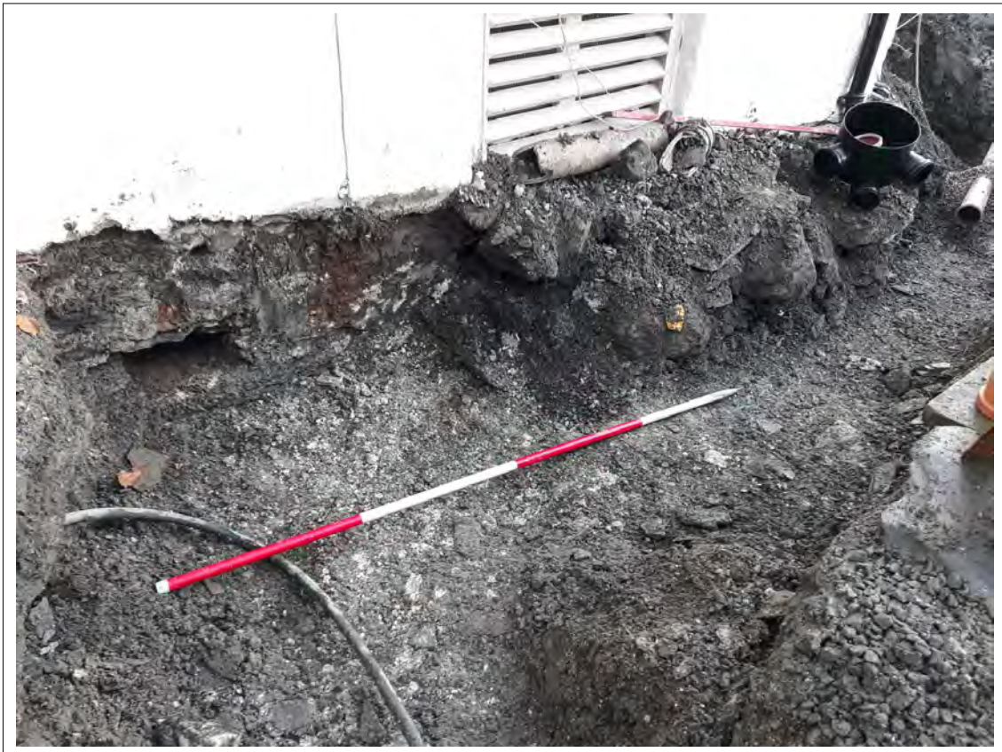
Plate 21. Drainage run to the NW of the house, with entrance for boiler services. View SE. 2m scale
