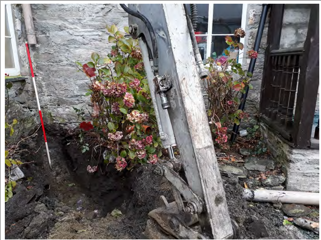
Plate 34. Drainage run to the SE of the house. View NE. 2m scale
