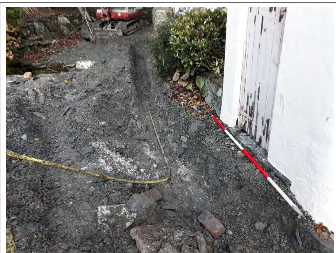
Plate 22. Drainage run to the NW of the house, deepened to reveal gas pipe. View NE. 2m scale
