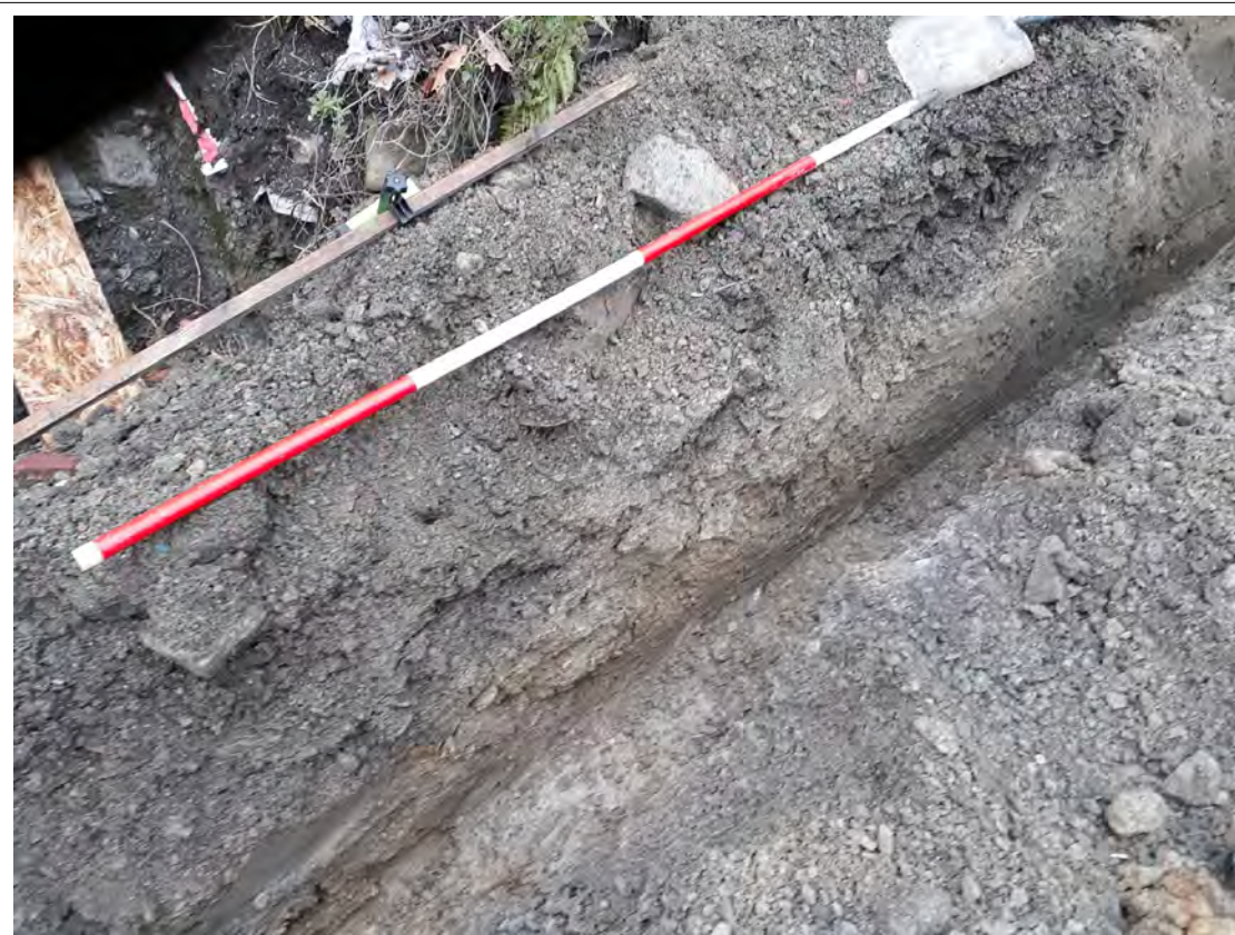
Plate 38. Drainage run to the SE of the house. View NW. 2m scale
