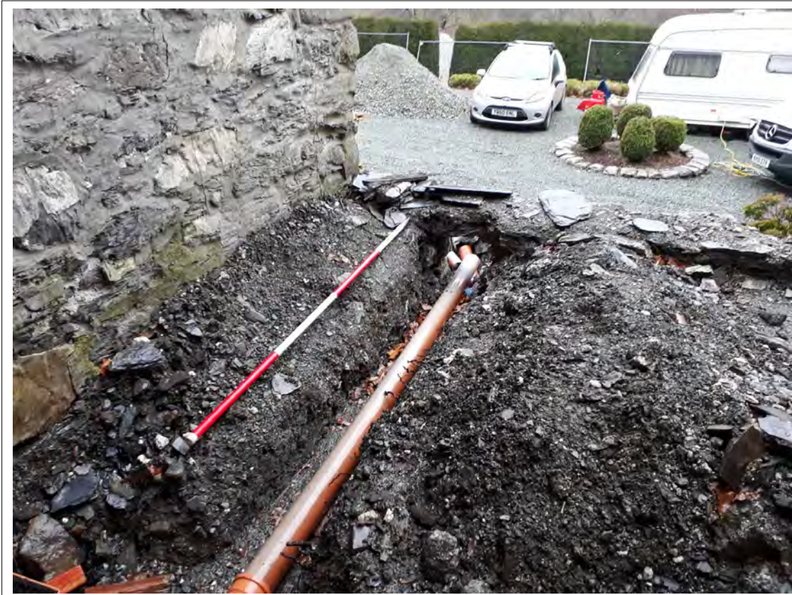
Plate 7. The front of the house (SW) with drainage works. View SW. 2m scale
