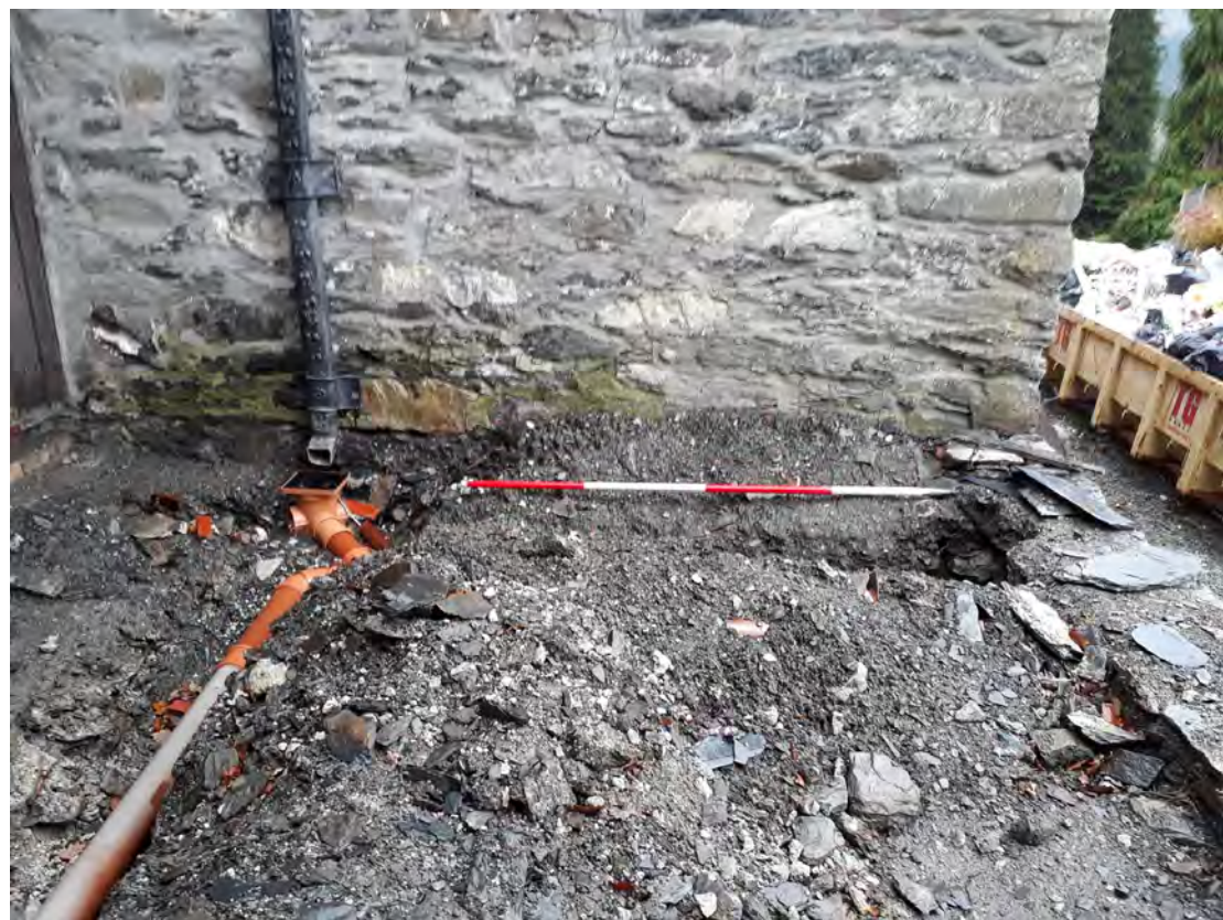
Plate 6. The front of the house (SW) with drainage works. View SE. 2m scale
