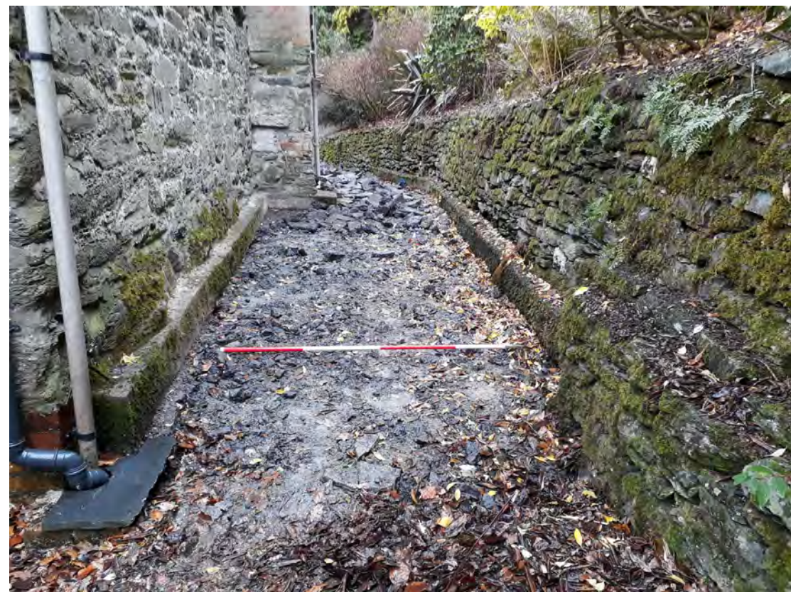
Plate 24. Breaking out of tarmac to the NE (rear) of the house. View NW. 2m scale
