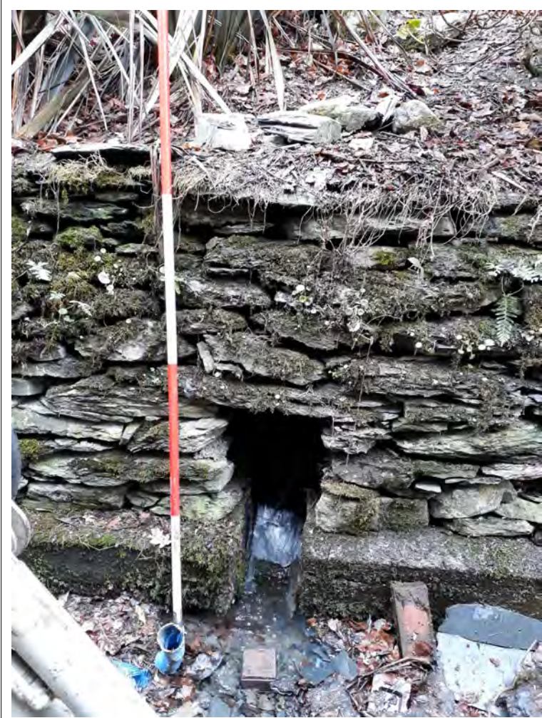
Plate 31. Drainage run to the NE (rear) of the house. Stream in culvert. View NE. 2m scale
