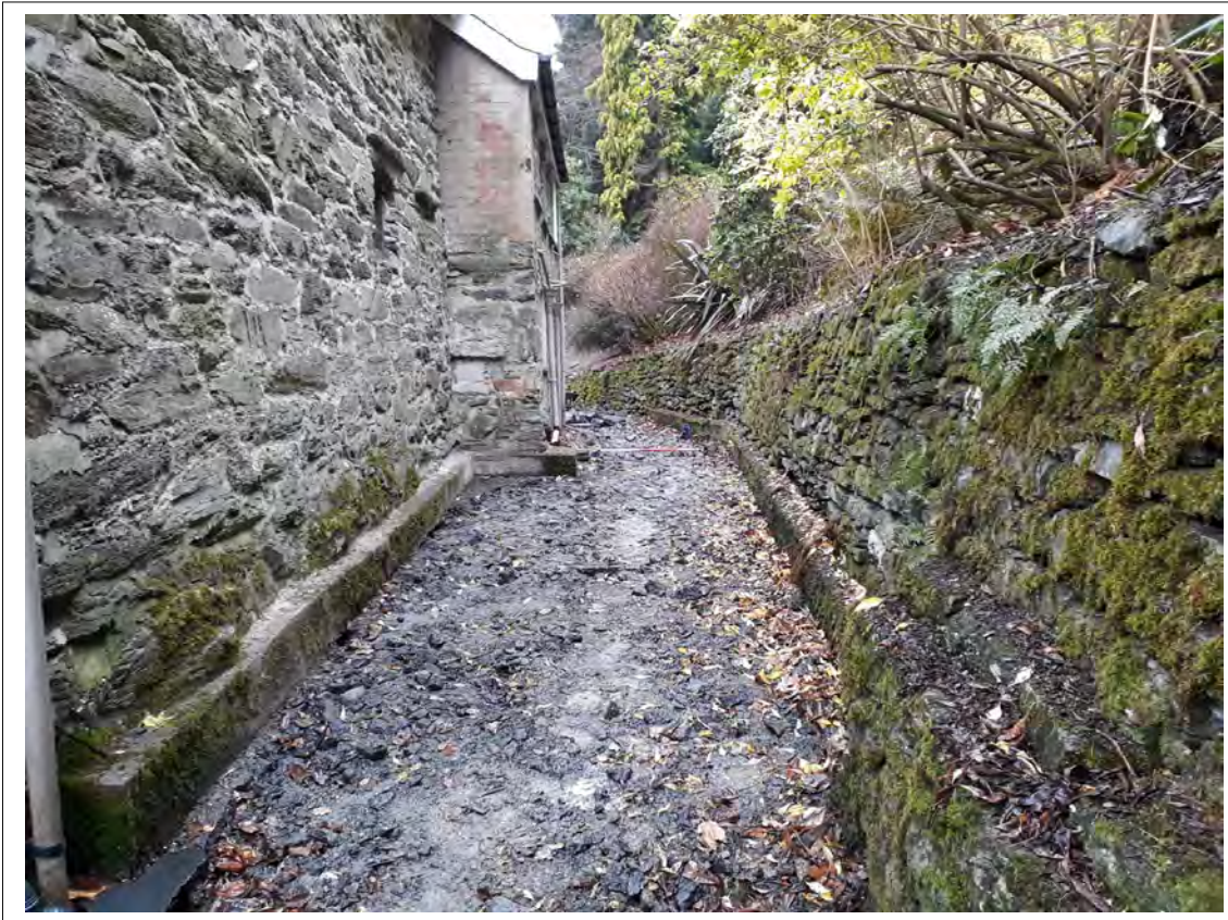
Plate 25. Breaking out of tarmac to the NE (rear) of the house. View NW. 2m scale
