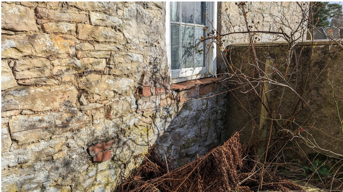
Plate 13: Rough nature of repairs to the southern elevation
