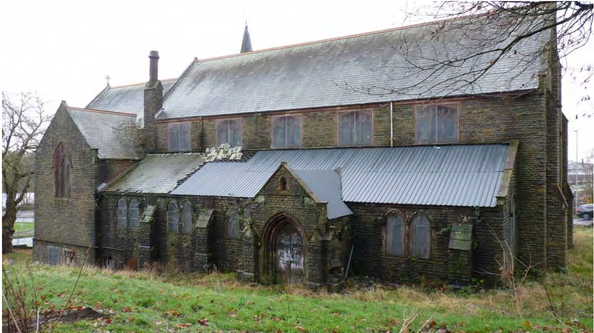
Photo 11: View of the north face of St Paul's church, from the edge of the proposed development area.
