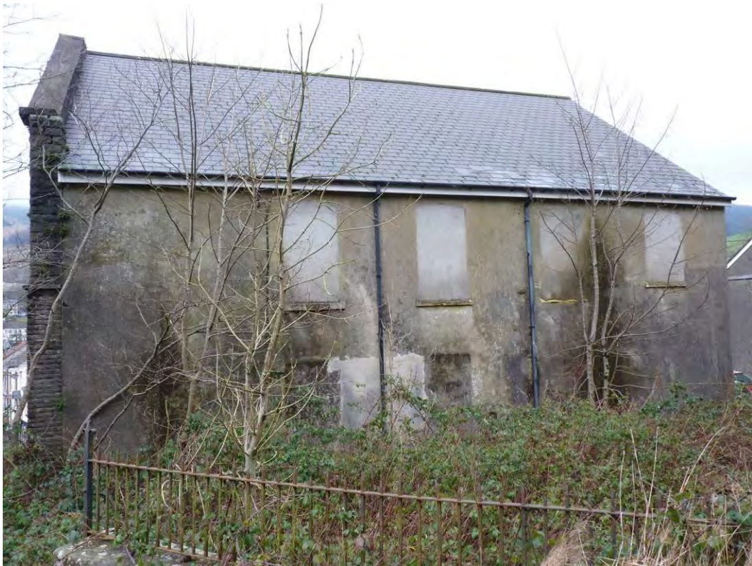
Photo 12: South-east elevation, with blocked openings. Those to the ground floor appear to have been blocked prior to rendering. View northwest.
