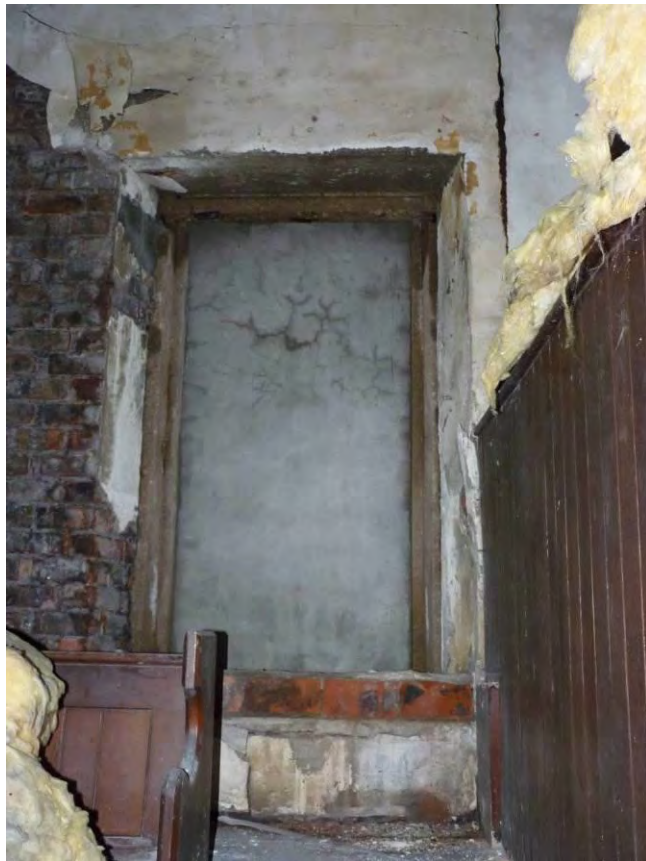
Photo 50: Blocked window opening on the 1 st floor, southwest gable wall. View southwest.
