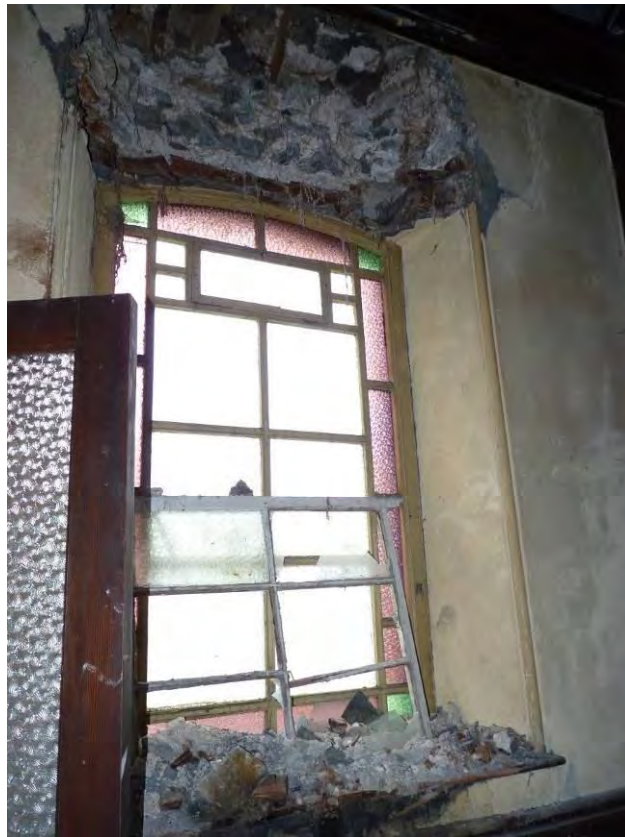
Photo 48: 1 st floor window in northwest wall, with collapsed lintel. View north.
