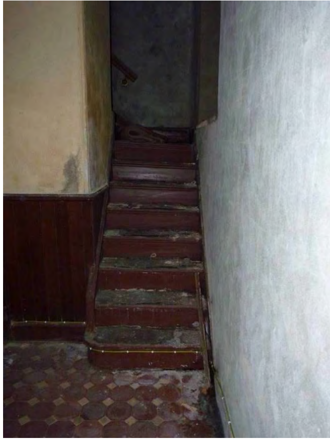
Photo 17: Staircase to the first floor on the southeast end of the vestibule, inaccessible due to rot.
