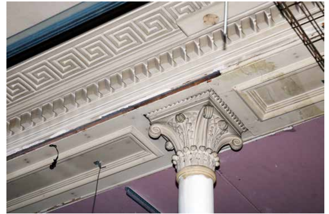
Section of meander and dentil plaster cornice with bolection moulded panel timber boxing, with the Corinthian capital of one of the cast iron columns on the first floor. IMG_7972.
