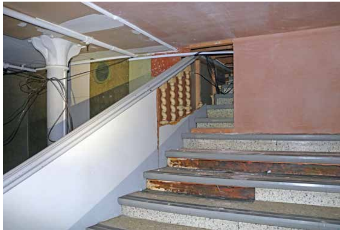
View of the staircase looking south-west, showing the solid boards obscuring much of the balustrading. (b(122)).
