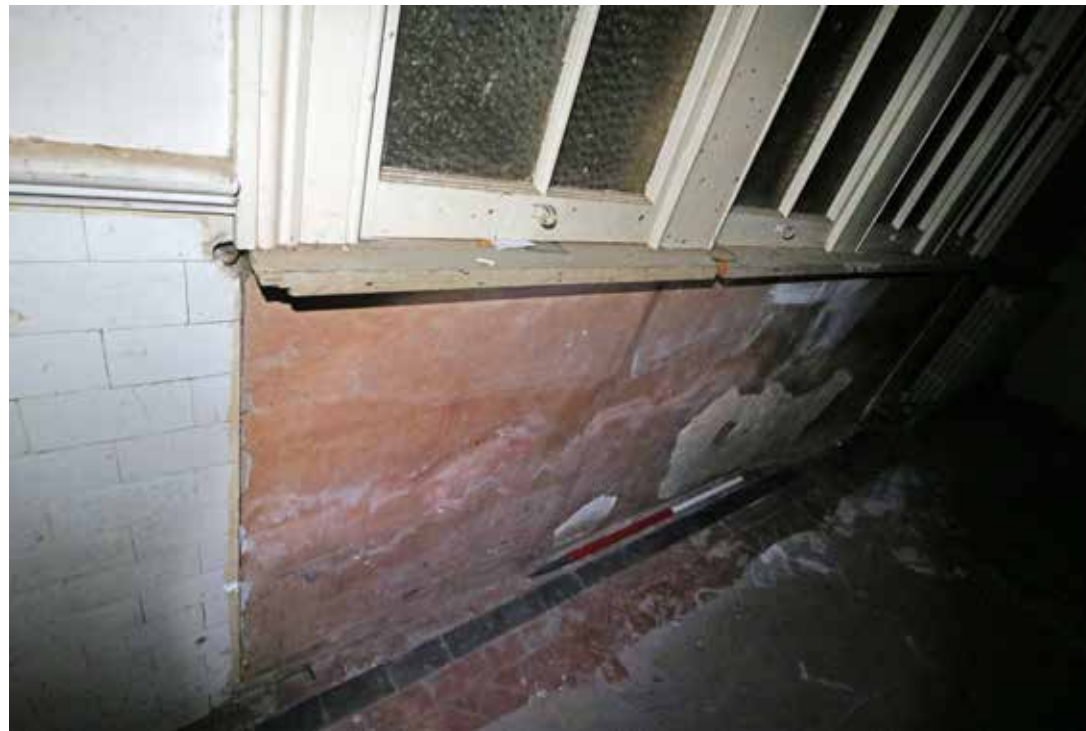
Detail of the join between the tiled finish of the north west wall and the rendered plaster finish beneath the four timber windows. IMG_8149.
