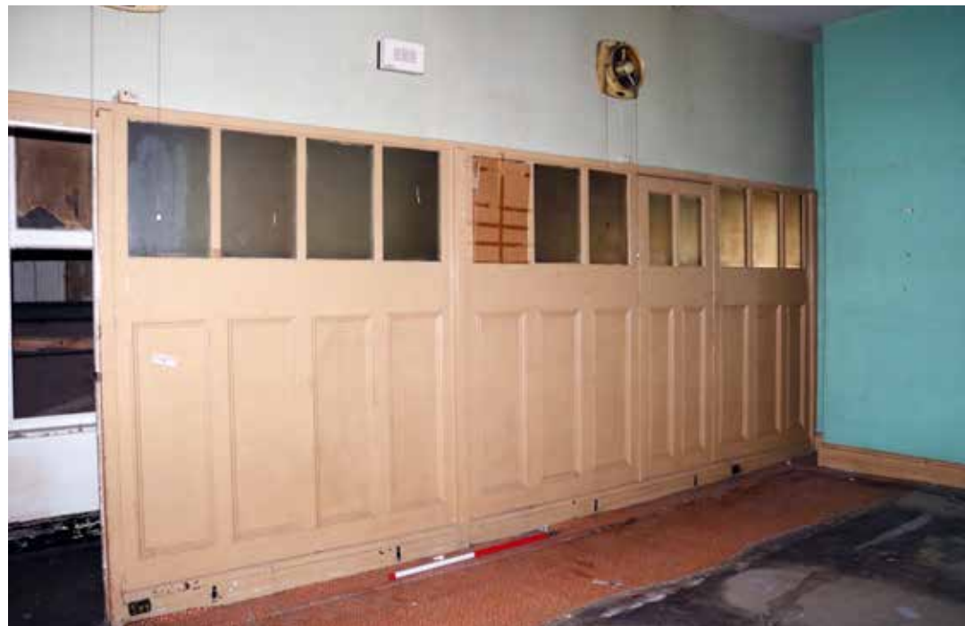
The rear side of the timber partition as seen from room 2/17. The inserted doorways can be seen in the first and fourth bays. IMG_7638.
