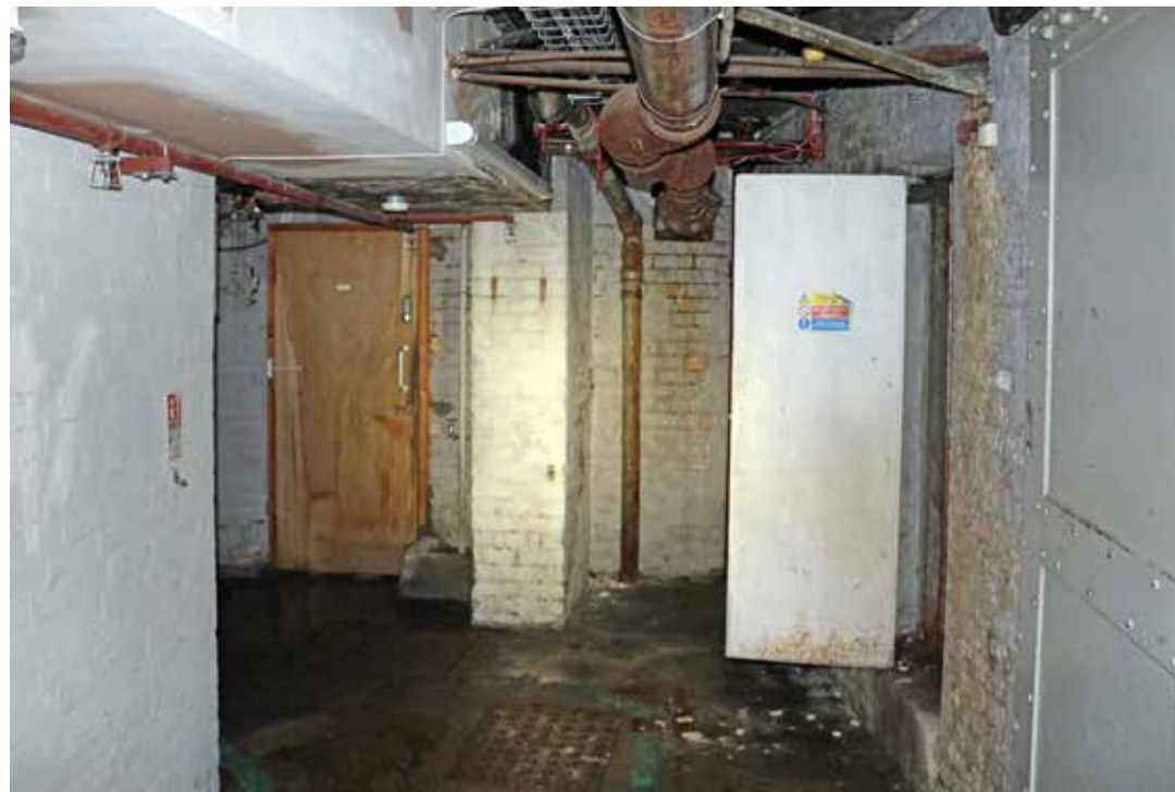
View of the north-west fire door showing the asbestos lining, looking north-east (b(77)).
