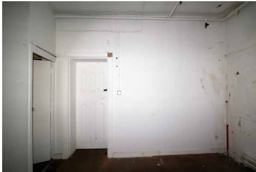
The rear of the south west door as seen from room I/19. IMG_7789.
