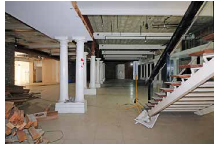
The rows of paired columns on the ground floor of the Chapel. IMG_8208.
