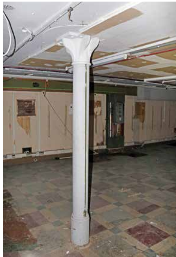
Simple 1889 column to the basement level. One of six within the basement. (b(124).JPG)
