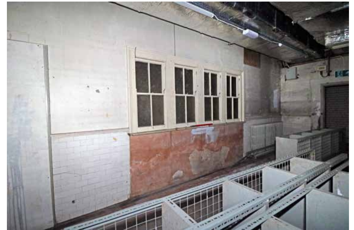
Elevation of the north west wall from 0/12, showing the windows with infilled wall beneath. IMG_8145.
