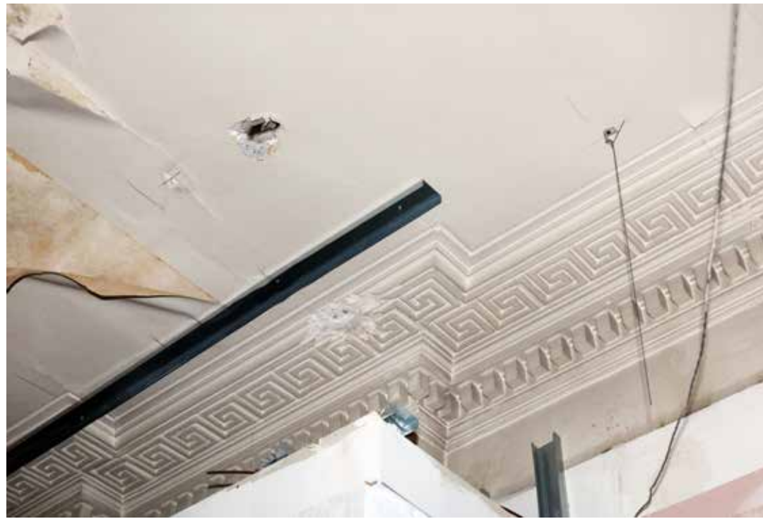
A section of the meander and dentil plaster cornice on the ground floor. IMG_7933.
