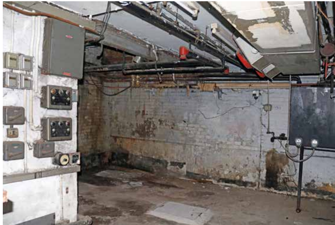
View of side room and Midland Electrical Manufacturing switches, B/02
