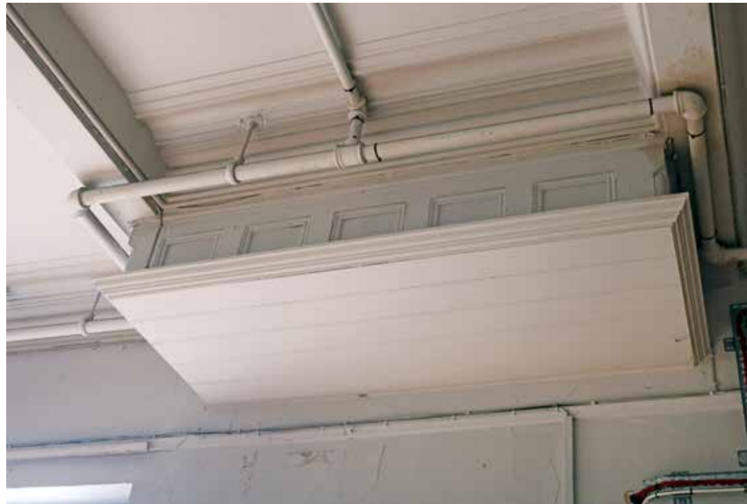
Ceiling of room 2/16 with c.1878 cornice and moulded timber panel boxing and historic service piping. IMG_7625.
