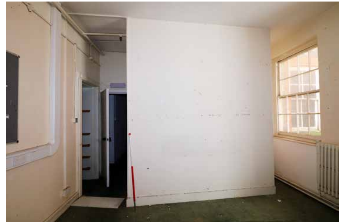
Room I/17 showing that the space behind the north east historic door has had timber shelving installed. IMG_7785.
