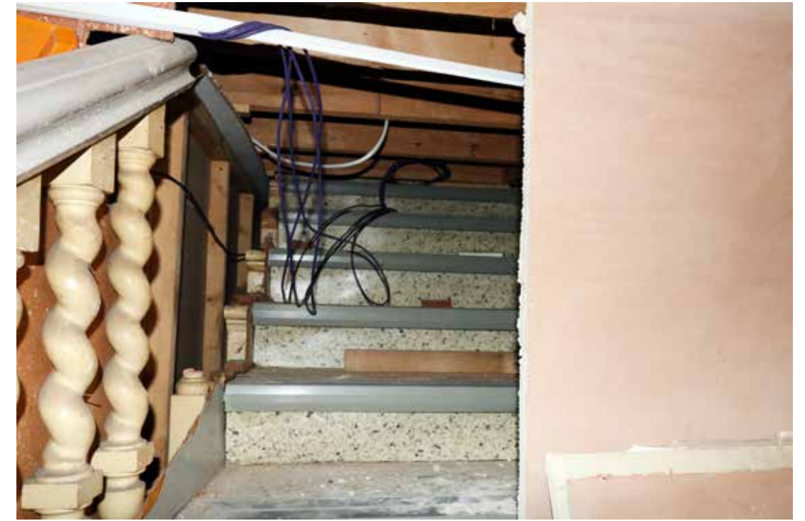
Detail of the historic balusters looking south-west, showing where balusters were cut off to accommodate the new floor above, looking south-west. IMG_0941.
