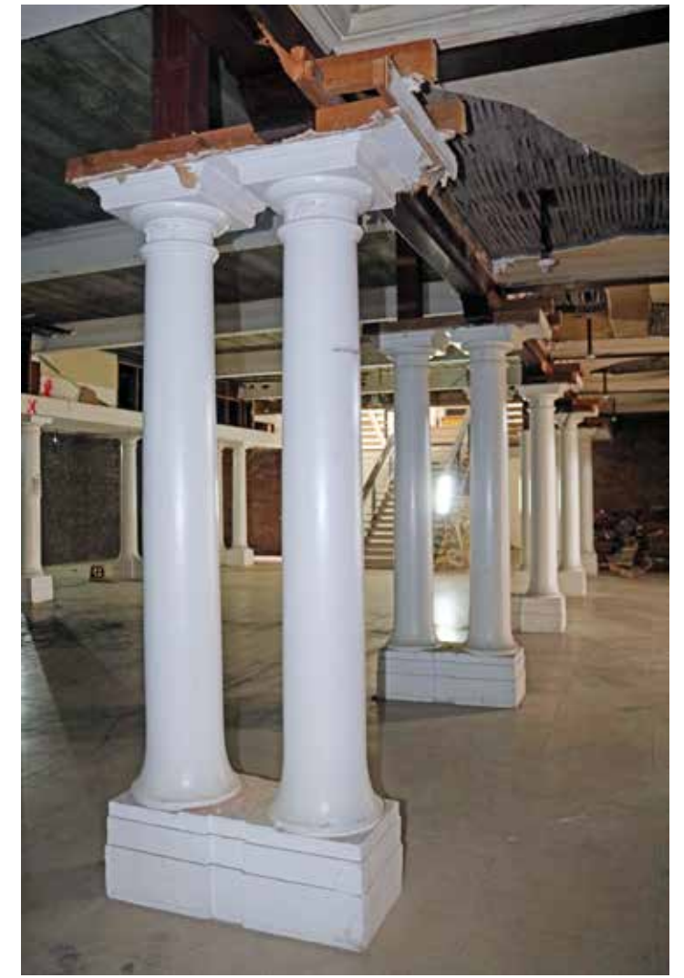
Detail of the ground floor columns; they are of a simple design and stood upon block pedestals. IMG_8217.
