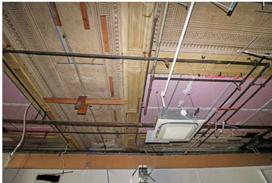
The meander and dentil plaster cornice on the first floor, with the bolection moulded timber boxing framing the historically blocked prism lightwells on the first floor. Also visible is a plaster ceiling rose and the anaglypta wallpaper. IMG_7958.
