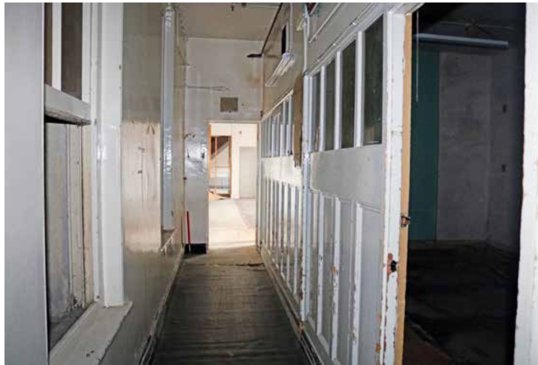
The timber partition wall as seen from the corridor, looking north west, with the blocked lightwell to the east. IMG_7634.
