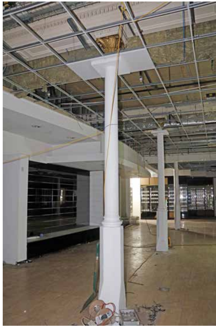
1889 columns on the east side of the ground floor shop floor, with their Corinthian capitals painted gold above the modern suspended ceiling. IMG_8050
