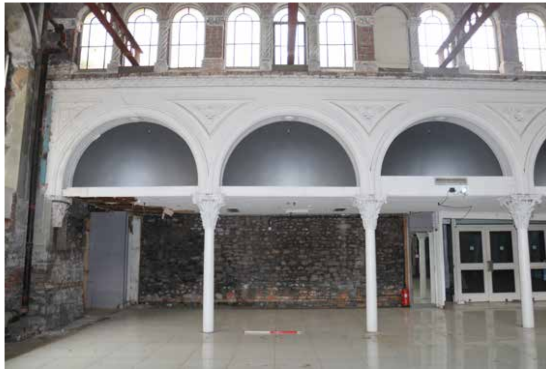
Side aisle of the Chapel on the first floor, where the original galleried seating once was. The intersecting ceilings through the archways are a later addition. IMG_7661.
