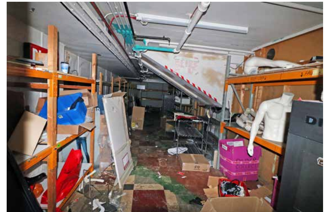
Modern plasterboard to the soffit and stringer of the staircase visible in B/10, looking north-west. (b(28)).
