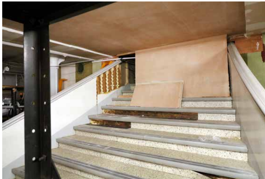
View showing where the vinyl has detached from the timber risers, looking south-west. IMG_0938.
