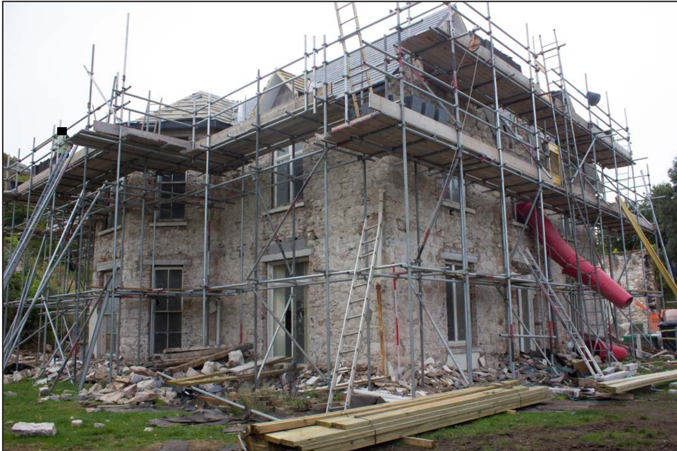
Plate 09: Oblique shot of eastern & northern elevations of Tanrallt Hall, Abergele Road, Llanddulas, Abergele - from the northeast - 2.00m scale
