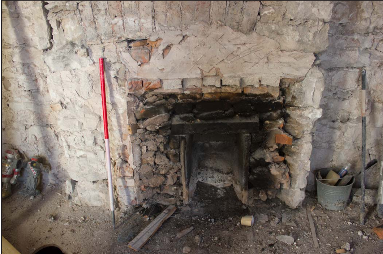
Plate 28: Lounge/Living Room, fireplace, ground floor, Tanrallt Hall, Abergele Road, Llanddulas, Abergele - from the east - 2.00m scale
