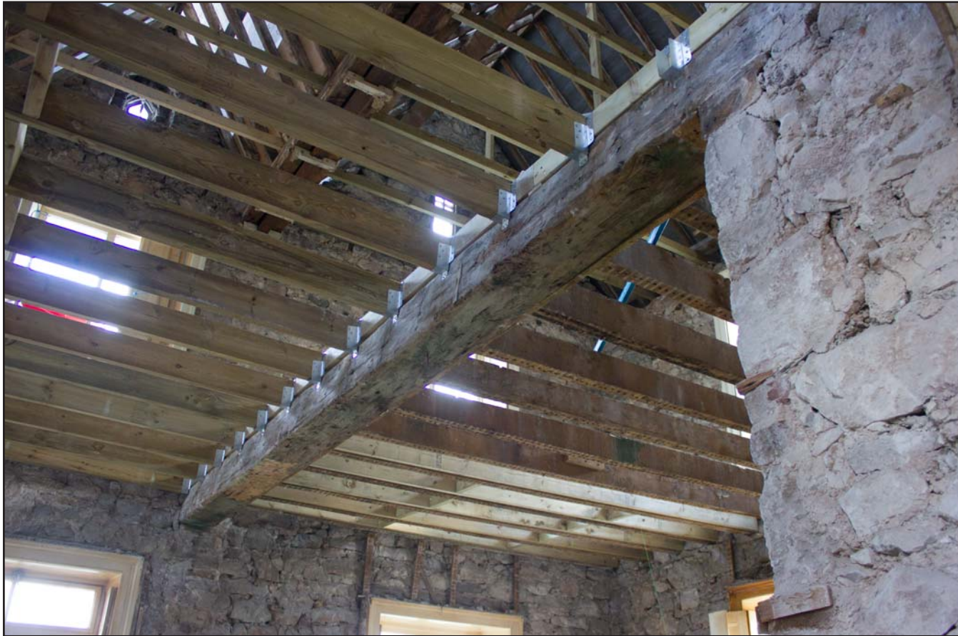
Plate 29: Lounge/Living Room, handhewn beam, ground floor, Tanrallt Hall, Abergele Road, Llanddulas, Abergele - from the east - no scale
