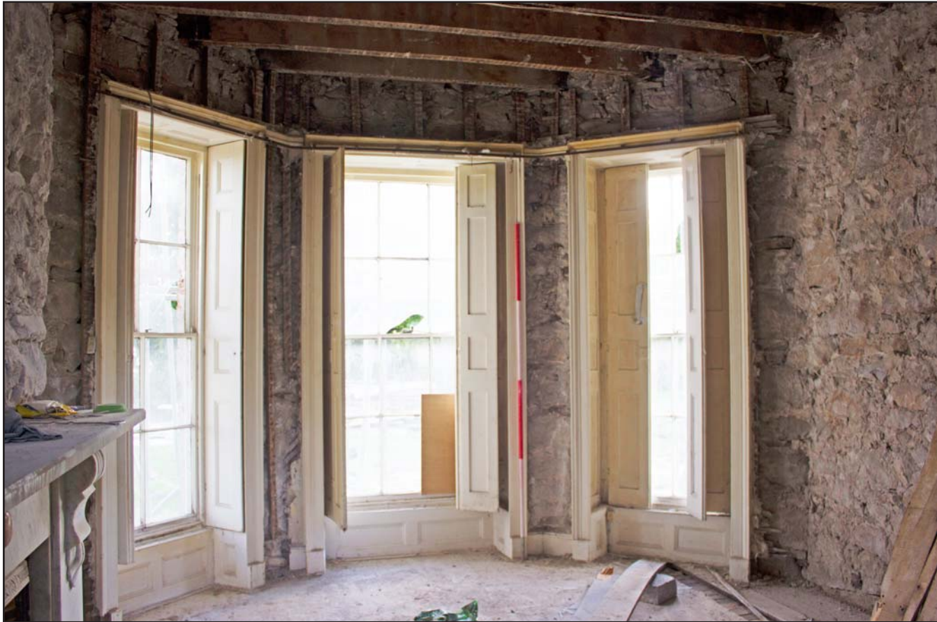
Plate 19: Living Room/Study, ground floor, Tanrallt Hall, Abergele Road, Llanddulas, Abergele - from the northwest - 2.00m scale
