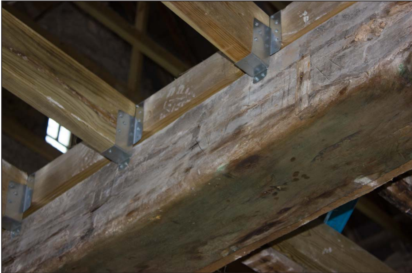
Plate 30: Lounge/Living Room, carpenter's marks on handhewn beam, ground floor, Tanrallt Hall, Abergele Road, Llanddulas, Abergele - from the east - no scale
