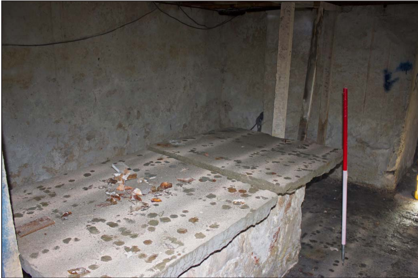
Plate 43: Store/preparation room, basement, Tanrallt Hall, Abergele Road, Llanddulas, Abergele - from the northwest - 1.00m scale
