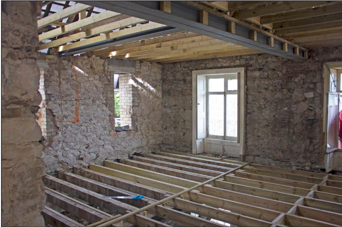
Plate 37: Bedroom 1/2, first floor, Tanrallt Hall, Abergele Road, Llanddulas, Abergele - from the southeast - no scale
