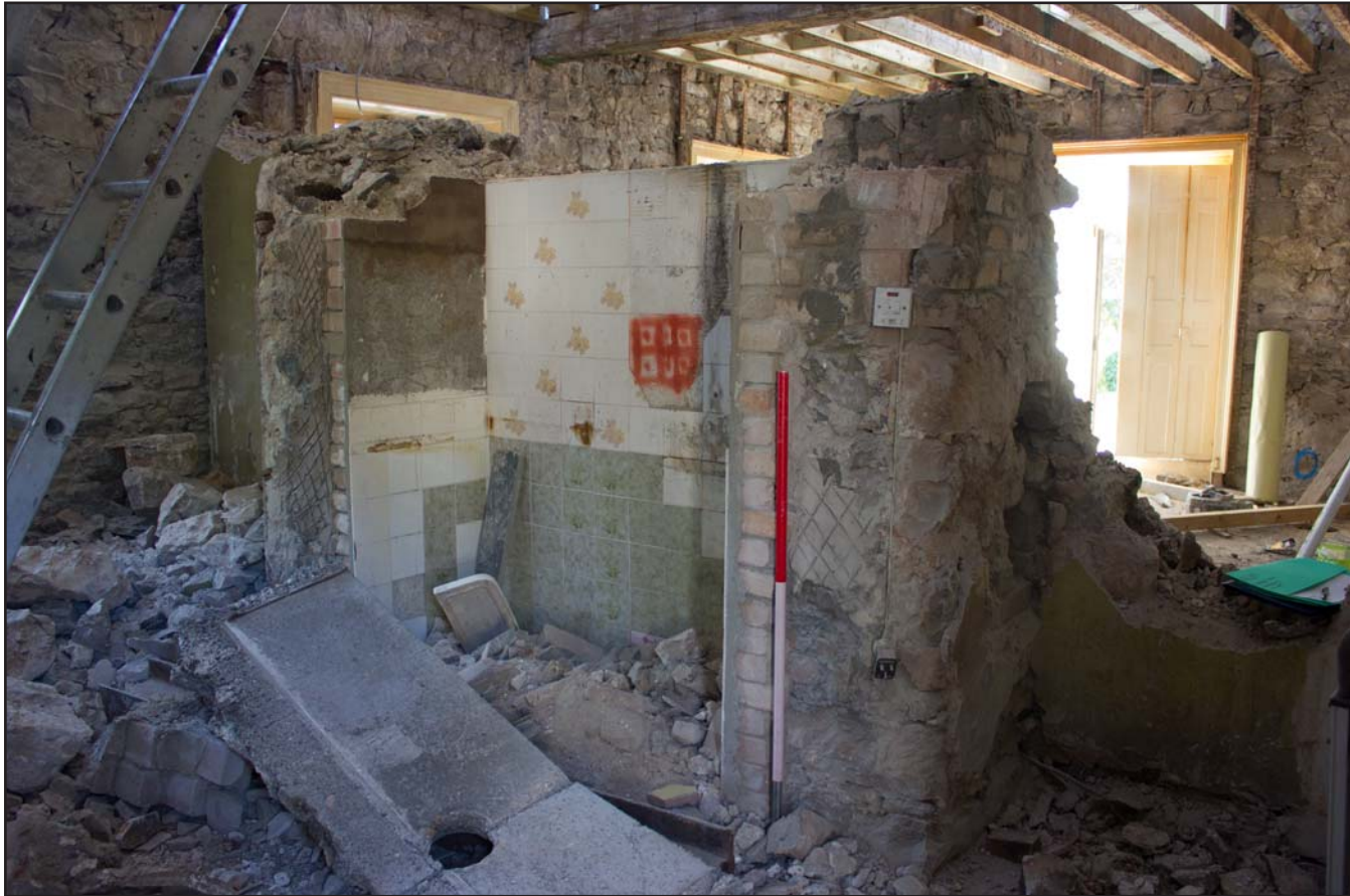
Plate 33: Utility/Kitchen, former kitchen hearth and chimney breast, ground floor, Tanrallt Hall, Abergele Road, Llanddulas, Abergele - from the north - 1.00m scale
