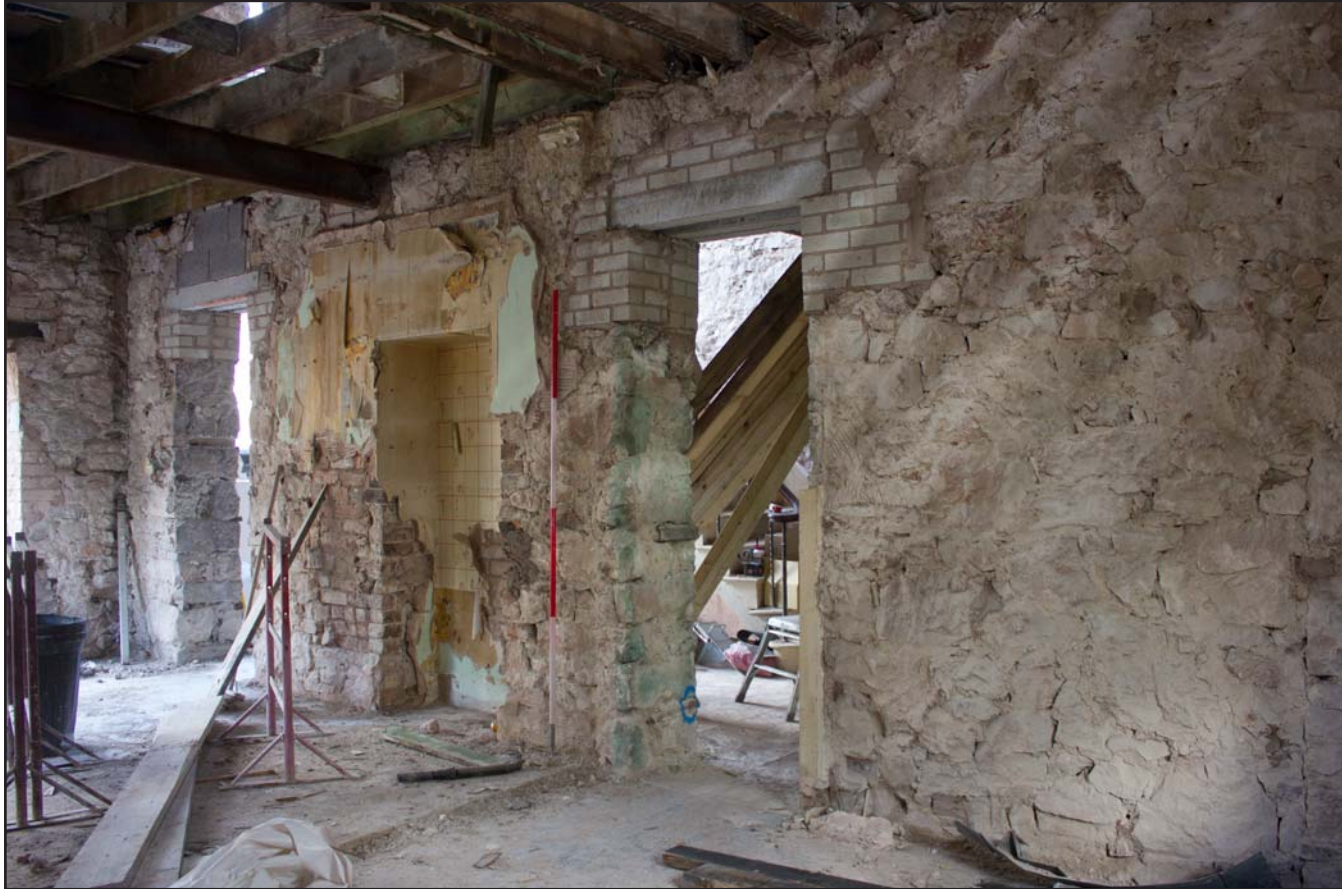
Plate 17: Kitchen/Dining Room, oblique shot, ground floor, Tanrallt Hall, Abergele Road, Llanddulas, Abergele - from the southeast - 2.00m scale
