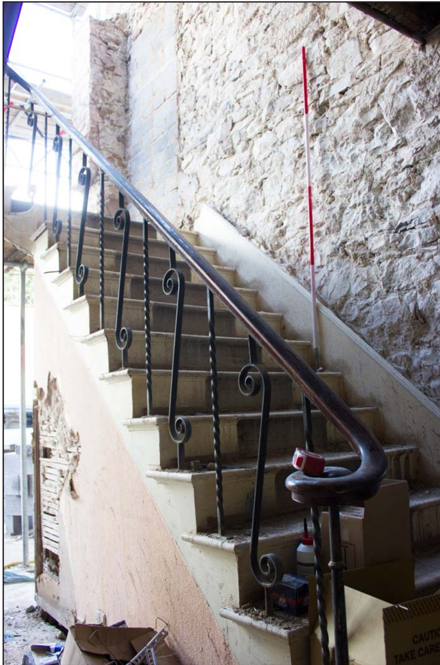
Plate 25: Hallway, Stairs, ground floor, Tanrallt Hall, Abergele Road, Llanddulas, Abergele - from the southeast - 2.00m scale
