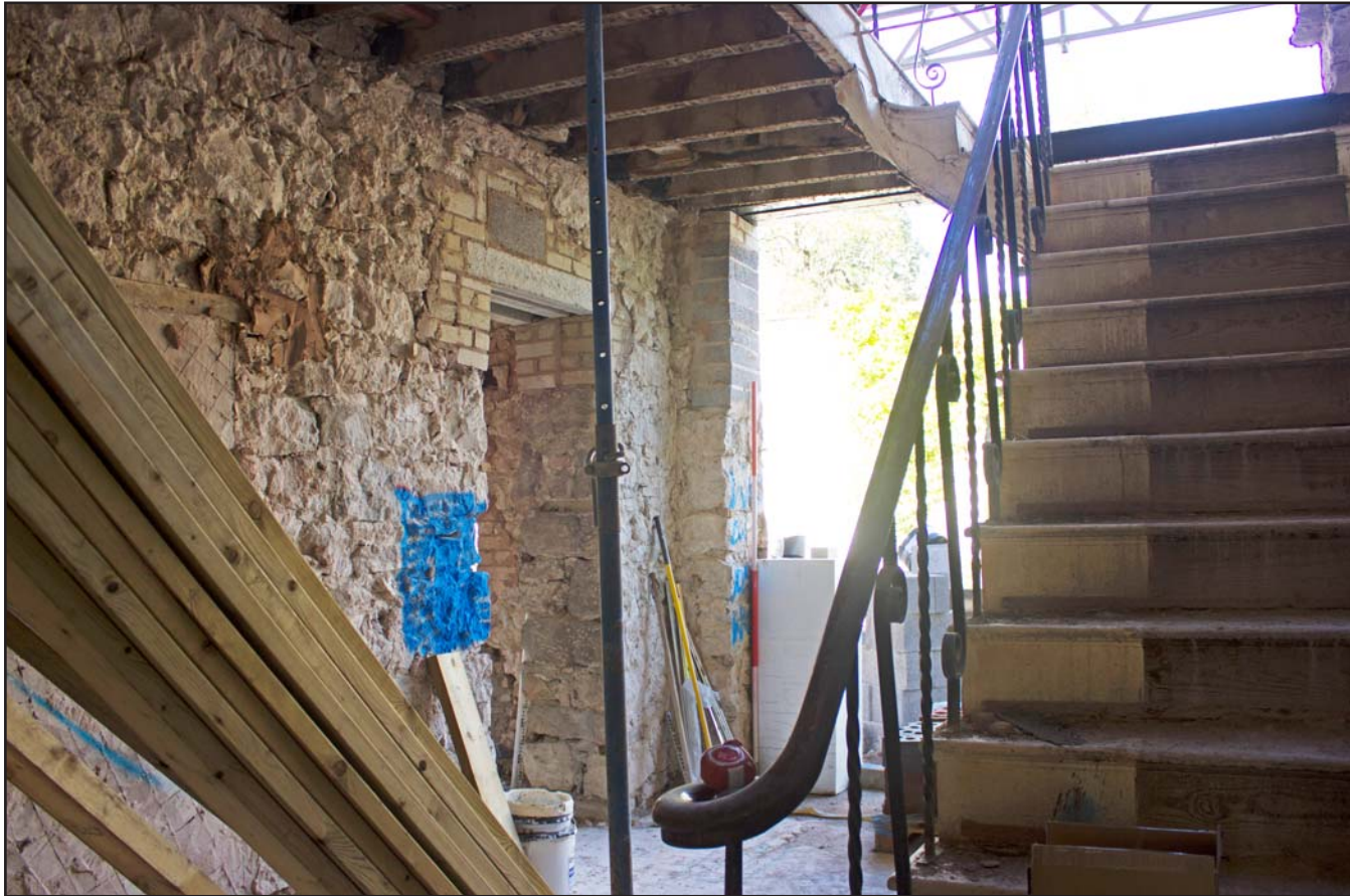
Plate 22: Hallway, ground floor, Tanrallt Hall, Abergele Road, Llanddulas, Abergele - from the northeast - 2.00m scale
