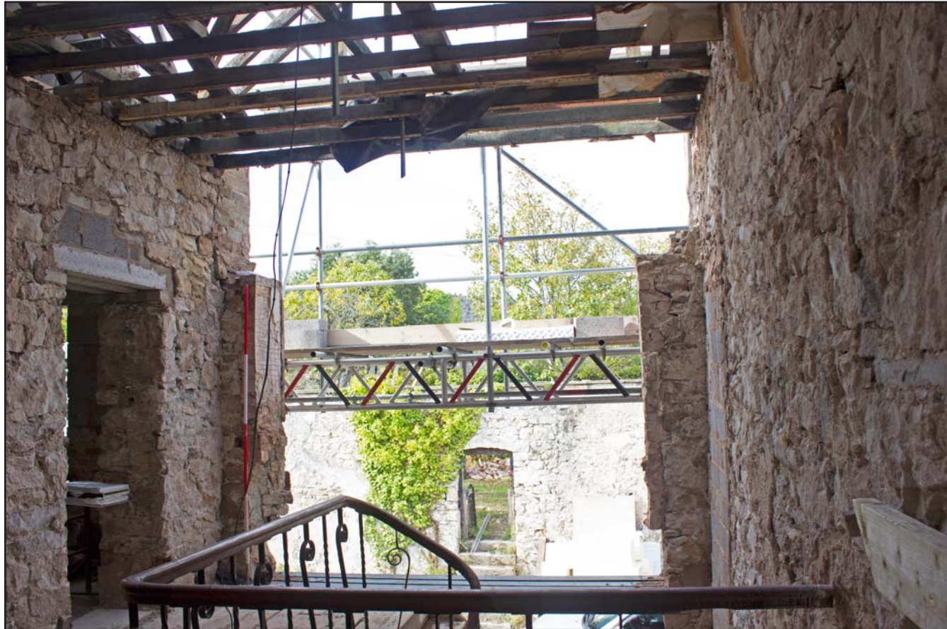
Plate 34: Landing, first floor, Tanrallt Hall, Abergele Road, Llanddulas, Abergele - from the northeast - 2.00m scale
