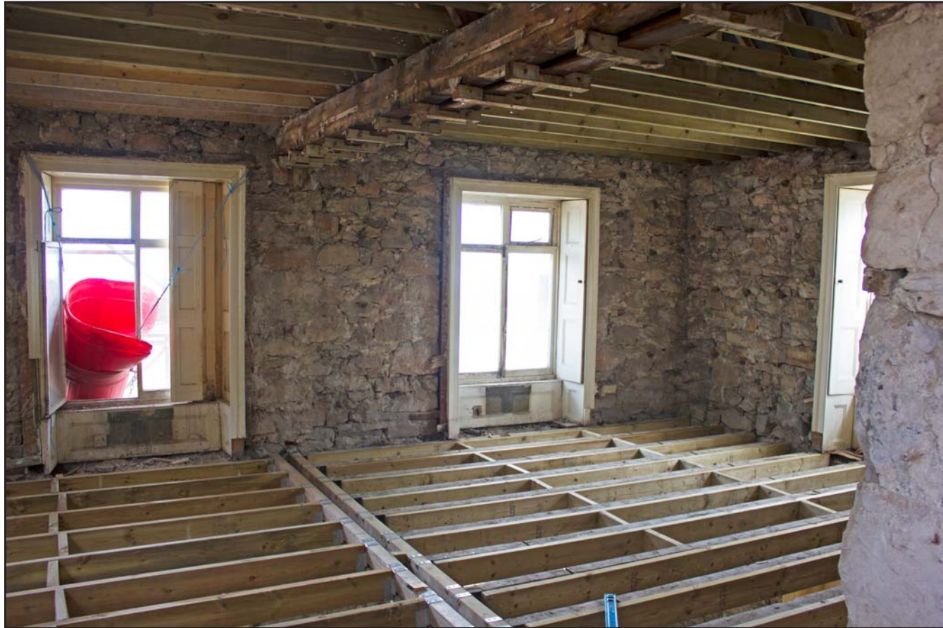
Plate 38: Bedroom 1/2, first floor, Tanrallt Hall, Abergele Road, Llanddulas, Abergele - from the southwest - no scale
