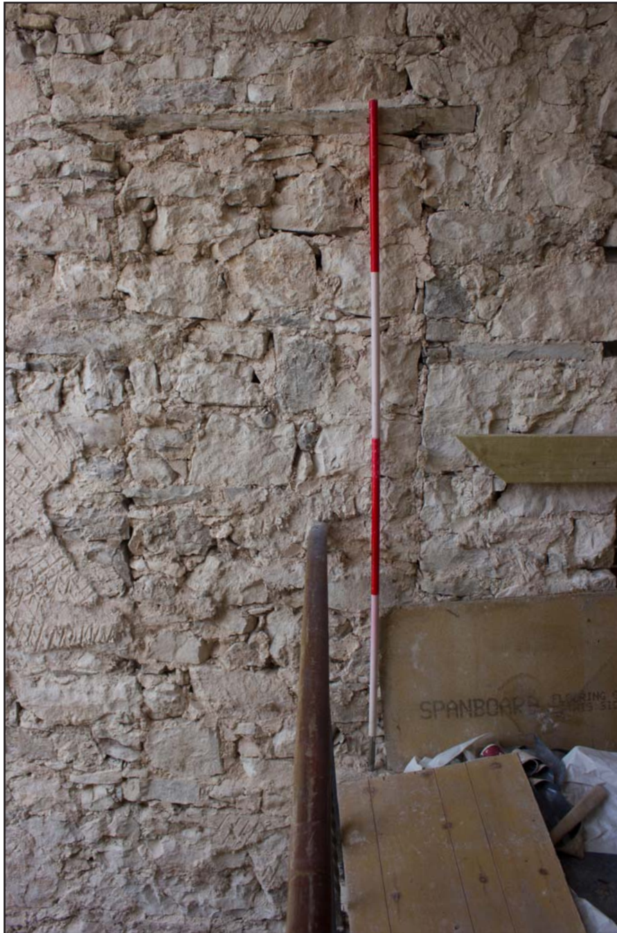
Plate 36: Landing, blocked door, first floor, Tanrallt Hall, Abergele Road, Llanddulas, Abergele - from the south - 2.00m scale
