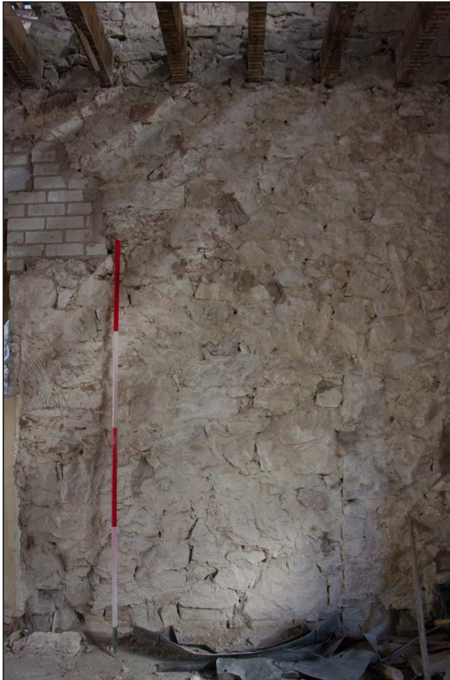
Plate 18: Kitchen/Dining Room, blocked door, ground floor, Tanrallt Hall, Abergele Road, Llanddulas, Abergele - from the southeast - 2.00m scale
