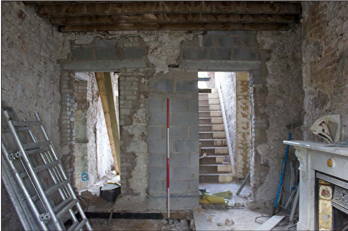
Plate 20: Living Room/Study, ground floor, Tanrallt Hall, Abergele Road, Llanddulas, Abergele - from the east - 2.00m scale
