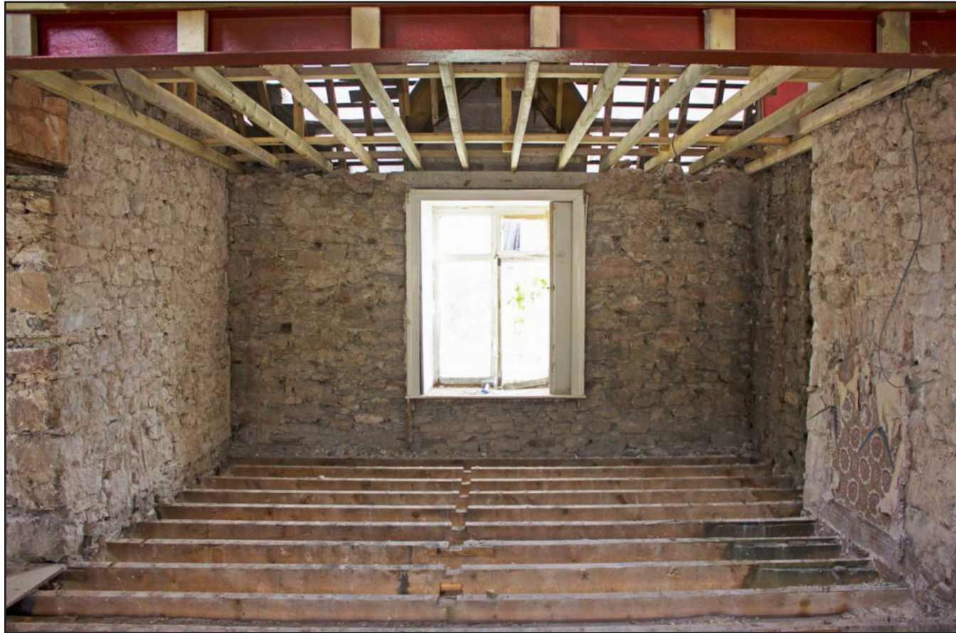
Plate 40: Bedroom 4, first floor, Tanrallt Hall, Abergele Road, Llanddulas, Abergele - from the west - no scale
