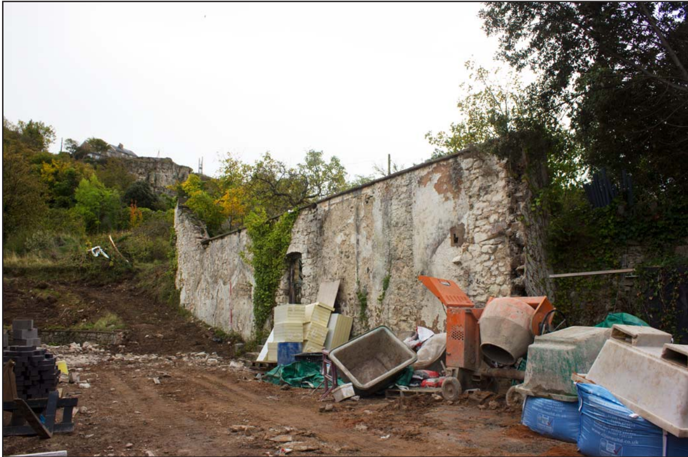
Plate 11: Stable yard wall of Tanrallt Hall, Abergele Road, Llanddulas, Abergele - from the northeast - 2.00m scale
