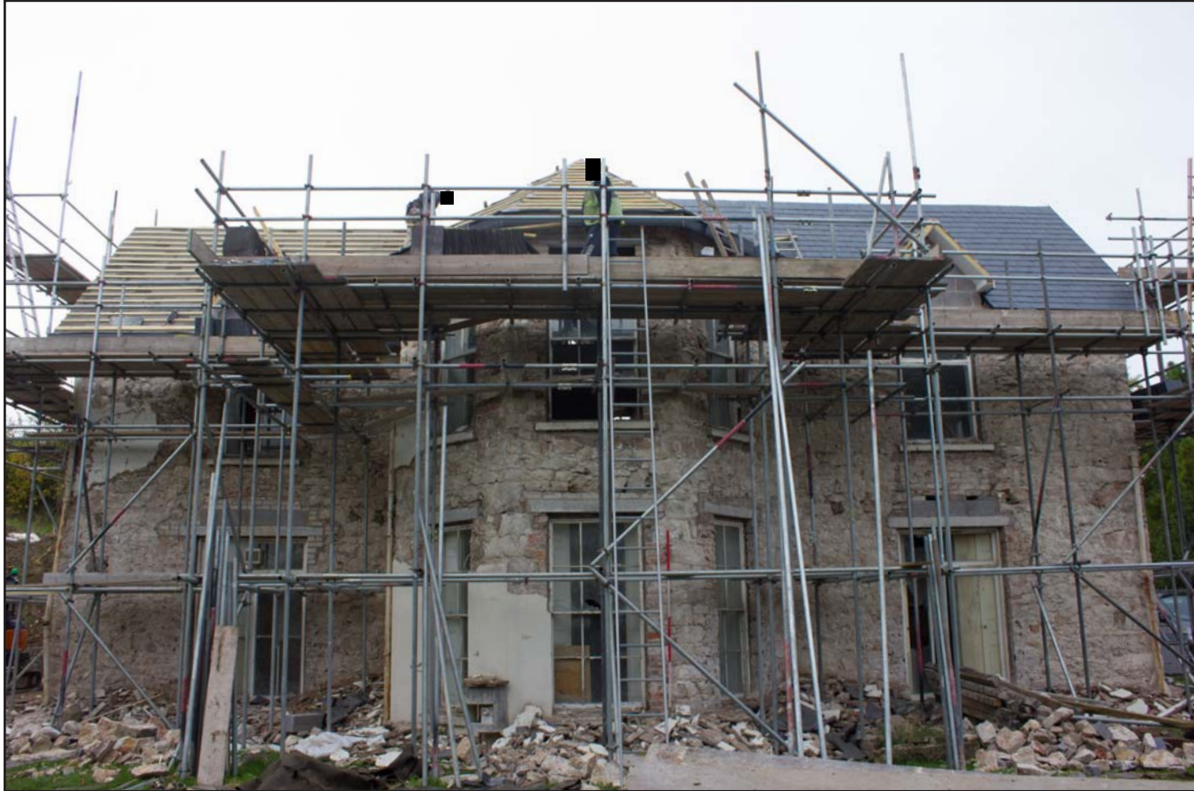
Plate 08: Eastern elevation of Tanrallt Hall, Abergele Road, Llanddulas, Abergele - from the east - 2.00m scale
